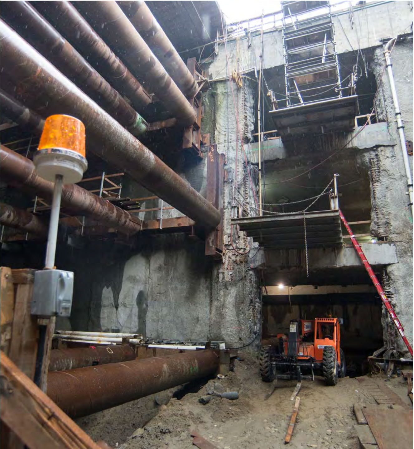
Looking west from the base of the elevator platform at the entrance portals to the station box levels, rain drizzles into the headhouse.
