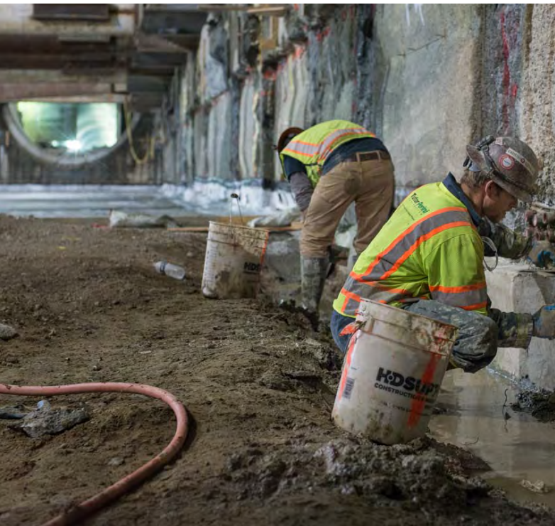
2 A smooth "rat slab" is poured into place, and waterproofing is installed
