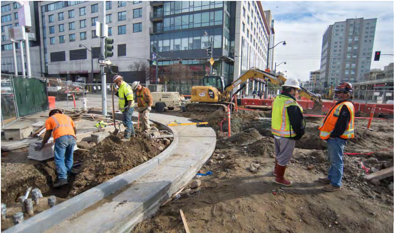
A new curb and gutter have been poured as part of street restoration efforts at the north corner of 4th and Townsend.
