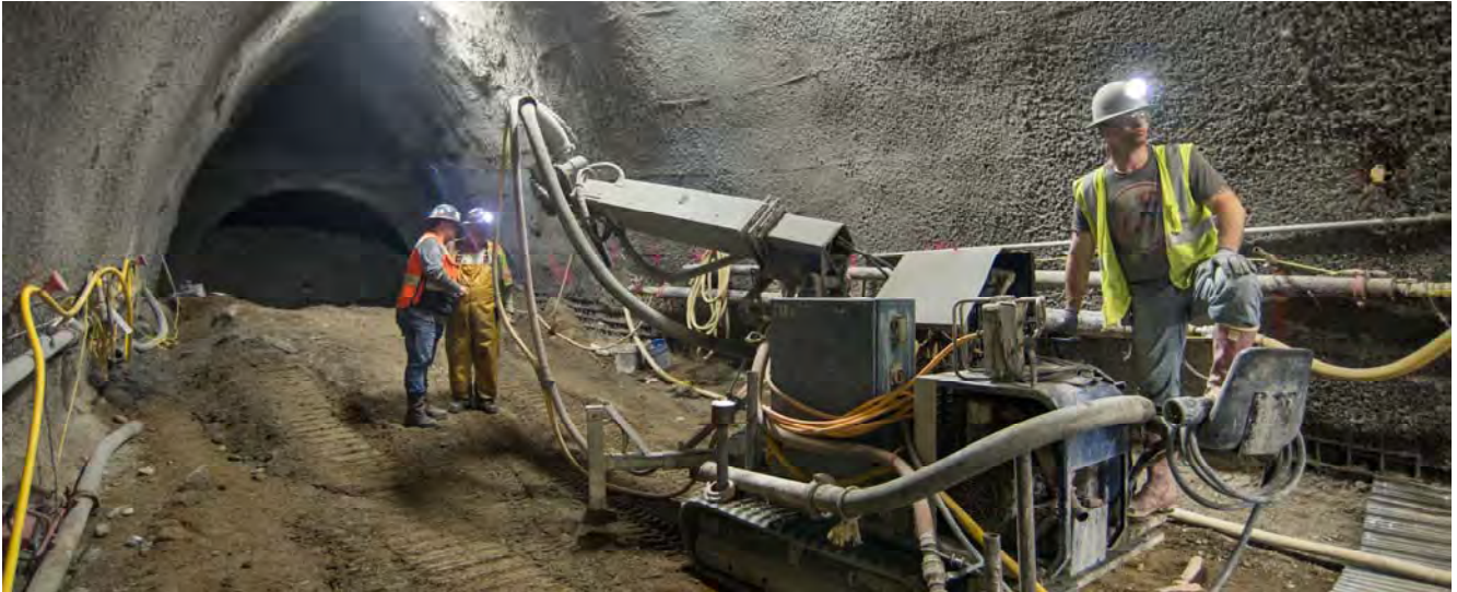
Workers move a shotcrete spraying machine out of the right side drift to the north platform cavern for maintenance.
