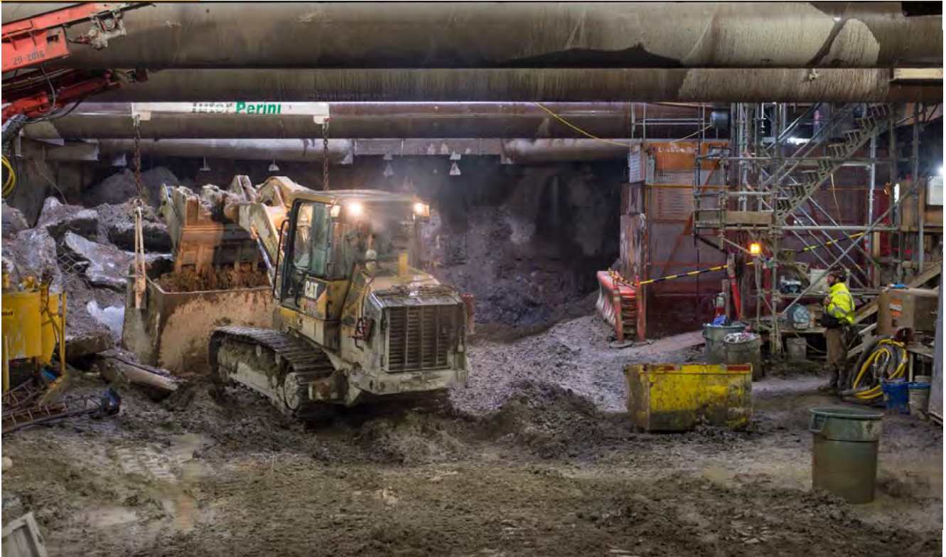
The overseer for the main access shaft in the headhouse, Armando, looks on as a bulldozer dumps a load of excavated material into the large steel bucket used to lift it to the
