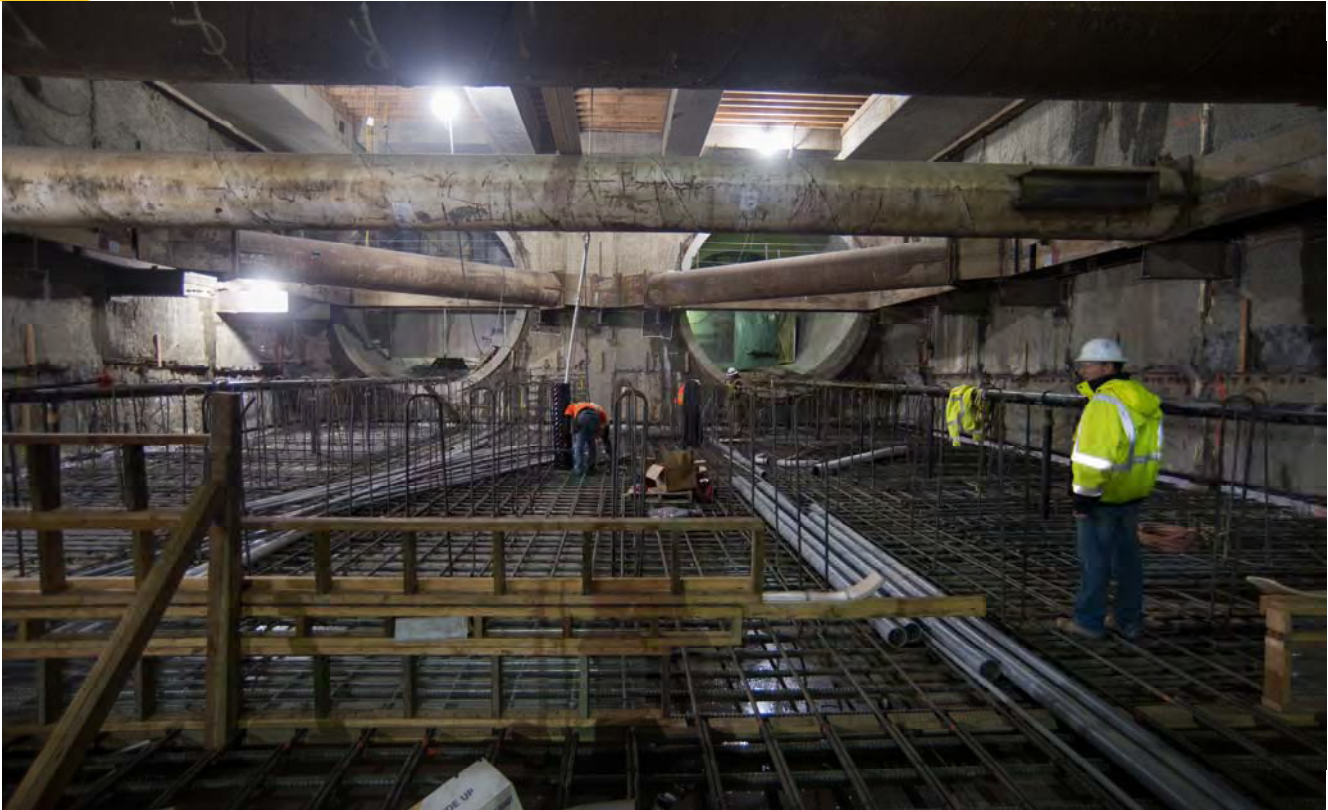
Workers have begun installing sections of a massive rebar cage at the bottom of the station box, called the invert or floor slab.
