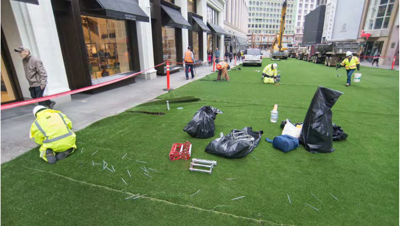
Workers pull up long tacks used to hold the green turf of the Winter Walk firmly in place.
