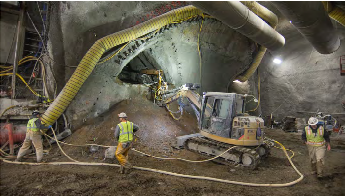
Crews have begun work to excavate the left side drift on the north end of the station platform cavern.
