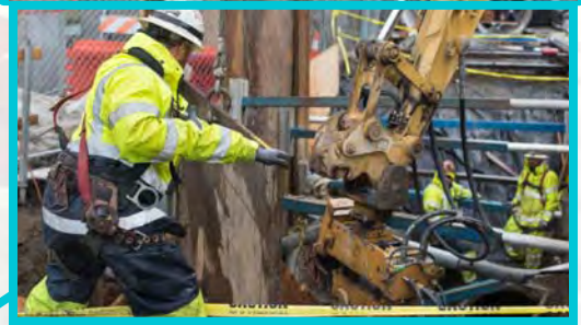
4th St. Surface Track, Systems (STS)
