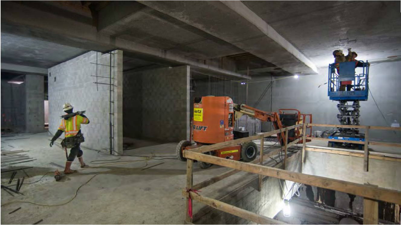
Interior walls and other structural elements are being installed on the upper two levels of the station box.
