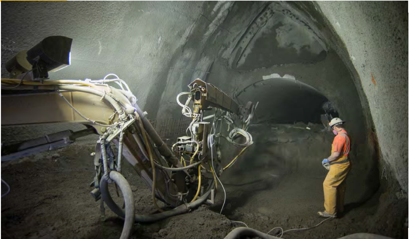
A worker uses a remote control to direct a shotcrete spraying machine at the end of the left side drift for the south platform cavern.
