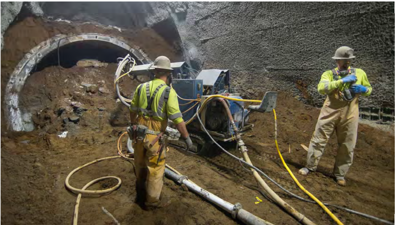
Two workers tend to a shotcrete spraying machine inside the right side drift of the north platform cavern excavation.
