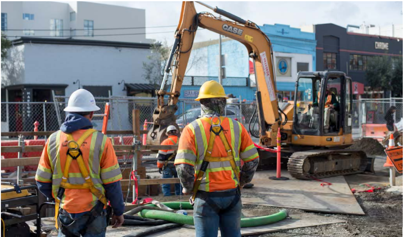
Workers pause to examine site conditions at the Brannan and Stockton intersection, where a number of utilities are being installed and upgraded.
