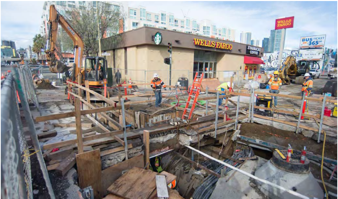
A crew at the intersection of 4th and Brannan works to rebuild a dense nest of utilities following the recent construction of a new manhole and sewer tie-in structure.
