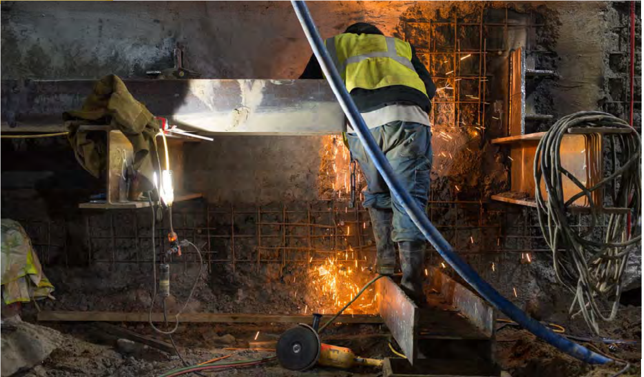
Sparks fall in a shower from a steel beam being installed as temporary bracing along the east wall of the station box.
