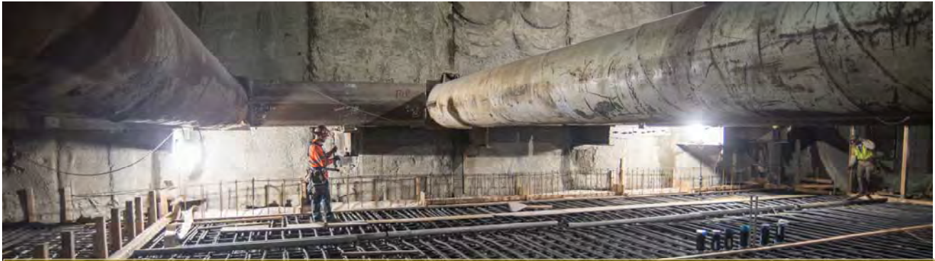
A worker installs rebar and vinyl waterproofing gaskets at the edge of a large rebar cage taking shape as part of the construction of the station box invert.
