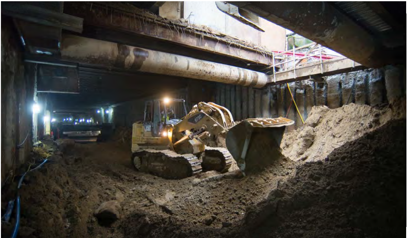
A bulldozer dumps another load of material removed during station box excavation, at the collection site below the Ellis Street access shaft.
