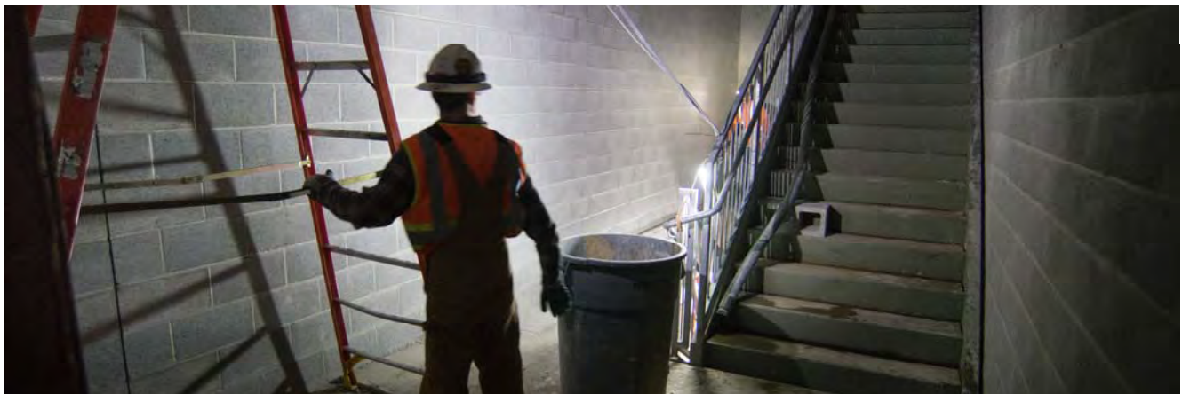
On the upper two levels of the station box, workers have been constructing interior stairwells at the north and south ends.
