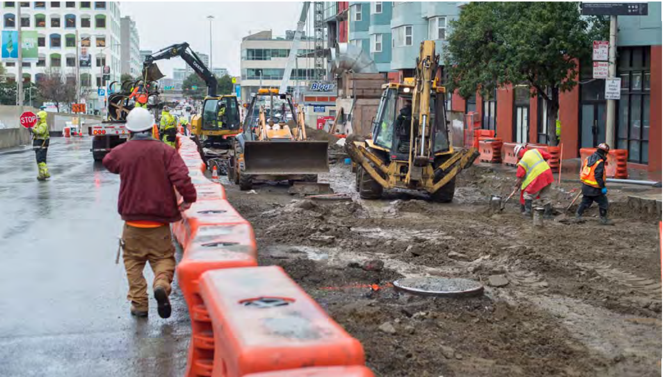
A crew coordinates the movement of traffic and equipment for utility installation and street restoration work south of Howard, on the west side of 4th.
