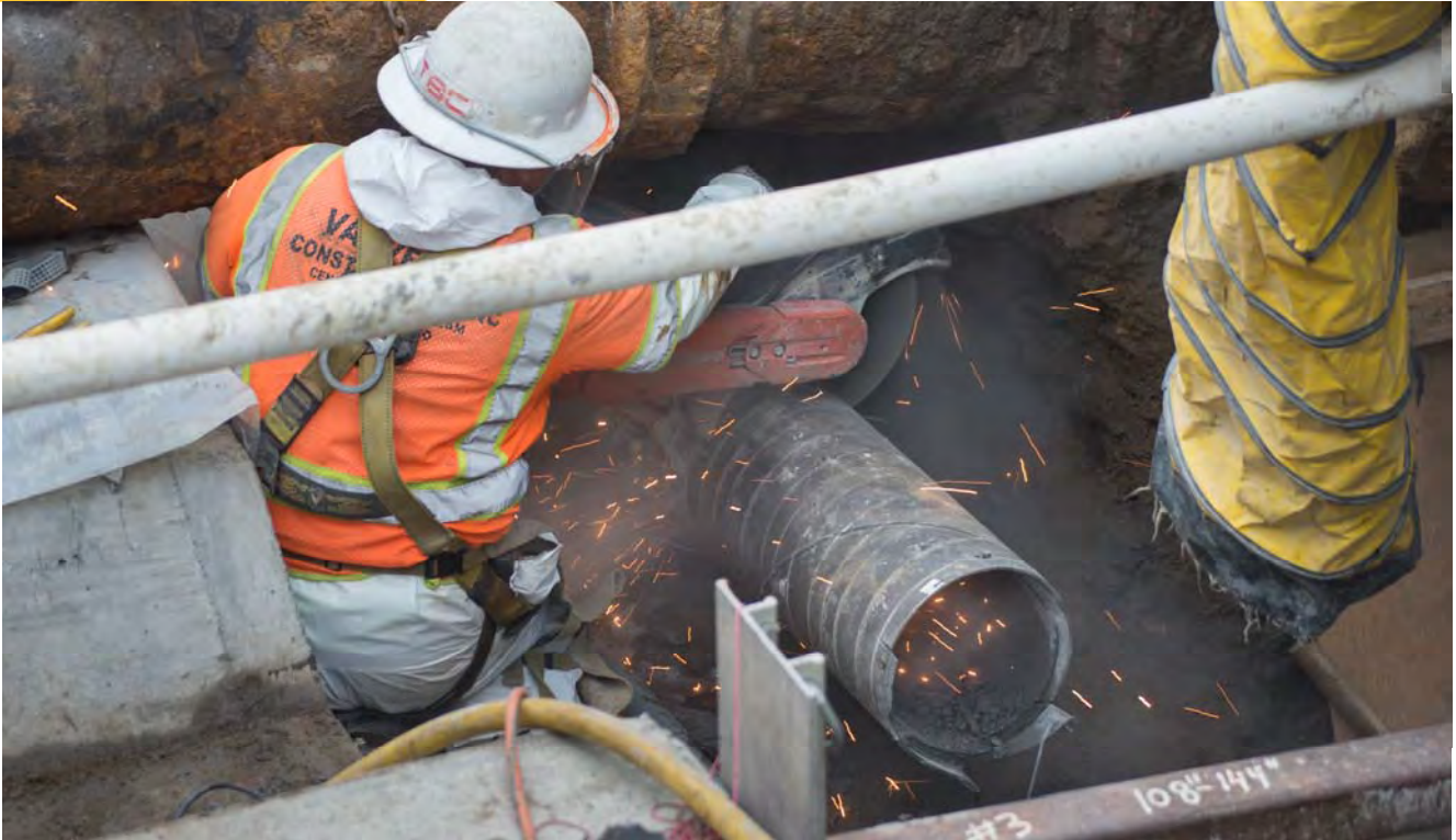
A section of water pipe is cut in a utility trench at 4th and Brannan prior to attaching a new section, located nearby.
