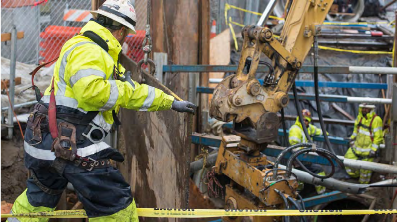
A worker swings a large steel panel into place, where it will be used as temporary shoring for a utility trench at Welsh Alley and 4th.
