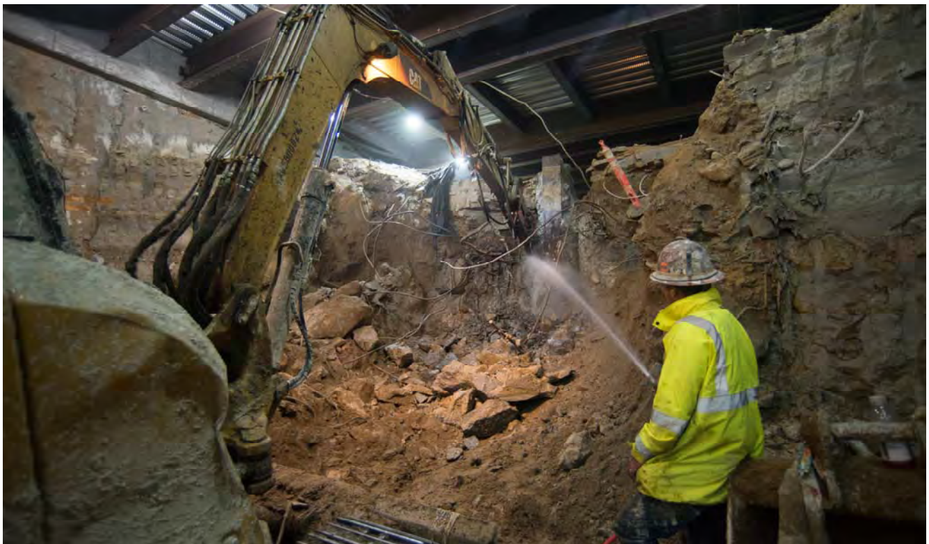
A worker helps keep dust down by spraying water on a jackhammer working on the concrete of the south station headwall.
