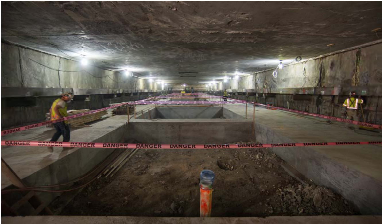
Workers have removed most of the temporary steel bracing inside the mezzanine level of the station box, revealing the future openings between the mezzanine and platform level below, yet to be excavated.
