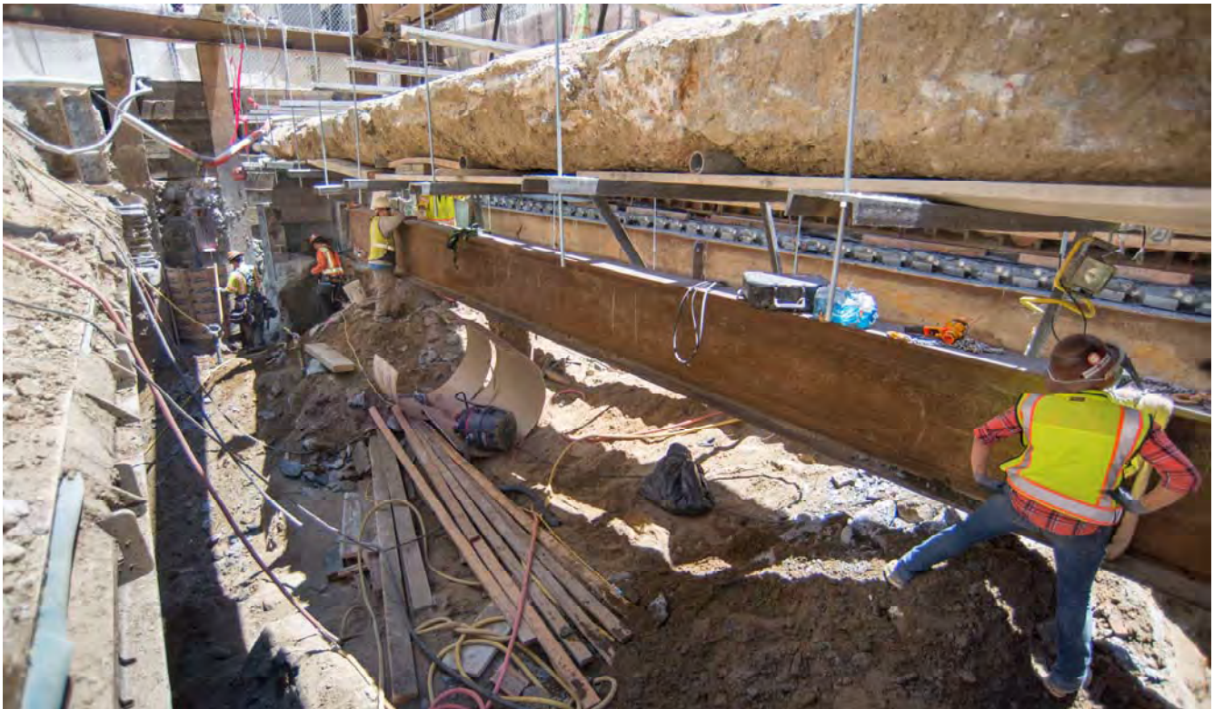
Steel beams are carefully being installed under an active utility duct bank on the north side of O'Farrell at Stockton. These beams will support this section of the station roof deck.
