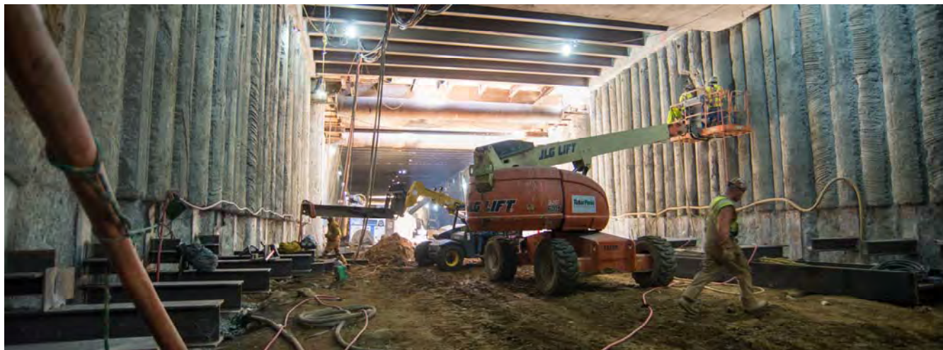
Two men use jackhammers to smooth portions of secant piles comprising the outer walls of the north concourse while short sections of I-beams are welded to the walls for holding future reinforcing.
