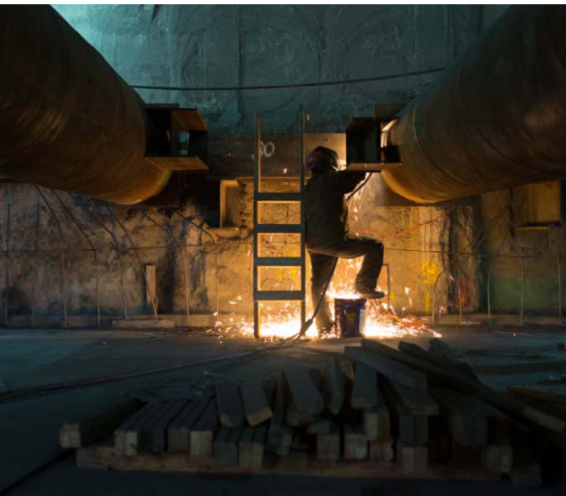
2 Temporary struts and walers used to reinforce the slurry walls are removed
