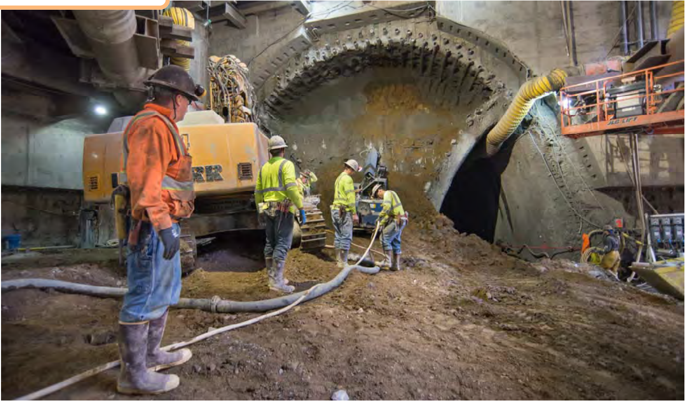
An operator fitted with a respirator and other safety gear uses a shotcrete spraying machine to temporarily cover an exposed section of earth inside the top header of the center drift, where SEM excavation is underway.
