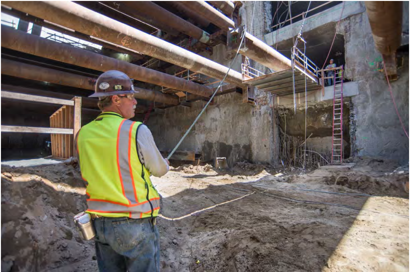
A site supervisor helps stabilize a large steel support during an operation to remove temporary supports from the mezzanine level of the station box.
