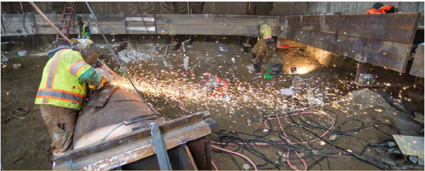
Sparks fly as a steelworker smooths edges of a steel bracket atop a strut, being prepared for installation at the north end of the station headhouse.
