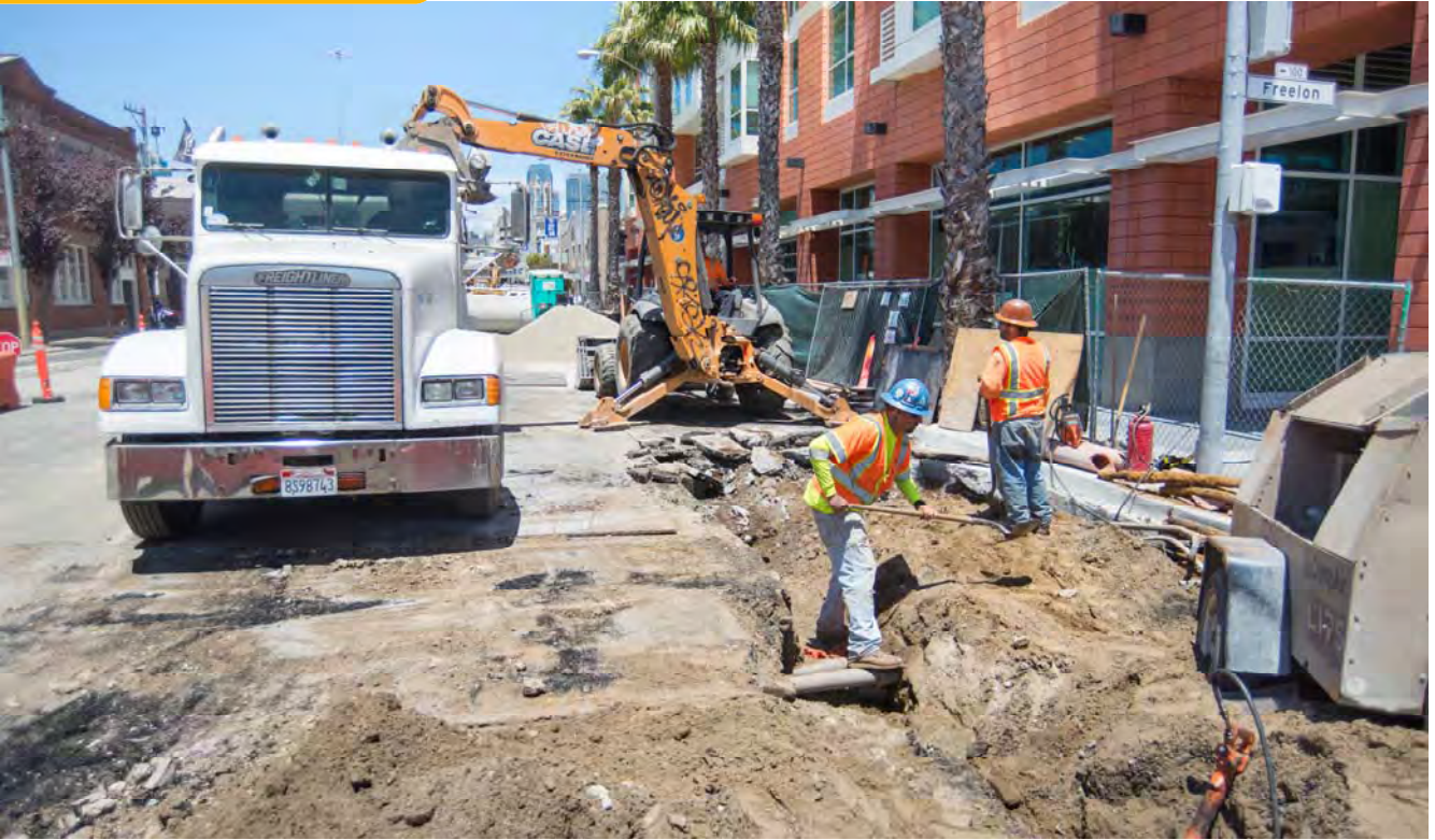
Workers use hand tools to uncover lateral utilities, so their locations can be marked ahead of future trench work.
