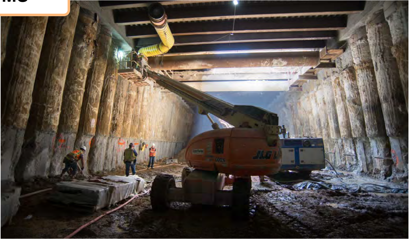
Workers prepare the tangent pile walls of the station box for drilling operations ahead of compensation grouting and the installation of temporary reinforcing.
