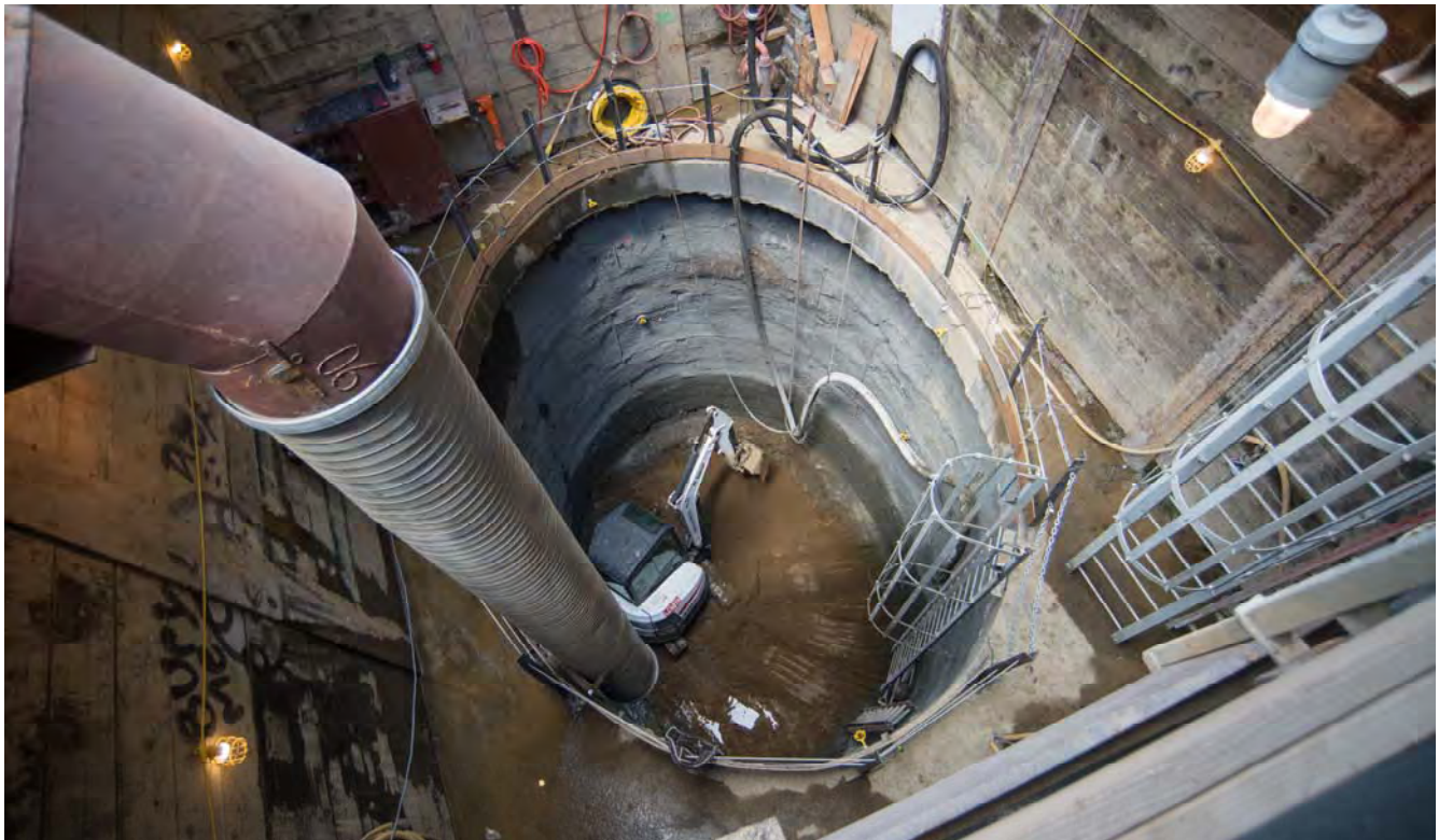
A small excavator collects excavated soil for removal at the bottom of the north access shaft. This shaft will eventually become an emergency exit stairwell for the station.
