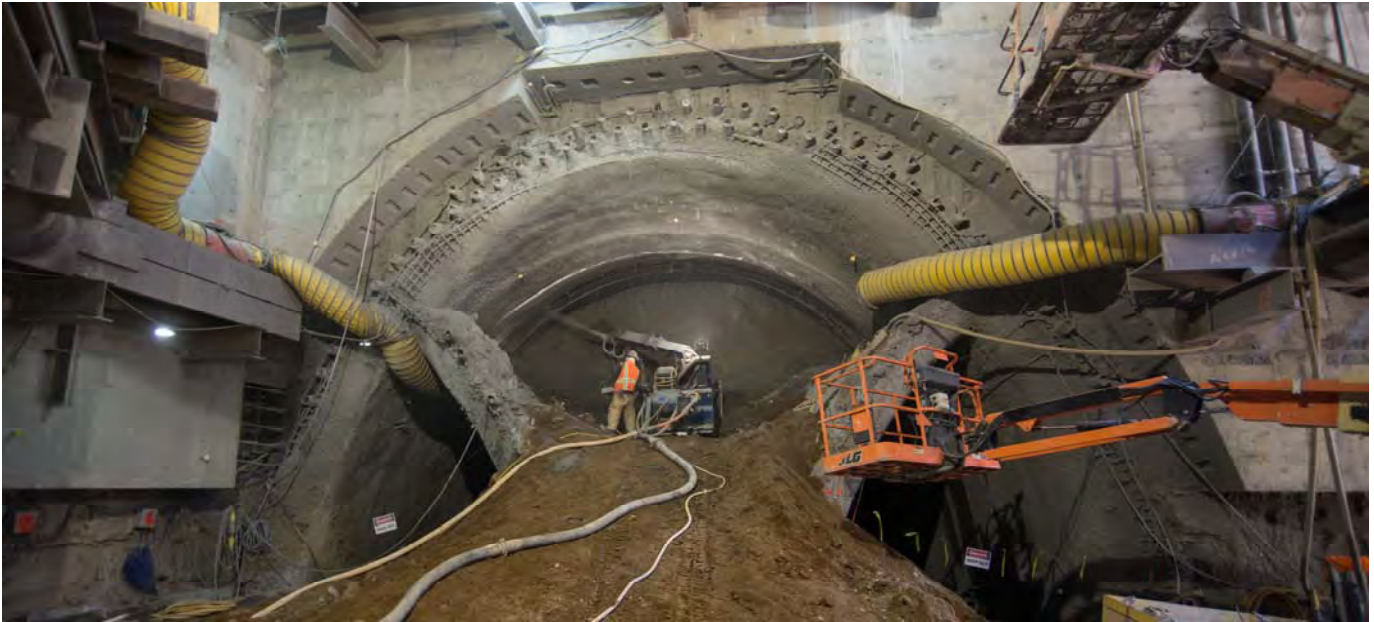
An operator fitted with a respirator and other safety gear uses a shotcrete spraying machine to temporarily cover an exposed section of earth inside the top header of the center drift, where excavation is underway.
