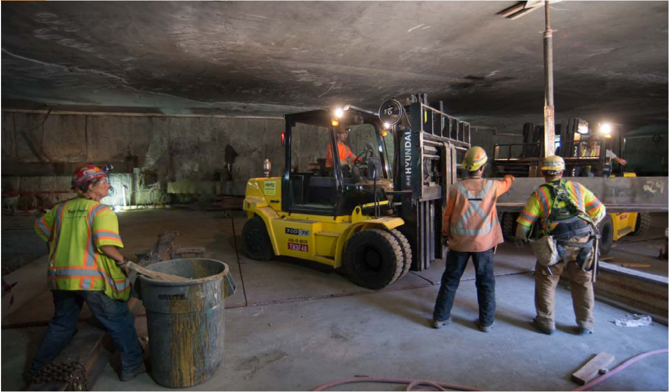
Two forklift operators slowly move a large steel beam used in temporary reinforcing into place near the access portal for the mezzanine level.
