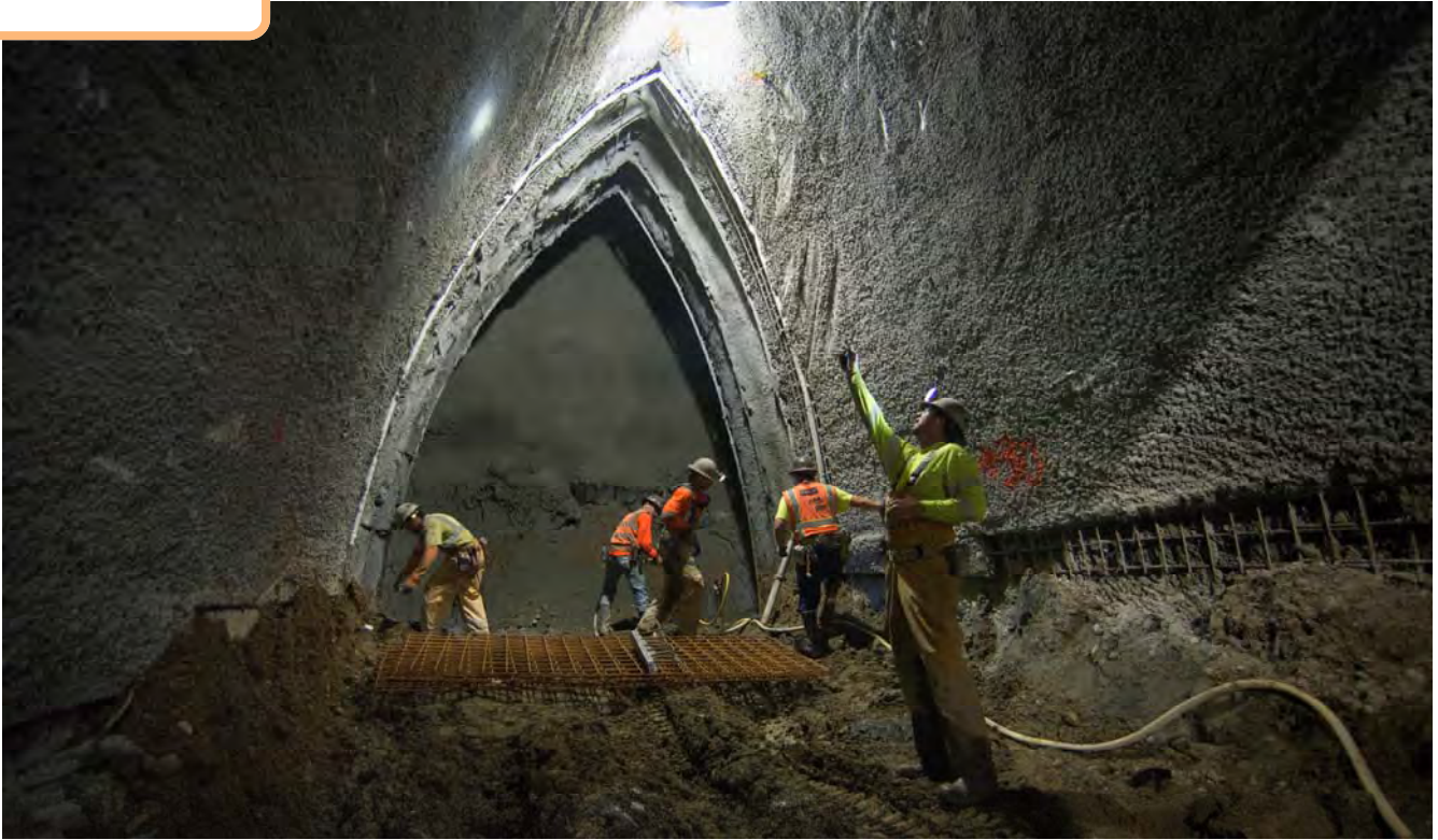
Air quality and movement is tested inside the right side drift, where workers prepare to install sections of steel mesh to reinforce the walls.
