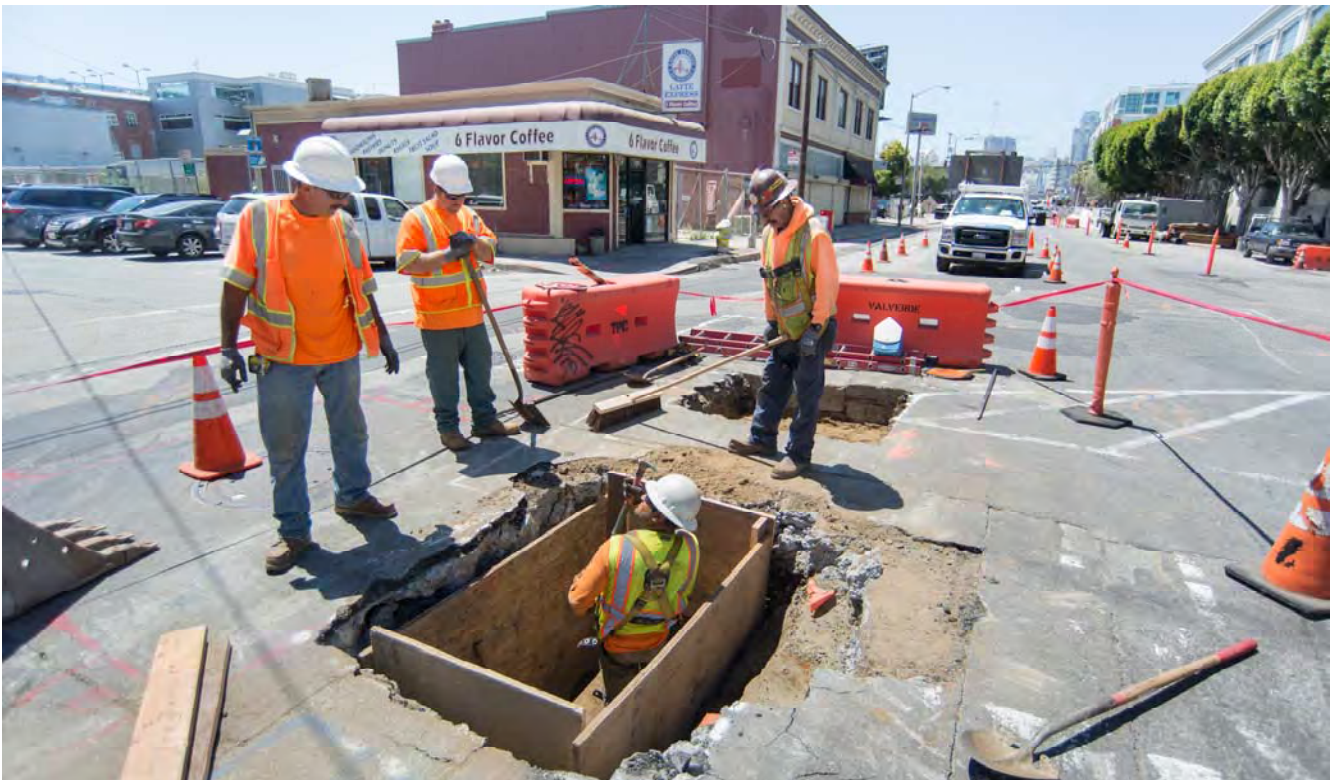
Workers are undergoing utility potholing in the middle of 4th at Bluxome.
