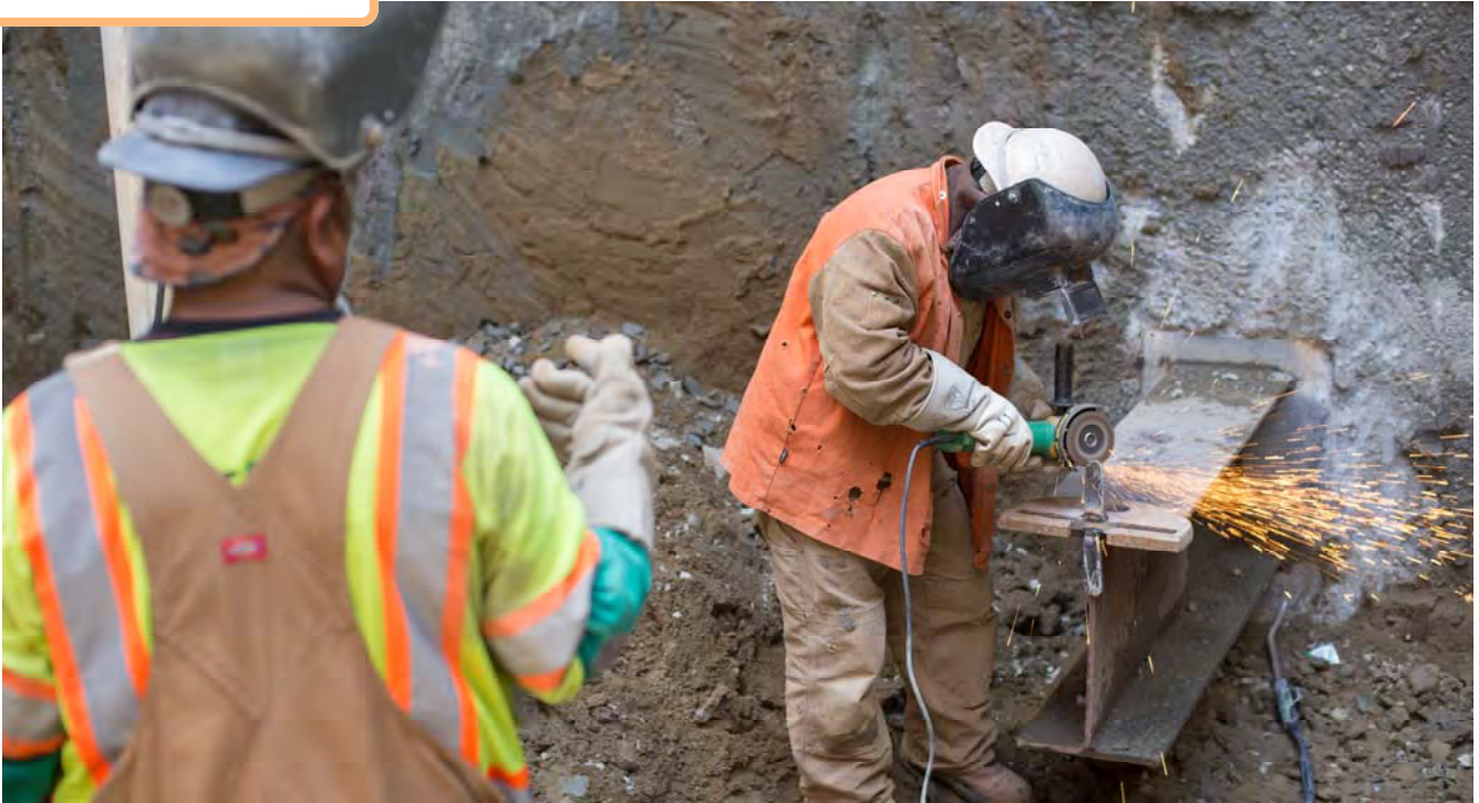
A worker uses an angle grinder to smooth the edges of two steel tabs used in temporary reinforcing being installed inside the headhouse.
