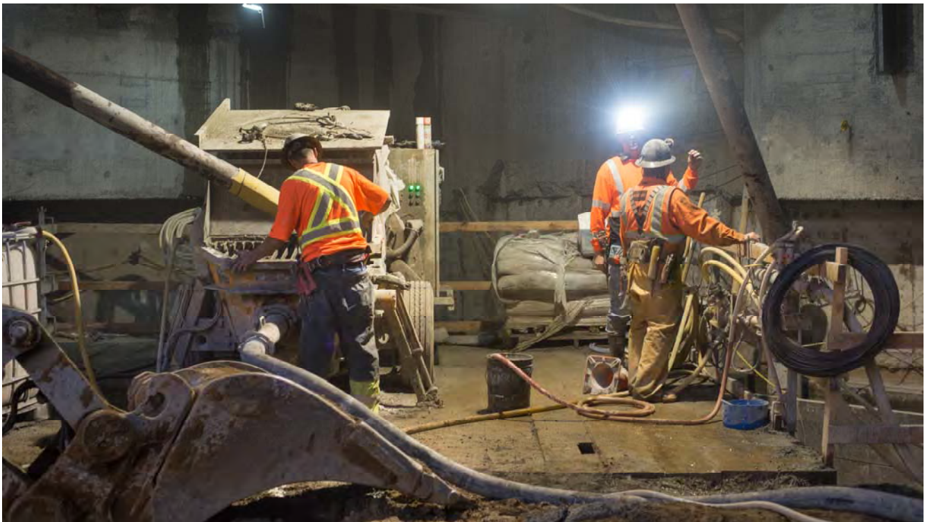
A crew at the bottom of the headhouse operates a concrete pump used to support shotcrete operations inside the station cavern entrance archway.
