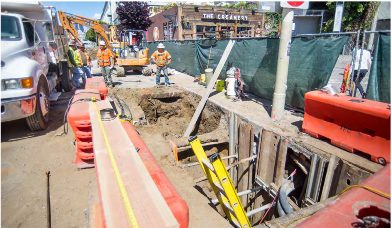
Existing utilities are exposed during the installation of a force main sewer pipe just north of Townsend on 4th.
