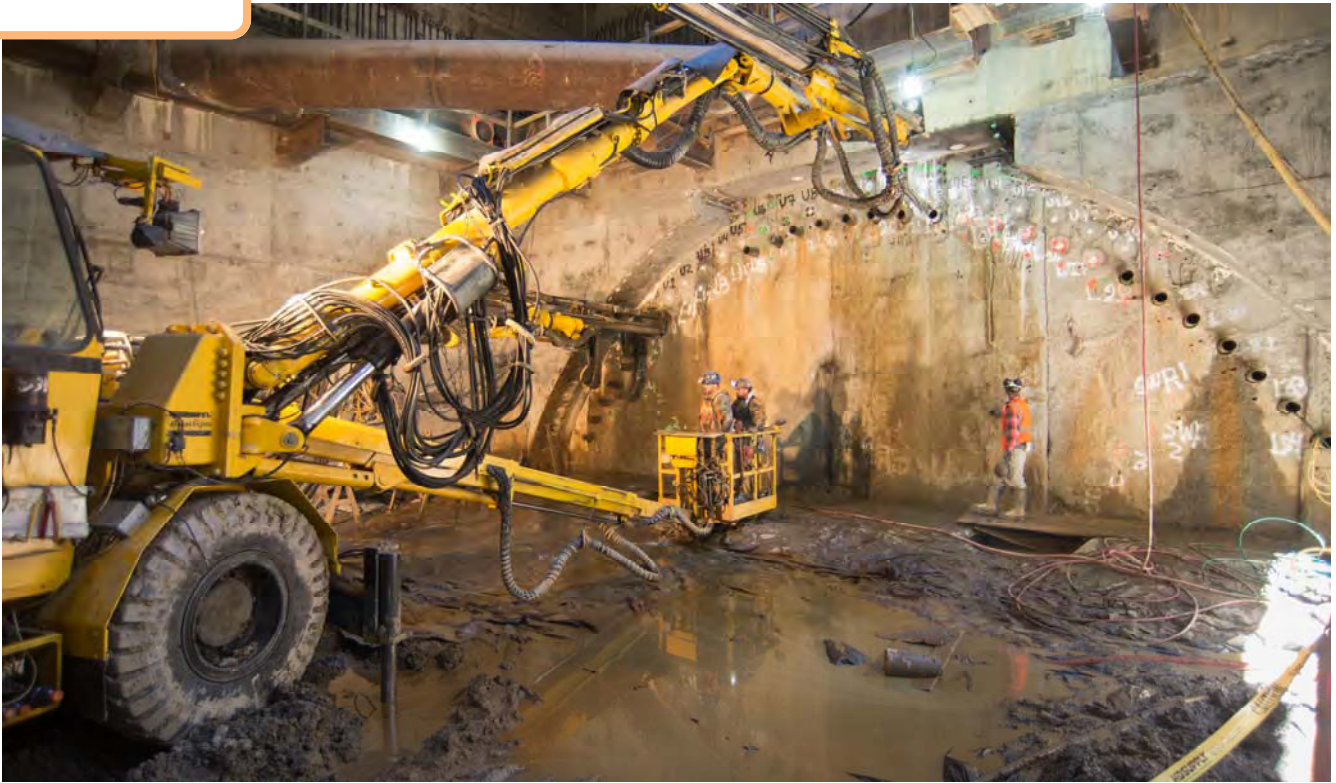
A large drilling machine is being used to conduct soil improvement work at the entrance archway for the future station cavern.
