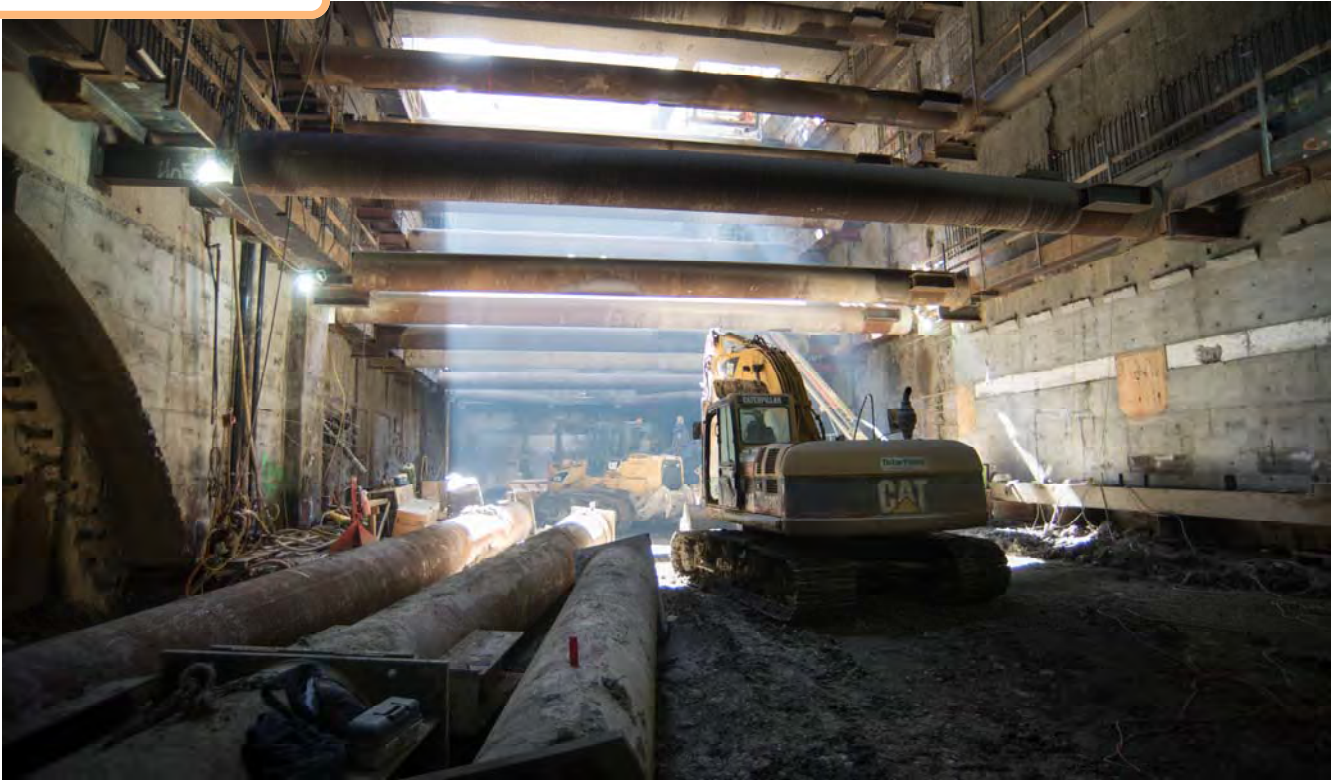
Light streams in the main access shaft for the Chinatown Station headhouse. Temporary steel reinforcing lays waiting to be installed.
