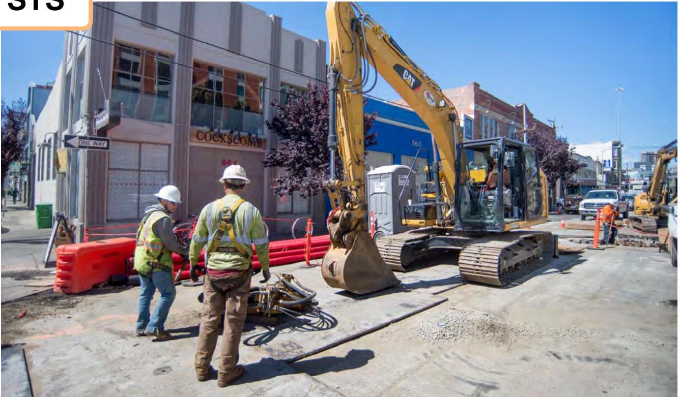
Equipment is checked and prepared prior to resuming work on a trench near Freelon and 4th.
