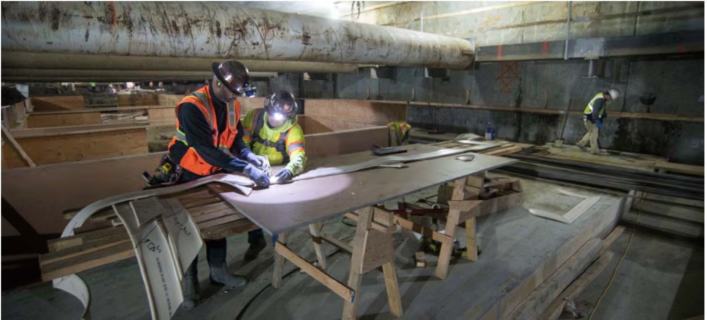
Workers assemble waterproofing gaskets used in concrete forms for the mezzanine level floor slab inside the Yerba Buena/Moscone Station.
