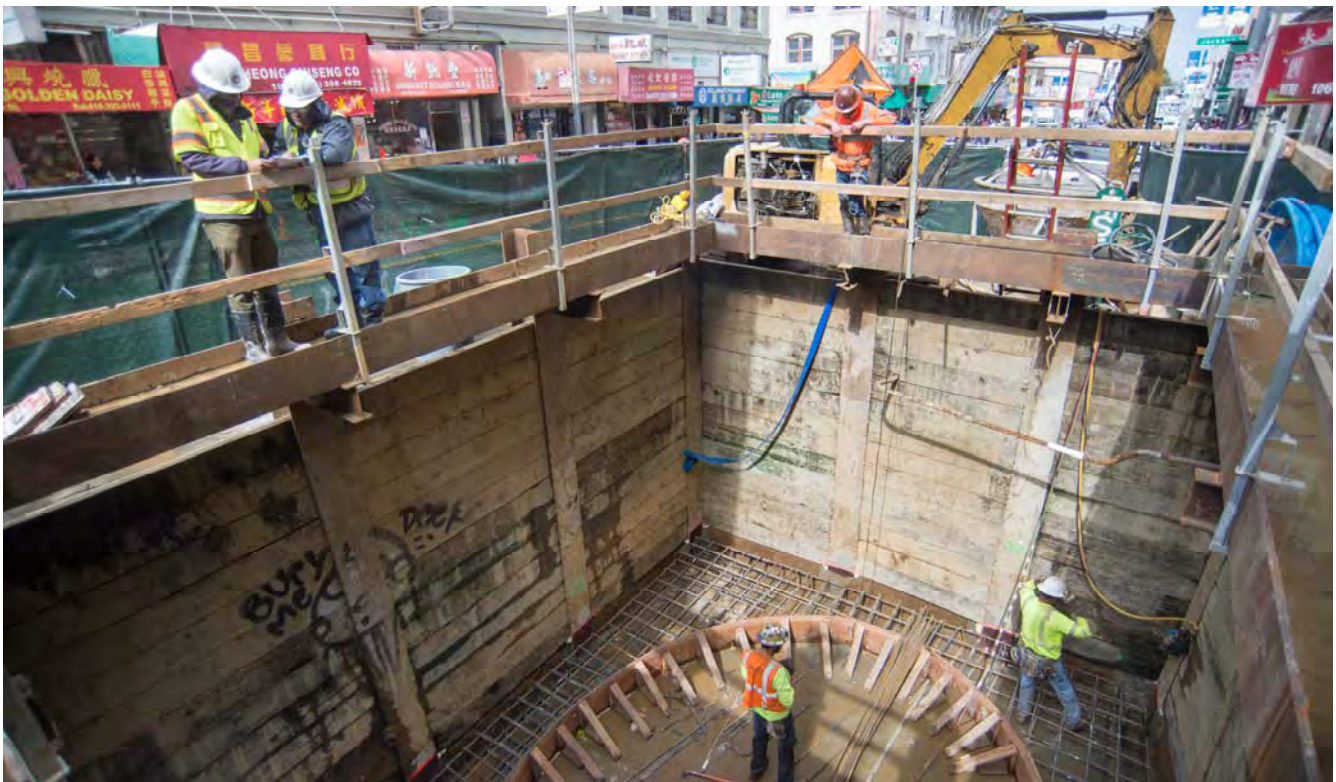
A crew is preparing to pour concrete for the construction of a structural slab inside the north access shaft for Chinatown Station.
