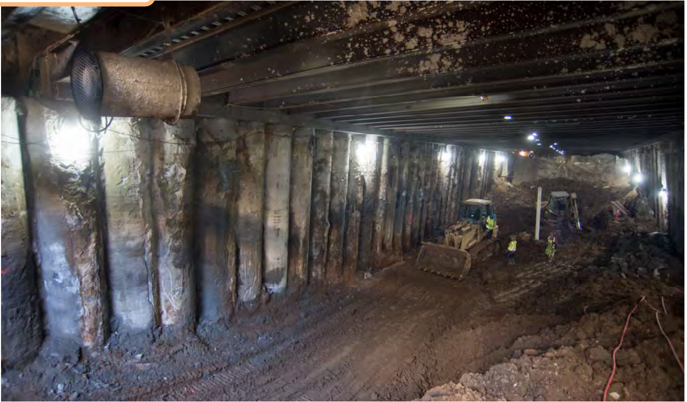
Work to excavate out the station box under Stockton between O'Farrell and Geary has begun.
