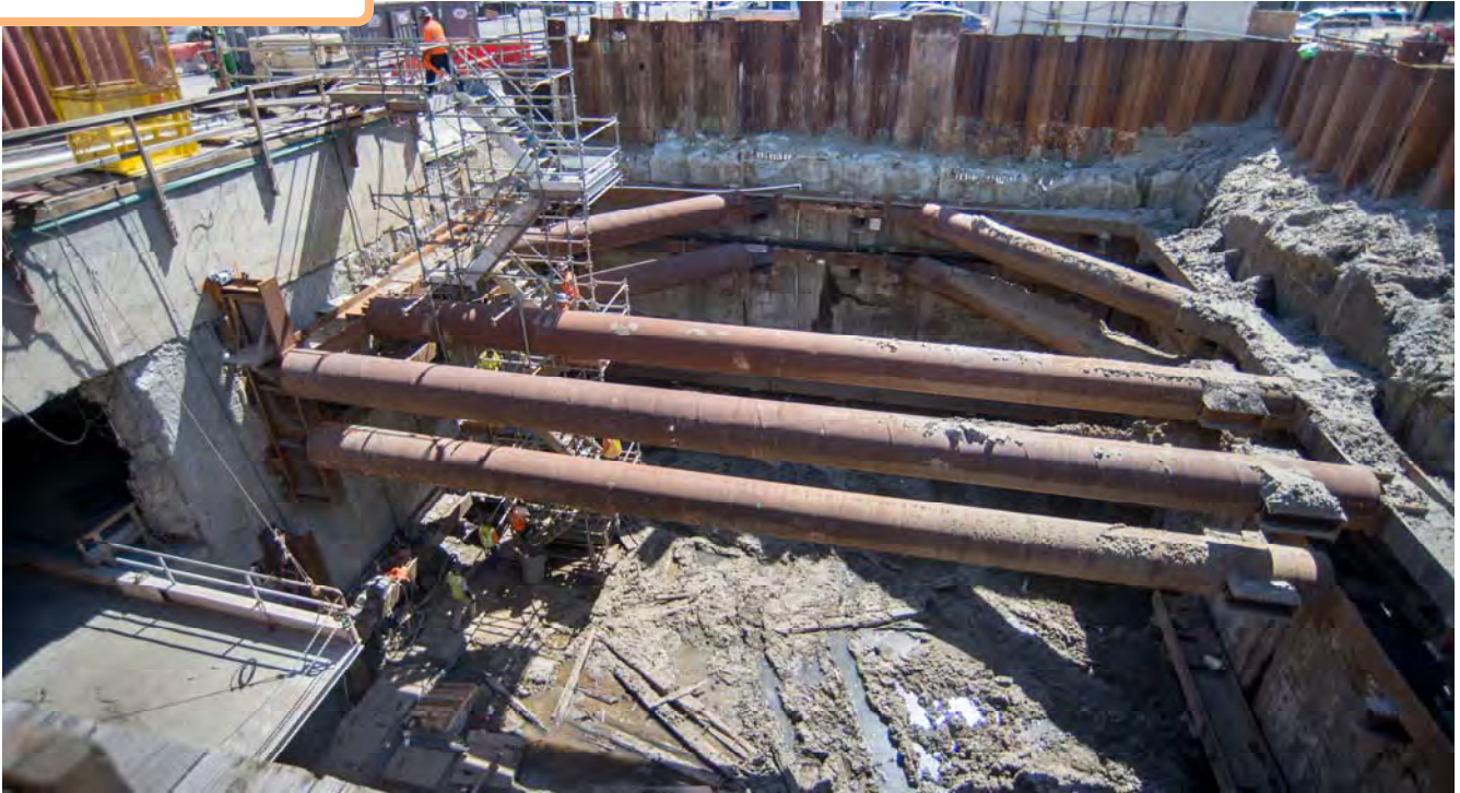
Temporary steel supports span across the headhouse site, while most of the work has recently been focused inside the station box.
