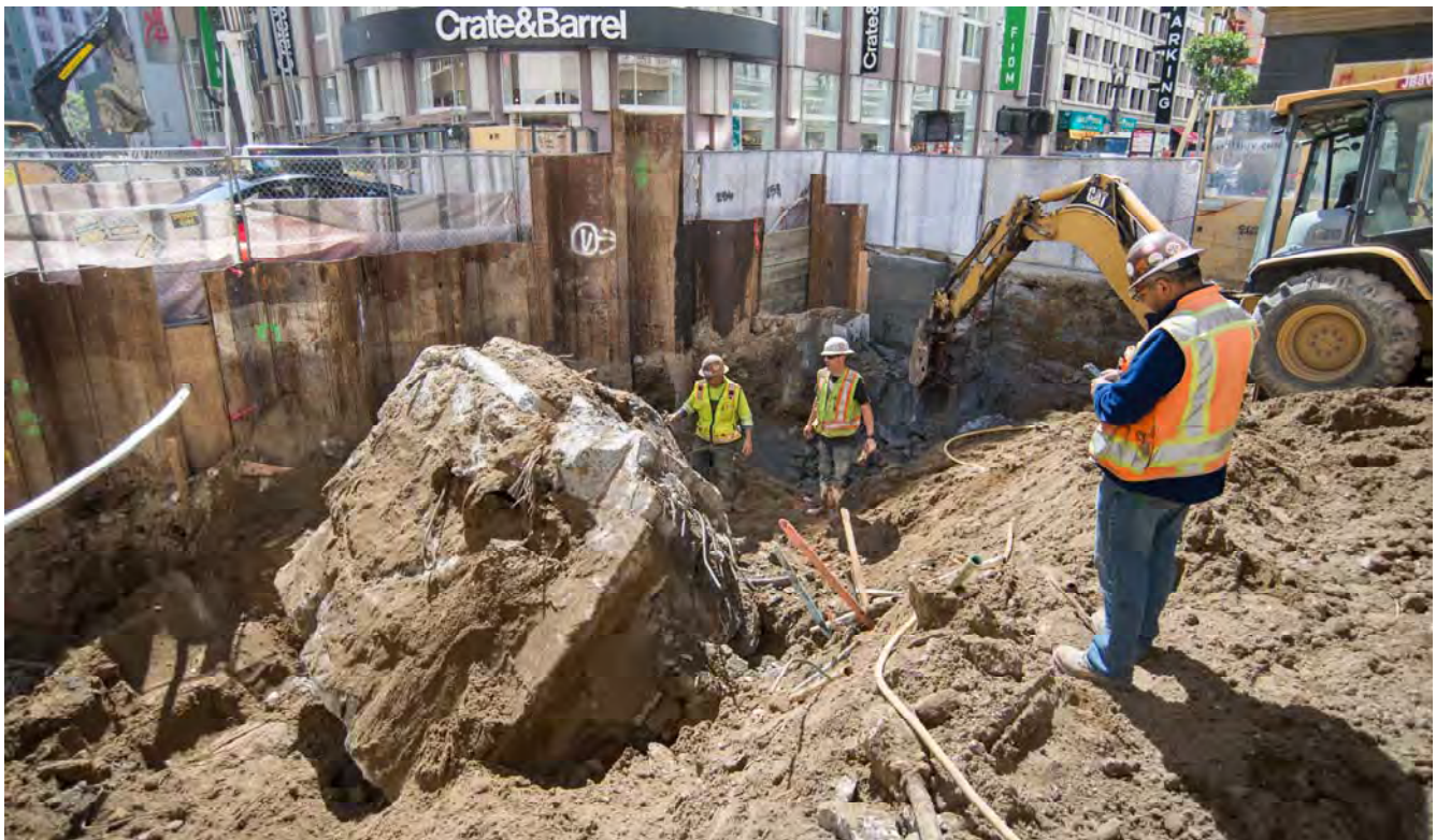
Men observe a large utility box unearthed north of O'Farrell, which will be demolished and removed to allow for site excavation and the installation of a new section of station roof deck.
