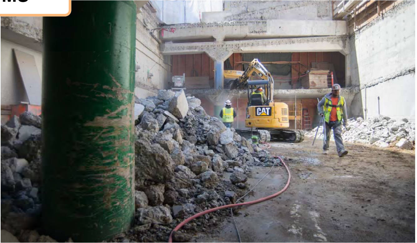
Workers are carefully removing floors and columns in a small area at the southeast corner of the Union Square Garage, where the future north station entrance will be located.
