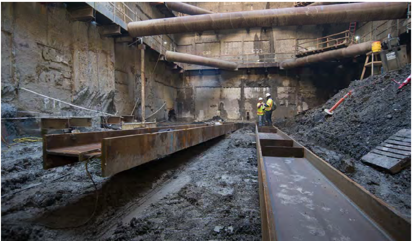
Two workers look over long steel I-beams, to be installed on brackets jutting from the slurry walls inside the station headhouse.
