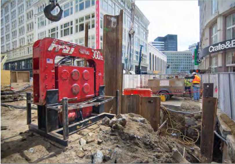
1 A large vibro-hammer is used to press sections of steel sheet piles into the ground
