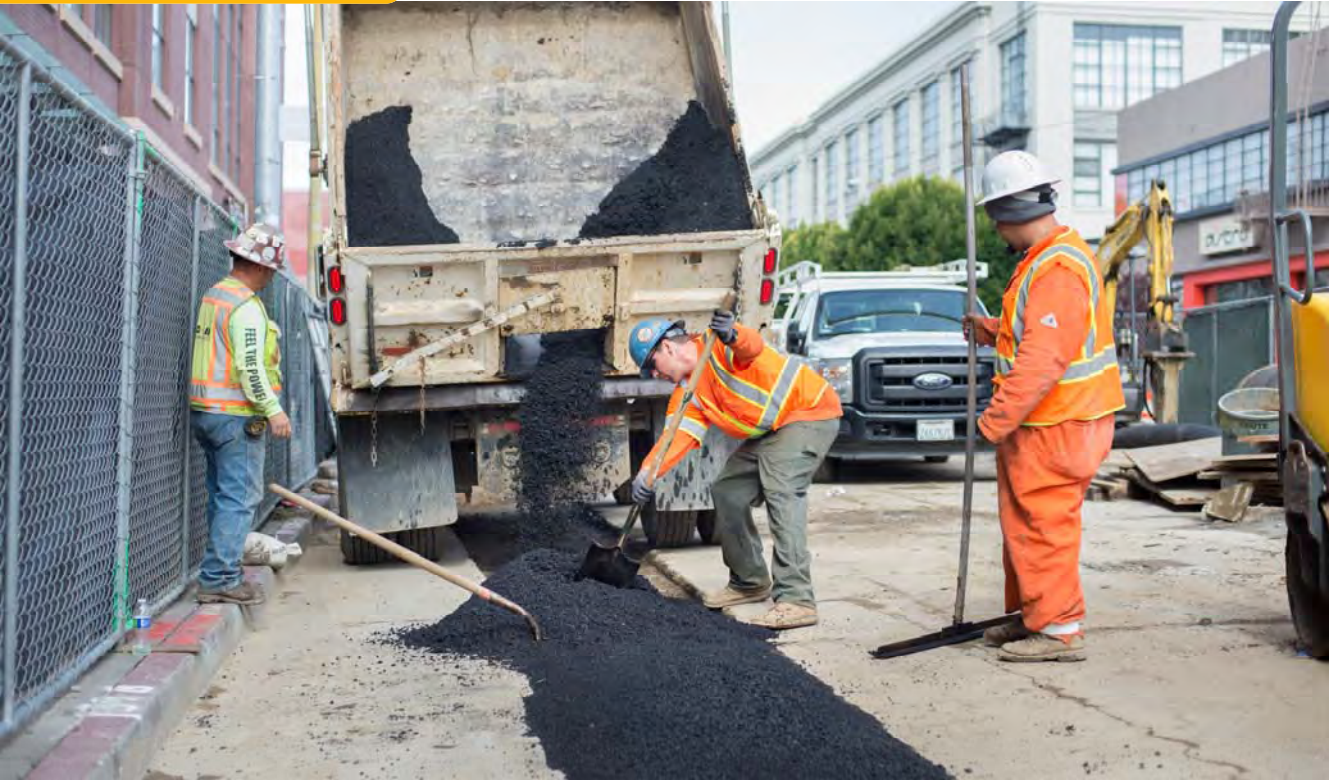
Just north of Townsend, a completed and backfilled section of utility trench gets covered in new asphalt.
