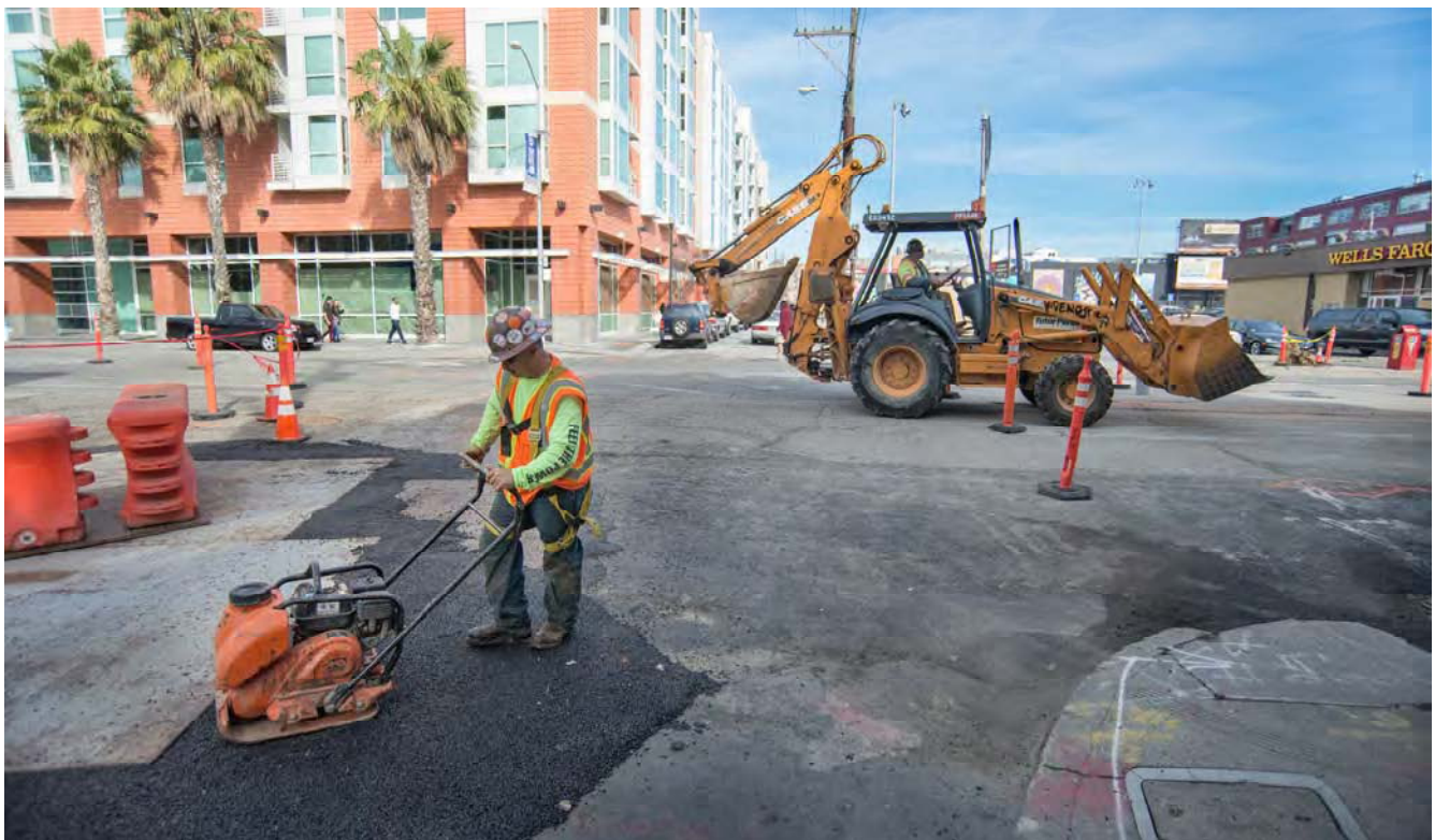
A worker compacts asphalt around a steel panel, while a backhoe operator moves materials around the work zone.
