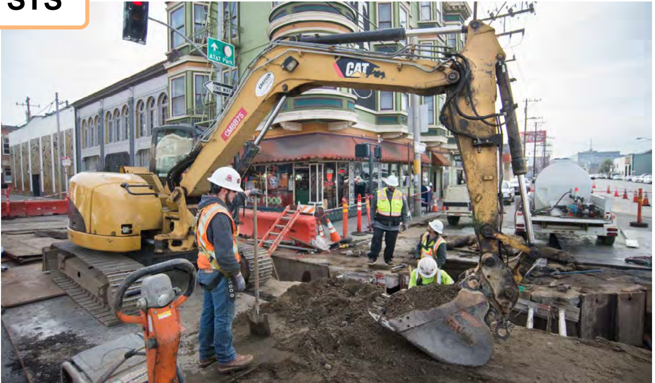
At the corner of 4th and Bryant, work to upgrade and relocate existing utilities is ongoing.
