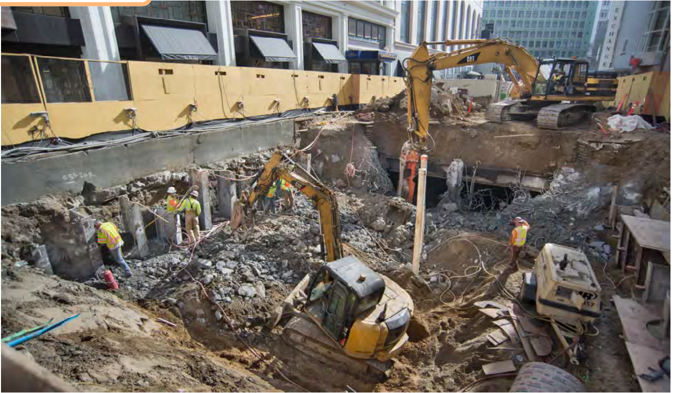
Workers break through the south headwall of the station, exposing the interior of the south concourse just south of O'Farrell.
