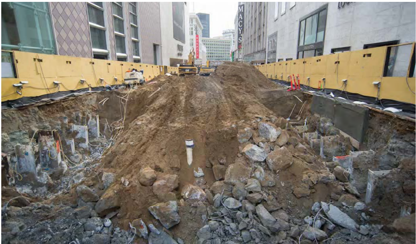
A partially-excavated site just south of Geary, where a section of station roof deck will be installed.
