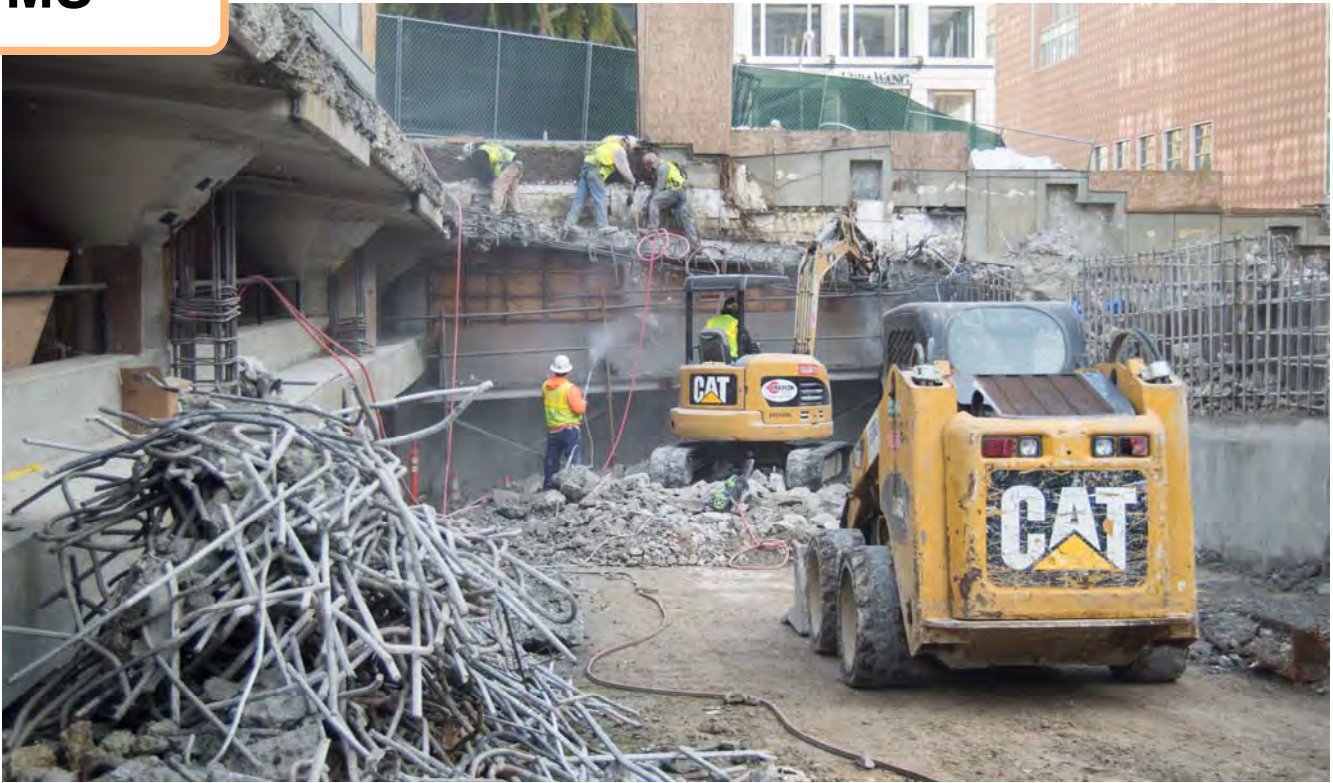
Rebar collected from demolished sections of the Union Square Garage roof lay piled while work to finish demolition goes on in the background.
