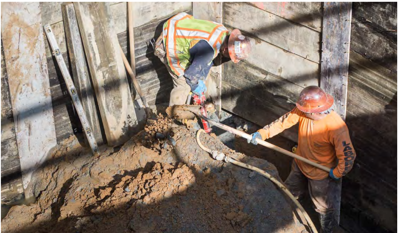
A worker uses a pneumatic spade to loosen hard soil while another removes it from near the shoring wall inside Chinatown Station's north access shaft.
