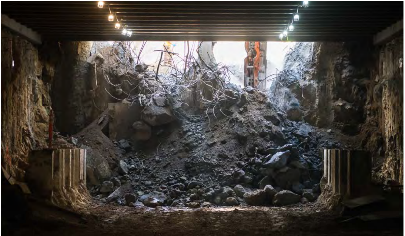
Light pours in the south concourse for the Union Square/Market Street Station, following the removal of part of the south headwall.
