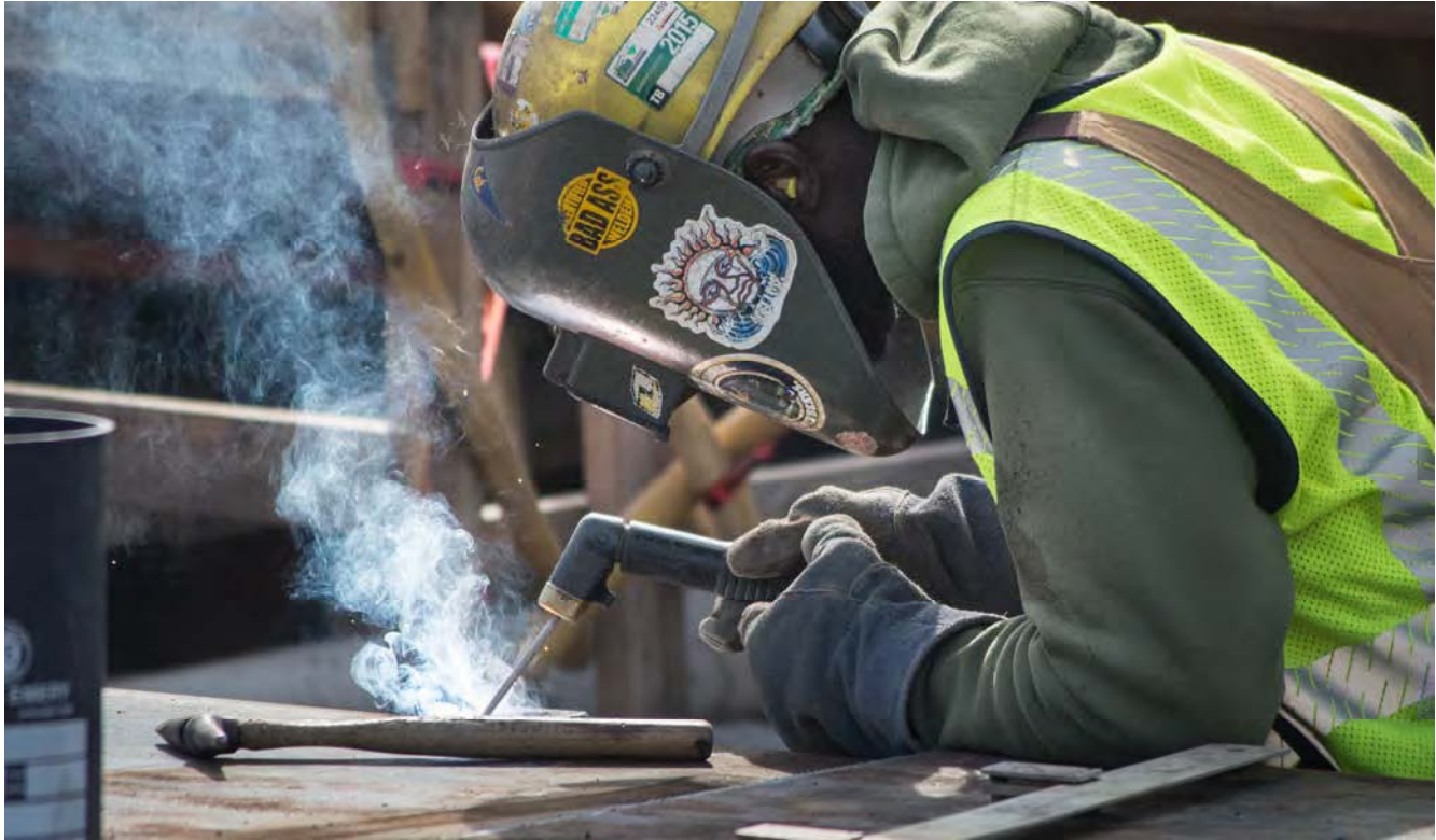
A welder works on steel panels at the Yerba Buena/Moscone Station site.
