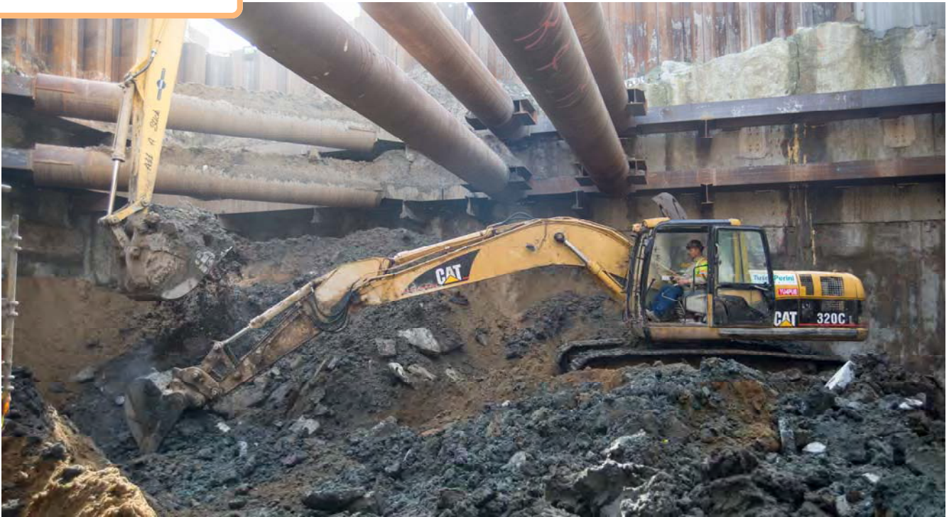
An excavator operator extends the arm out to drop soil precisely under where the surface excavator operator lowers his bucket.
