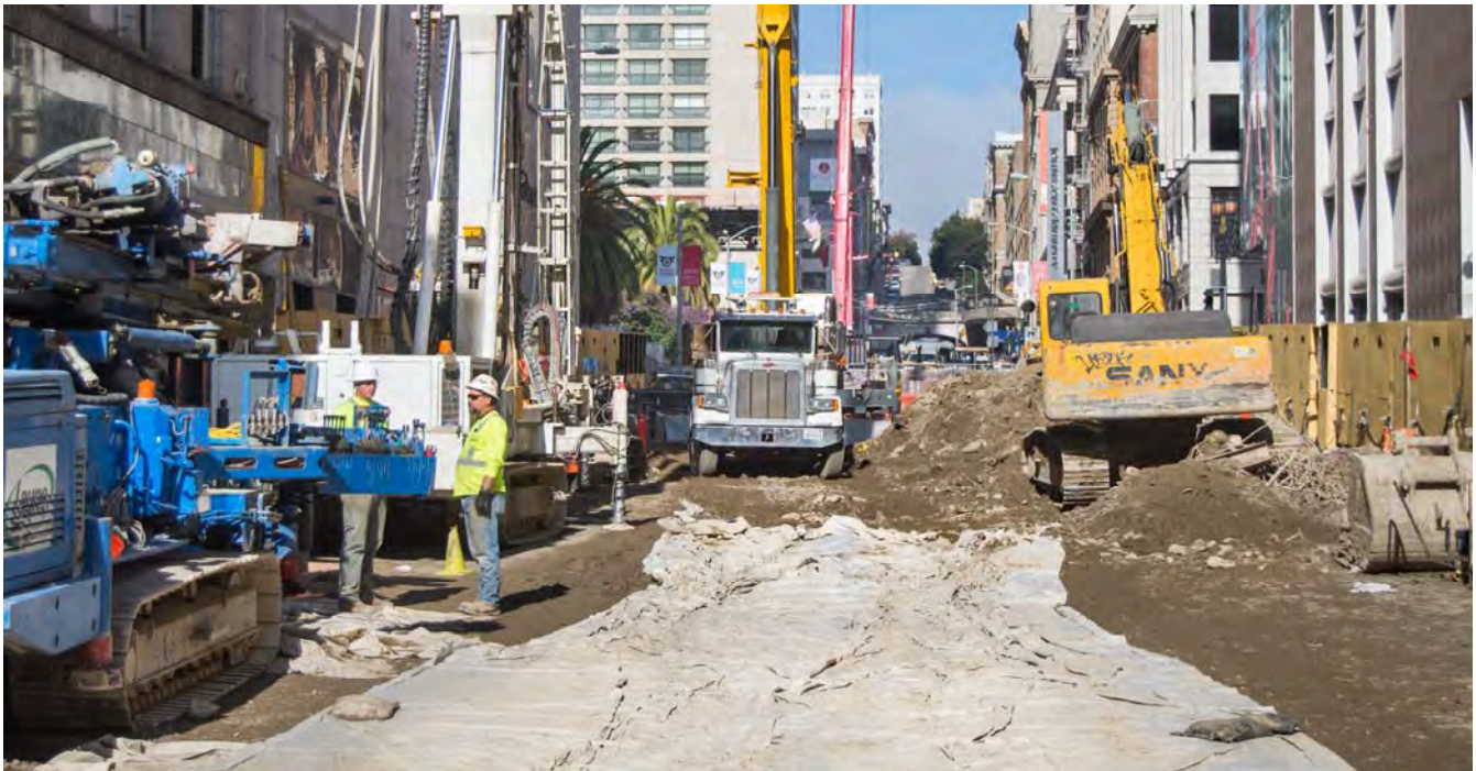
With work restarting after the holidays on Stockton between Ellis and Maiden Lane, drill rigs have been set up to conduct soil improvement work.
