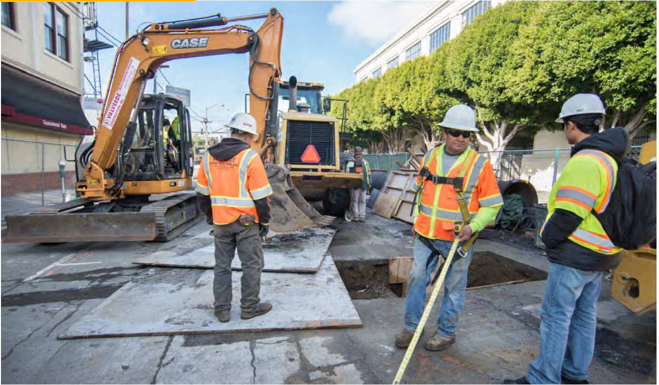
Workers measure an opening being covered by steel plates at the end of the work day.
