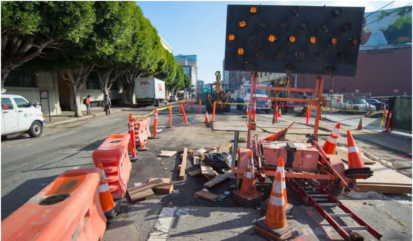
Arrow signs, barriers, and cones help drivers navigate the ever-changing landscape of 4th Street, where utility work is ongoing.
