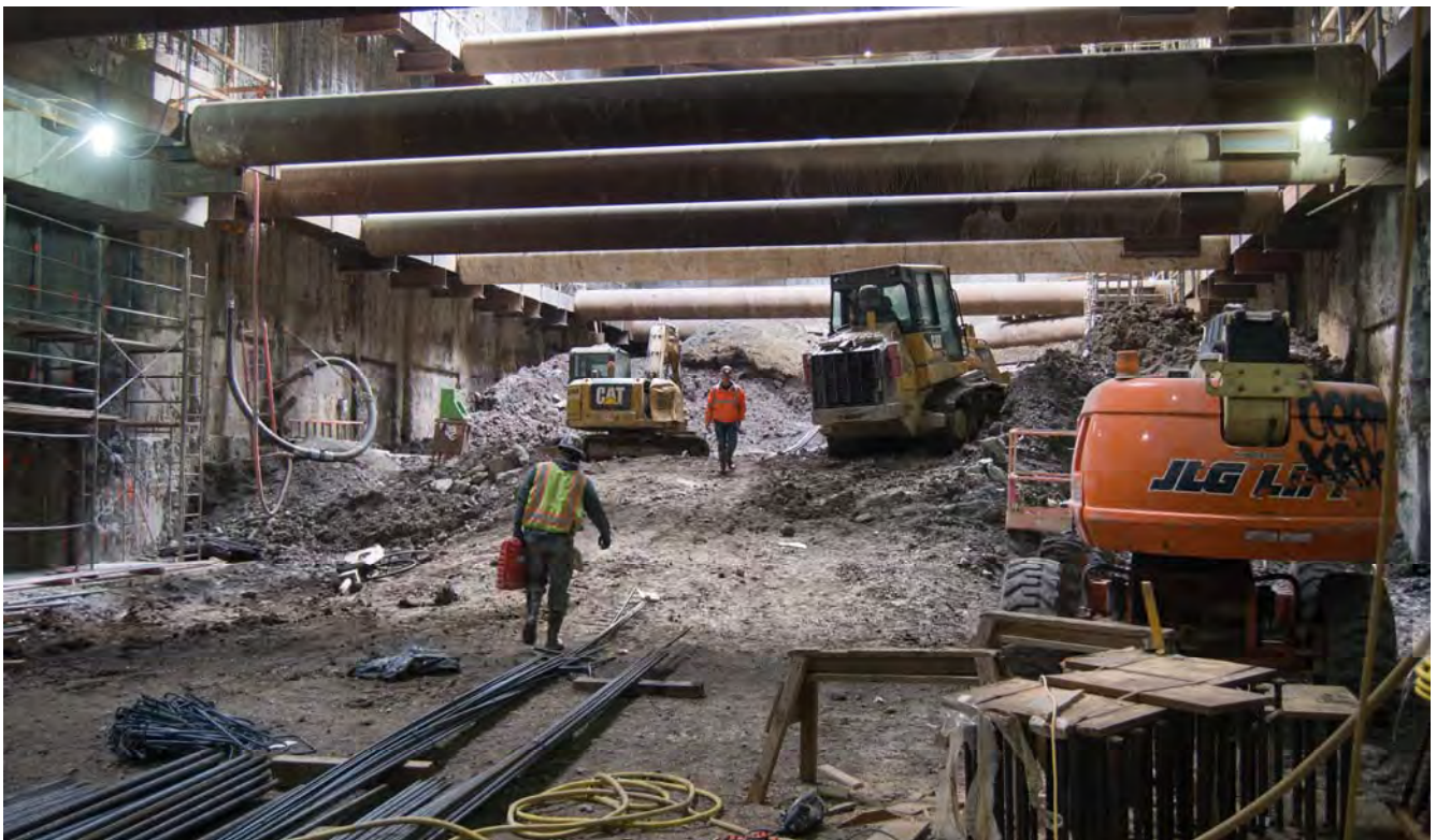
Temporary steel supports loom overhead at the bottom of the current level of excavation inside the headhouse.
