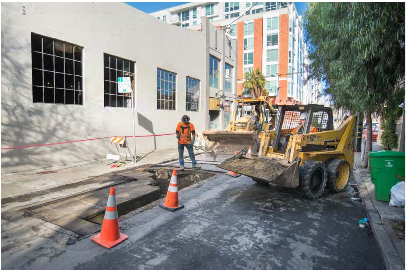
Workers fill in part of a trench used to locate existing utilities below ground on Freelon Alley.
