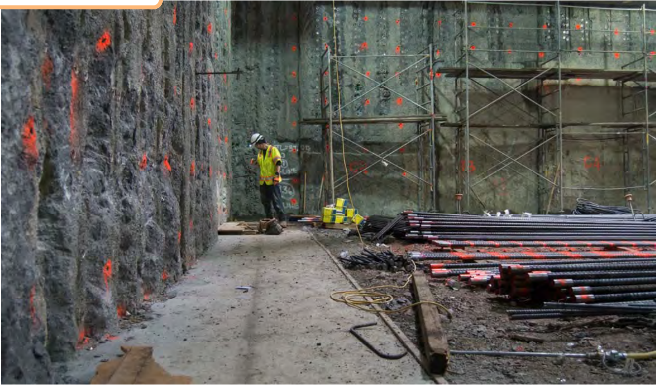
Holes drilled in the slurry wall for rebar fitting are inspected at the north wall of the headhouse.
