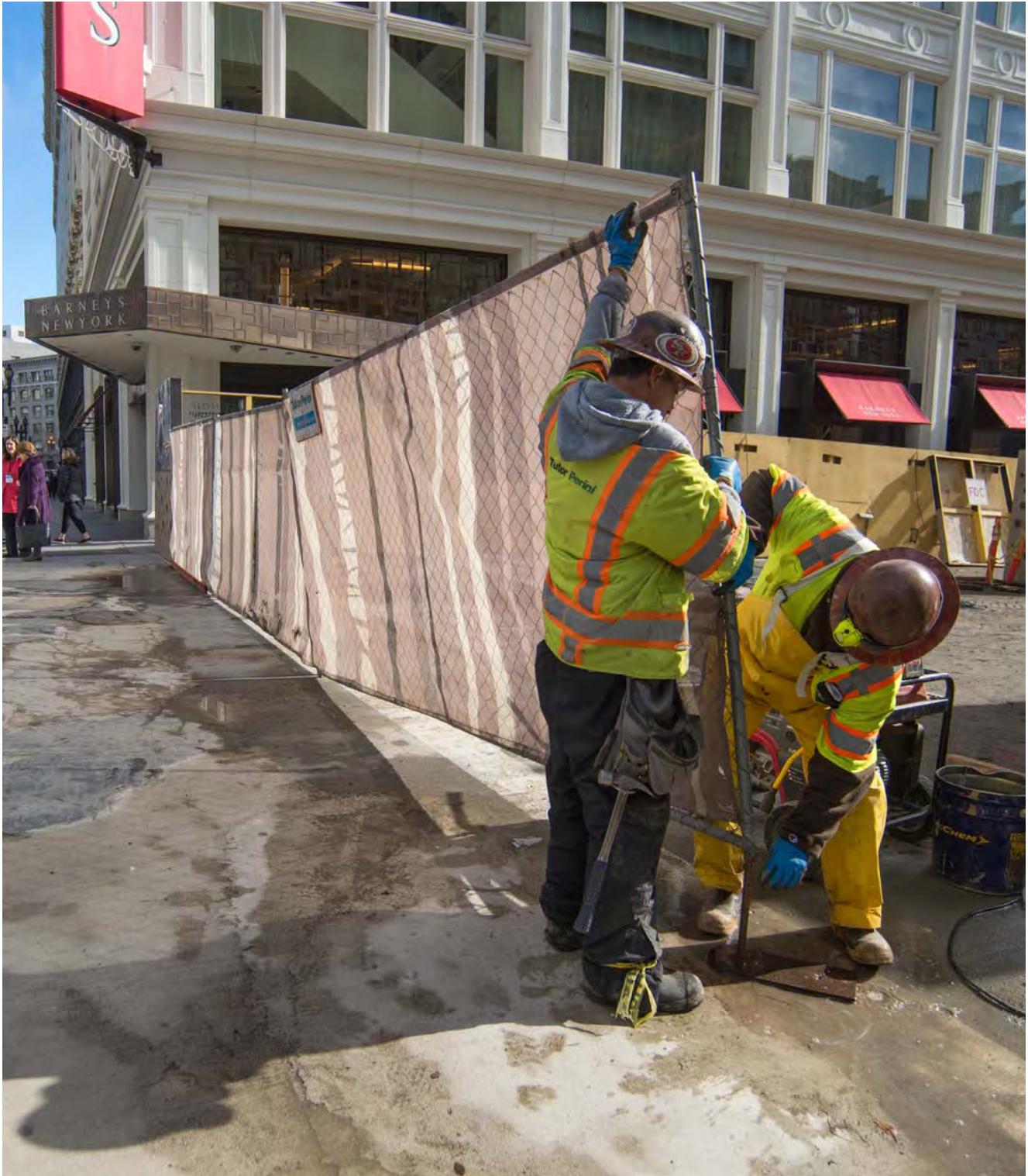
Two workers reinstall safety fencing at the north end of the work site between O'Farrell and Ellis on Stockton, following the end of the holiday work moratorium.
