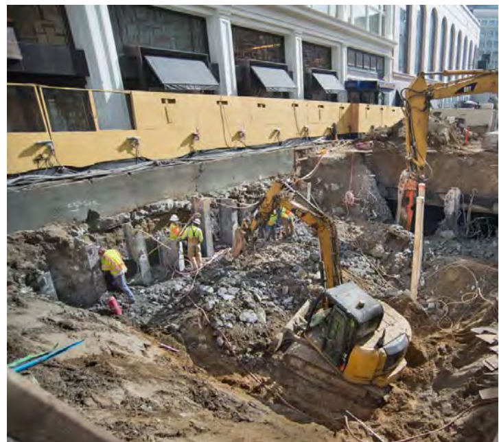
3 Excavation begins at the remaining work sites to finish the station roof
