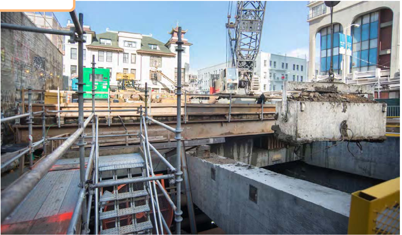
A bucket of excavated material is lifted from the station headhouse interior, at the surface of the structure on Stockton Street.
