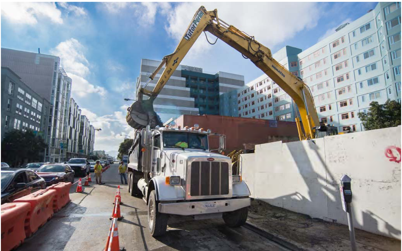
An excavator fitted with a long arm loads a dump truck with earth excavated from the station box, on the north side of Folsom west of 4th.
