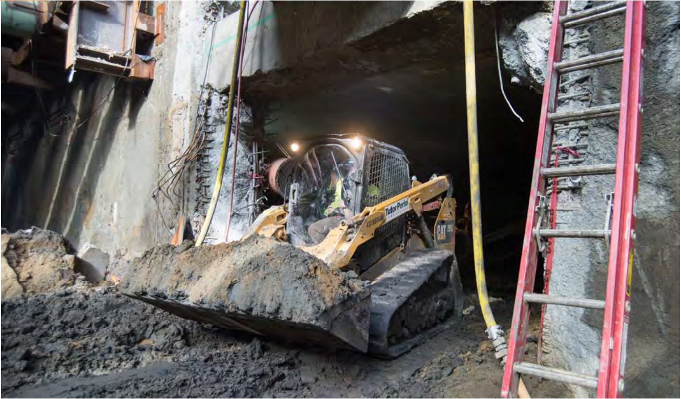
A bobcat with a bucket full of soil removed from the station box interior emerges from the access portal on the east side of the headhouse site.
