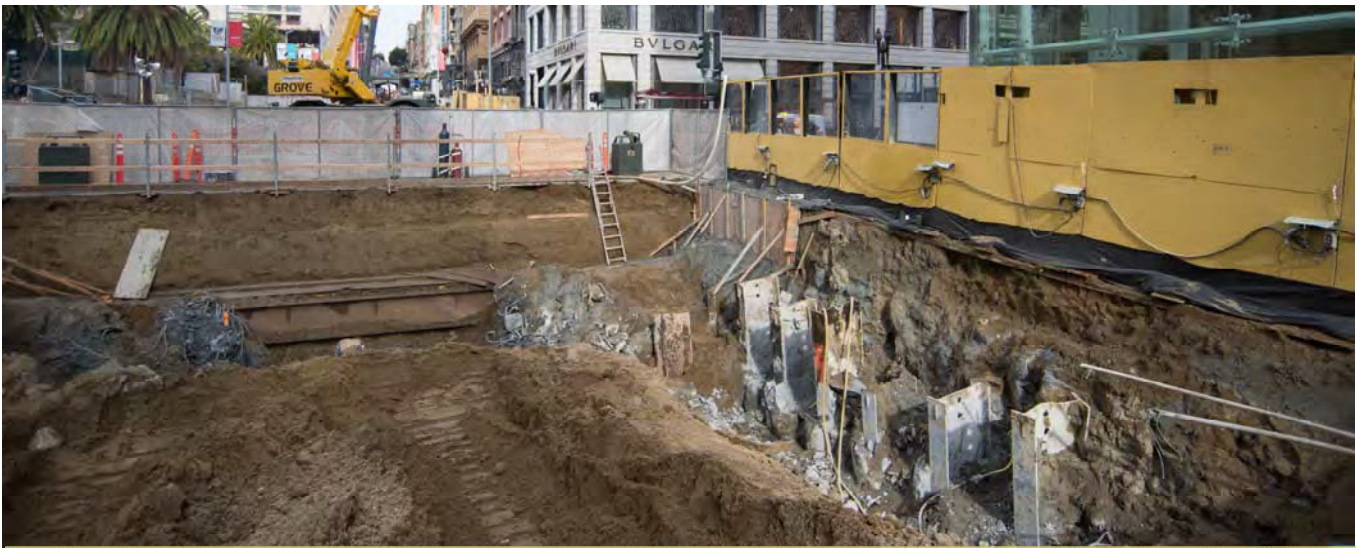
Steel beams jut from structural piles installed just south of Geary Street on Stockton, where site excavation is underway.
