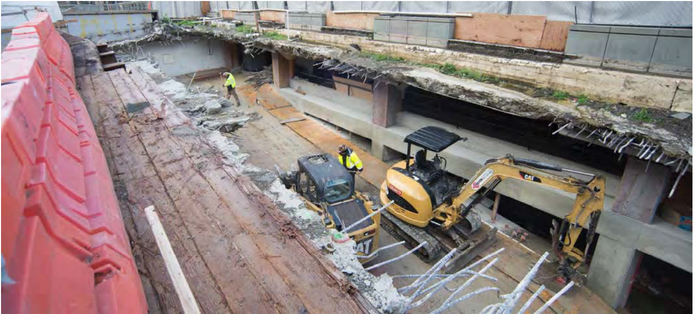
Rebar extends past sections of concrete being carefully demolished at the southeast corner of the Union Square Garage, where work to construct the future north station entrance has been underway.
