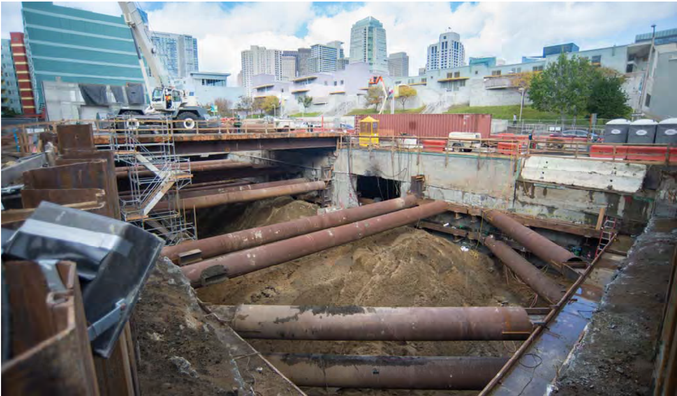
Temporary steel supports span the width and the corners of the Yerba Buena/Moscone Station headhouse, while excavation of the station box is underway under 4th Street.
