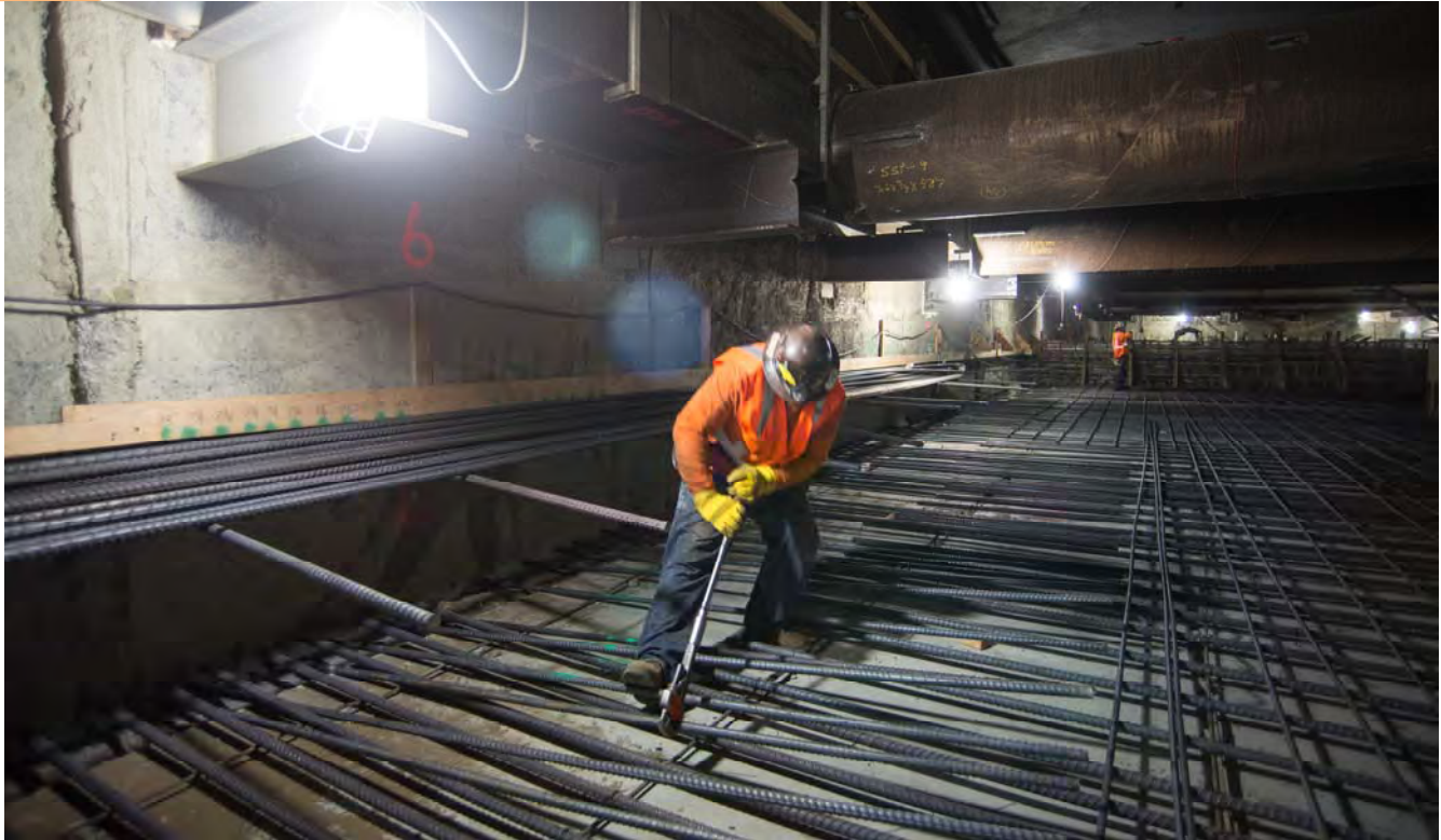
A worker uses a large wrench to screw sections of rebar into the exterior slurry walls. This is done to tie in all the rebar cages with each other, creating structural strength.
