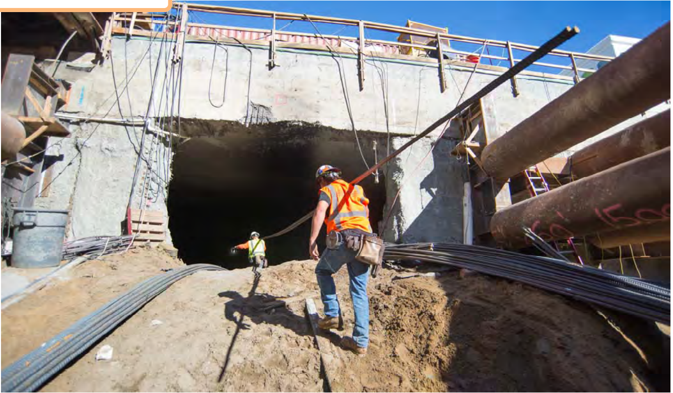
Workers bring in each strand of rebar one at a time, installing them inside the station box.
