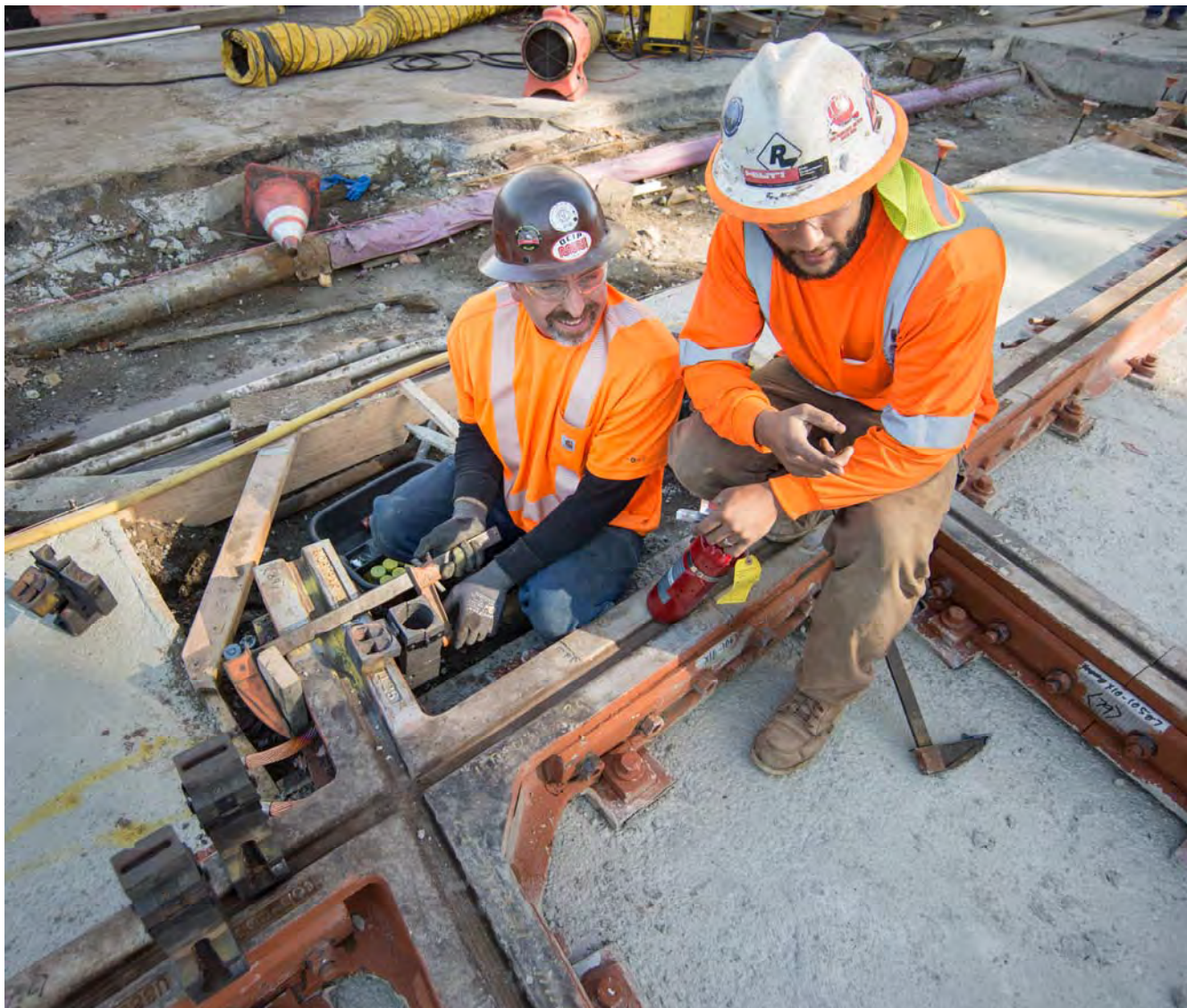
Two men discuss work at the 4th and King intersection, where a new track configuration was installed.
