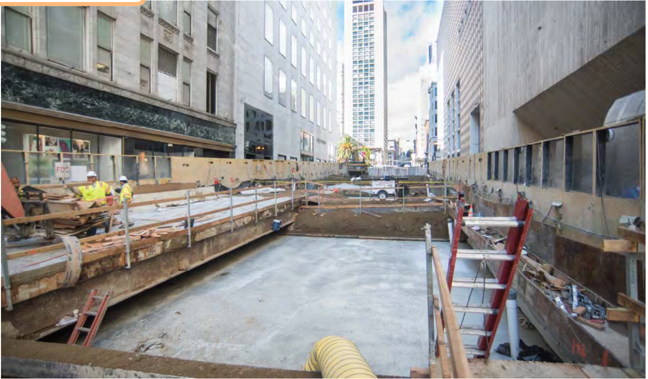
One of the last sections of roof deck to be installed between Geary and O'Farrell on Stockton Street, before being backfilled and graded.
