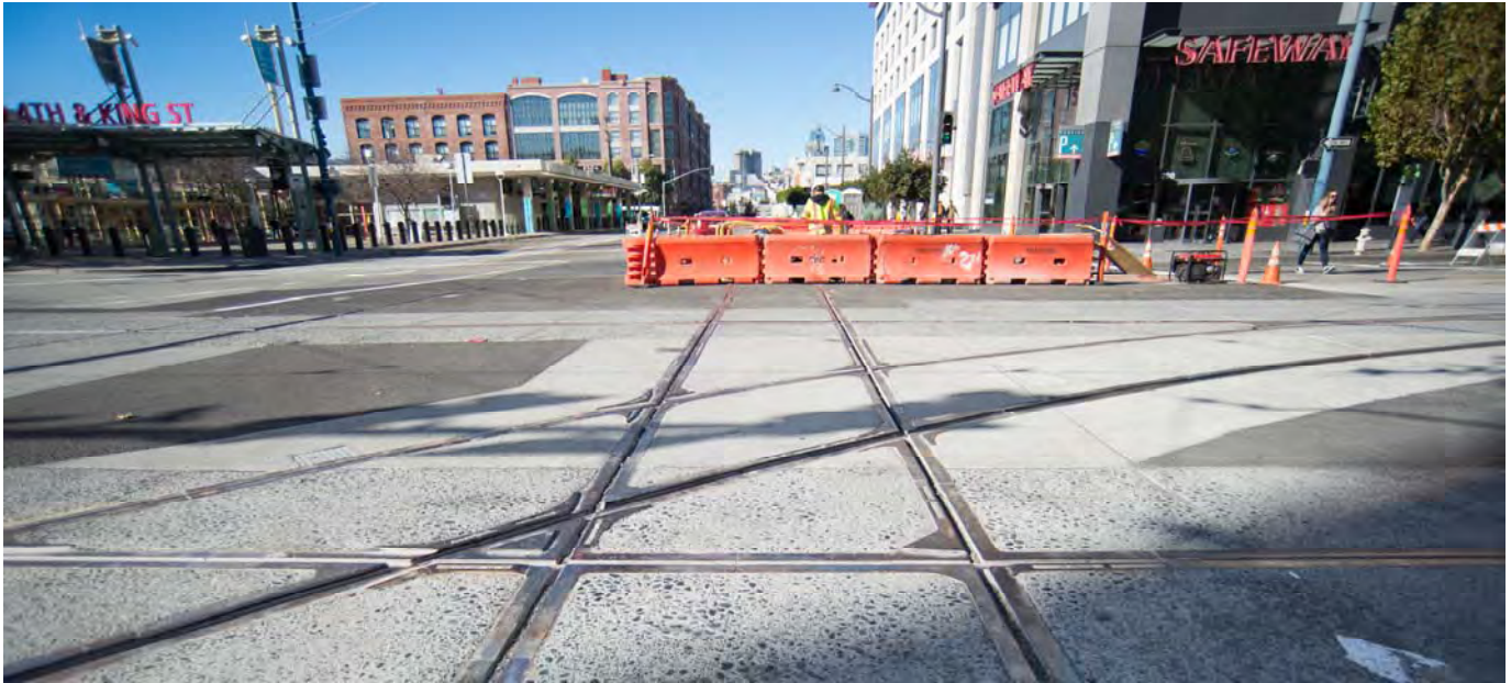
Northbound tracks now sit in the intersection of 4th and King, part of a new track configuration installed in two phases, most recently over the week of Veteran's Day.
