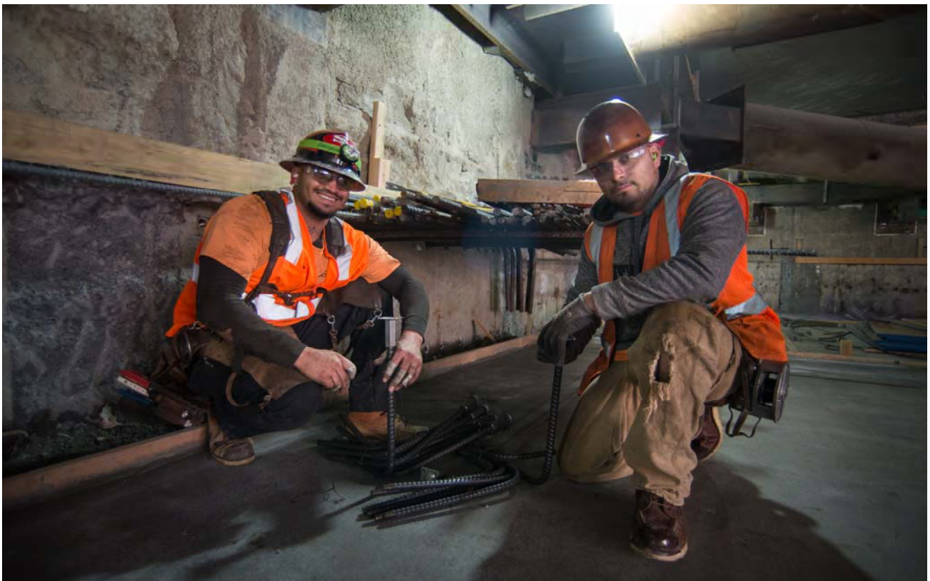
Two workers pose before installing rebar in the exterior slurry walls of the station box under 4th Street.
