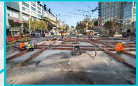
4th St. Surface Track, Systems (STS)
