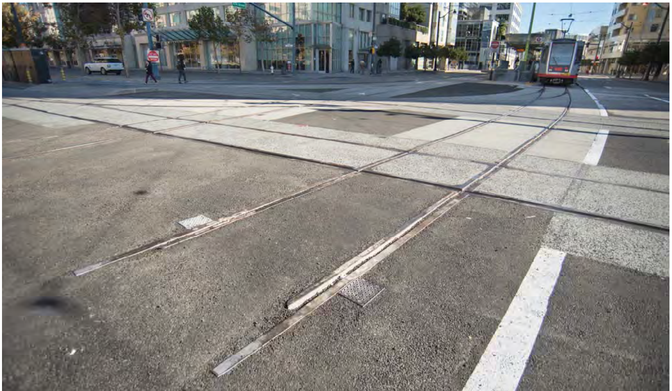
Temporary "ghost" tracks show the direction up 4th Street, where future T Line trains will travel once the Central Subway has opened.
