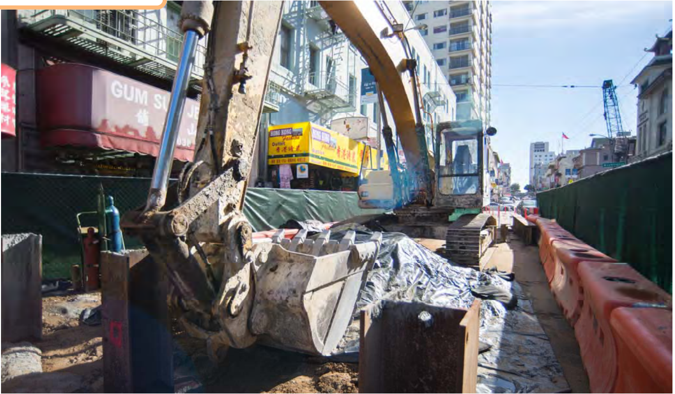
Ground has been broken to construct the north access shaft, where an emergency stairwell will be constructed at the northeast corner of the station.
