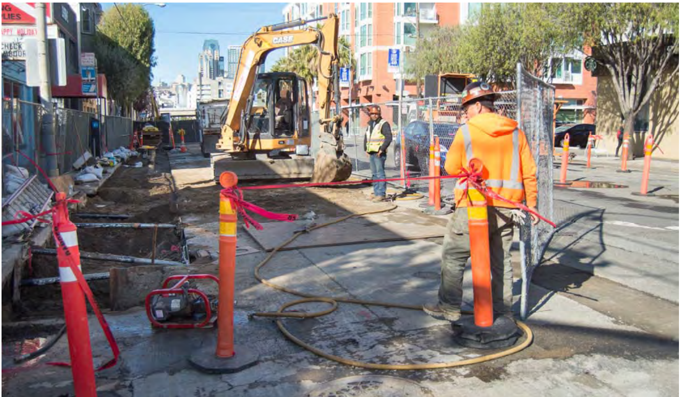
Once utilities in this area were installed, workers backfilled the trench and repaved part of the street.
