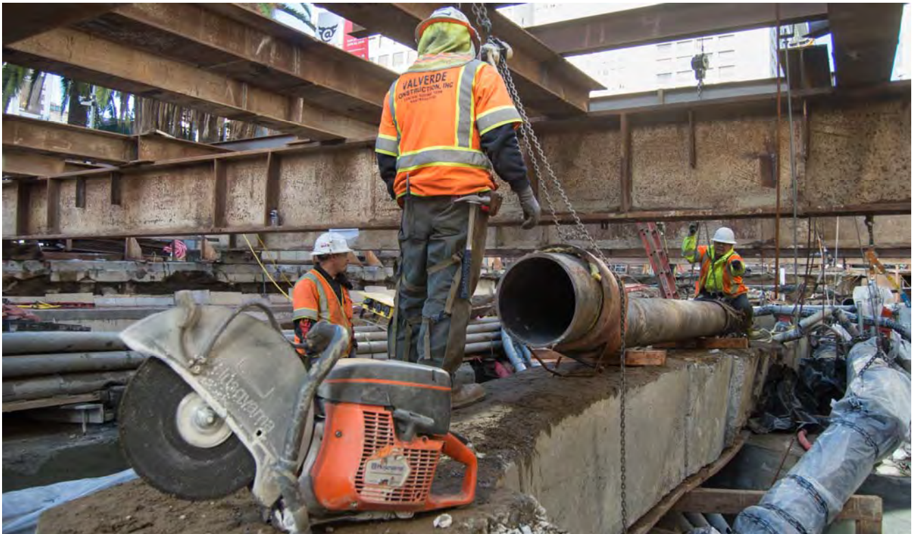
A crew removes temporary sewer pipes suspended beneath the steel truss network laid over Stockton between Maiden Lane and Geary.
