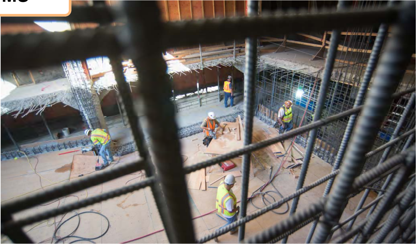
Carpenters and ironworkers share space inside the reconstructed ramp at the southeast corner of the Union Square Garage, where new vehicle ramps are being reconstructed.
