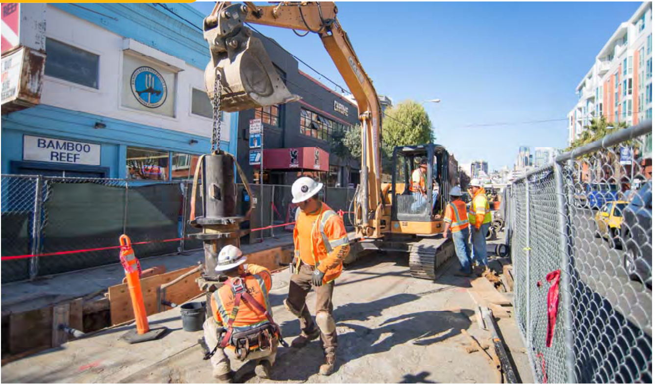
A new section of high pressure water line is installed in a trench on the west side of 4th Street, just north of Brannan.
