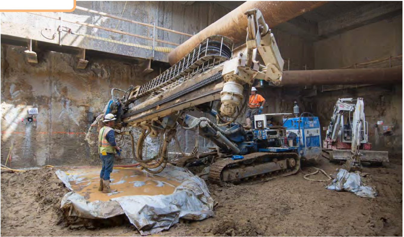
Workers use a drill rig to pump a grout-like solution into surrounding soil, to help waterproof the station headhouse and improve surrounding soil.
