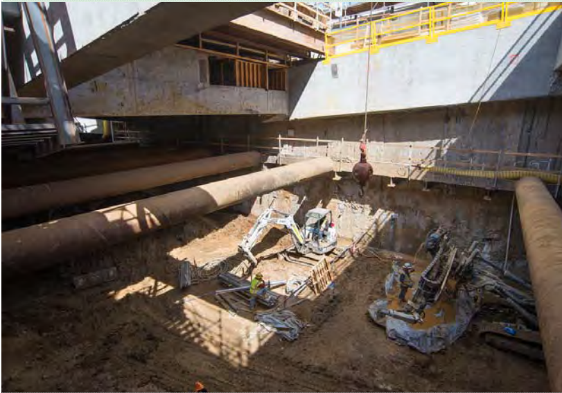
1 Workers use earth-moving equipment to collect material in the central access shaft
