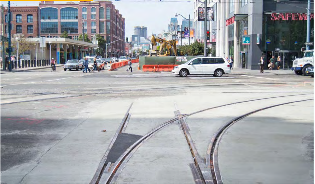
Tracks leading up 4th Street and a temporary surface pad mark where track interchange upgrades were made over Labor Day weekend.
