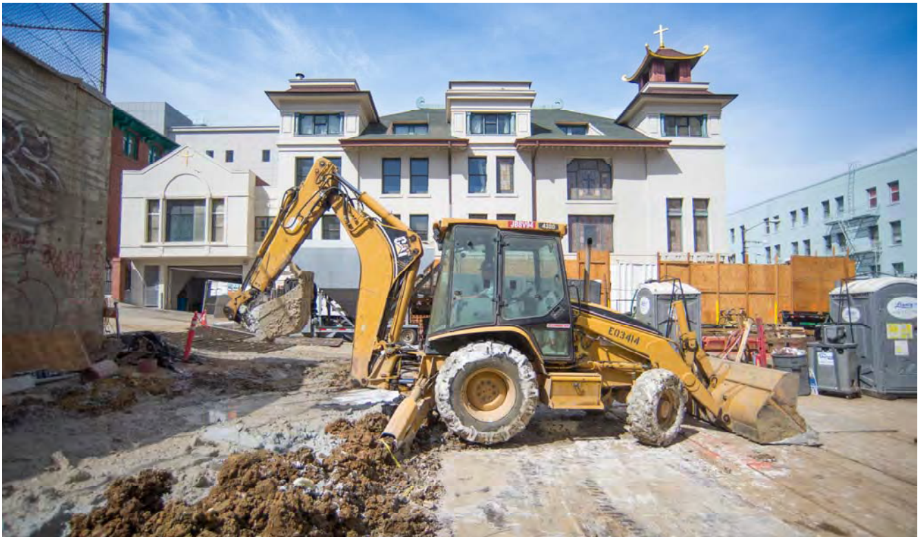
A backhoe moves excavated and slurry material around the roof deck area during drilling operations below.
