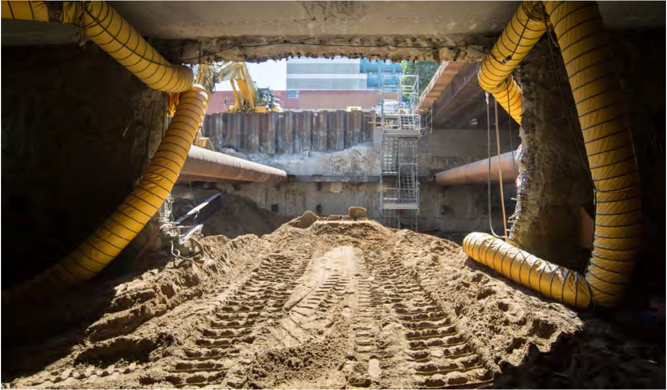
A view out of the access opening created when station box excavation began. This opening will eventually be widened as excavation efforts progress.
