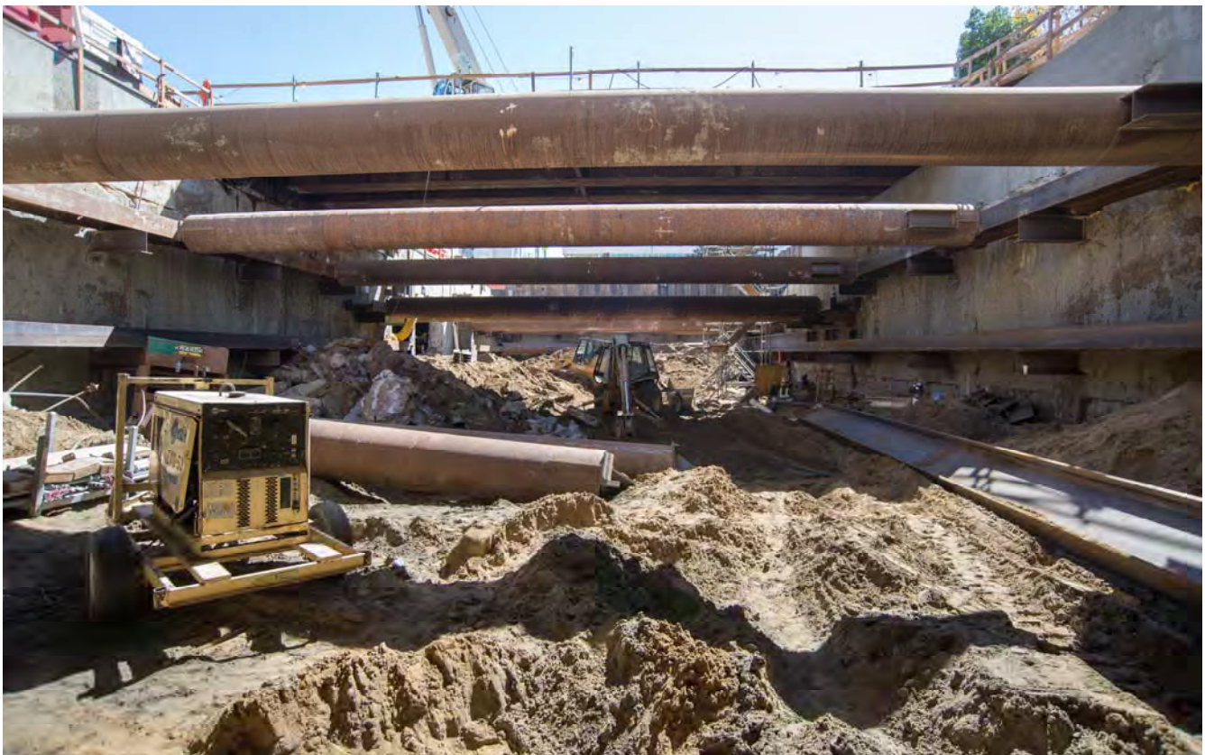
Steel supports span the width and length of the station headhouse. These supports are temporary and will eventually be replaced by reinforced concrete structural elements.
