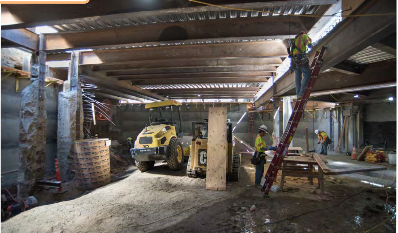
Before the contractor can backfill the site and restore the roadway, work to install corrugated steel panels, rebar, and finally concrete is completed.
