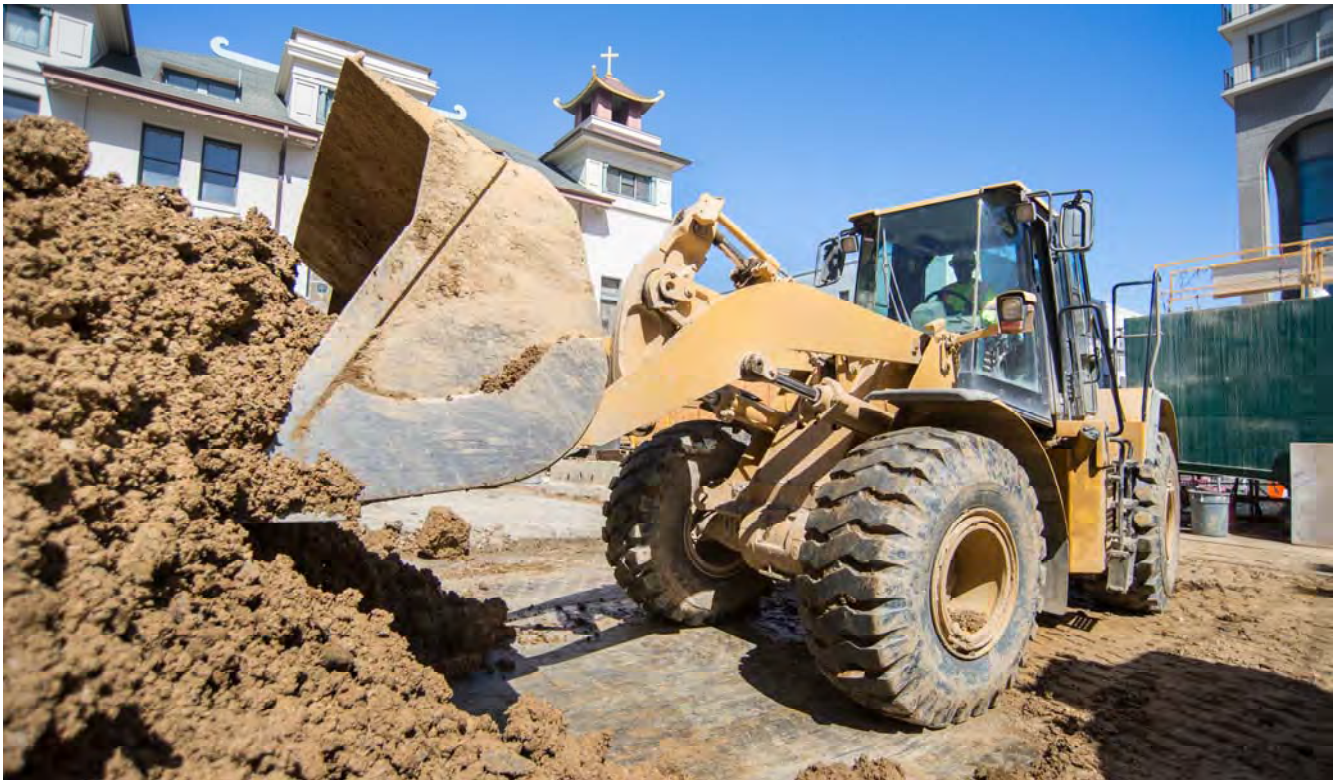
A loader operator moves excavated material around the staging area where dump trucks line up to be loaded.
