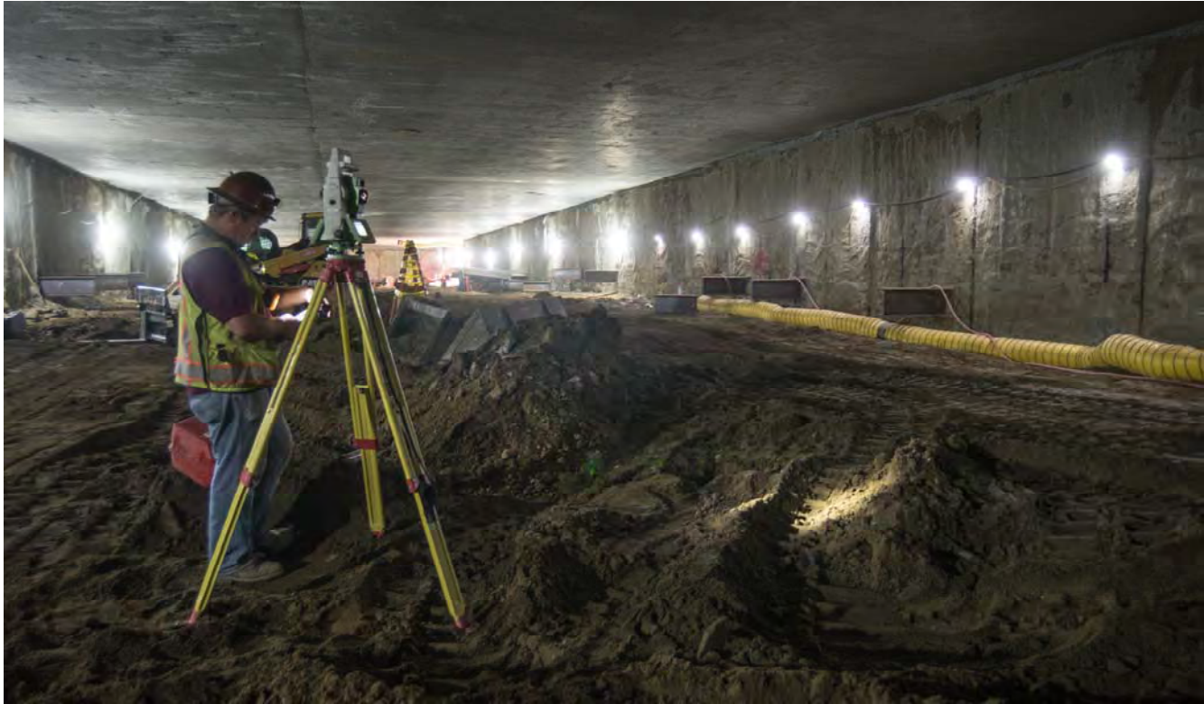
A surveyor marks down measurements inside the north end of the partially-excavated station box.
