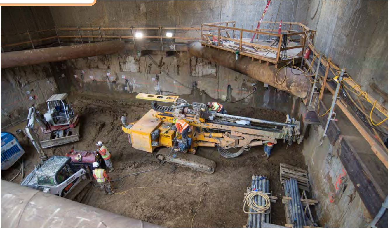
A drill rig is set up against one of the station headhouse's exterior walls to engage in soil improvement activity.
