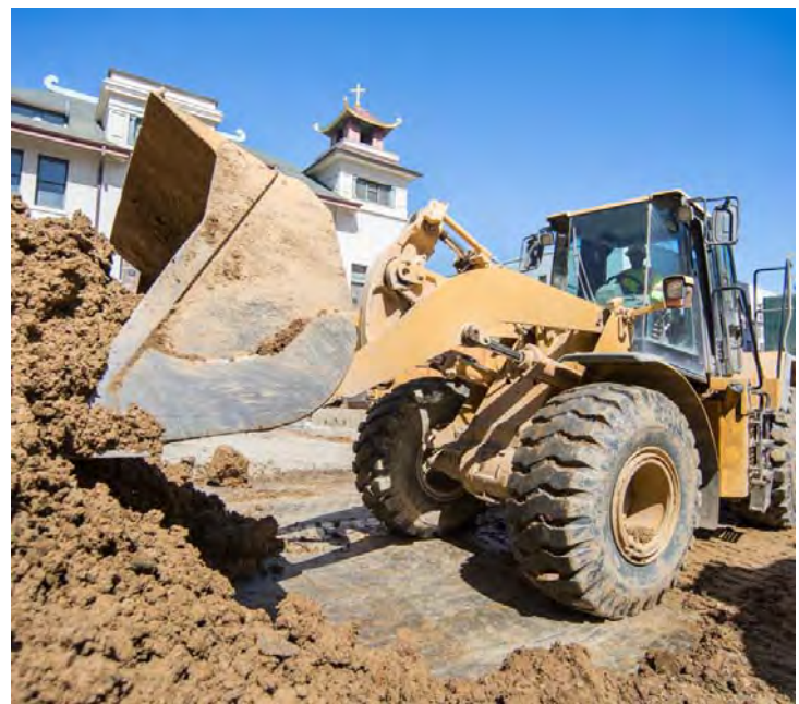
3 Material is piled to be offloaded onto waiting dump trucks at Washington St.
