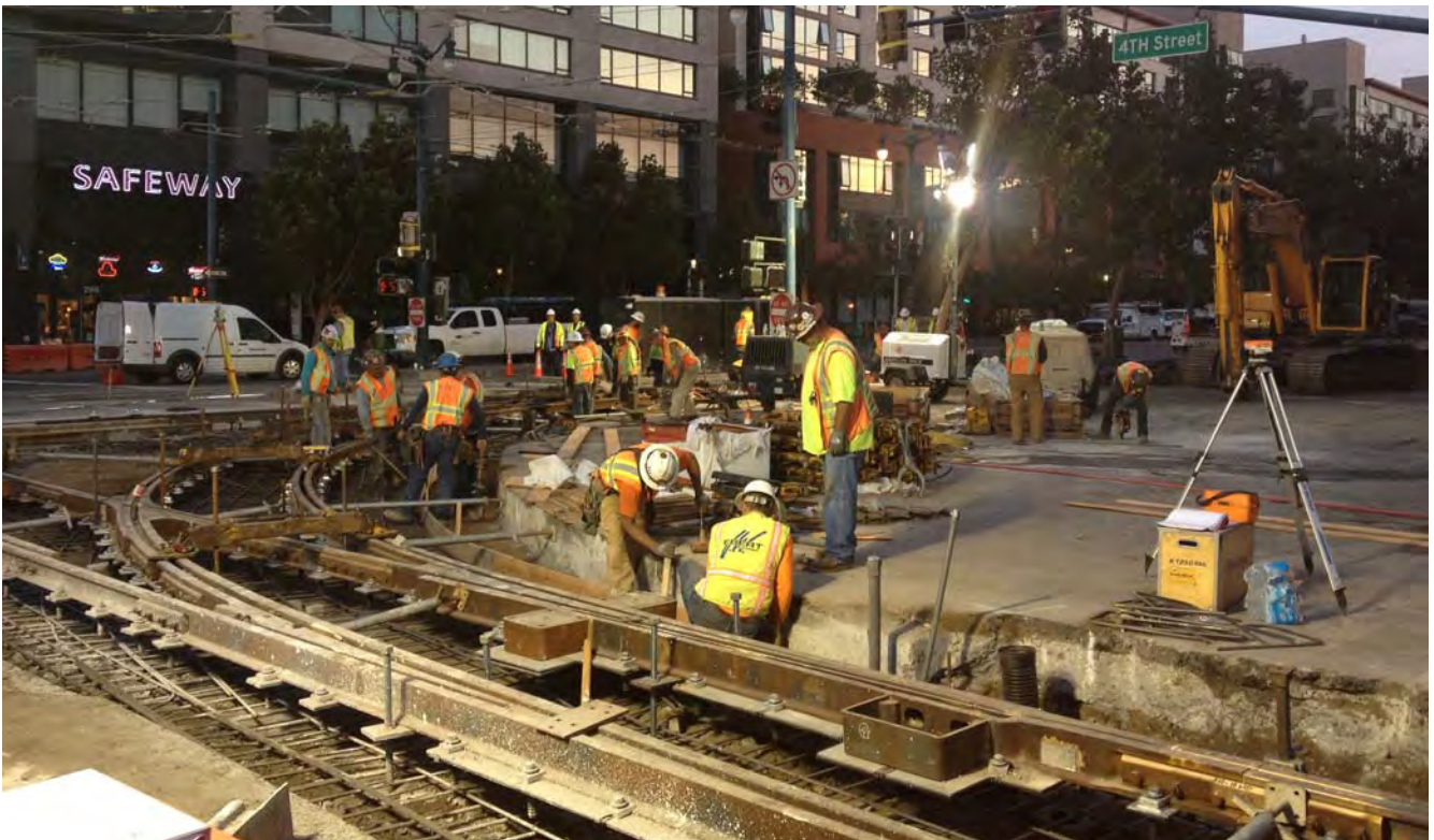
A new track interchange is "hung" prior to pouring the new, reinforced concrete base.
