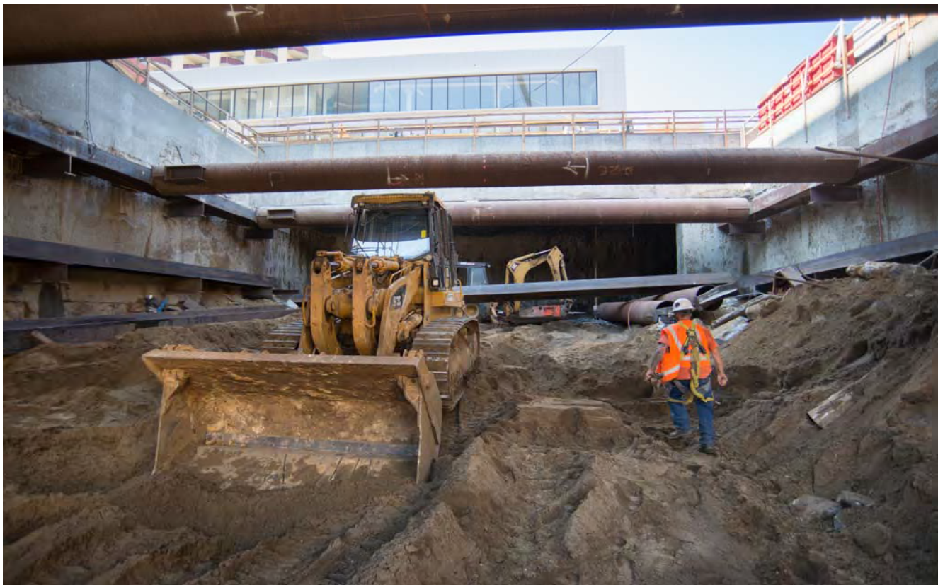
As excavation of the Yerba Buena/Moscone Station headhouse has progressed, steel supports have been temporarily installed.
