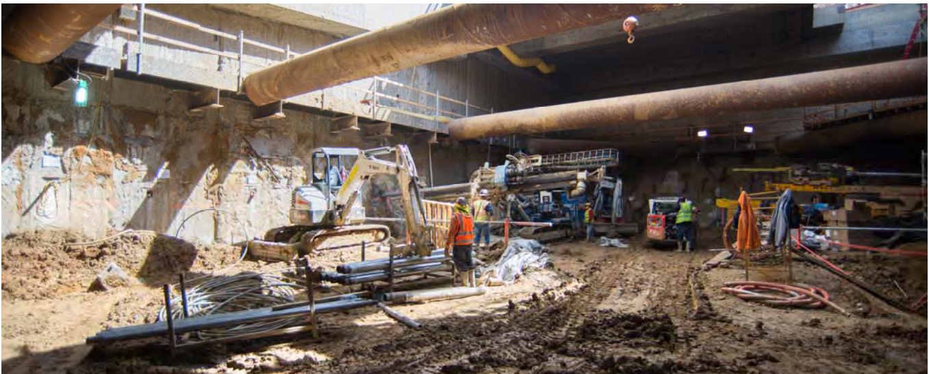
Workers operate drilling and grouting equipment to waterproof the inside of the Chinatown Station headhouse, while excavation is temporarily paused.
