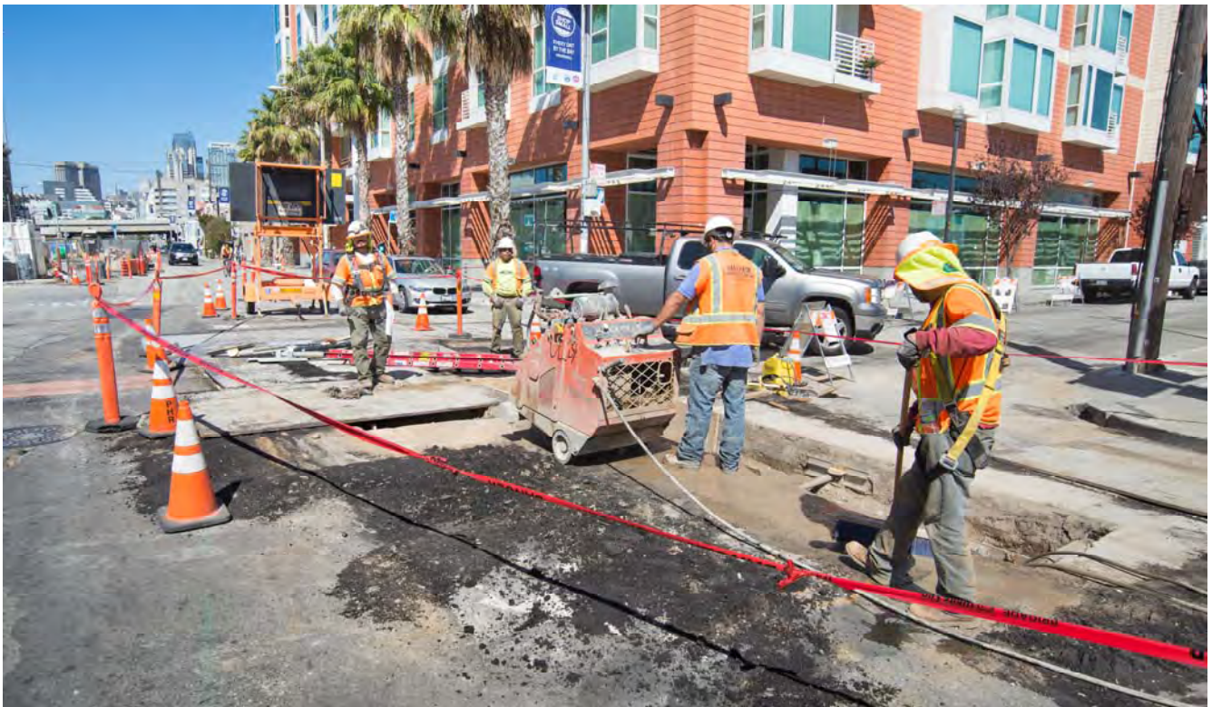
Workers upgrade a century-old water line on 4th Street at Freelon Alley. Work to upgrade utilities along the surface portion of the alignment is ongoing.
