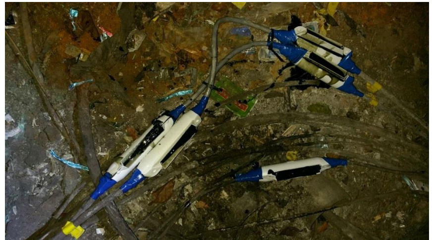
Temporary solution for corroded at MMT
