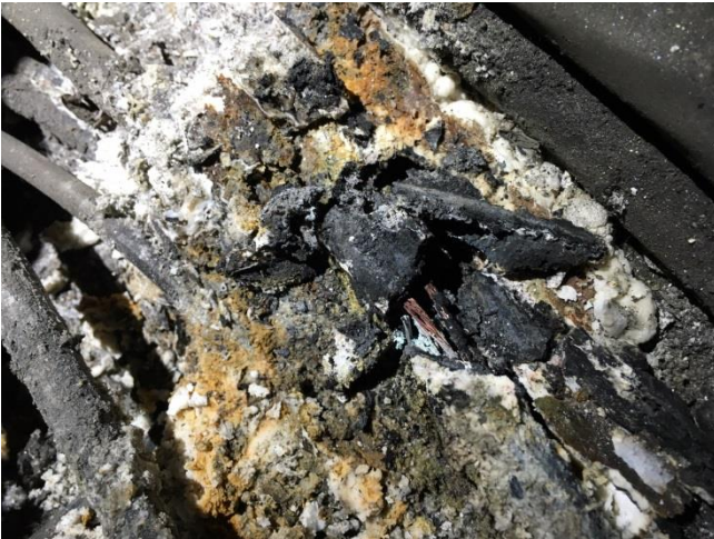
Insulated track switch power wiring corroded at MMT
