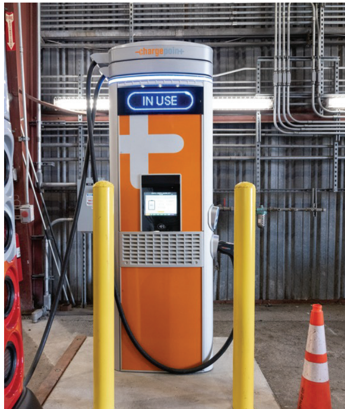
Figure 6-5: Charging Station at Marin Facility
