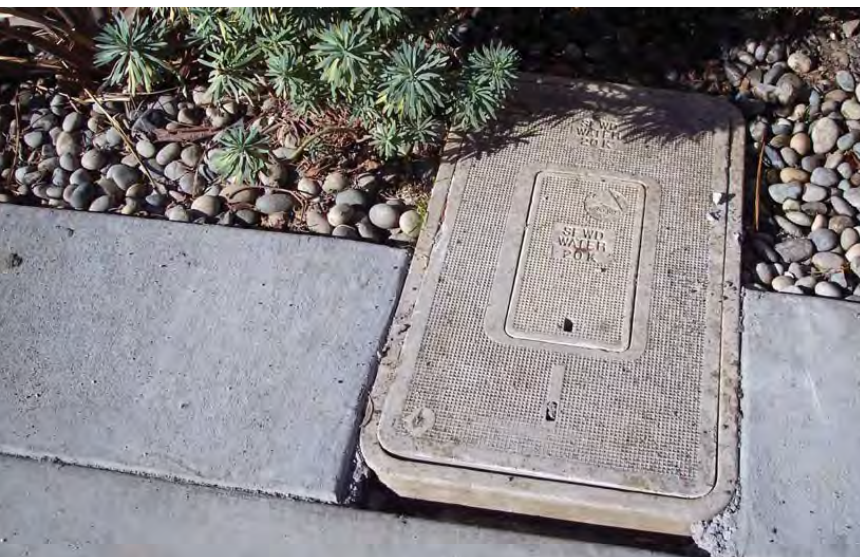
▲ Utility vaults may be located within planting areas as long as access is maintained
