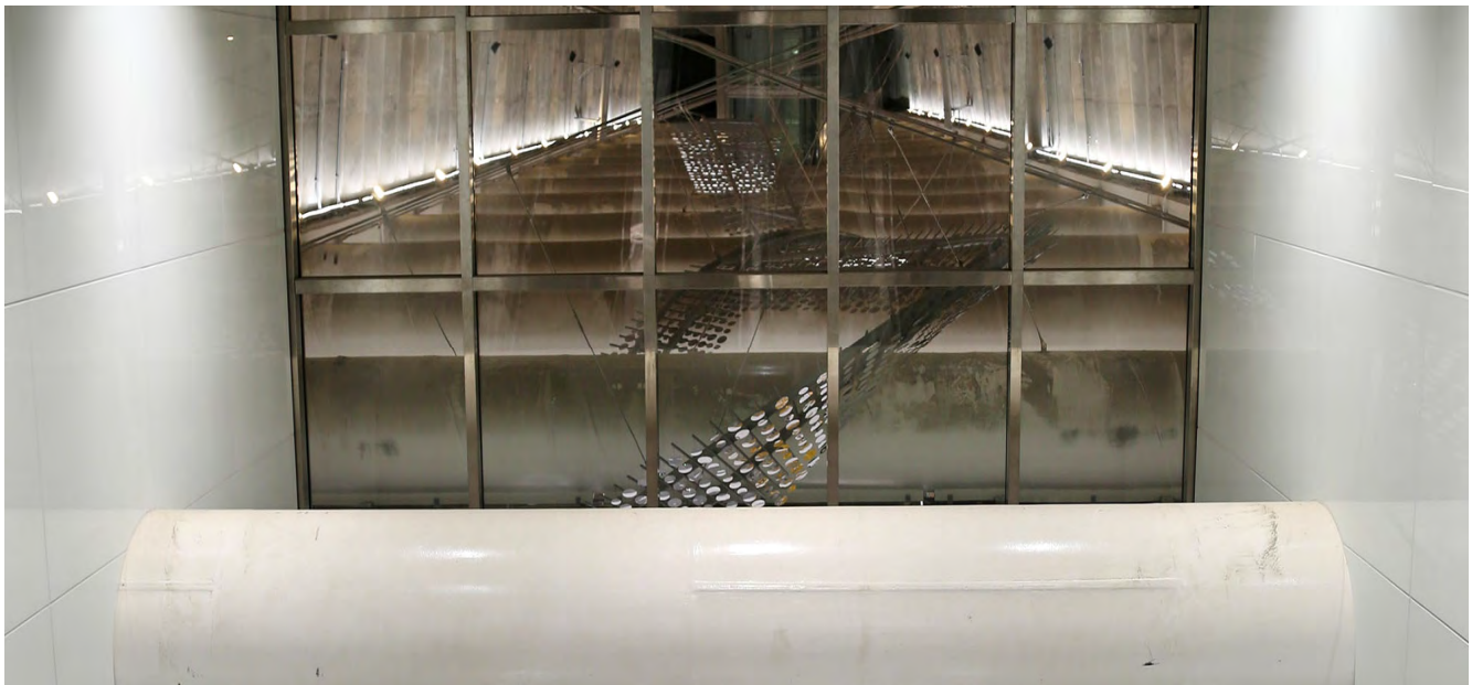
View of seismic bracing above the platform
