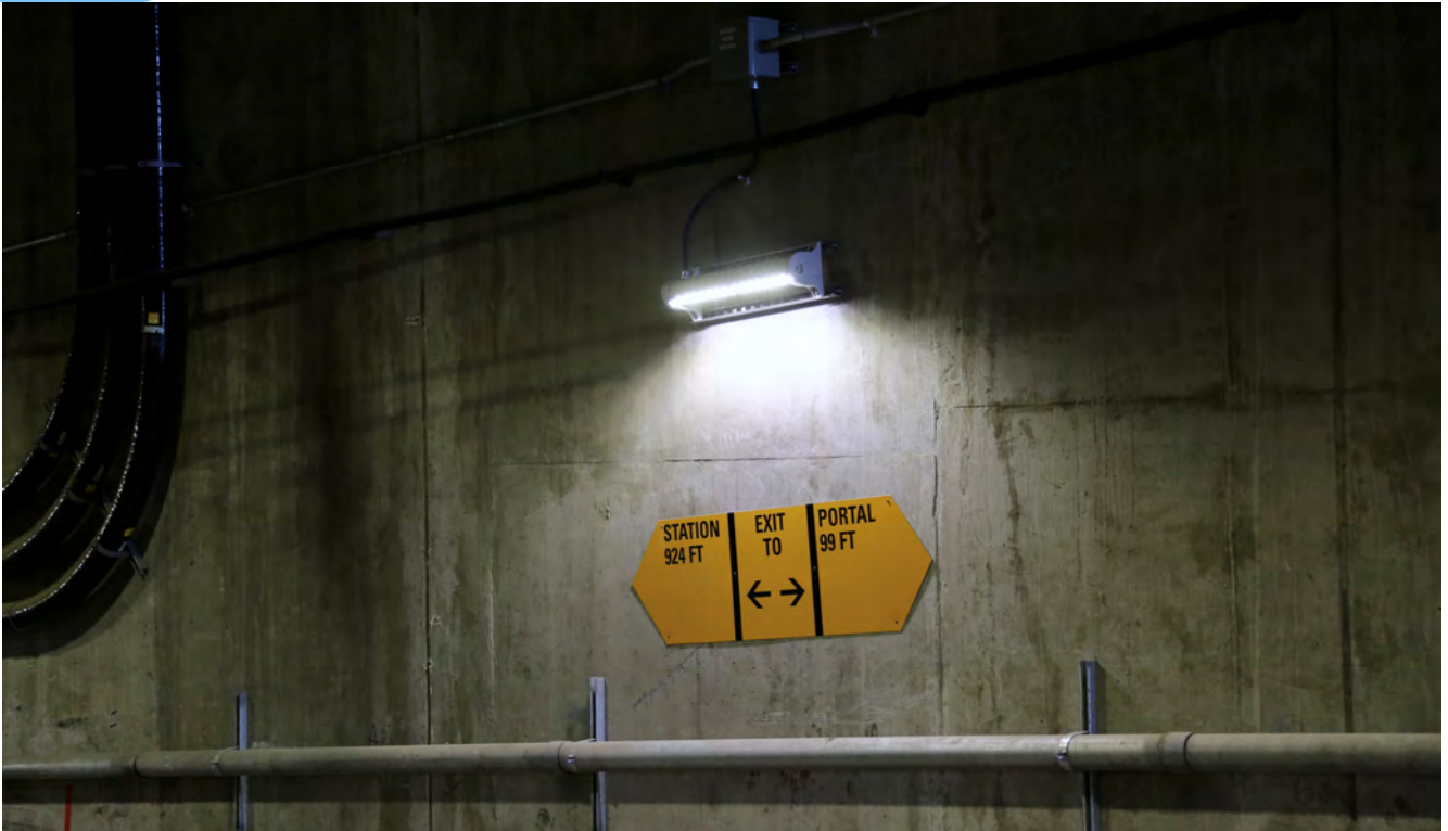
Signage in place in the tunnel
