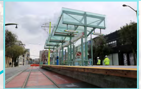
4th St. Surface Track, Systems (STS)
