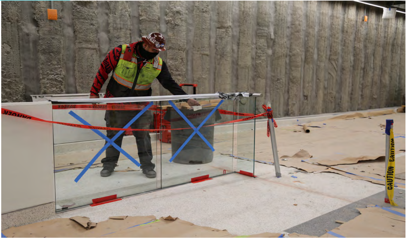
Part of the railing to guide people through the station
