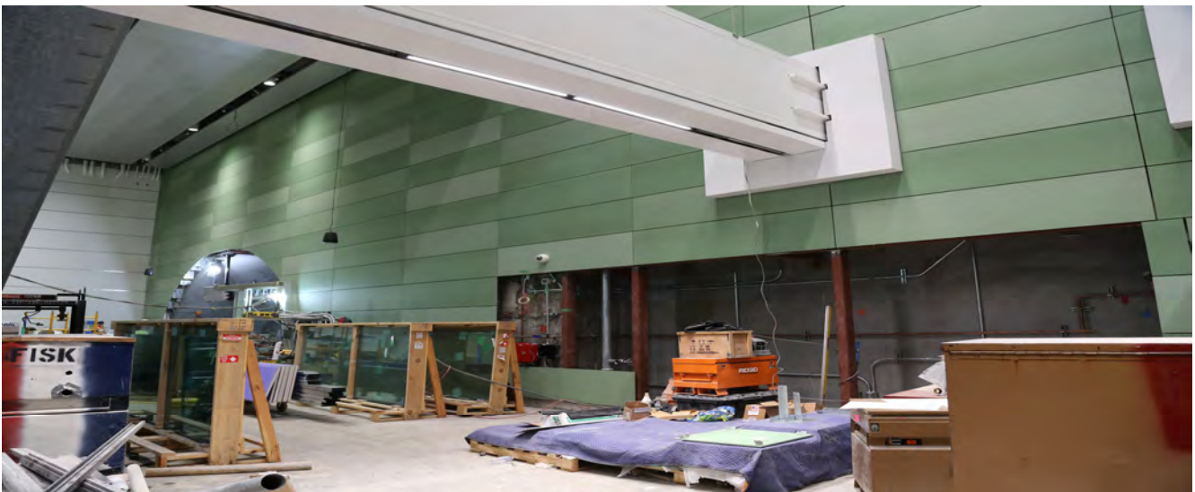
Chinatown station, progress on the wall sliding and the MEP behind it
