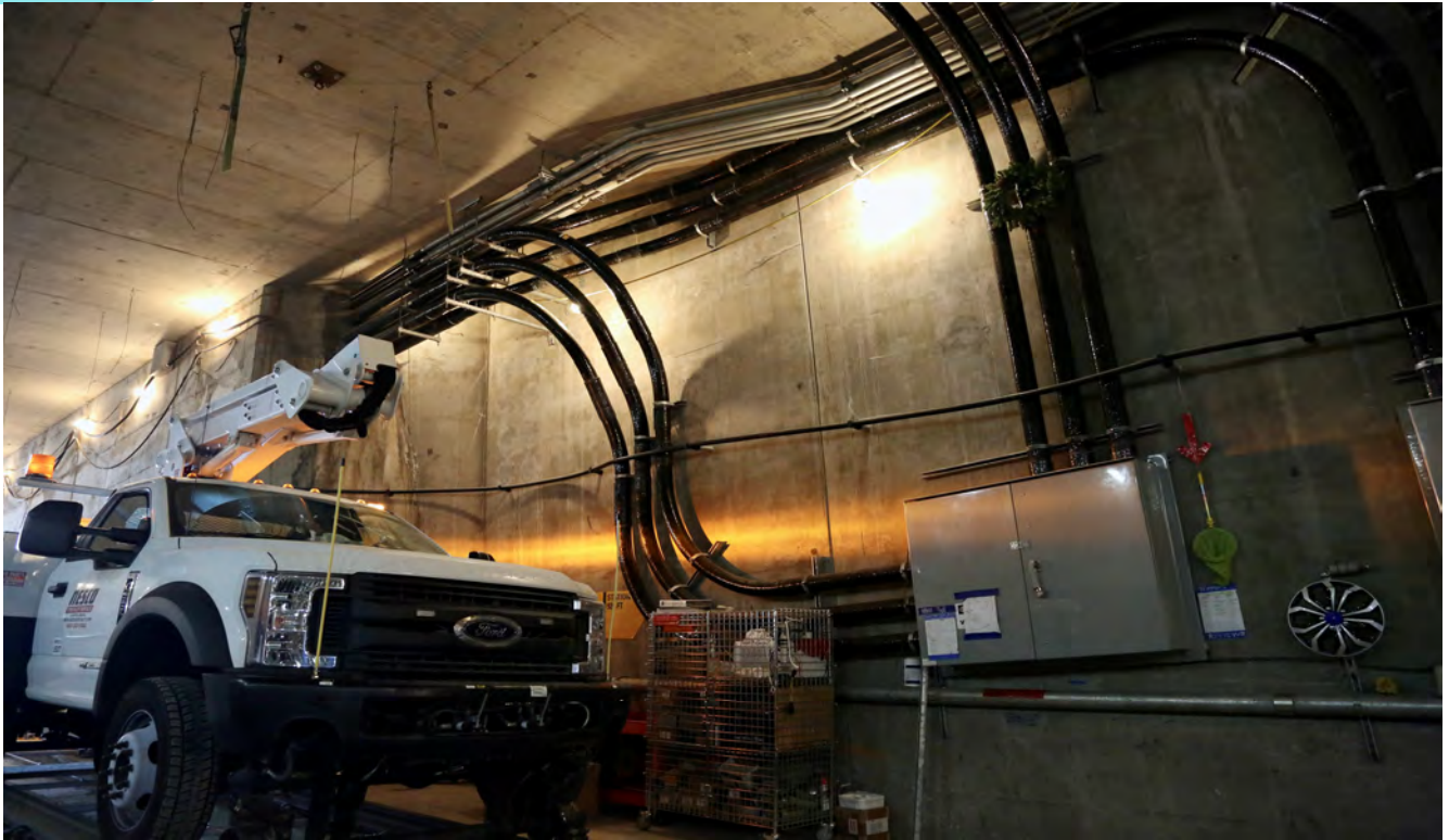
Inside the portal, looking at the conduit on the wall
