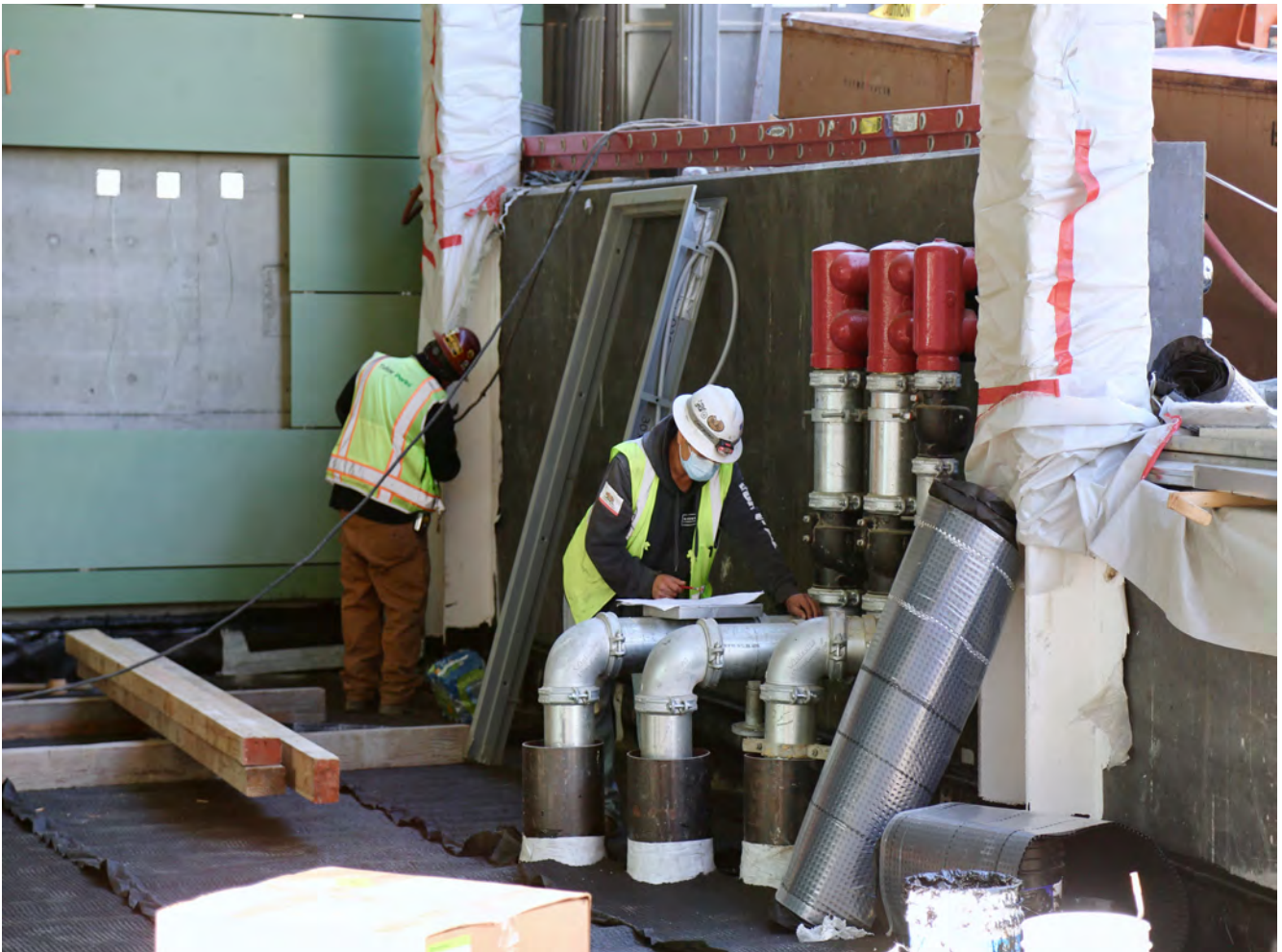
Workers reading plans to ensure that everything is in place before the concrete pour
