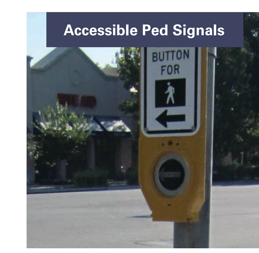
Accessible pedestrian push buttons are easily located by the visually impaired and provide audible signals for pedestrians crossing an intersection.
