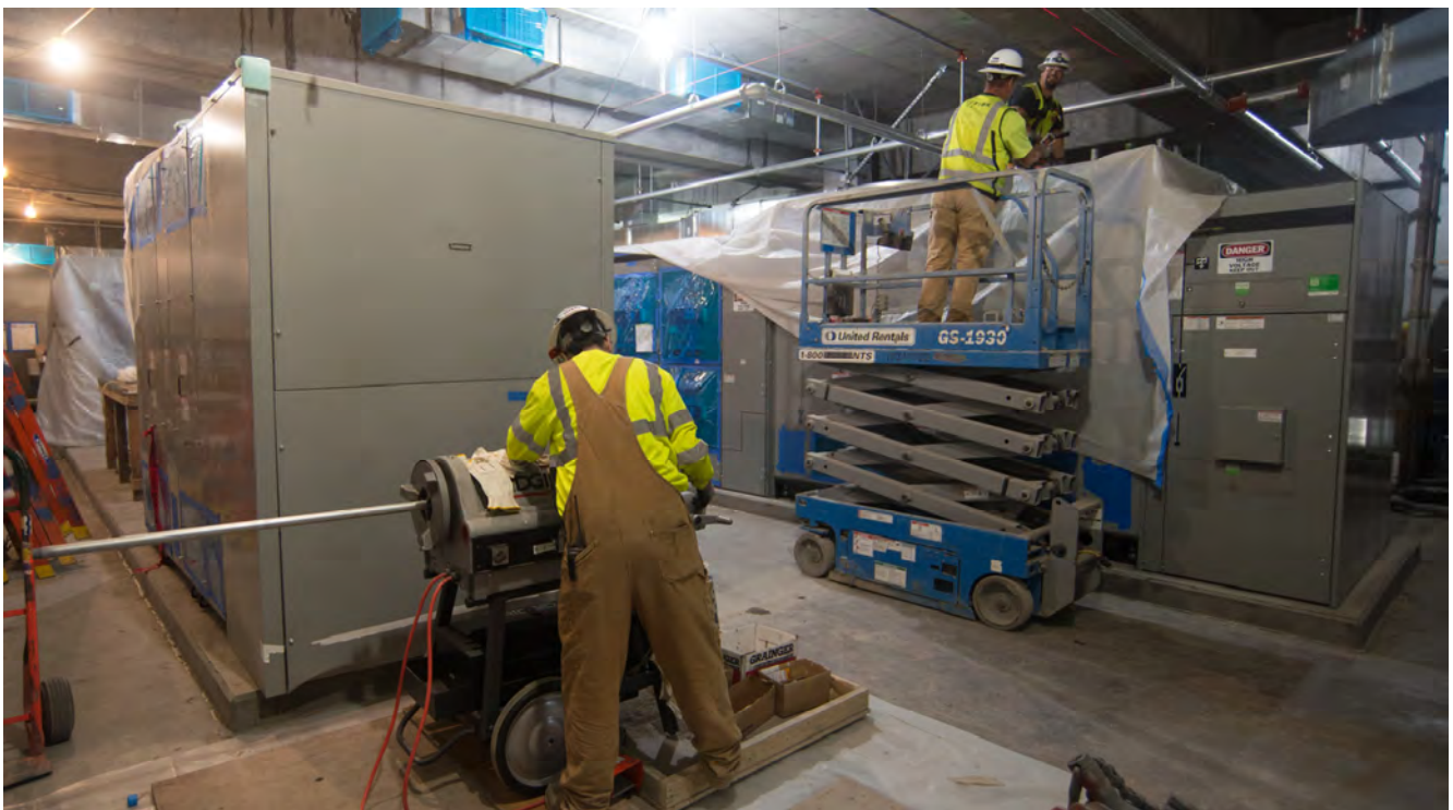
A worker operates a conduit threading machine while associates install lengths of conduits nearby, inside the Chinatown Station headhouse.
