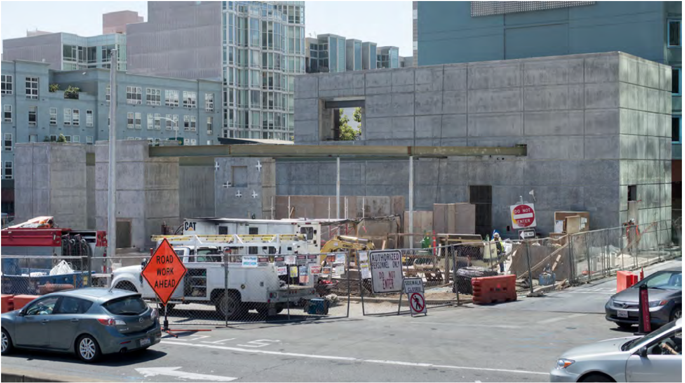
Steel framing for the Yerba Buena/Moscone Station entrance structure has been installed, as seen from across 4th Street at Clementina.
