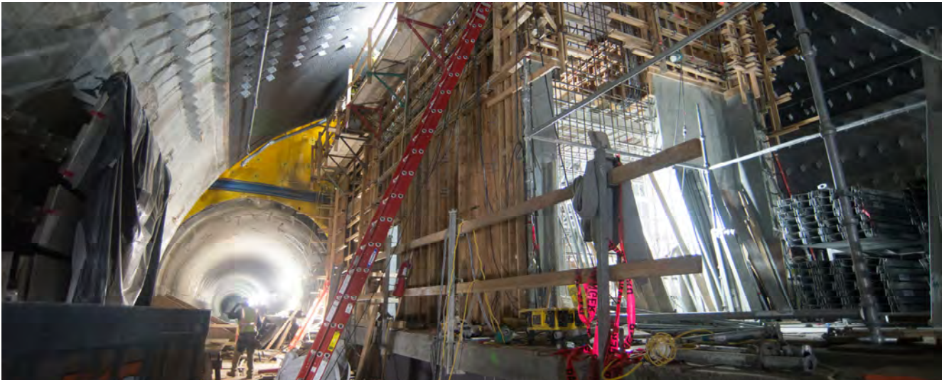
Formwork has been installed to build reinforced concrete walls for a stairwell at the north end of the Chinatown Station platform.
