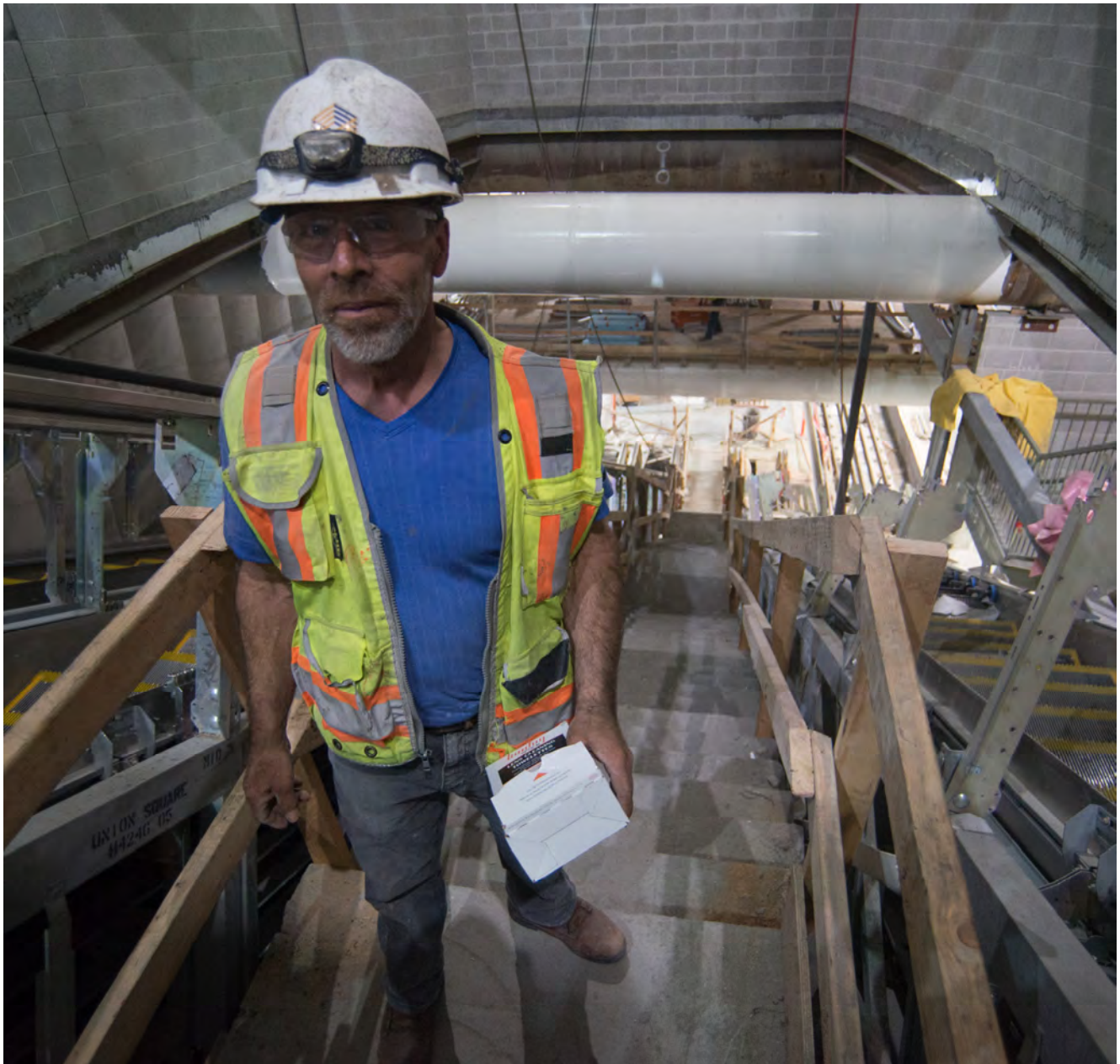
A worker pauses along the south stairs leading to the station platform from the concourse level. Three escalators are being installed adjacent to this staircase.
