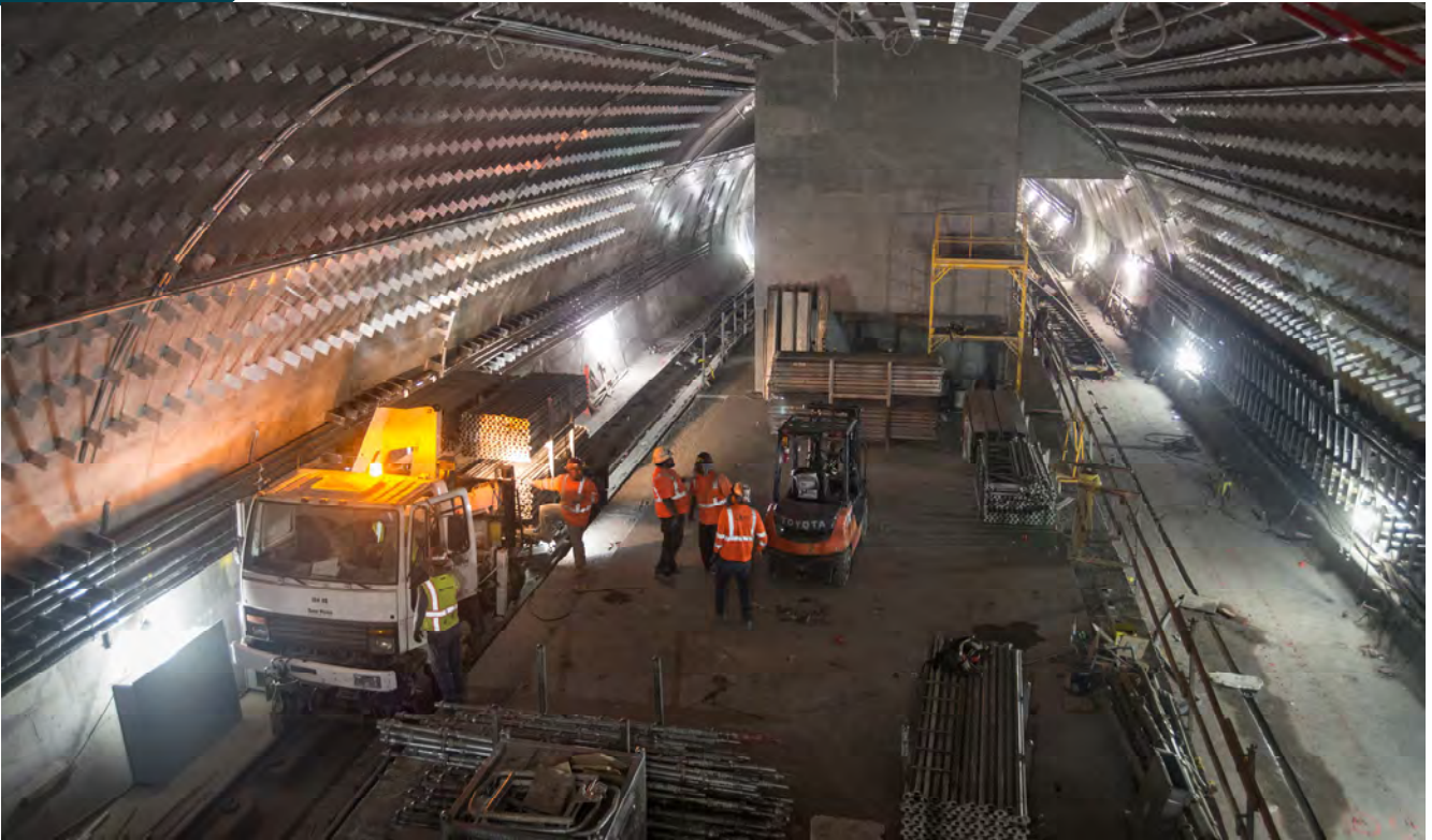
Looking south, a yellow light flashes on a utility vehicle preparing to ferry scaffolding materials out of the Chinatown station cavern.
