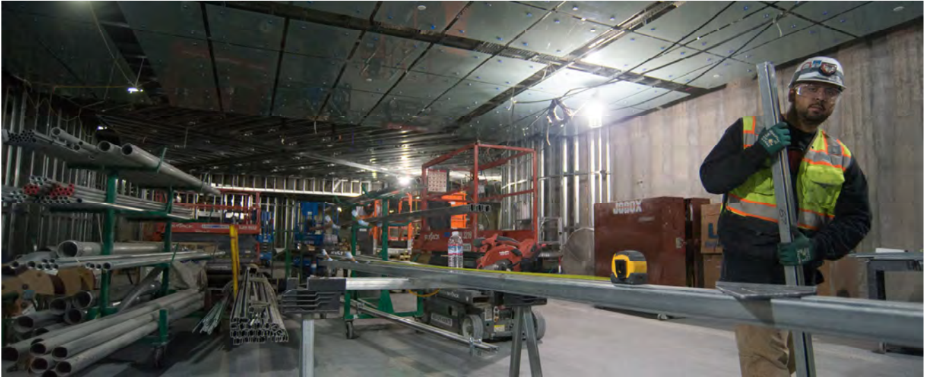
A partially-completed ceiling panel array can now be seen above a worker carrying a piece of steel framing used as part of interior construction inside the south concourse for Union Square/Market Street Station.
