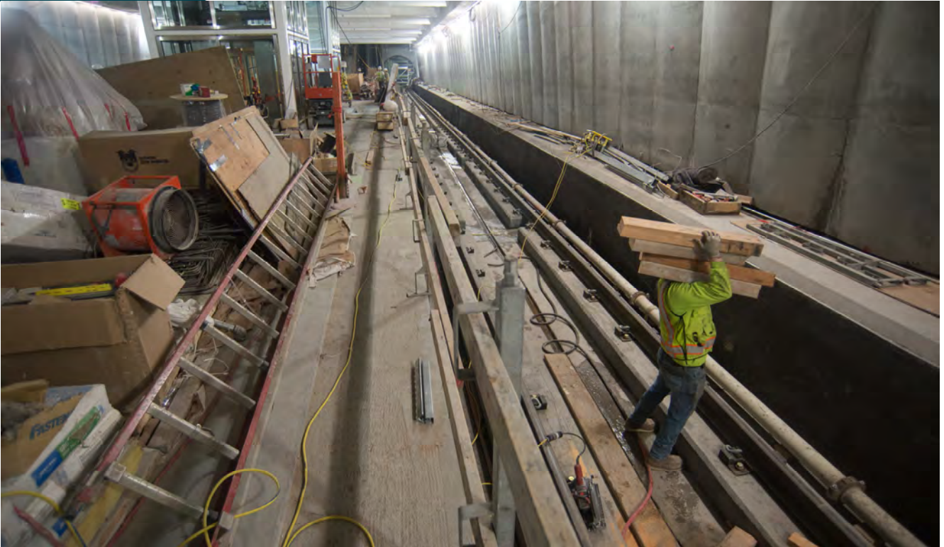
A worker loads up pieces of cribbing used alongside the southbound track adjacent to the Union Square/Market Street Station platform.
