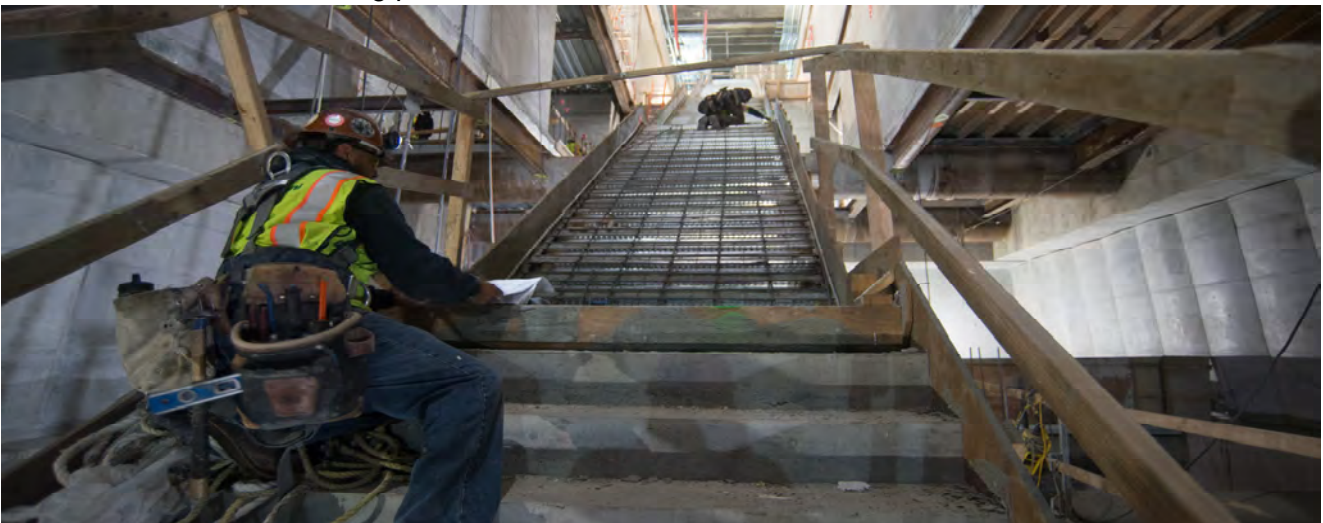
Rebar and formwork are installed to continue building the north staircase leading to and from the concourse level and Union Square/Market Street Station platform.
