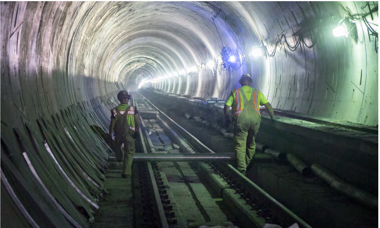
Two workers inside the southbound tunnel between Union Square/Market Street Station and Chinatown Station roll a section of pipe up to be placed as part of utility work inside the tunnel.
