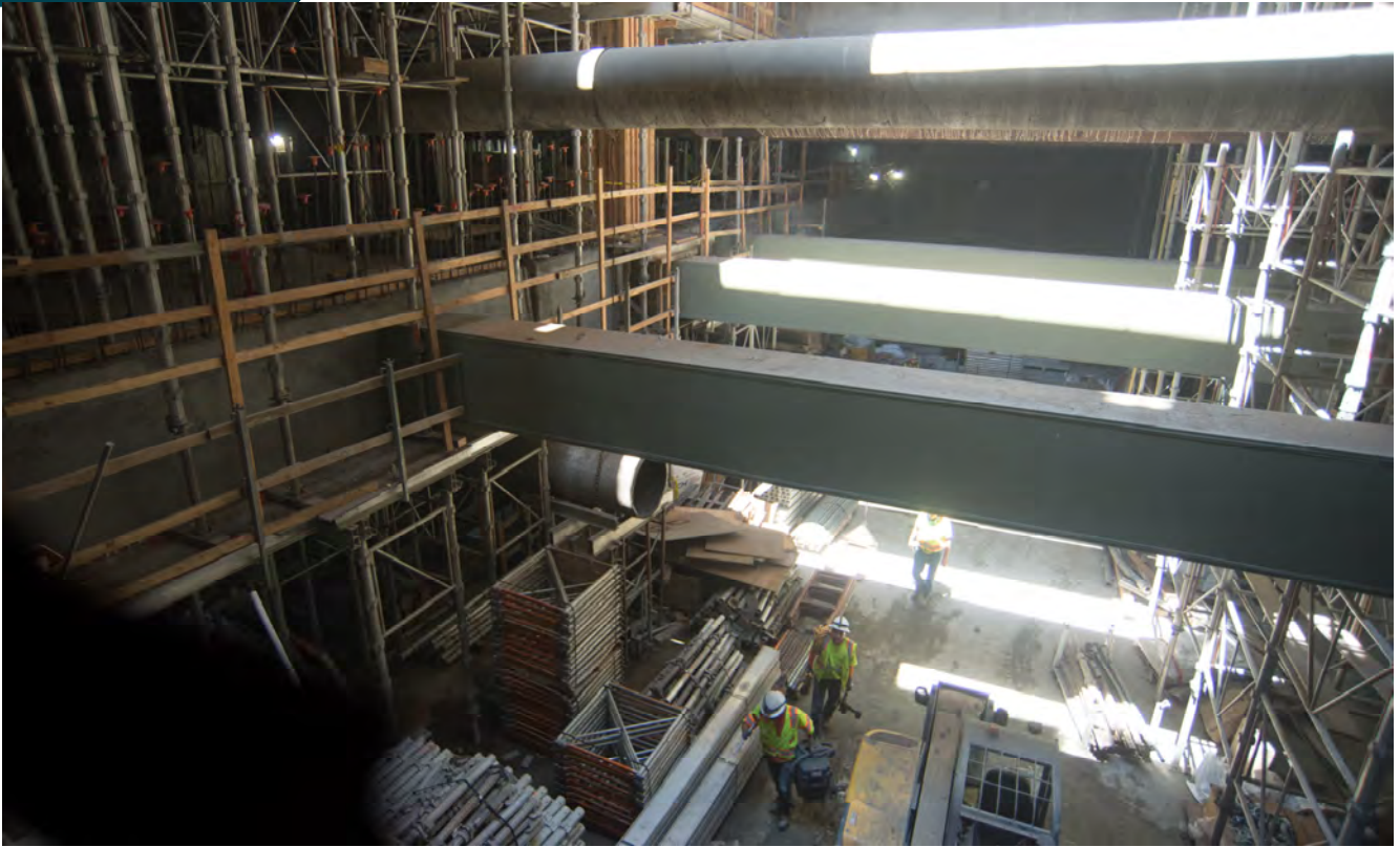
Workers head for the crew elevator toward the end of their shift, looking north inside the Chinatown Station headhouse.
