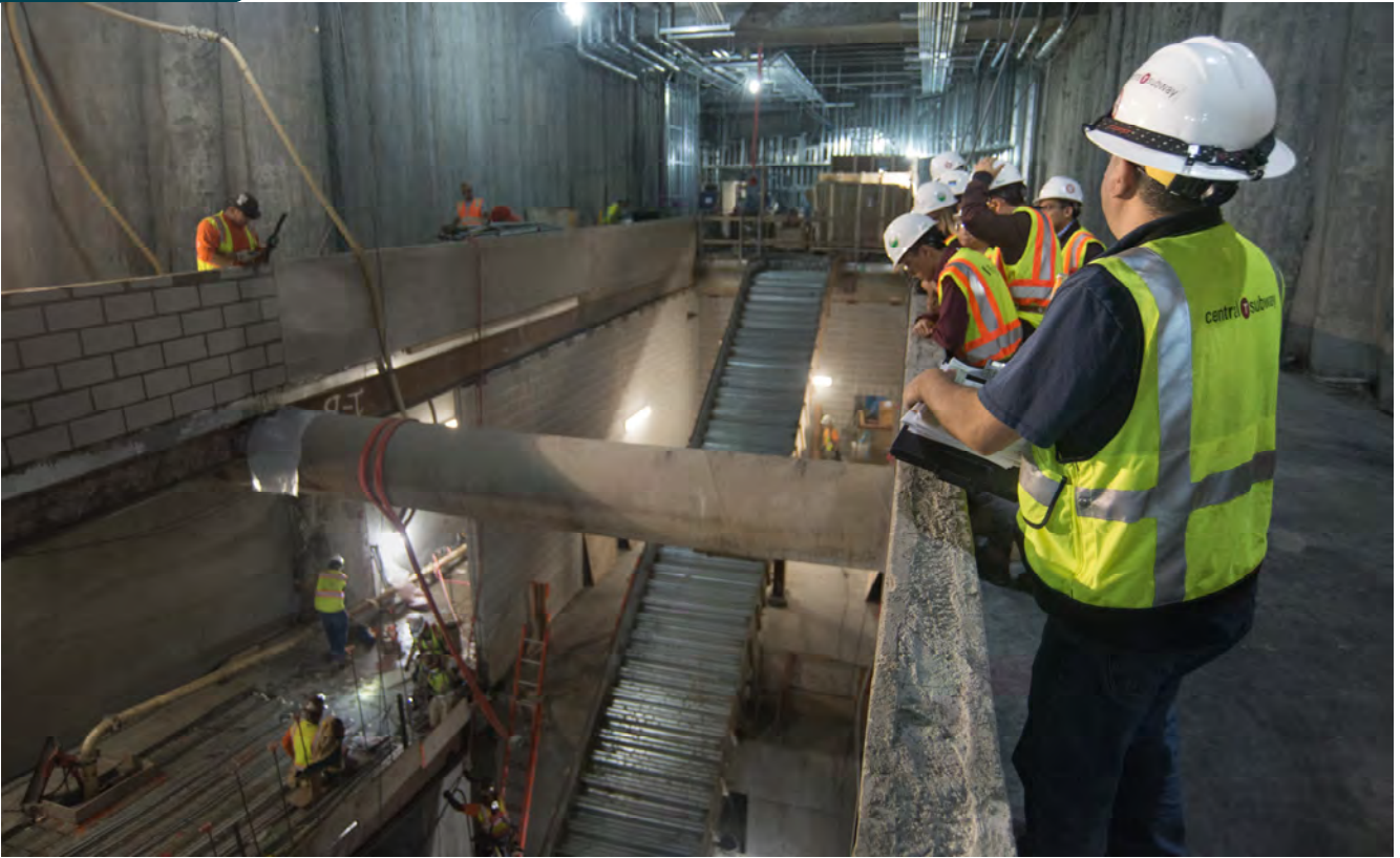
Engineers look over work at the north end of the Union Square/Market Street Station concourse, where interior walls and the concourse-to-platform staircase are being built.
