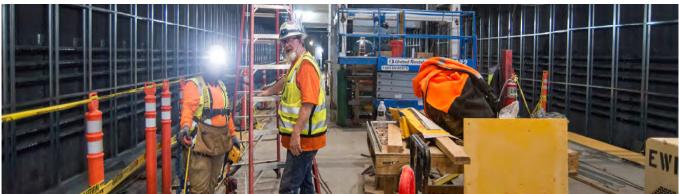
Crews continue fitting steel brackets for glass elevator panels, as well as other interior elements on the platform level of Yerba Buena/Moscone Station.
