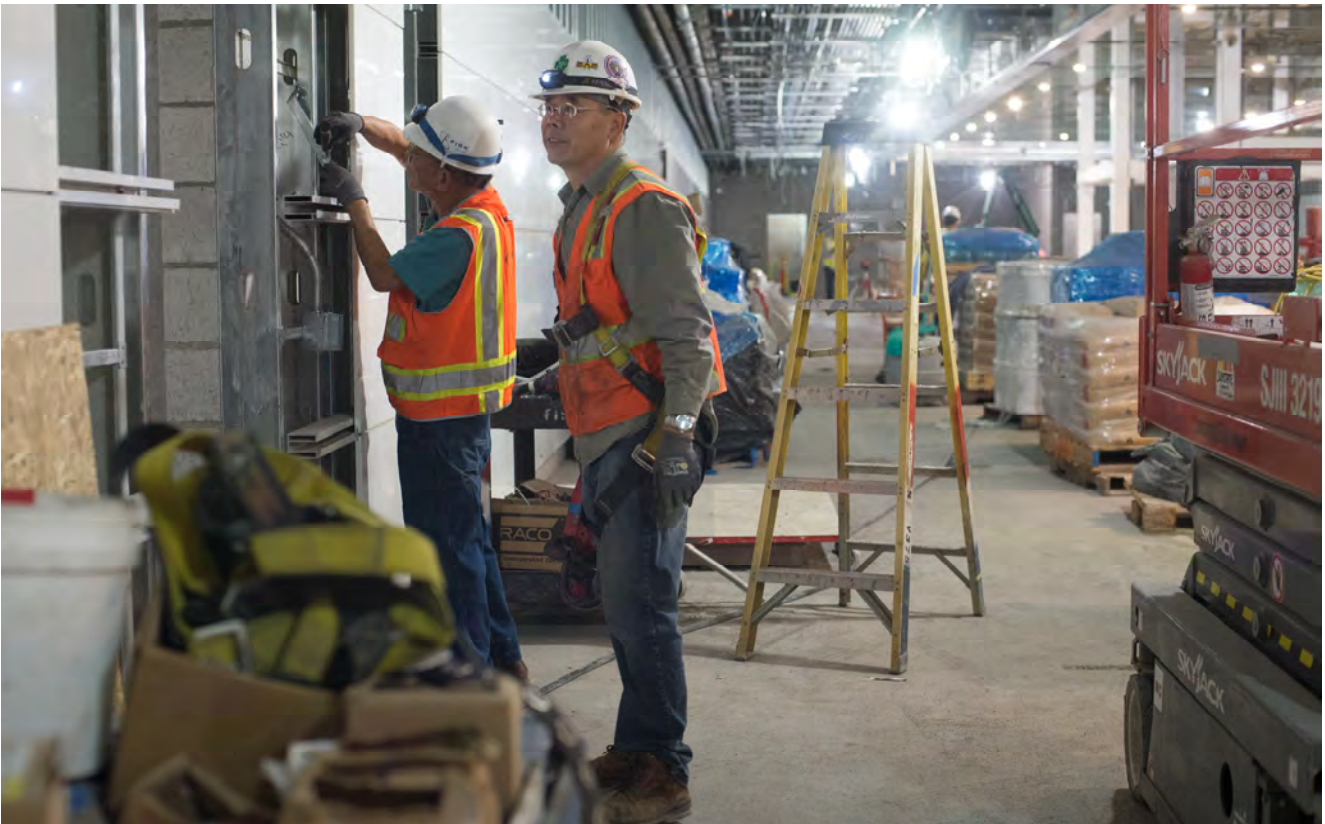
Brackets and conduits are installed on the west side of the Yerba Buena/Moscone Station's concourse level.
