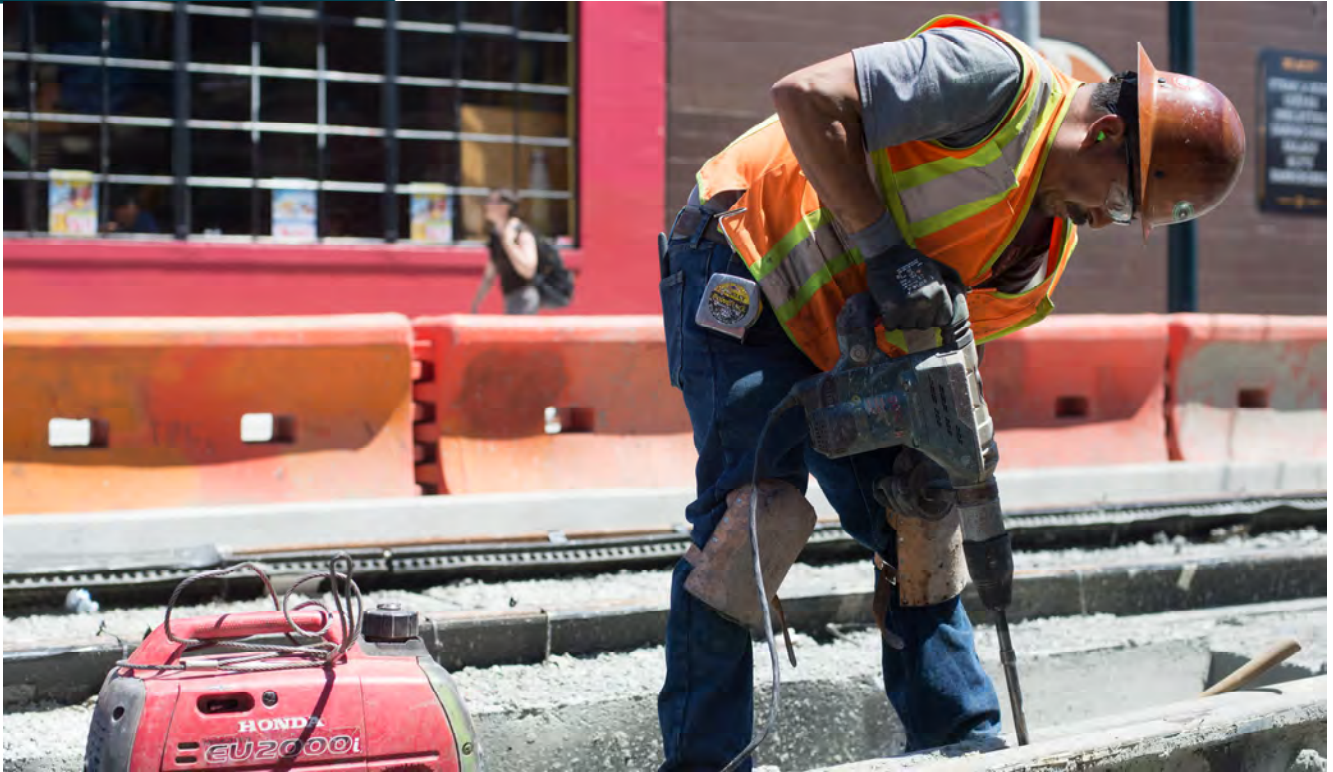
A worker uses an electric jackhammer to remove excess material from between rails at a crossover switch near 4th and Bluxome.
