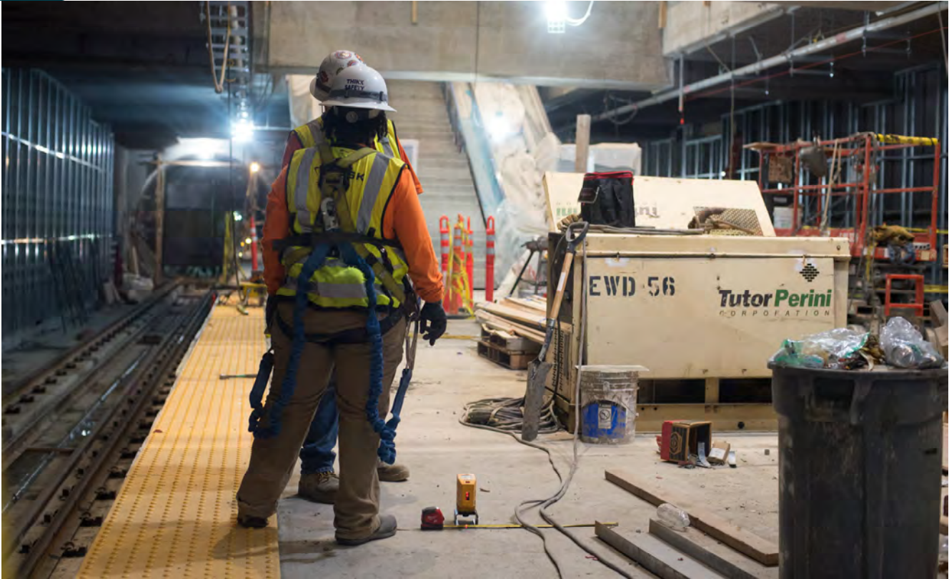
Workers stand by recently-installed hazard warning/tactile paving tiles along the north-bound track side of Yerba Buena/Moscone Station.
