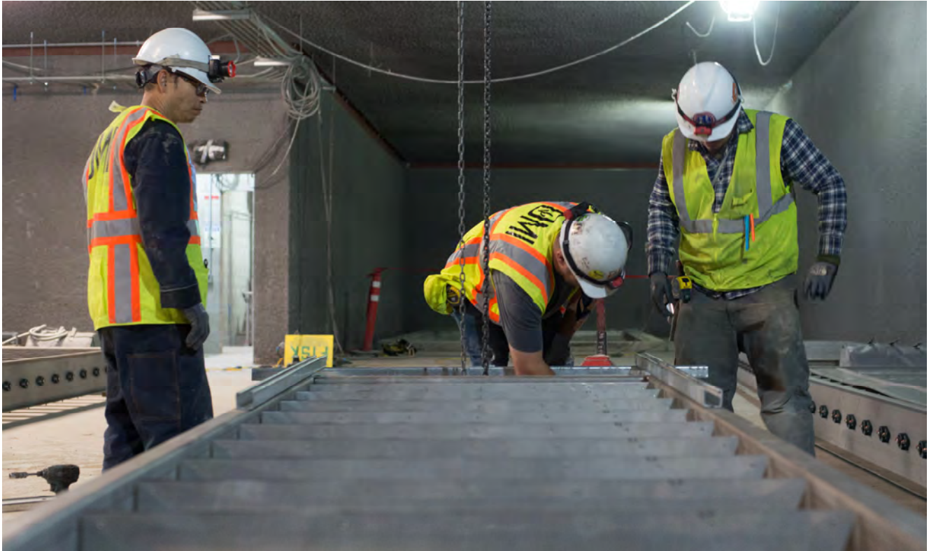
Dampers for the high-volume ventilation and tunnel exhaust system are being assembled on the mezzanine level of the Yerba Buena/Moscone Station box.
