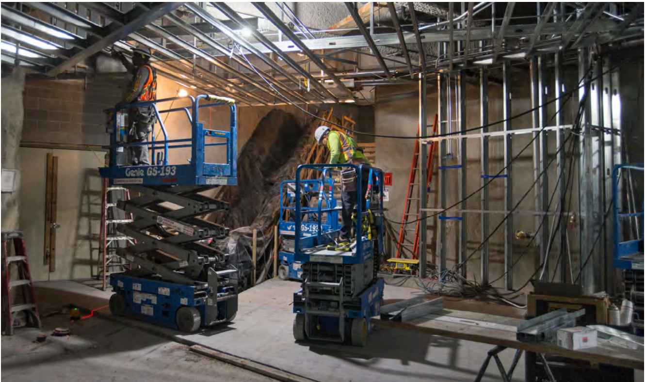
Steel framing for walls and ceiling panels is being added to the south concourse for Union Square/Market Street Station.
