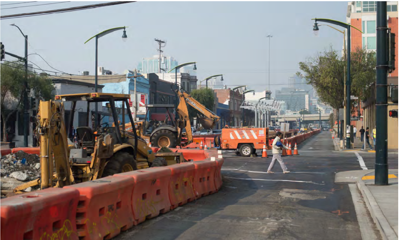
Just south of the 4th and Brannan surface station platform, utility upgrade and installation work is underway in SoMa.
