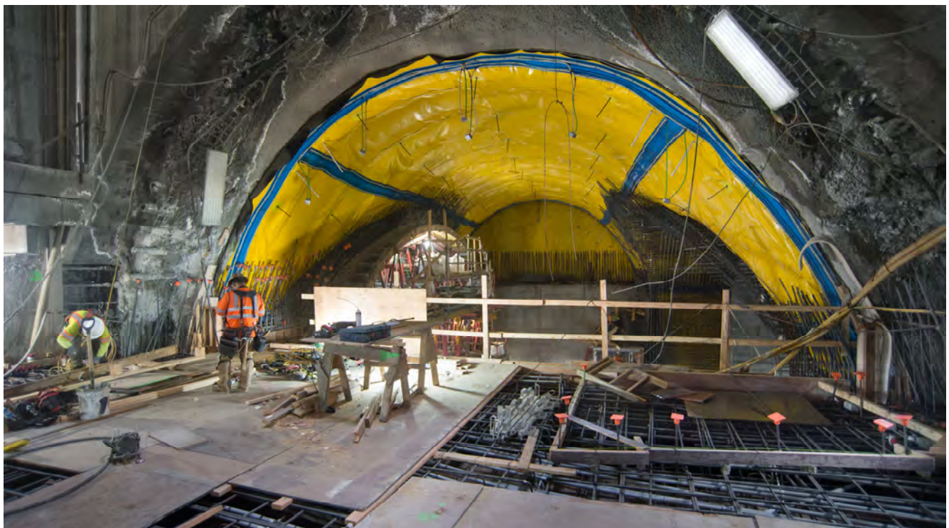
Rebar and utility conduit installation work continues to build the last section of concourse-level floor slab inside the Chinatown Station headhouse, where future passengers will enter and exit through fare gates under the cross-cut cavern archway.
