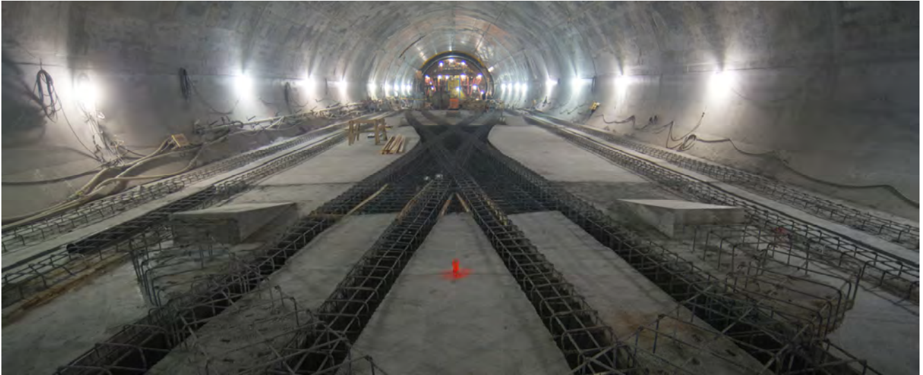
Steel reinforcing for future track foundations marks the X-shaped crossover inside the Chinatown Station track crossover cavern.
