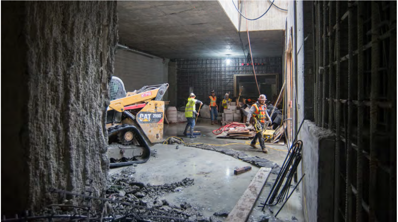
Crewmembers pass through an area on the mezzanine level of the Yerba Buena/Moscone Station headhouse where demolition work is underway to create an opening in the west slurry wall, allowing for a future ventilation structure.
