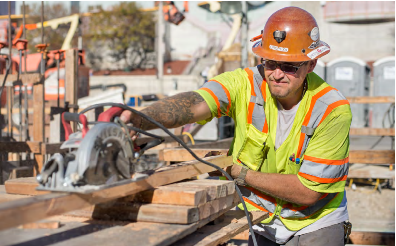
A carpenter rips a 2x4 at the surface level of the Yerba Buena/Moscone Station head-house, to be used as part of concrete forms.
