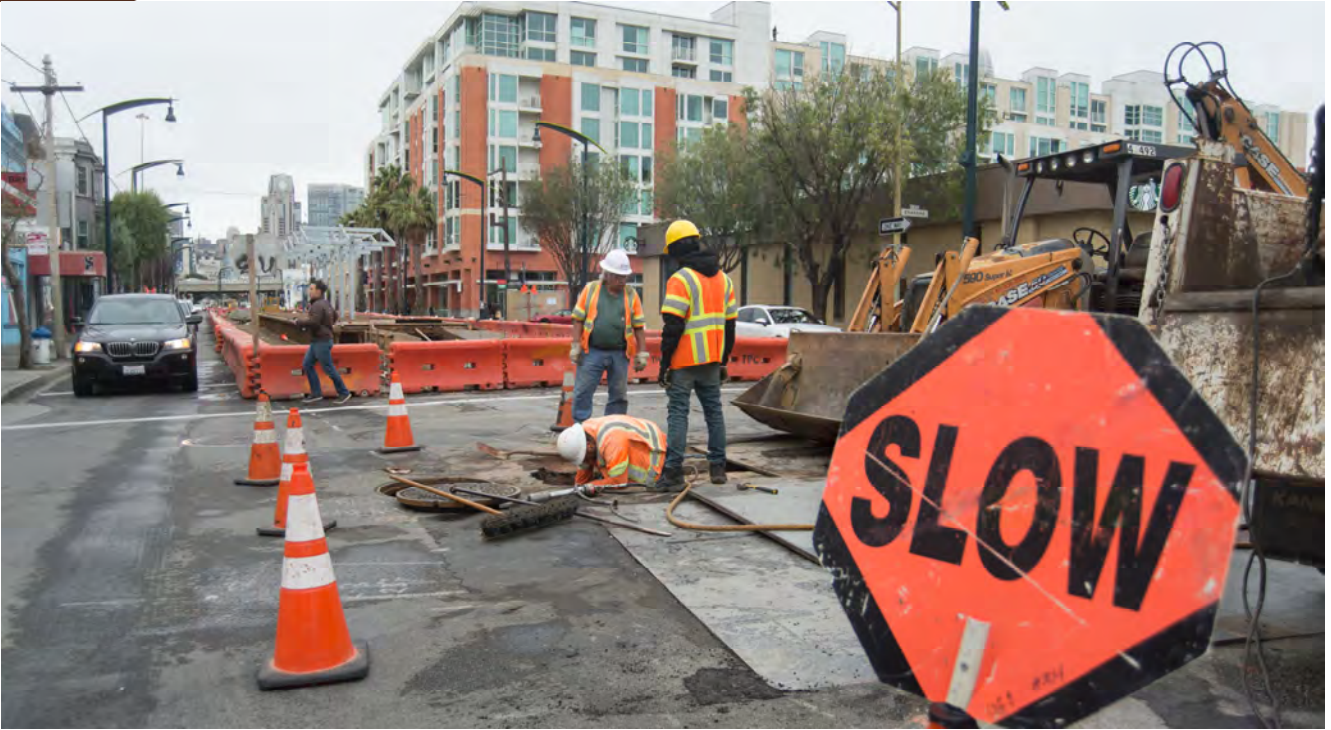
Trenching work has begun to upgrade water lines at the 4th and Brannan Intersection, ahead of roadway restoration work there.
