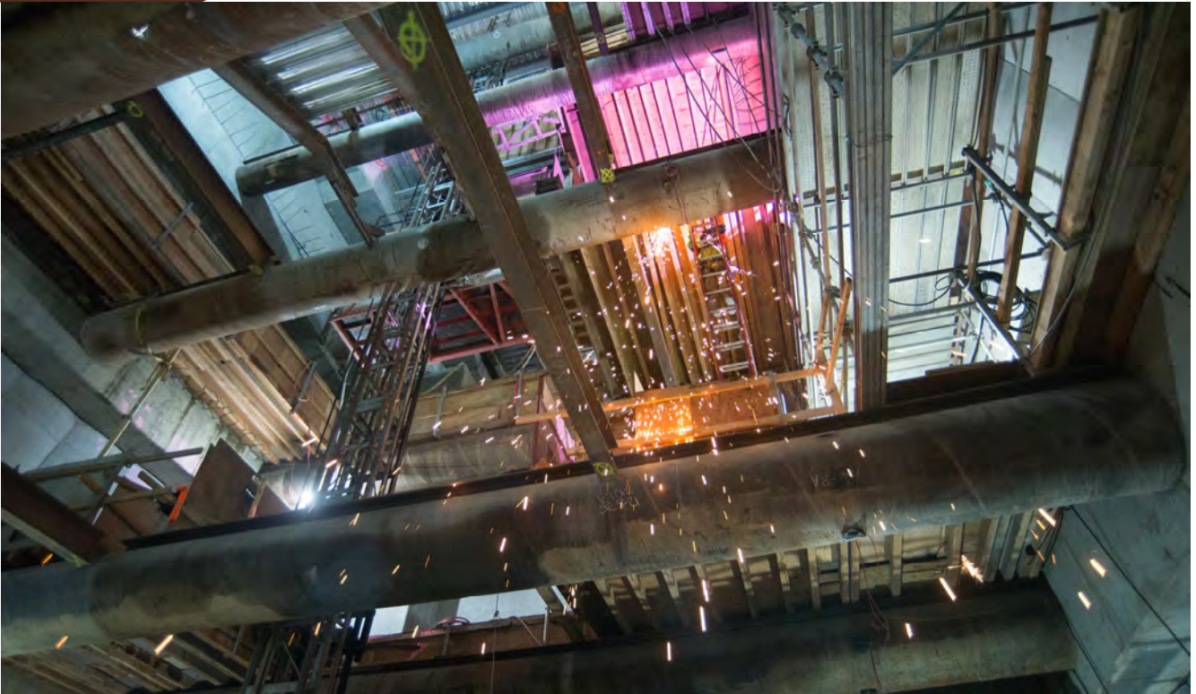
A shower of sparks falls from work to remove temporary shoring and install new sections of floor deck at the north end of the Union Square/Market Street station box.
