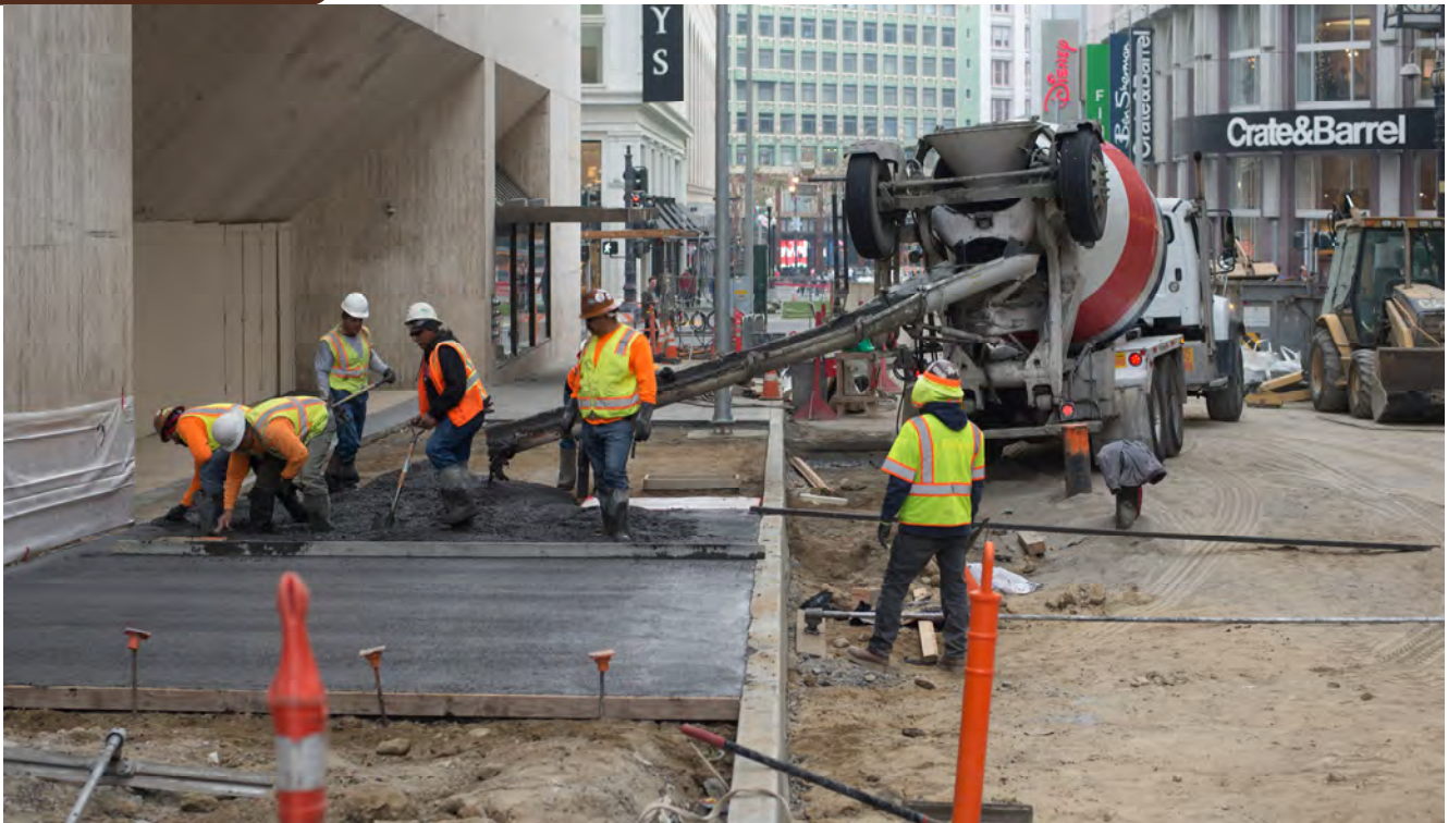
A new section of sidewalk begins to take shape during a concrete pour as part of sidewalk and roadway restoration work along the east side of Stockton north of O'Farrell.
