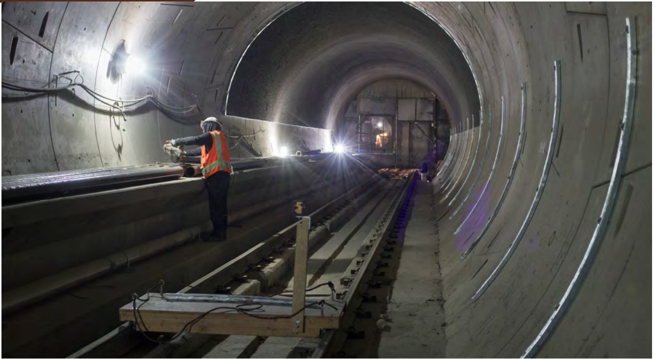
In the southbound tunnel just north of the Yerba Buena/Moscone Station platform, a worker fashions sections of pipe to be installed as utility conduits in the twin tunnels.
