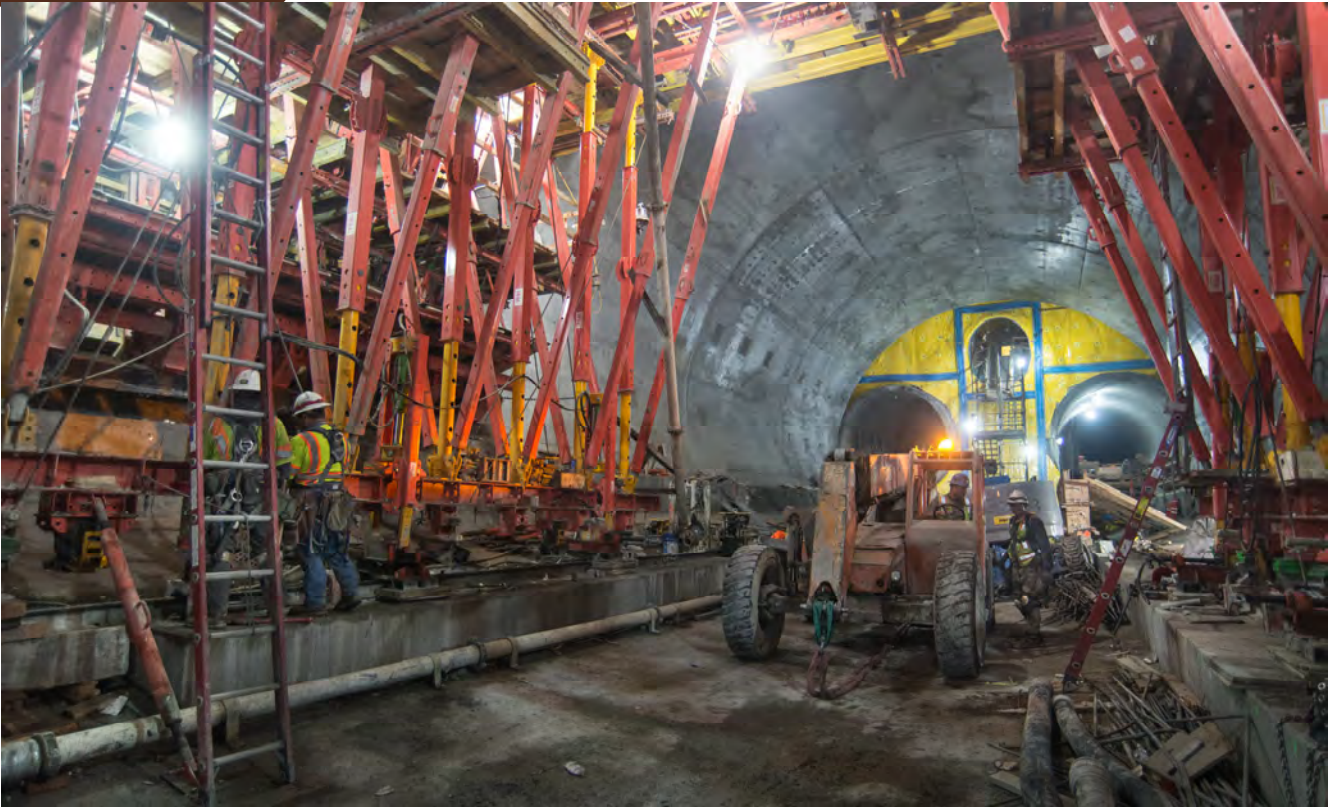
A Skytrak forklift rolls slowly underneath the large red truss structure used to place concrete forms inside the Chinatown Station platform cavern.
