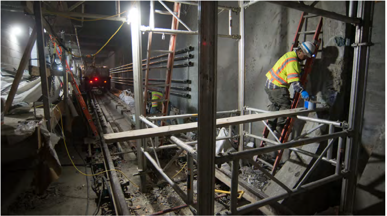
Workers patch concrete at the circular tunnel opening where the southbound track meets the Yerba Buena/Moscone Station platform.
