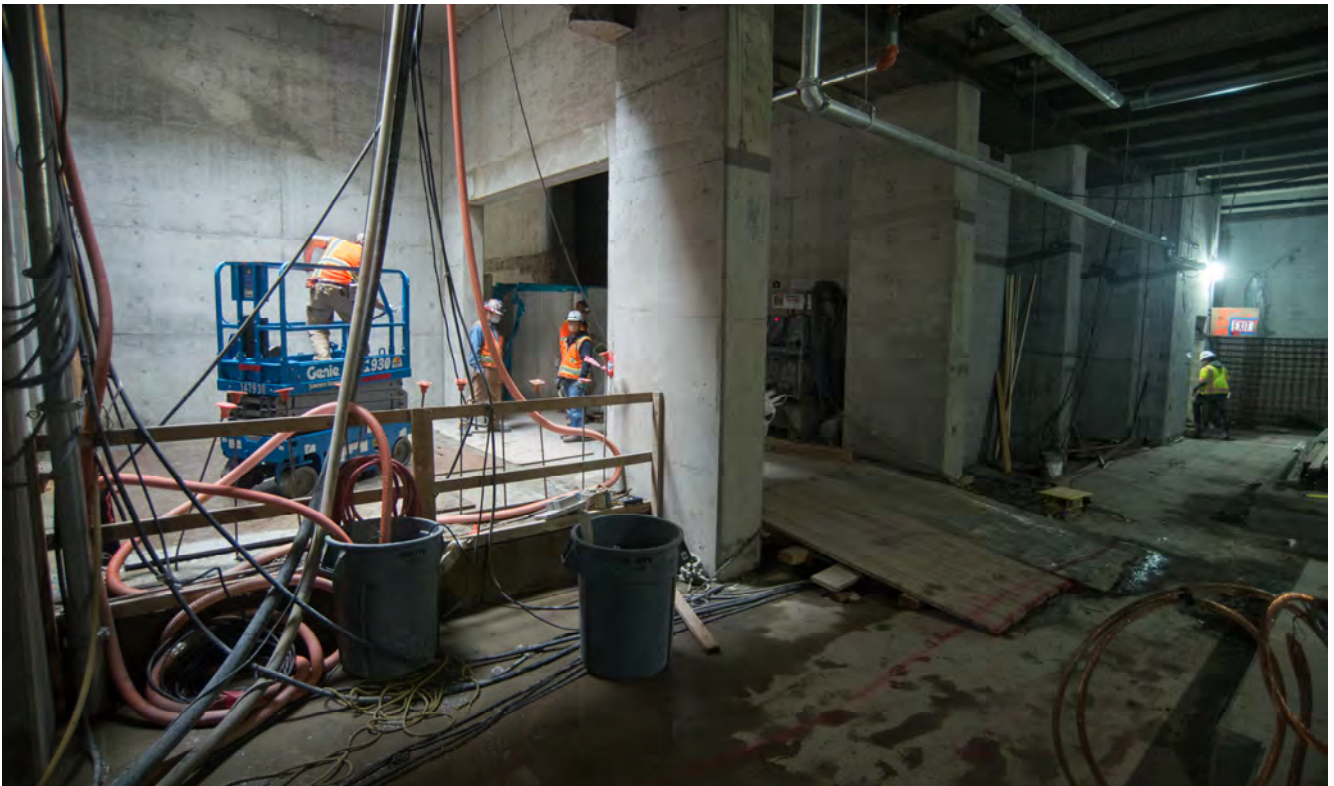
A crew positions a scissor lift at the bottom of the access shaft adjacent to the Union Square Garage, inside the north concourse of the Union Square/Market Street Station.
