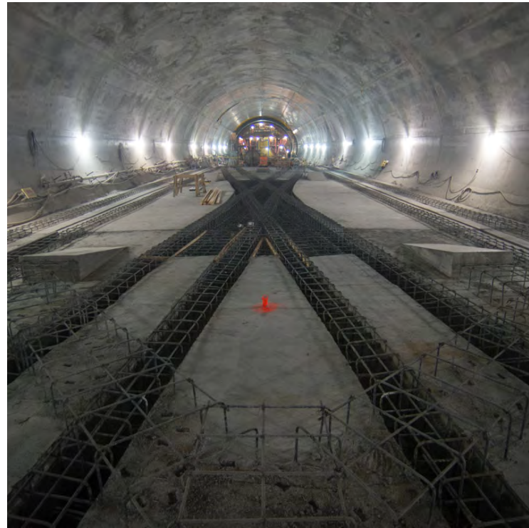
3 Once track installation reaches the track crossover cavern it will switch over to the southbound tunnel.
