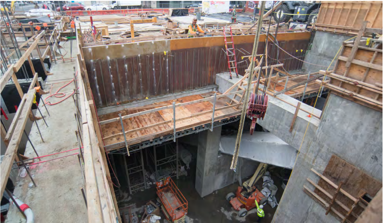
Temporary scaffolding has been built to aid access for building concrete forms toward construction of the future station entrance structure at the surface of 4th Street.
