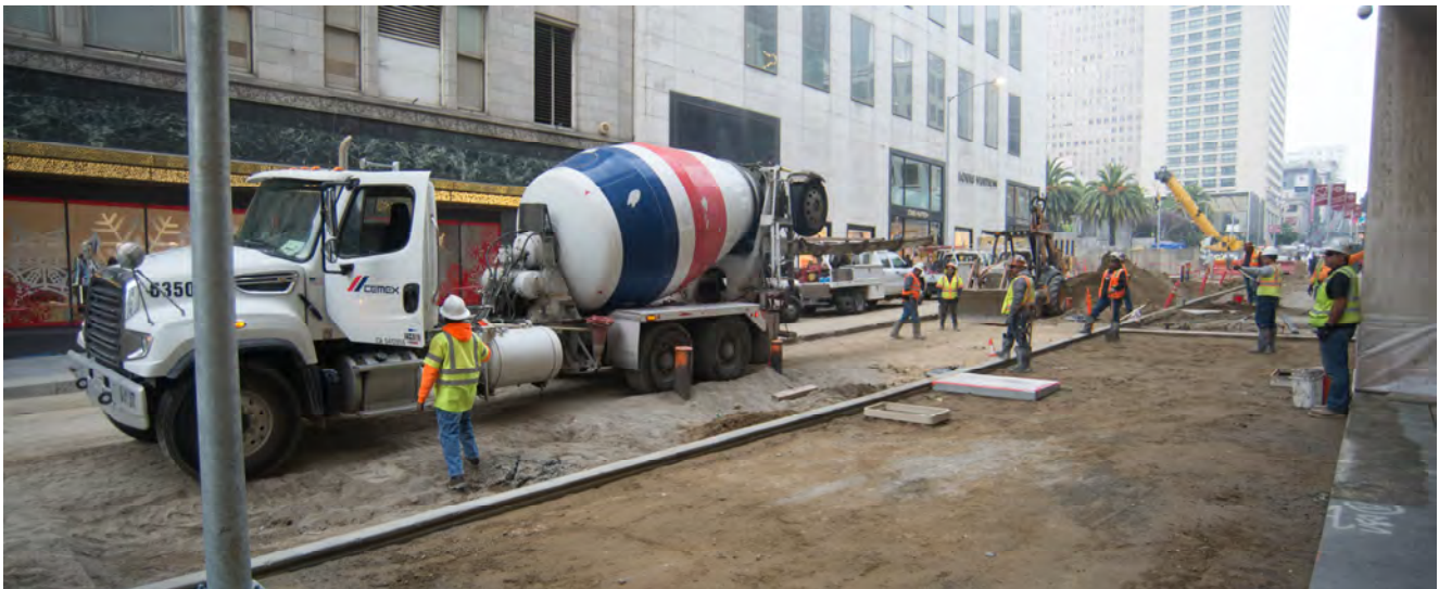
A concrete truck is positioned adjacent to a large area where concrete will be poured to rebuild a large section of sidewalk along the east side of Stockton south of Geary.
