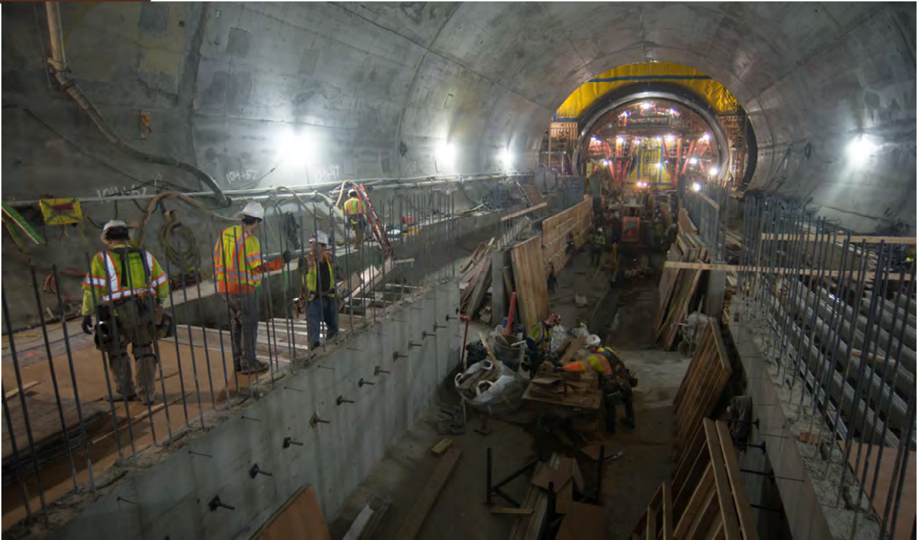
Workers inside the Chinatown Station platform cavern have been building support walls for the future platform level floor slab.
