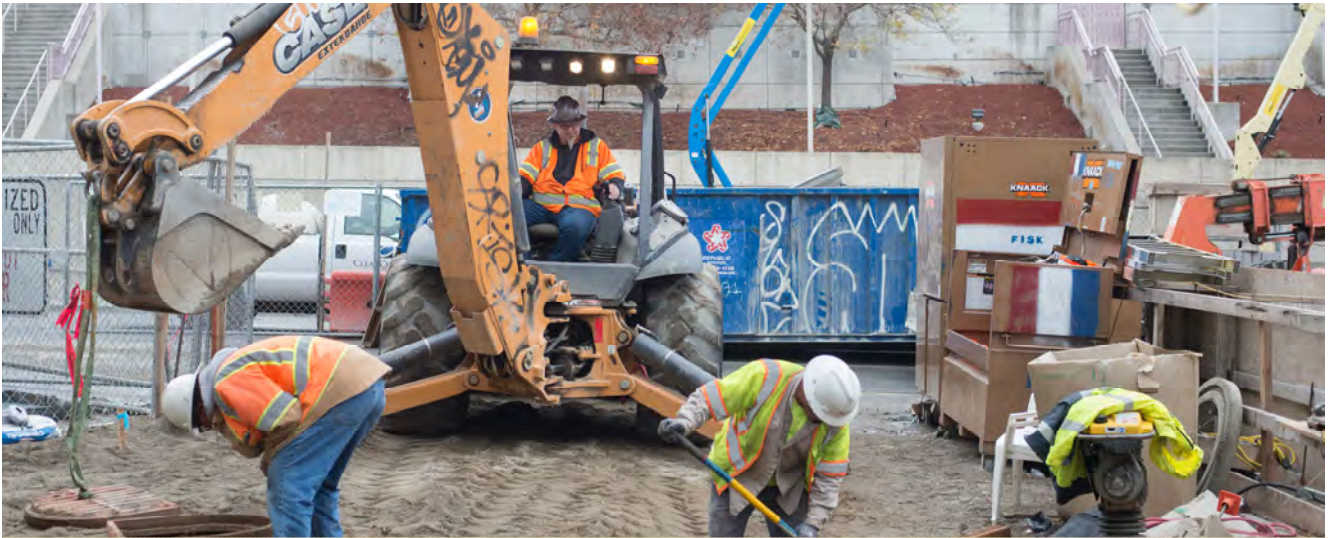
A crew removes materials from the soil as part of regrading work where Clementina Alley approaches 4th Street, adjacent to the YBM headhouse.
