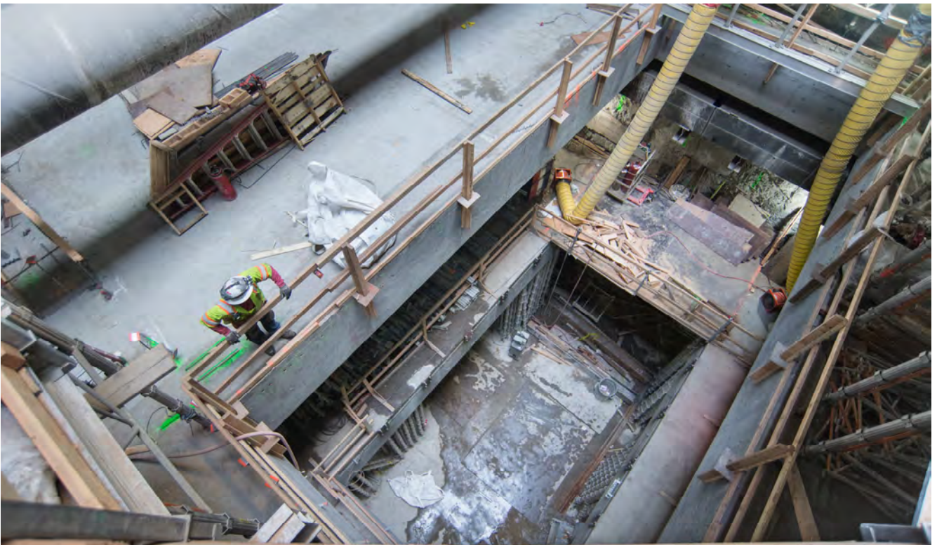
A worker on the concourse level floor slab looks across an access shaft on the east side of the Chinatown Station headhouse.
