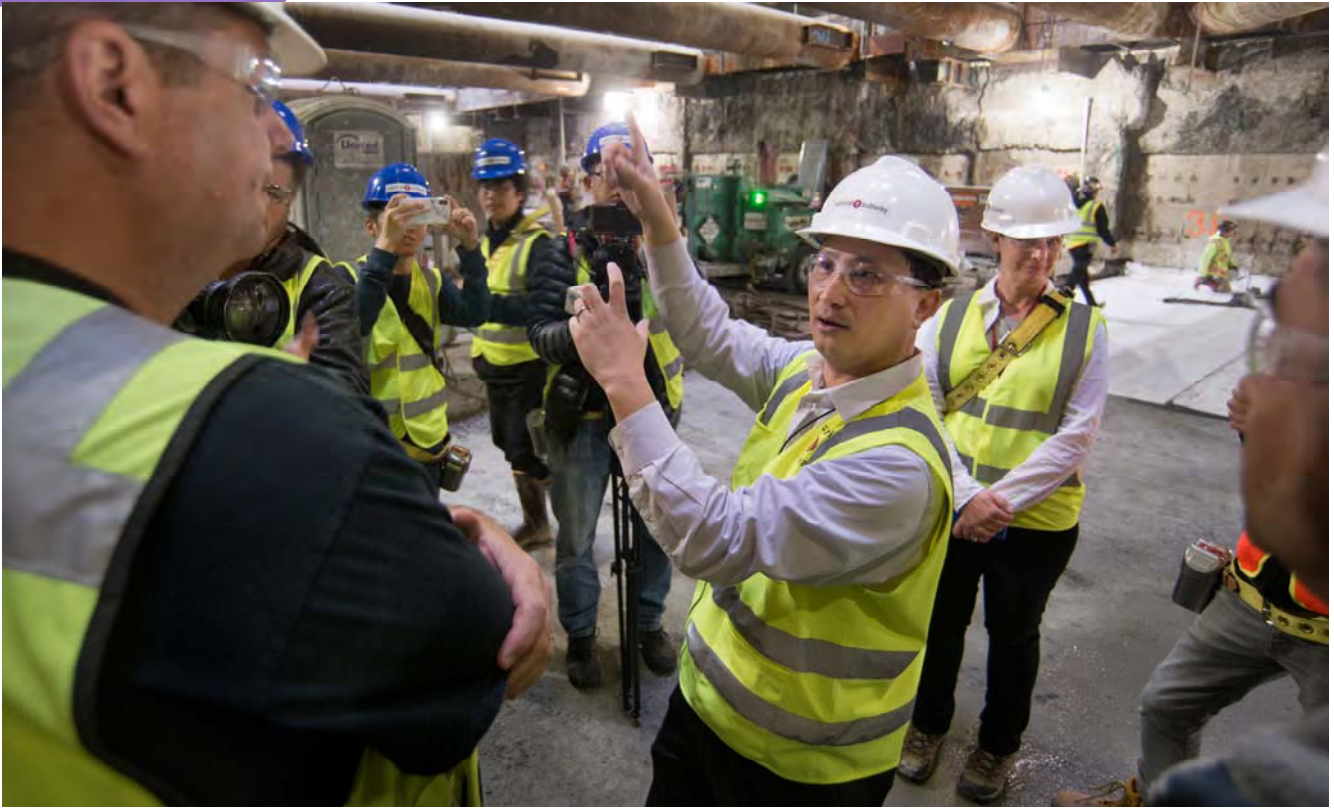
Central Subway Program Director Albert Hoe gives Mayor Mark Ferrell an overview of Chinatown Station construction at the bottom of the headhouse.
