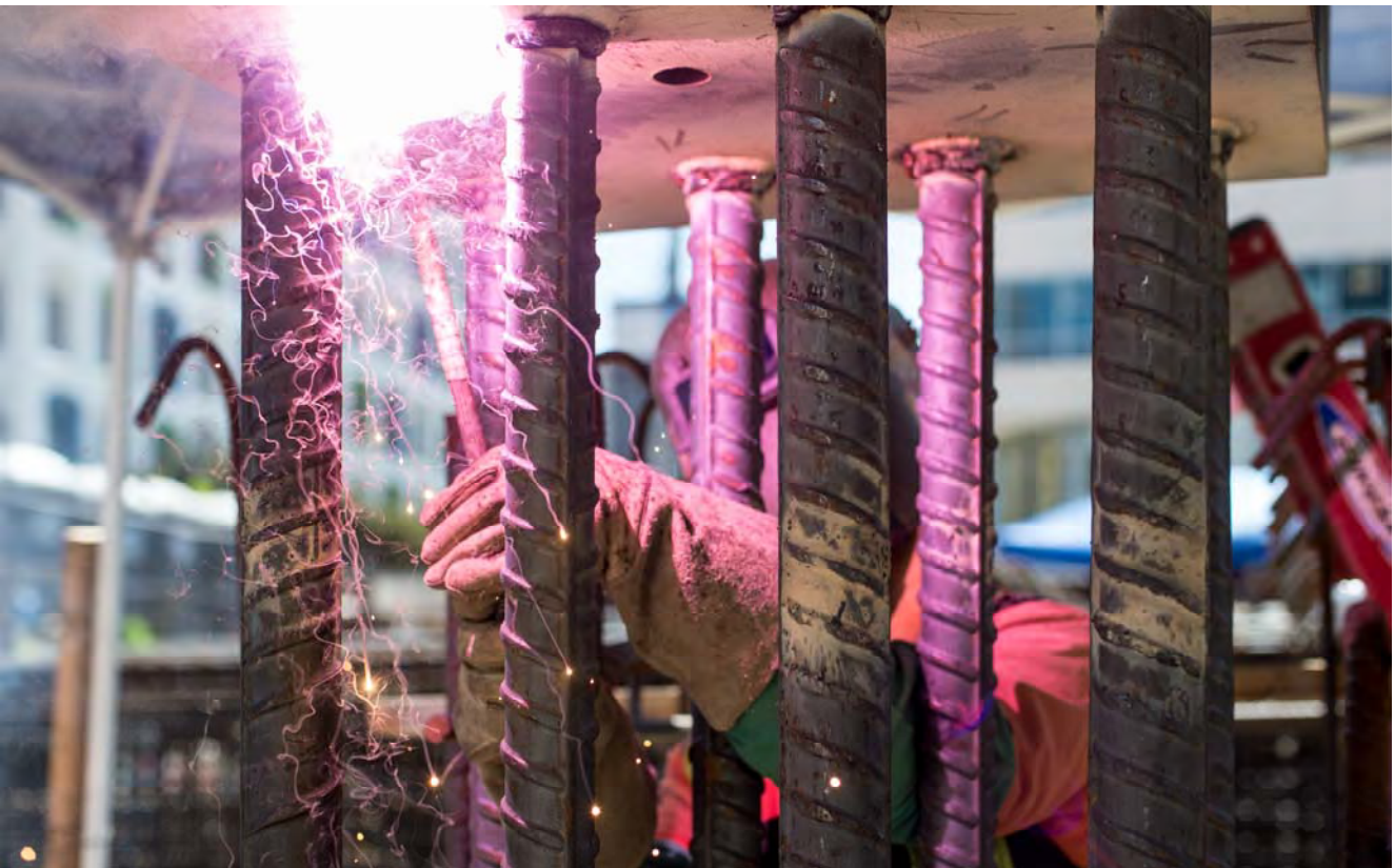
A welder attaches a steel plate to the top of large gauge rebar intended to be used as part of a future transit-oriented development atop the south end of the Yerba Buena/Moscone Station headhouse structure.
