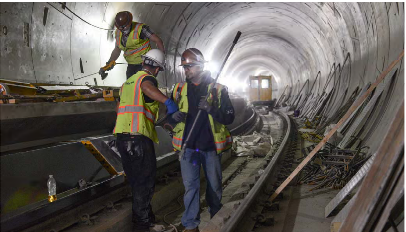
Workers inside the northbound tunnel just before the Market Street S-curve prepare steel concrete forms for re-use further north.
