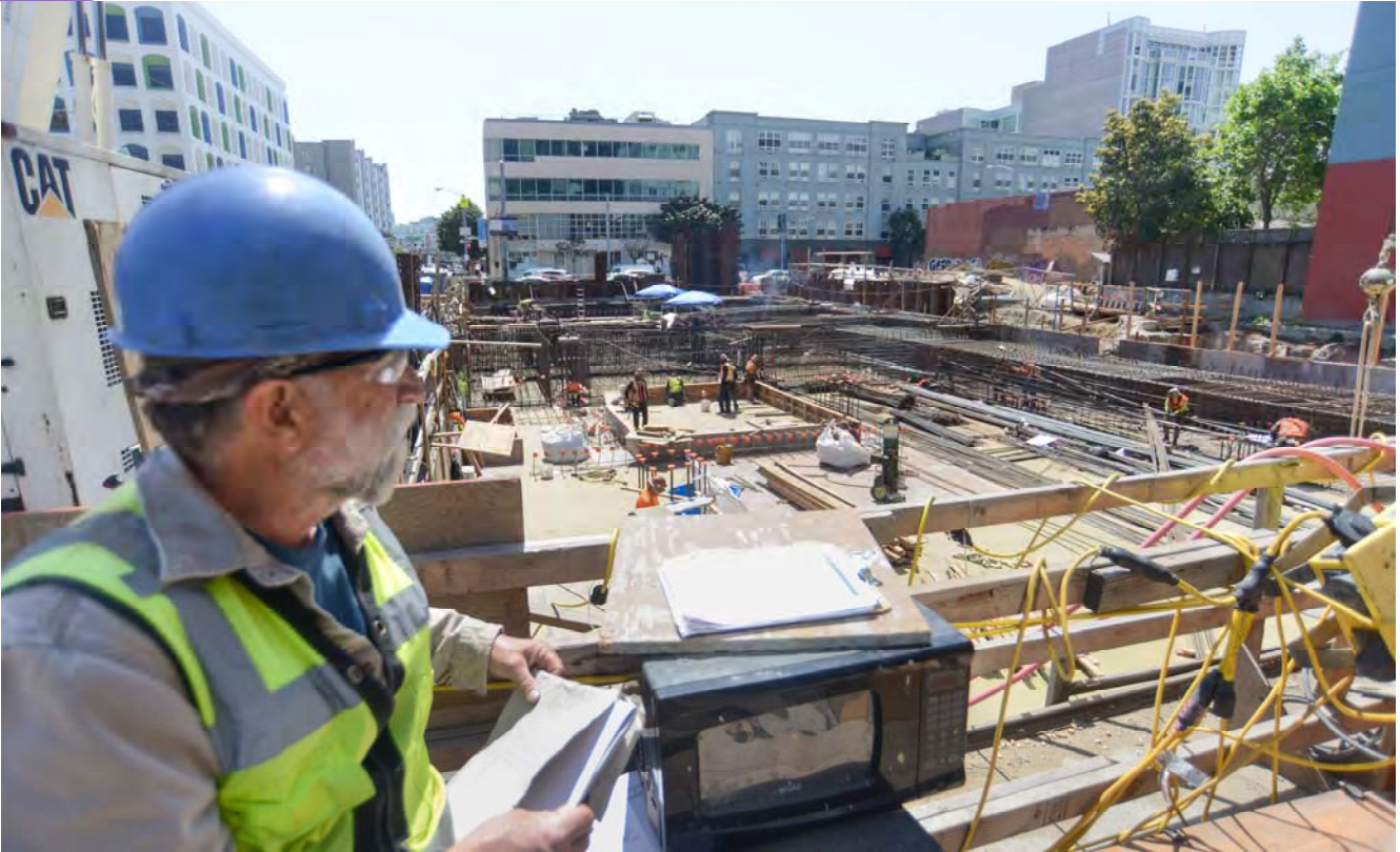
A supervisor reviews rebar installation documents as workers atop formwork inside the Yerba Buena/Moscone Station headhouse build massive rebar cages which will become part of the reinforced concrete roof slab.
