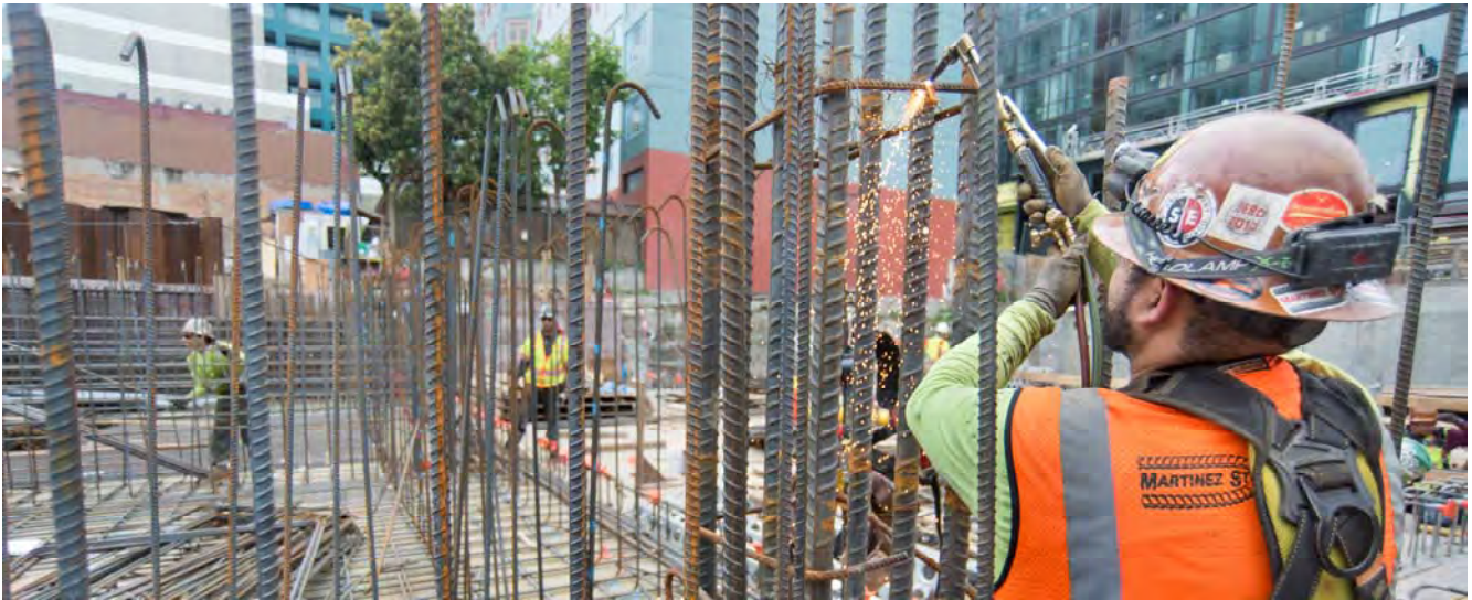
Small pieces of connecting rebar used during transport are cut and removed as large gauge strands are put into place for future headhouse roof reinforcing.
