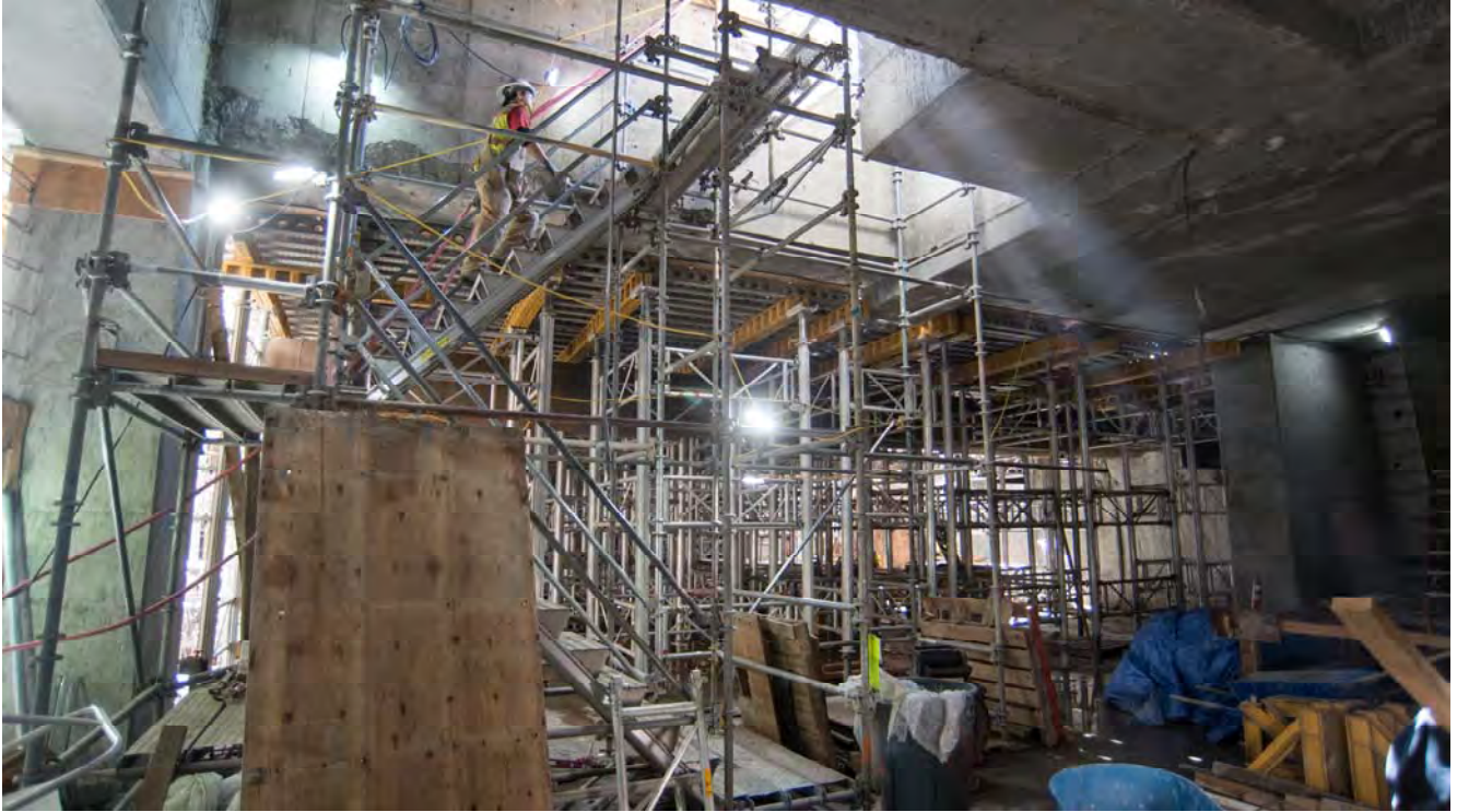
A complex scheme of scaffolding and concrete forms are being installed inside the Yerba Buena/Moscone Station headhouse, where roof slab construction has begun.
