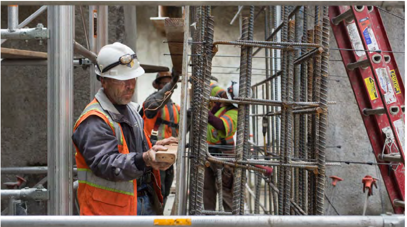
A crew on the mezzanine level of the headhouse assembles concrete forms adjacent to a rebar cage, which will eventually become an internal support wall.
