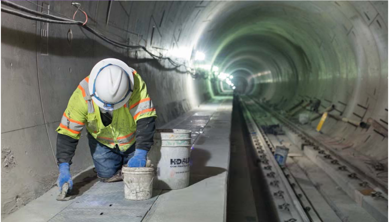
Workers are following up to smooth everything out following the installation of new sections of track walkway inside the southbound tunnel.
