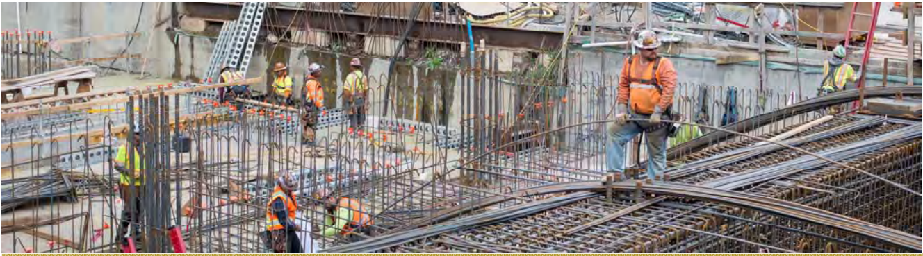
Men pass long strands of rebar to each other during construction of the massive rebar cages for the Yerba Buena/Moscone Station headhouse roof.
