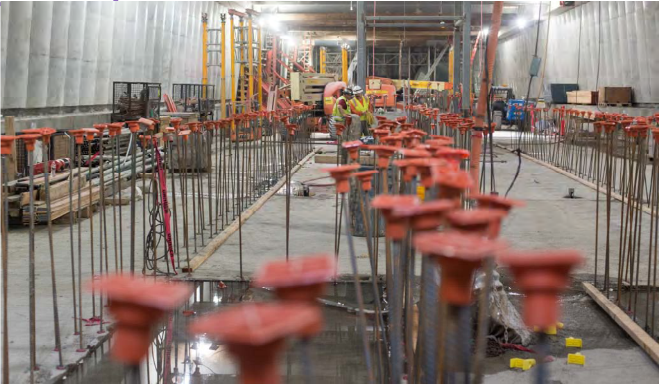
A forest of capped rebar strands are going in as part of initial work to construct the Union Square/Market Street Station platform.
