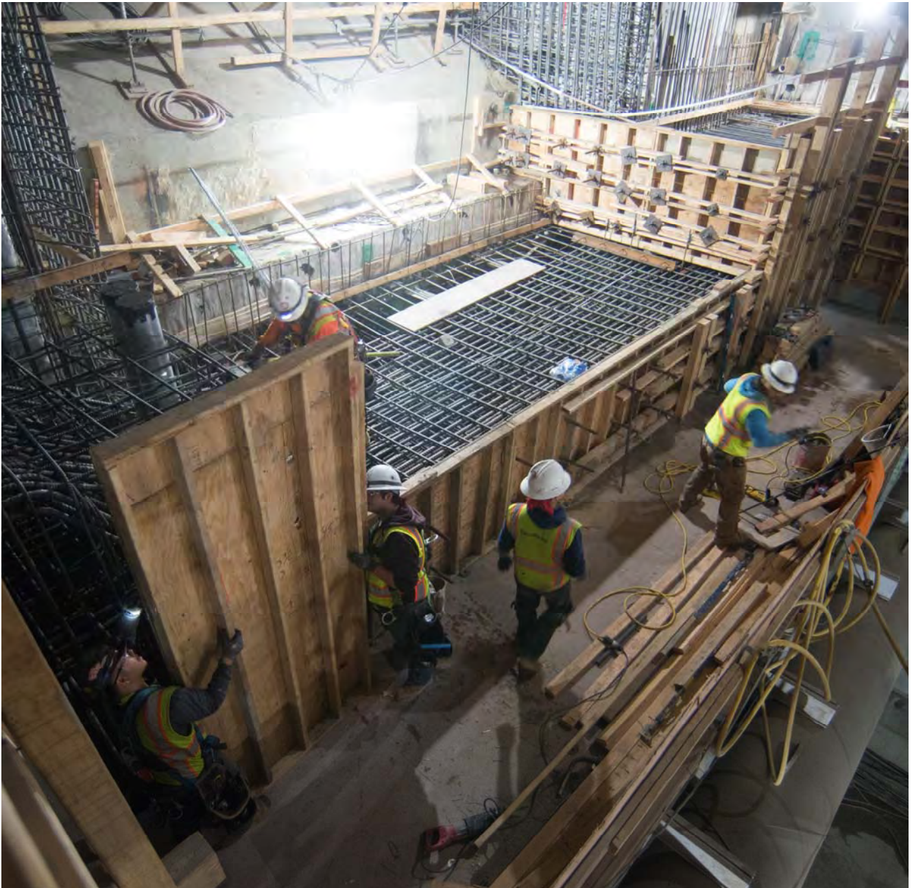
Concrete forms are assembled surrounding massive rebar cages at the Union Square/Market Street station box's south headwall, to construct a shelf which will act as a mid-way footing for stairs and escalators.
