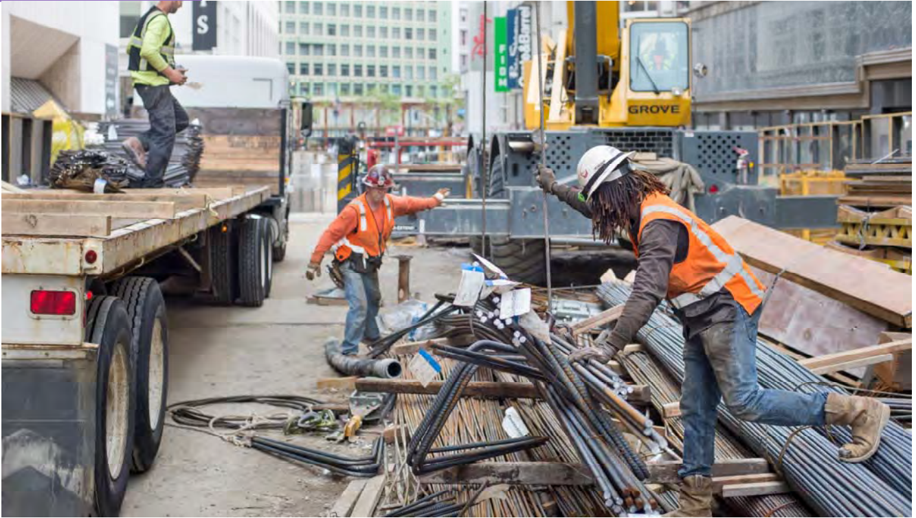
Men unload bundles of rebar off a flatbed, to be brought into the Union Square/Market Street station box from the staging area north of O'Farrell.
