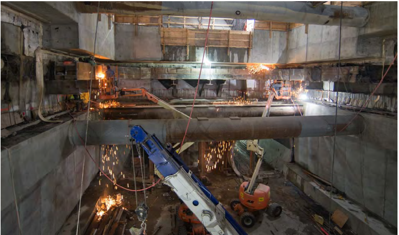
The last few sections of temporary bracing are being removed from the south end of the Union Square/Market Street station box.
