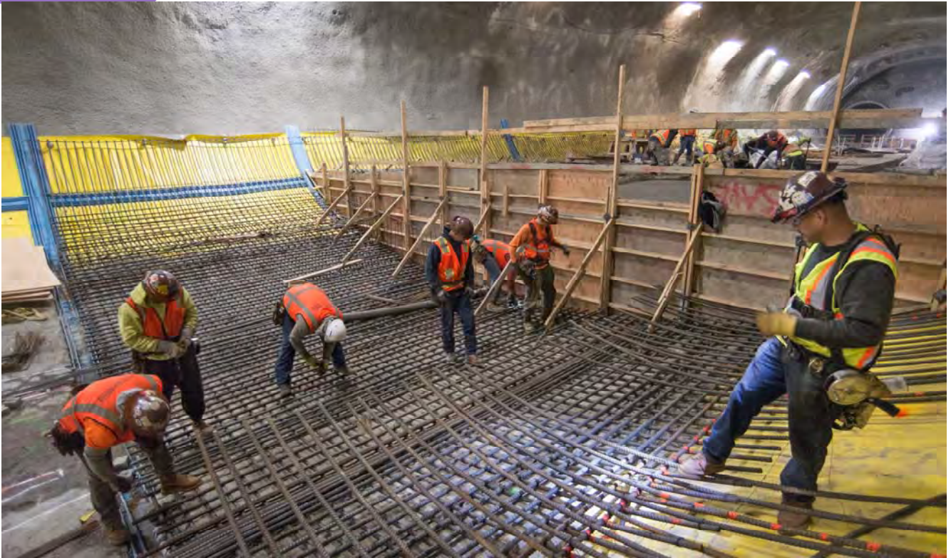
A crew assembles the rebar cage for the invert of one of the last sections of the Chinatown track crossover cavern, south of the future station platform cavern.
