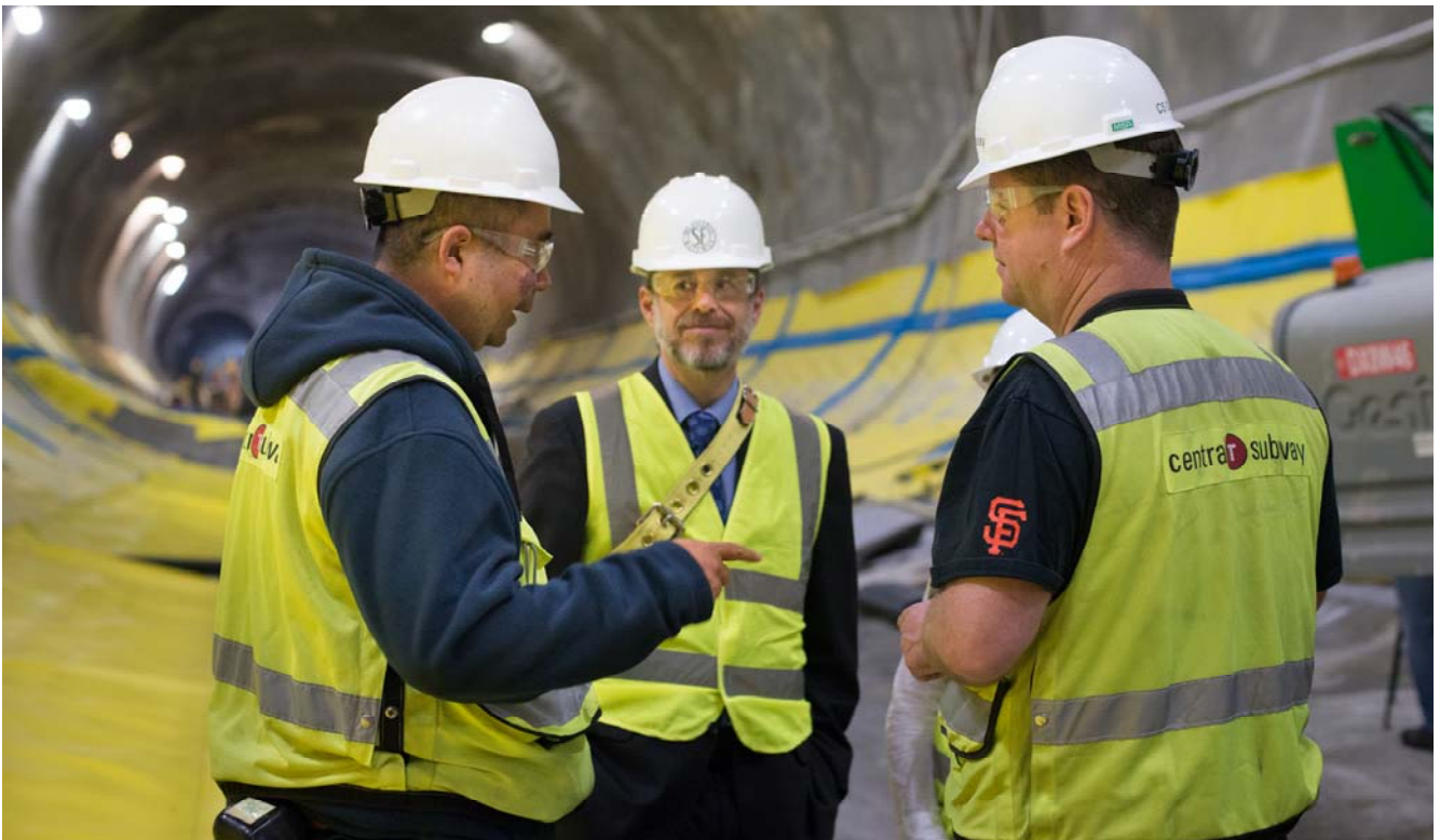
Looking south inside the Chinatown platform cavern, Central Subway Resident Engineer Wyman Lee discusses station construction with Mayor Mark Ferrell and SFMTA Director Ed Reiskin.
