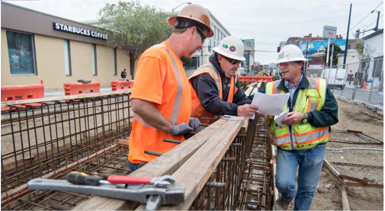
Workers look over site plans at the 4th and Brannan surface station platform, where utility conduits are being installed.
