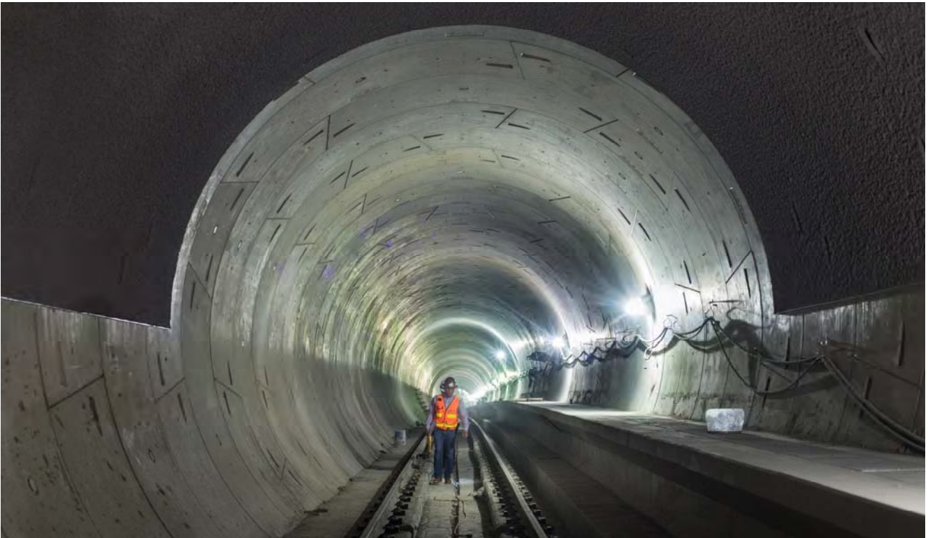
Two men move quietly down the southbound tunnel toward the Yerba Buena/Moscone Station platform.
