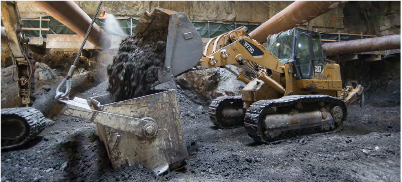
A bulldozer loads a large steel container one bucket at a time. This container is used to remove all excavated material excavated from the headhouse and station cavern.
