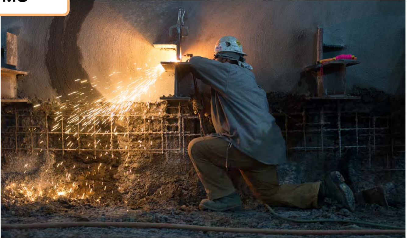
Sparks fly as a worker precisely cuts steel brackets to align with each other ahead of installing even larger reinforcing steel inside the station box.
