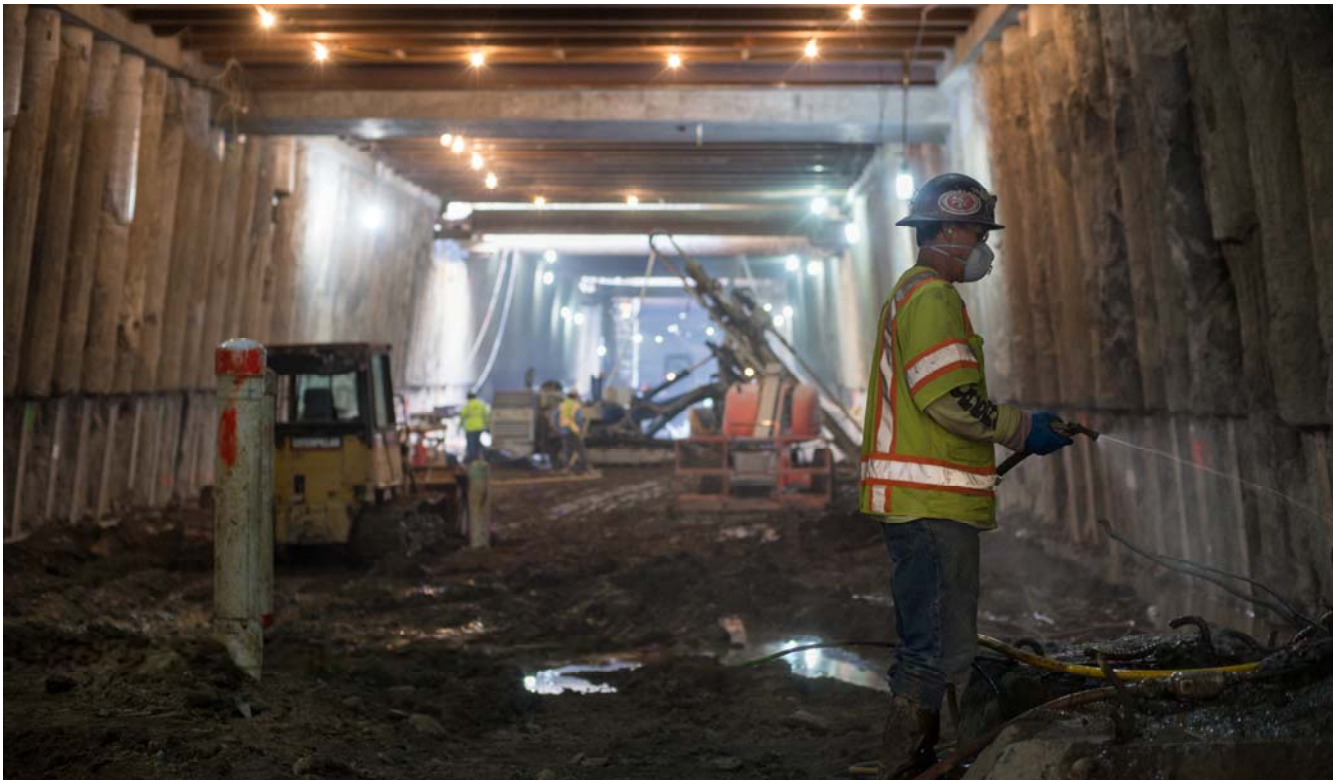
A long view looking north under Stockton Street, down the full length of the station interior. Water is sprayed on jackhammering to keep dust down inside the station box, at the south headwall.
