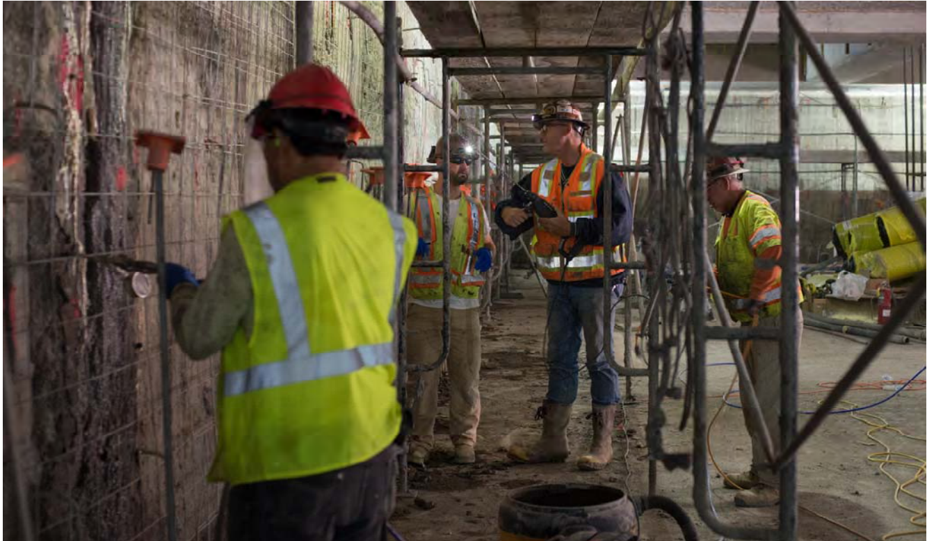
Workers drill holes to install rebar against the outer slurry walls of the station box. Sheets of waterproofing and finally the finished outer station walls will be installed against them.
