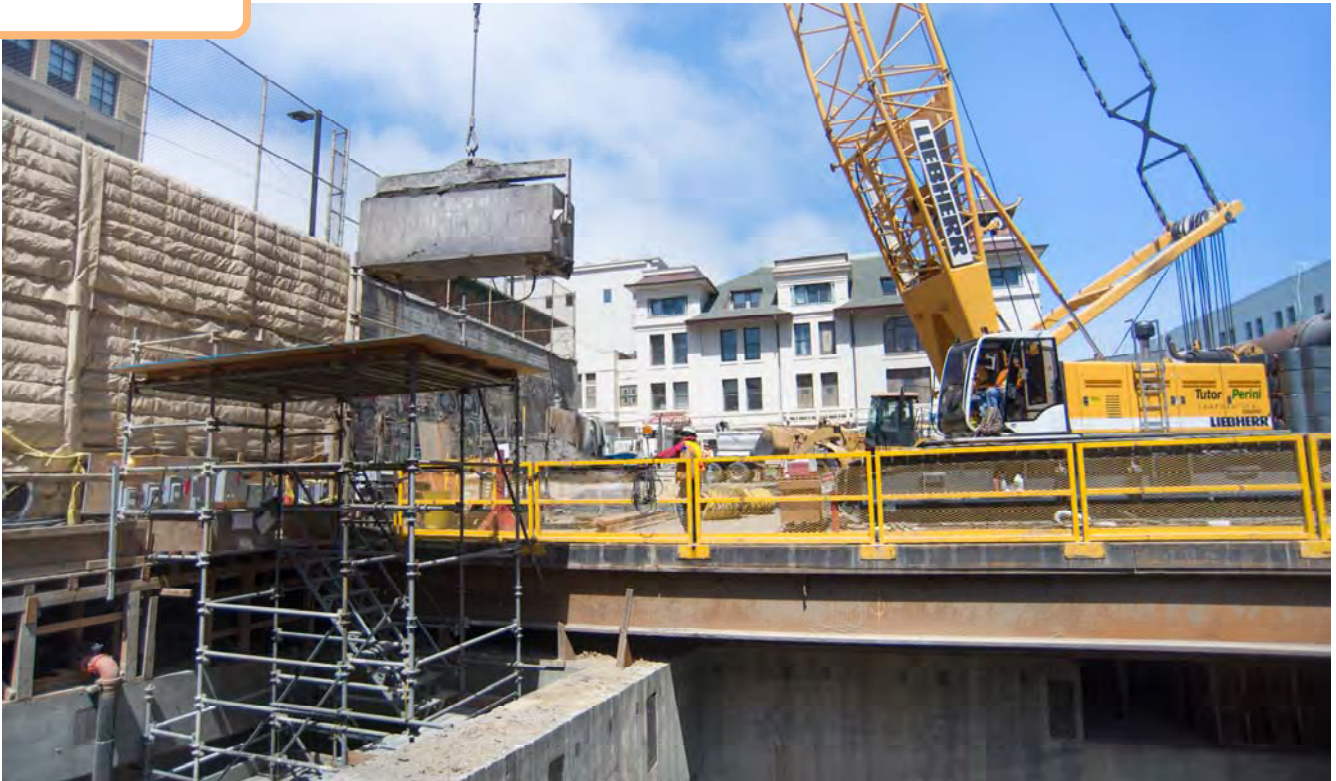
Atop the roof deck, a crane operator slowly swings the large steel bucket used to remove excavated material from inside the station headhouse.
