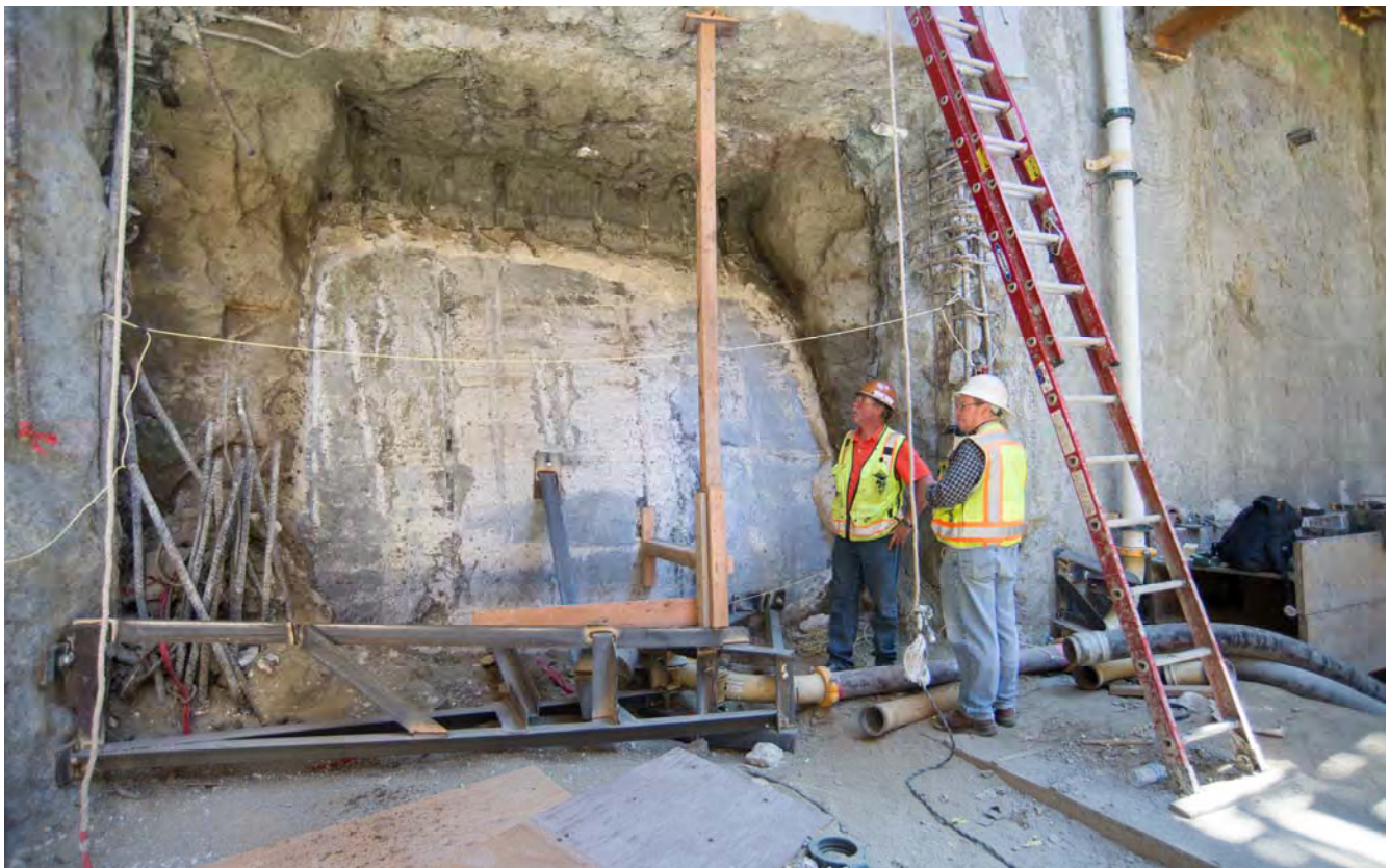
The shell of the southbound tunnel is seen exposed, adjacent to the slurry wall of the headhouse. Sections of tunnel inside the station box will be demolished, and a permanent floor slab will be built in their place.
