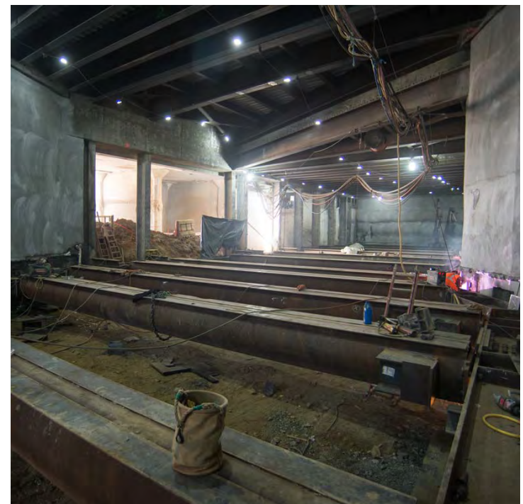
3 Brackets, walers, and struts are installed before the next phase of excavation begins.
