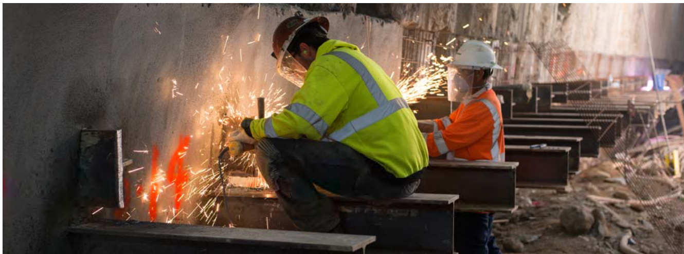
Workers use angle grinders to smooth edges of brackets ahead of water installation inside the station box.
