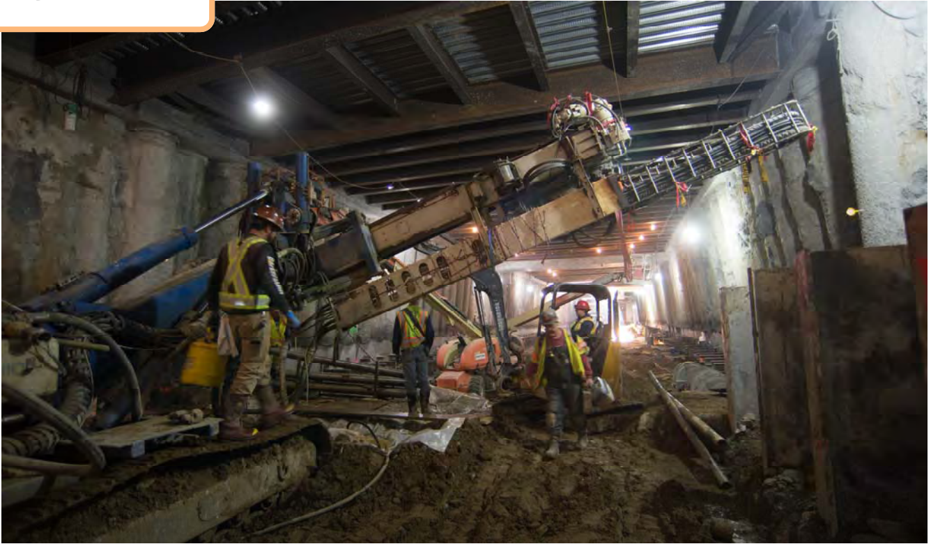
Workers step around equipment and machinery at the south headwall, where a drill rig is being used for compensation grouting work.
