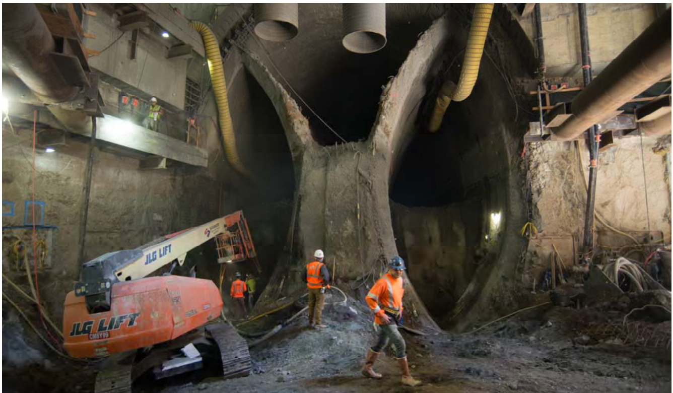
Workers spray a fibrous quick-hardening slurry solution called shotcrete on the outer walls of the cross-cut cavern following excavation to prevent against ground movement.
