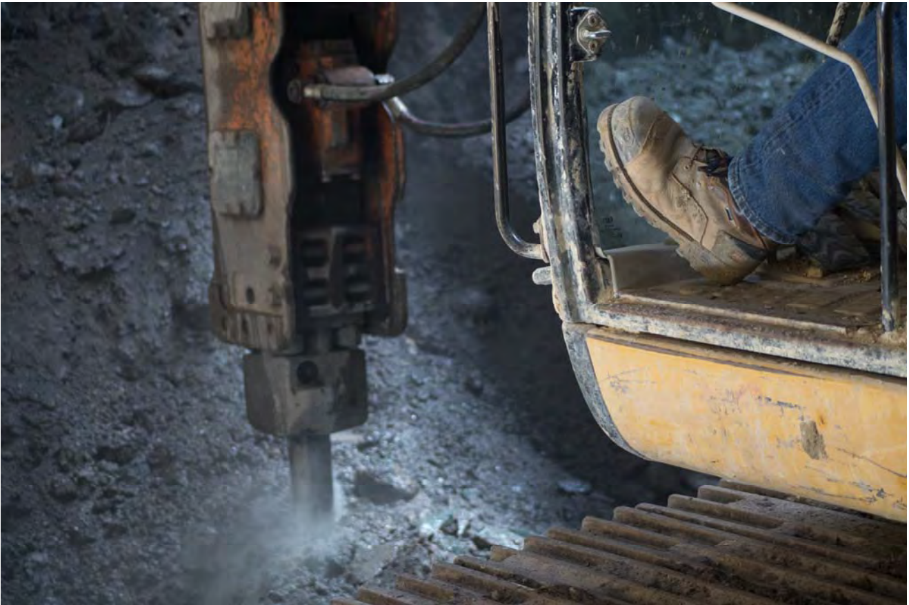
A jackhammer pulverizes bedrock uncovered during excavation work inside the Chinatown Station headhouse.
