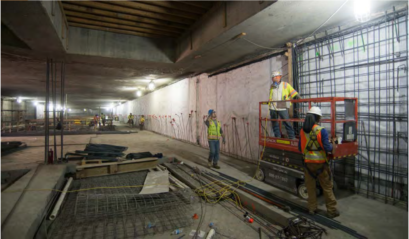
Workers prepare the walls of the station box for installation of rebar, concrete, and waterproofing materials.
