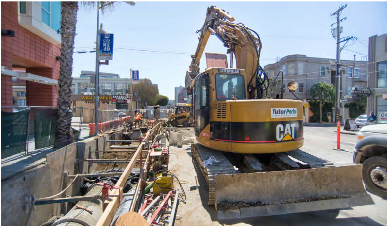
New dual sewer lines are being installed on the east side of 4th between Brannan and Bryant.
