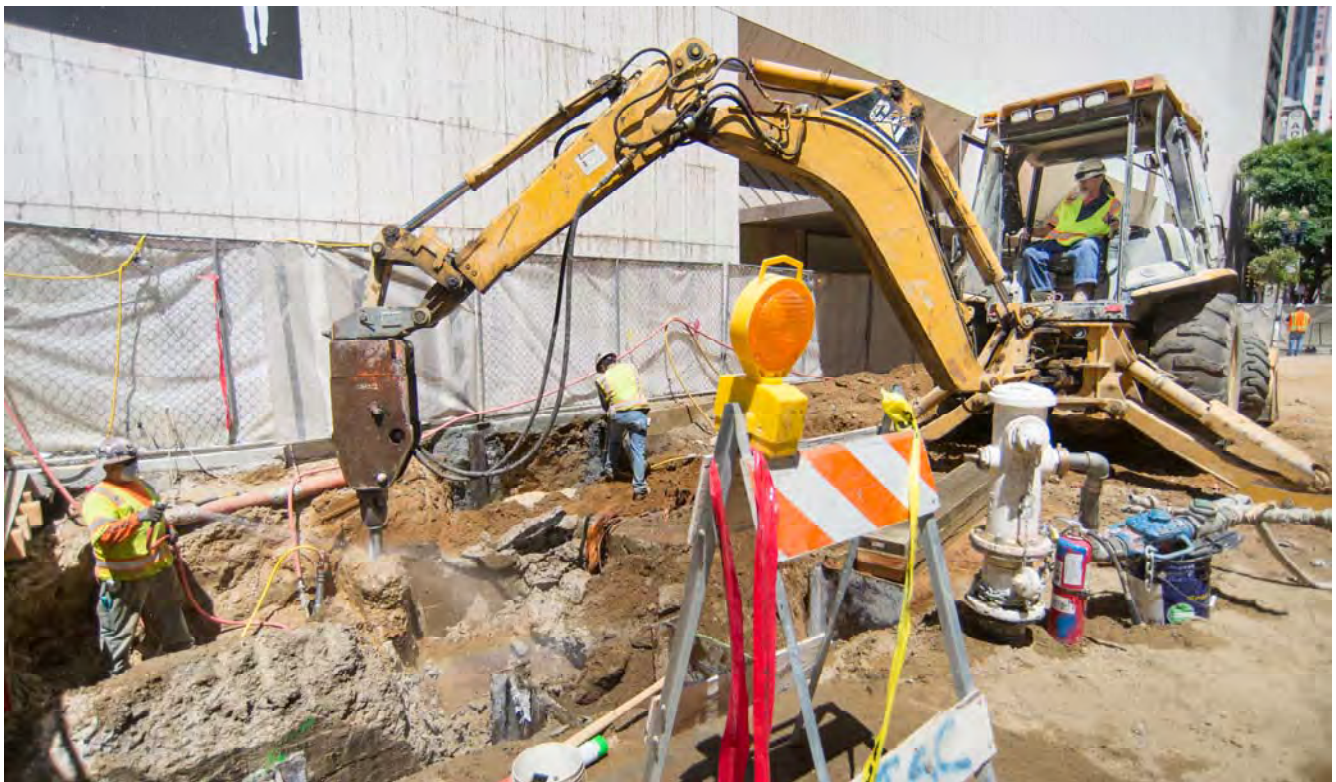
Old utility vaults and abandoned basement walls are removed on O'Farrell prior to site excavation and the construction of an emergency exit staircase.
