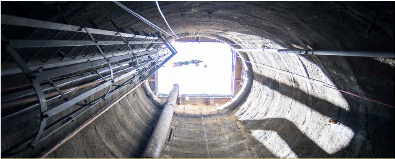
View looking up from the bottom of the north access shaft for Chinatown Station. The shaft is located on the east side of Stockton between Jackson and Washington.
