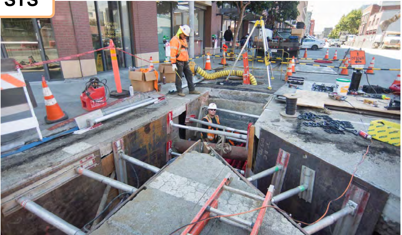
Utility trenches split off at Bluxome, where new conduits and other utilities are being installed and relocated.
