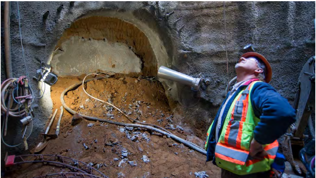
A worker peers toward the surface dozens of feet above, from the bottom of the north access shaft, where a connecting tunnel is being excavated.
