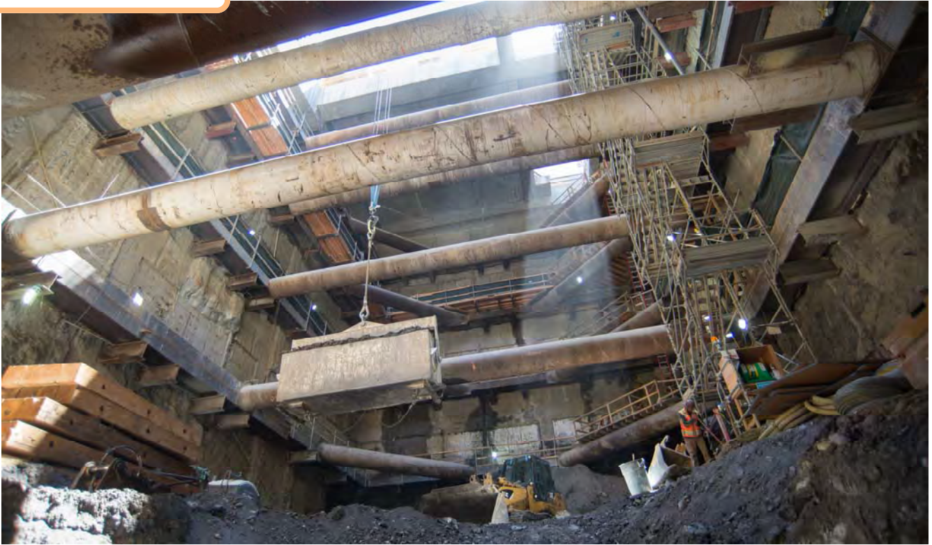
Large struts span the width of the headhouse to provide stability against the exterior slurry walls, while the steel bucket used to lift excavated material is carried to the surface.
