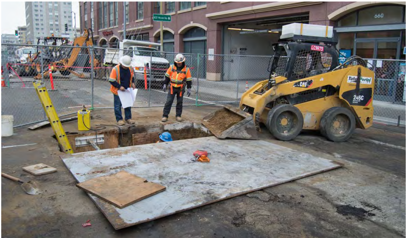
Workers search through site plans to identify utilities found while conducting potholing operations along 4th Street, near Bluxome.
