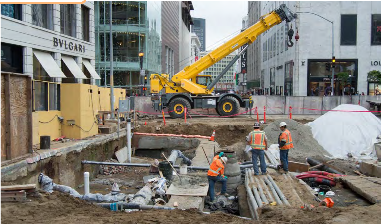
Workers make sense of a web of utilities being installed and upgraded atop the recently-constructed north concourse roof deck, on Stockton between Maiden Lane and Geary.
