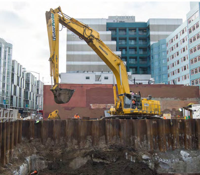
2 More soil is excavated, exposing the top portion of the next level of the station box.
