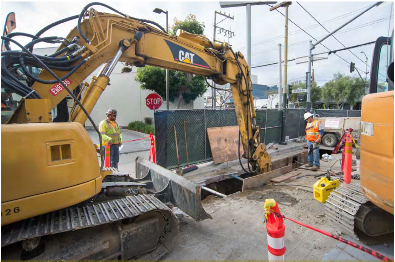
Workers carefully use machinery to aid in the installation of a high-pressure water line in a trench just south of Brannan on 4th.
