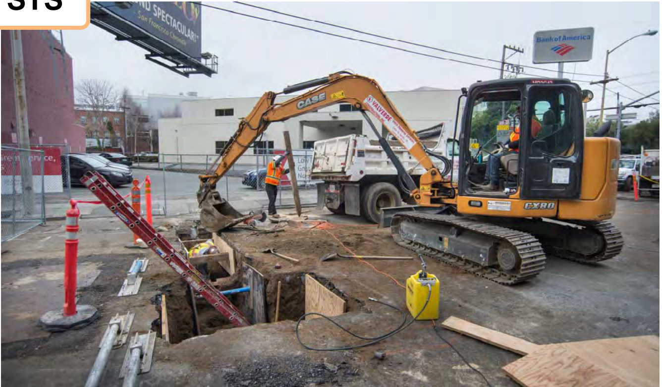
A small trench marks where utility potholing work is being conducted, on the west side of 4th Street just south of Brannan.
