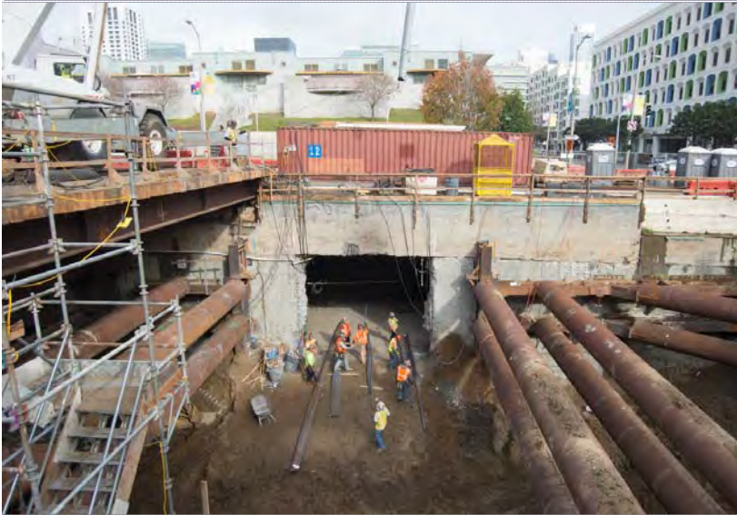
1 With the first level excavated, workers install rebar and a concrete slab.
