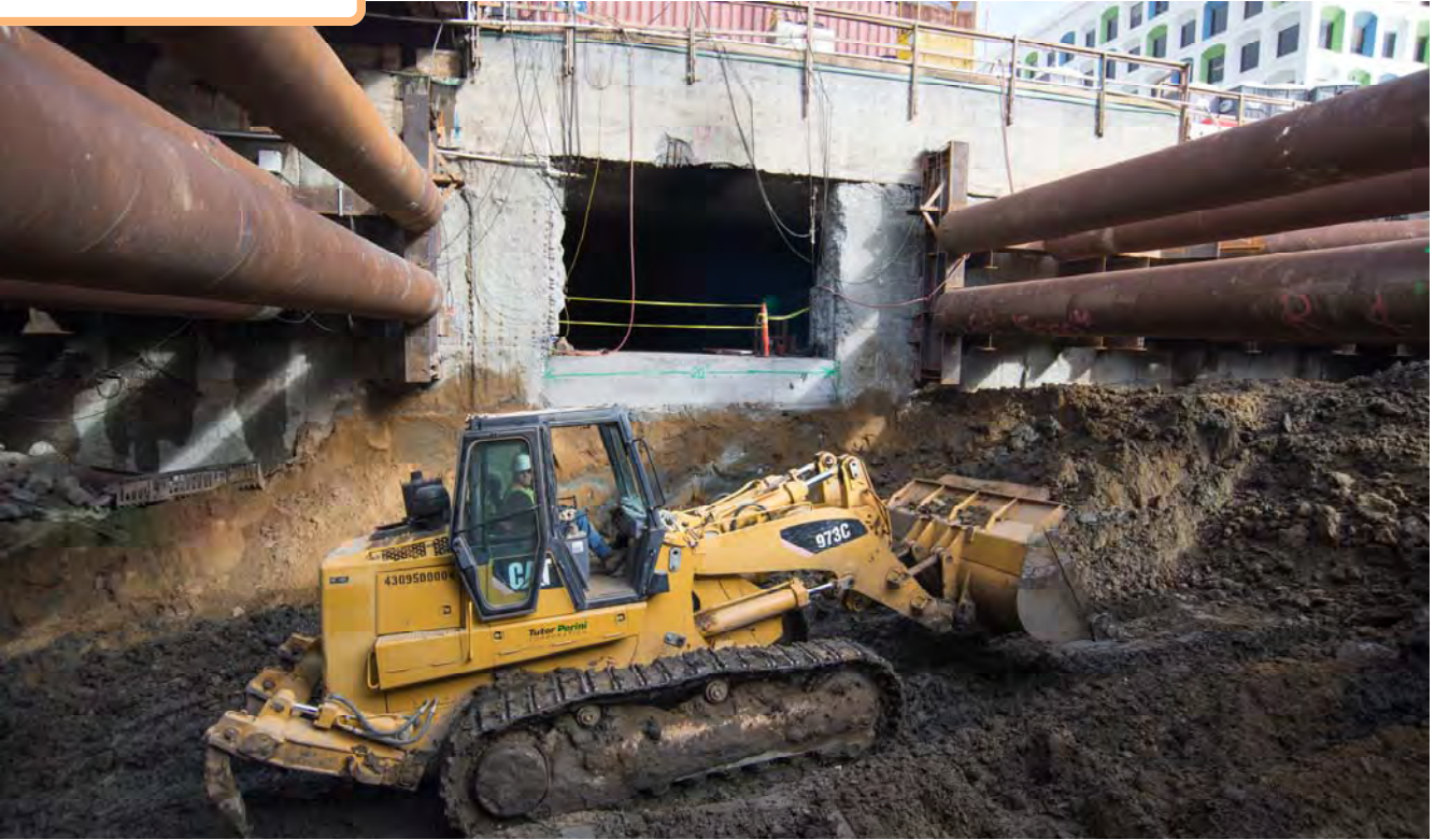
A bulldozer pushes material to where it can be removed inside the station headhouse.
