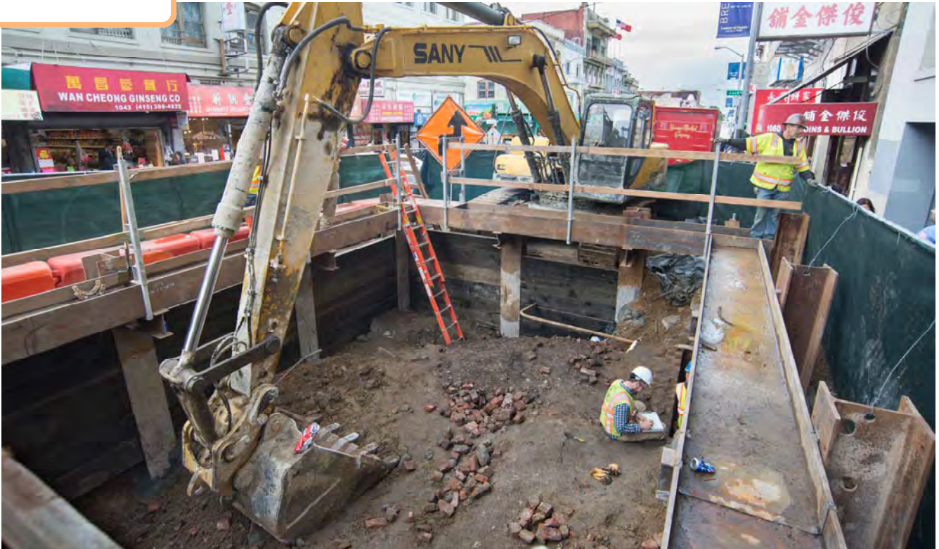
A new site involved in station construction at the north end of the station, where a shaft is being excavated for the construction of a future emergency access stairwell.
