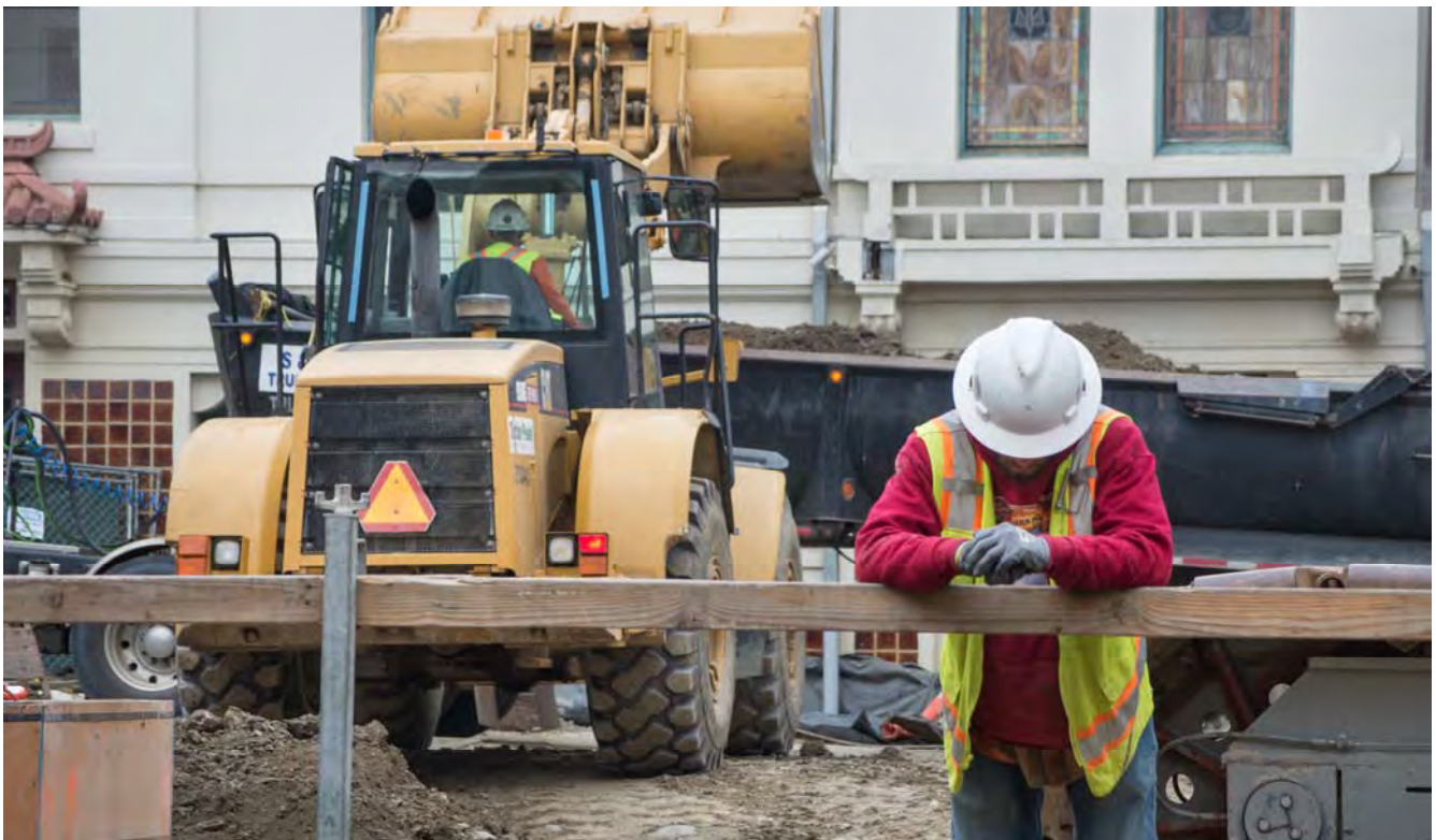
A flagger at the main access portal fence watches the steel bucket get lowered into place, while a loader dumps material into a dump truck in the background.
