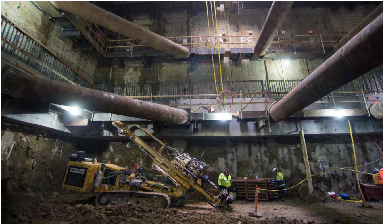
A drill rig used in waterproofing work is illuminated by work lights and a small access shaft far above.
