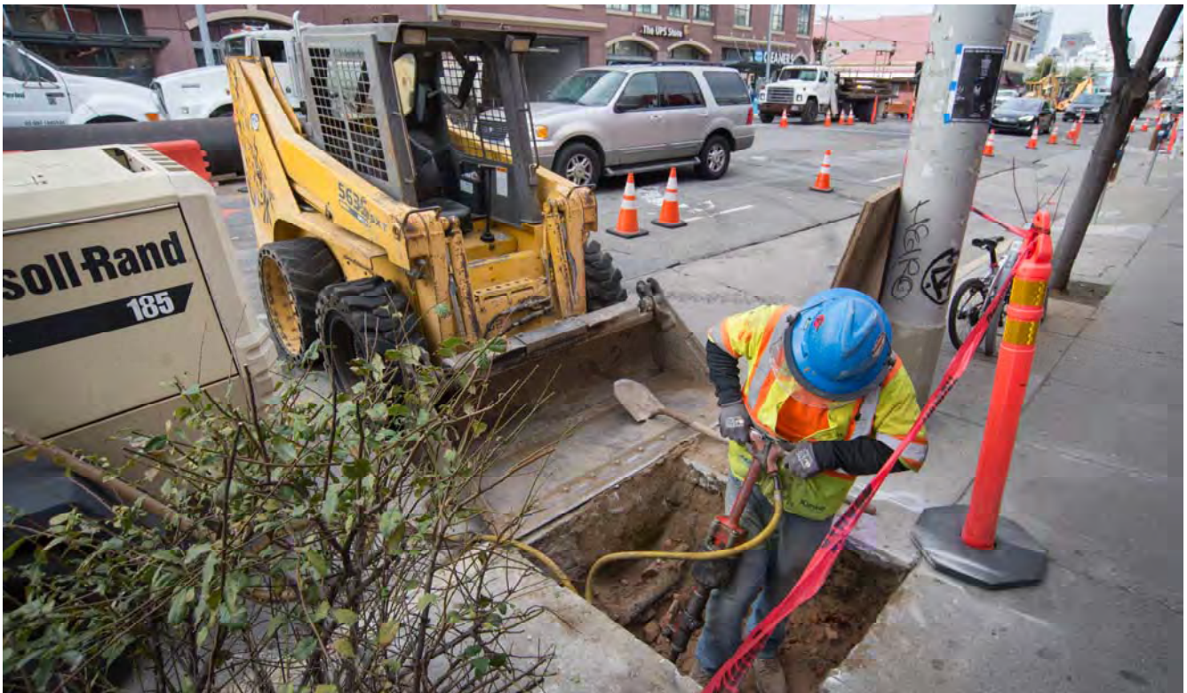
A worker removes hardened material where an OCS pole foundation is slated to be installed on 4th Street.
