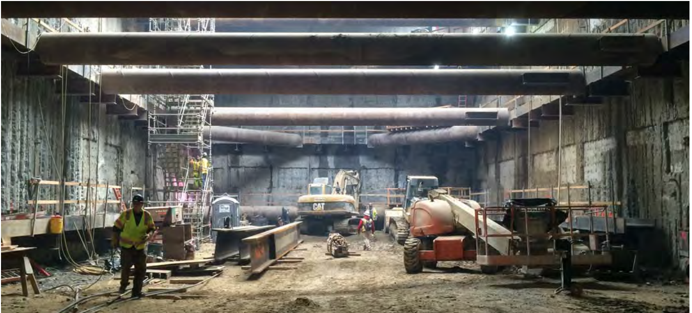
Large steel beams and other temporary structural reinforcing elements can be seen being prepared inside the Chinatown Station headhouse.
