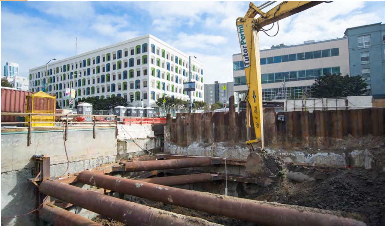
An excavator fitted with a long arm removes material excavated from the station box, temporarily collected inside the headhouse structure.
