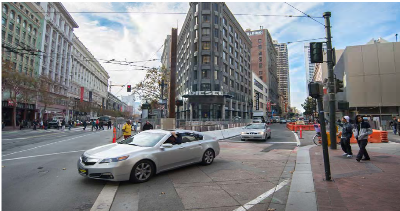
After completing the roof deck of the south concourse, backfilling, and restoring a lane of the roadway through the site, cars travel down Ellis to cross Market Street.
