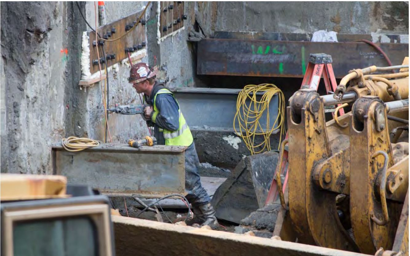
A worker drills pilot holes for rebar set to be installed in the face of one of the exterior slurry walls of the headhouse structure.
