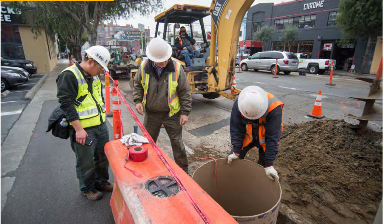
A site inspector observes foundation installation work for an overhead catenary system (OCS) pole, set to be installed here for the surface portion of the alignment.
