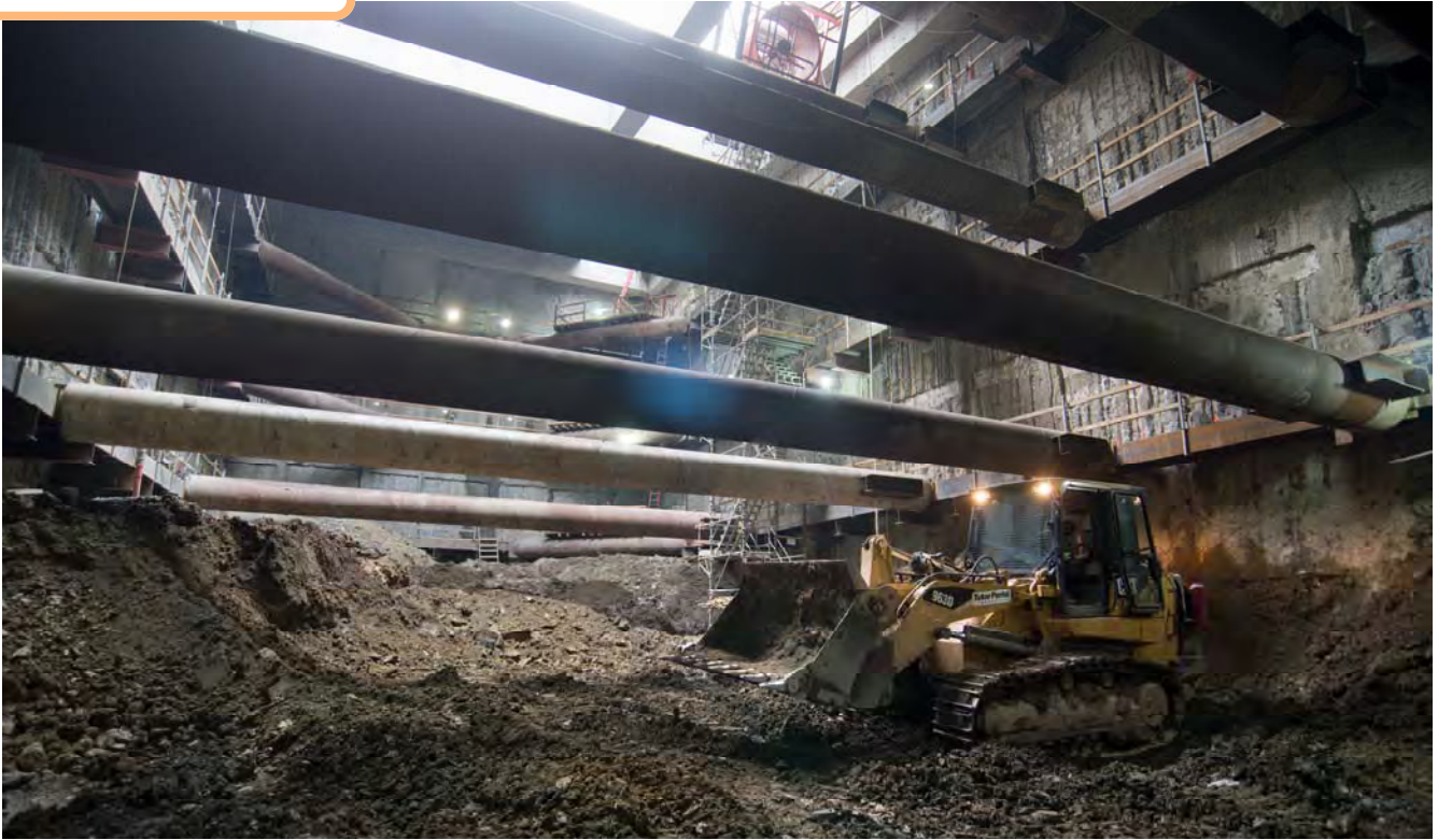
At the bottom of the headhouse, a bulldozer operator moves material to where it can be loaded in a large steel bucket to be lifted to the surface.
