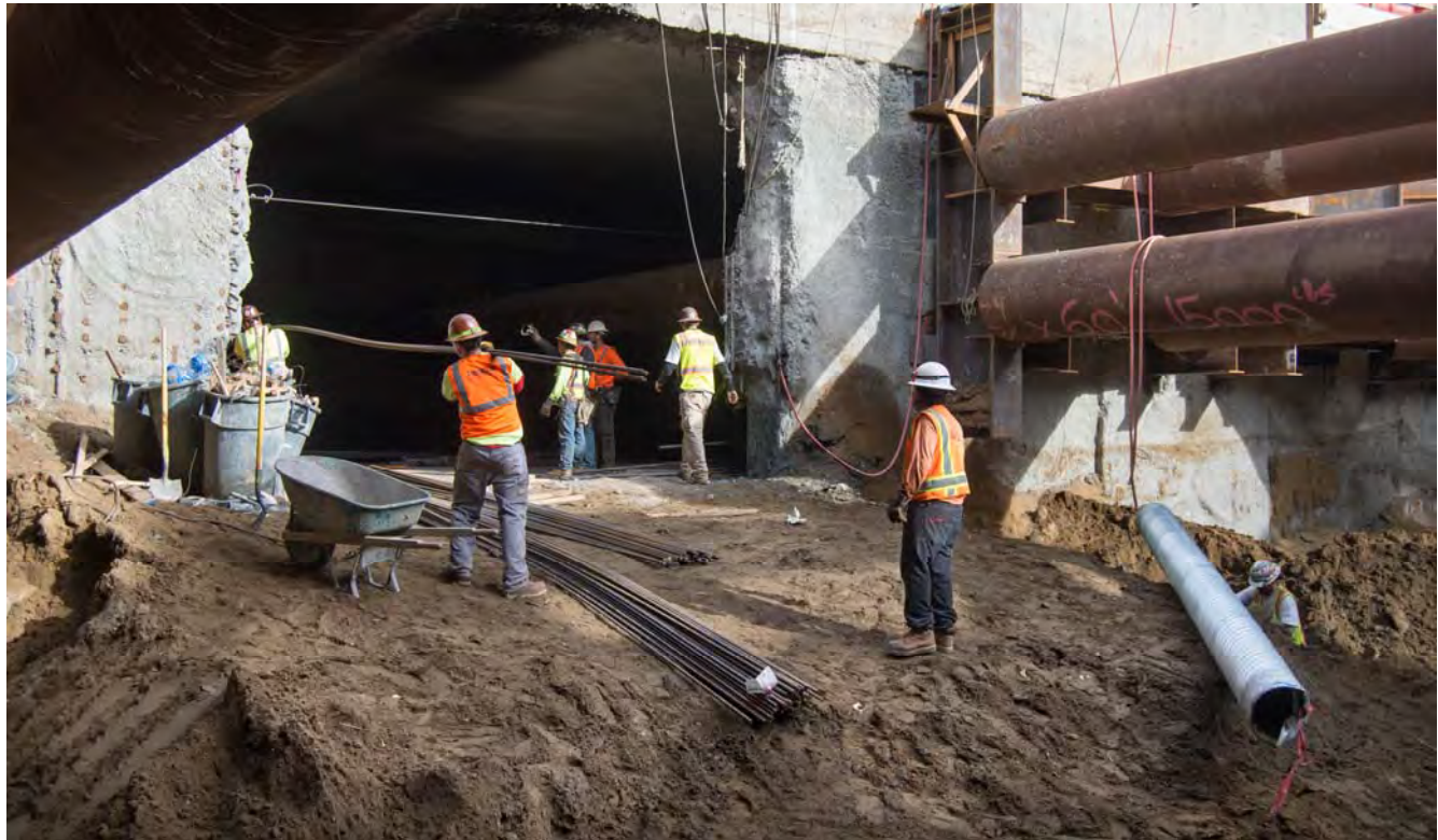
Workers lift long strands of rebar to carry them inside the station box, where a large, reinforced concrete slab is being constructed.
