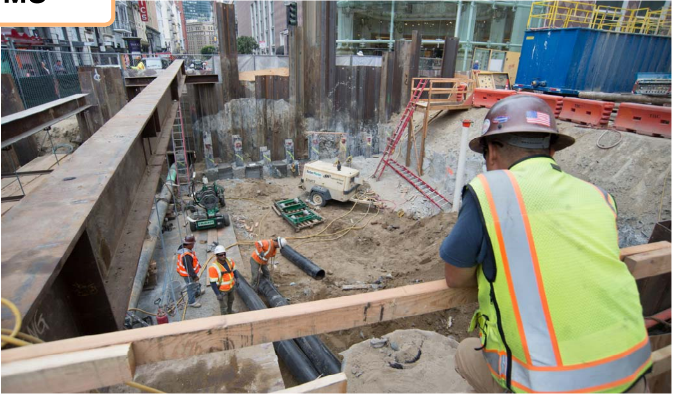
Workers begin installation of a sewer line on the south side of the intersection at Geary and Stockton prior to station concourse roof installation.
