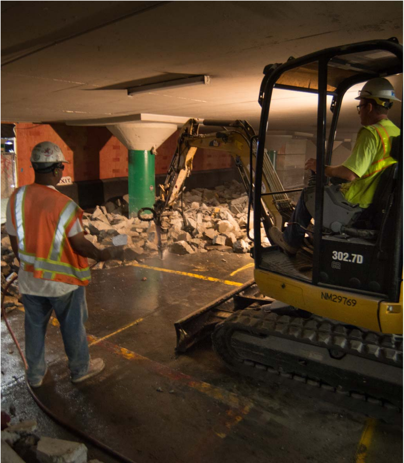
Dust is kept down during floor slab demolition inside the Union Square Garage by spraying a light mist of water onto material being broken apart.
