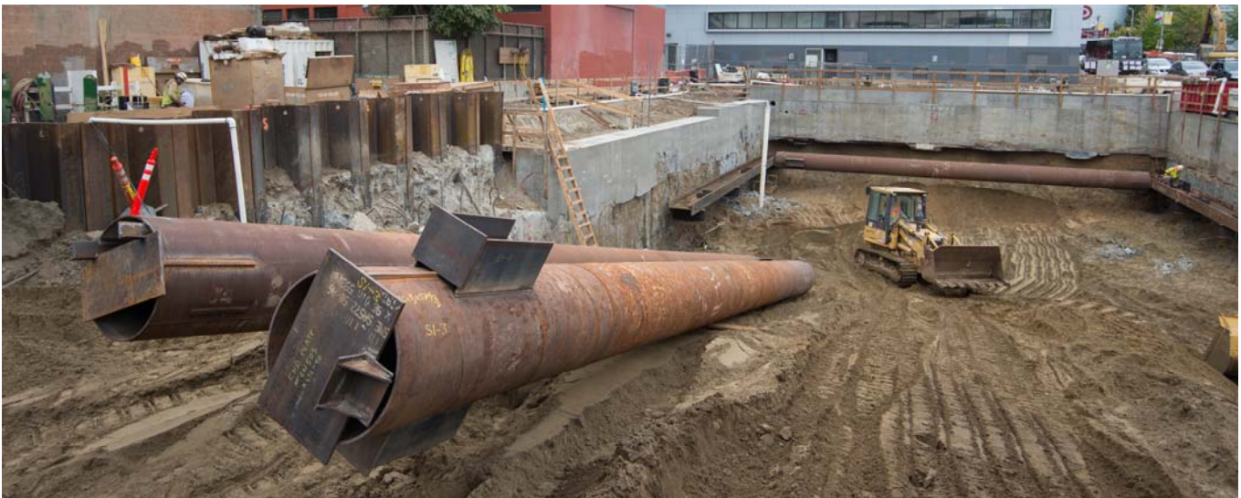
Steel cylinders called “walers” are used as temporary supports during excavation of the Yerba Buena/Moscone Station headhouse.
