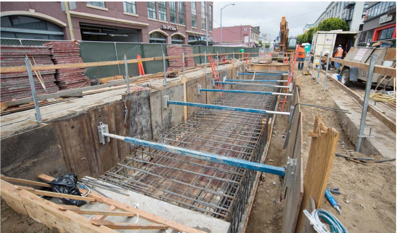
An exposed rebar cage prior to pouring concrete for a sewer upgrade on 4th Street south of Bluxome.
