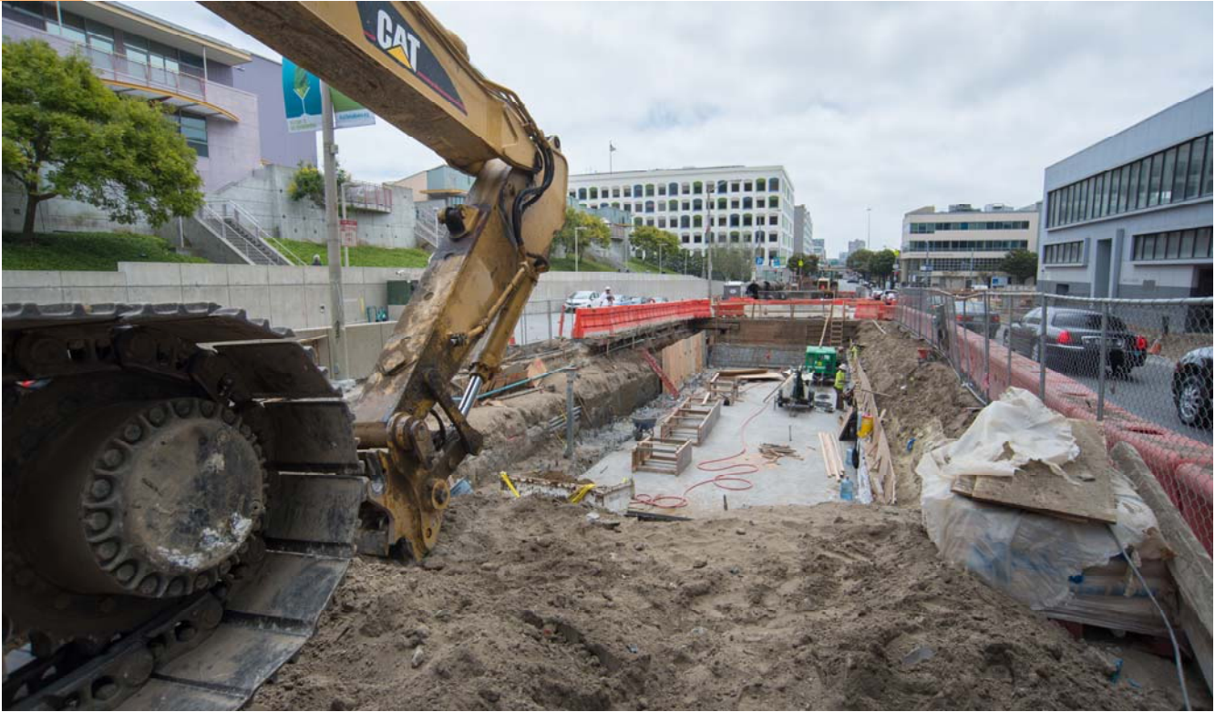
An excavator waits while the last section of roof deck for the station platform structure is being constructed in the background.
