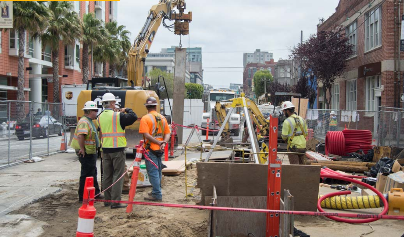
Sheet pile installation for trenching operations just north of Welsh Alley on 4th Street in SoMa.
