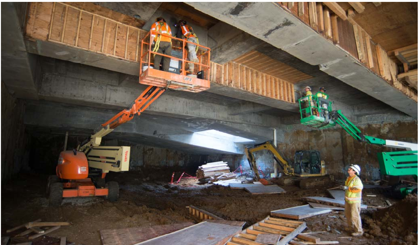
After the first level of excavation was completed under the roof slab, workers then removed what concrete forms had been exposed and left behind.
