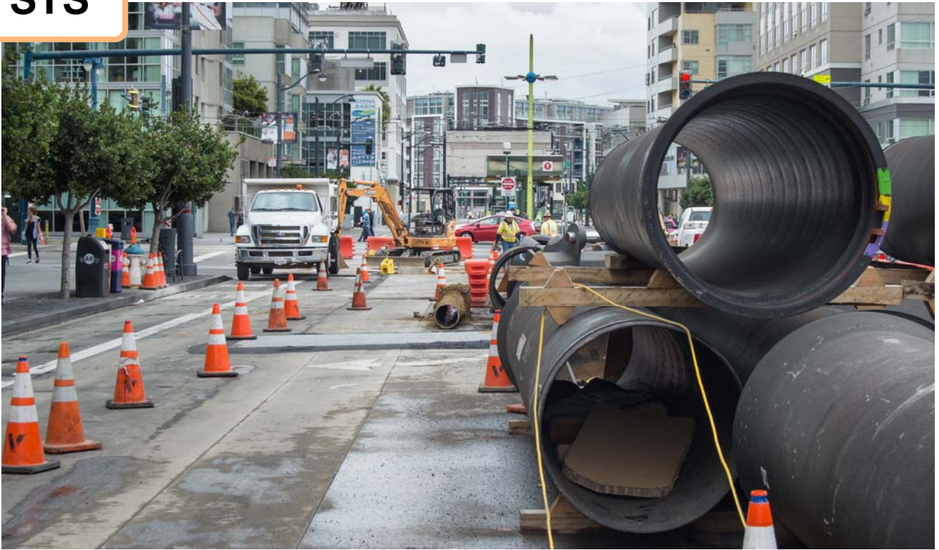
Sewer pipes waiting to be installed overlook utility work near the intersection of 4th and King.
