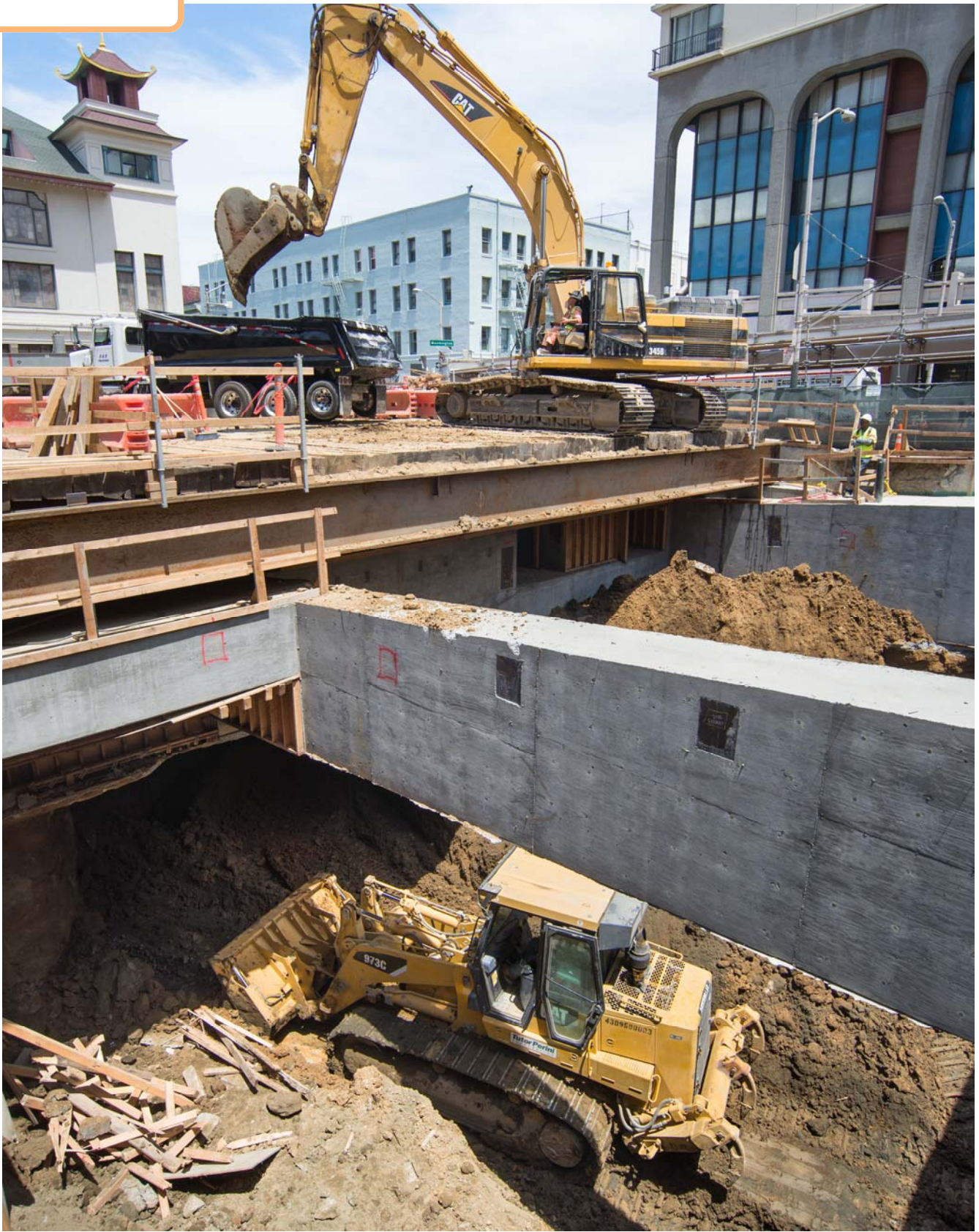
A bulldozer brings out soil and other materials removed from under the Chinatown Station roof slab, while an excavator pulls it up and fills a waiting dump truck.
