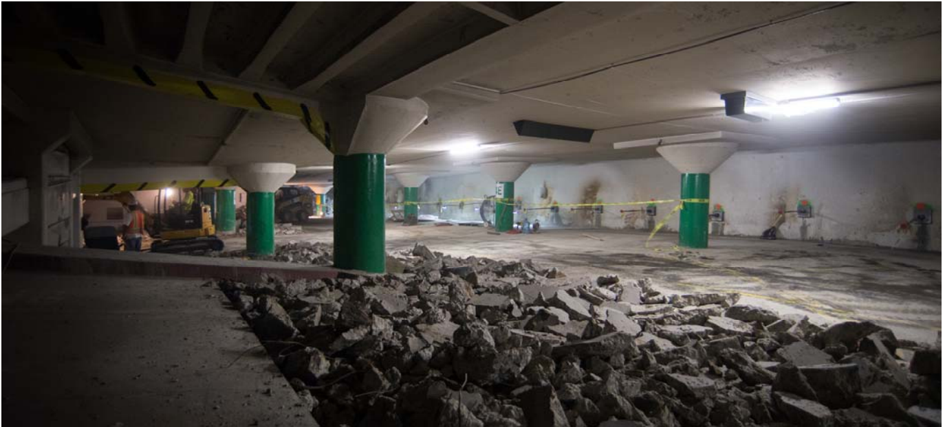
Broken concrete marks where demolition efforts have begun on the bottom level of the Union Square Garage. The southeast corner of the garage will be demolished to make room for a station entrance structure.
