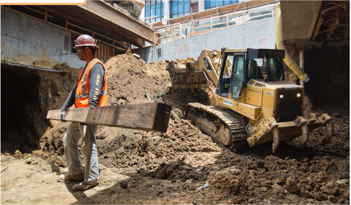
A worker removes boards left over from concrete forms under the roof slab.
