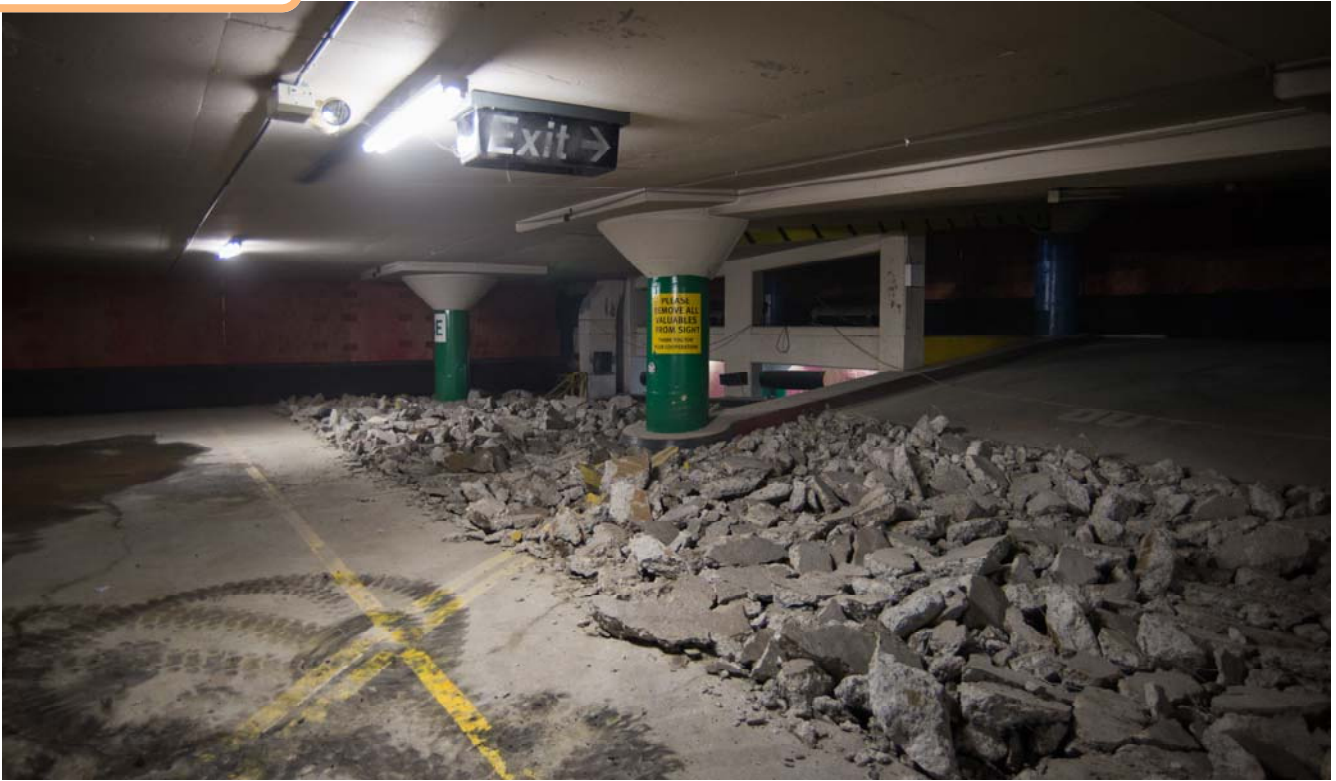
Portions of the southeast corner of the Union Square Garage are being demolished, prior to the construction of the north station entrance, there.
