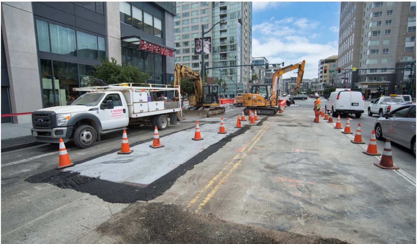
Trenching work on 4th Street just north of King, temporarily covered by steel plates.
