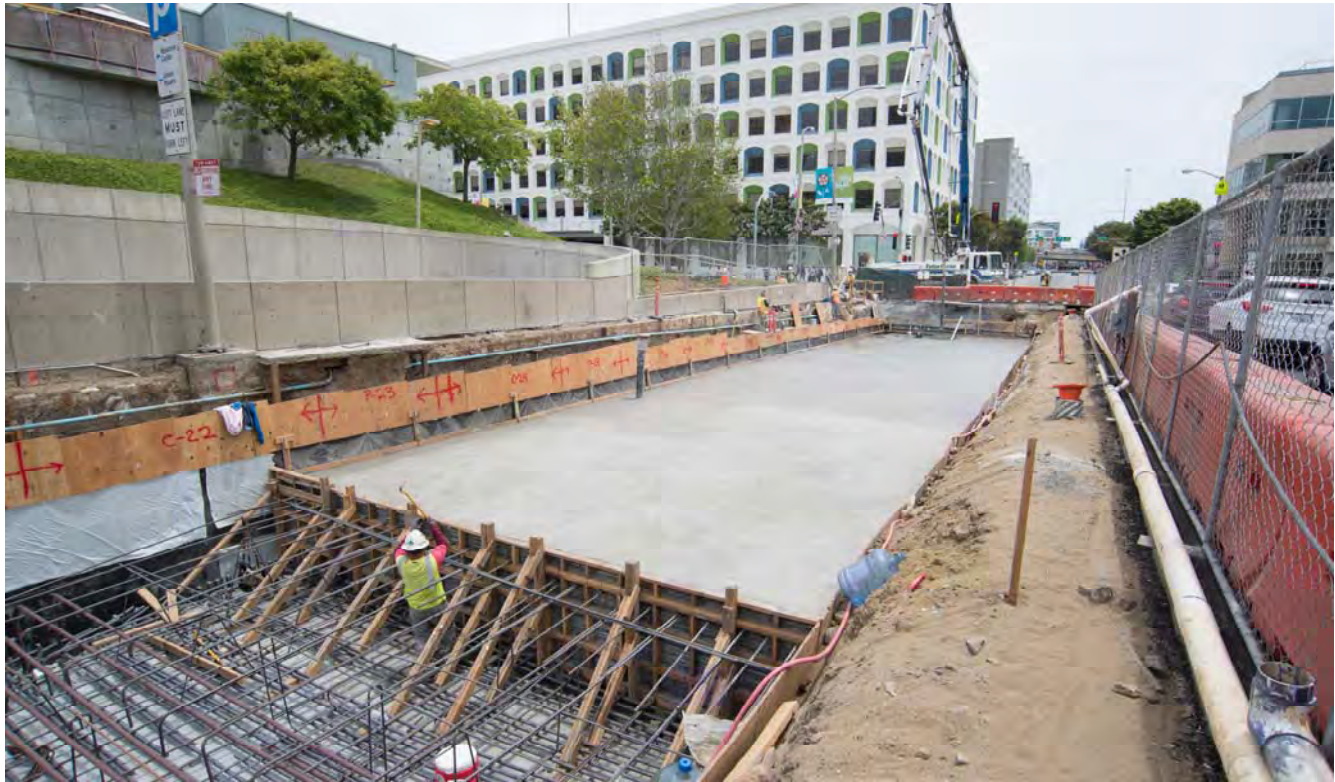
Each section of roof slab is composed of reinforced concrete, and is several feet thick.
