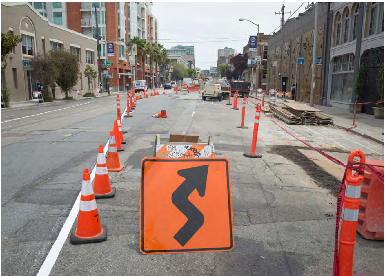
Signage marks a temporary detour near the intersection of 4th and Bryant. Work to relocate and upgrade existing utilities is underway here.
