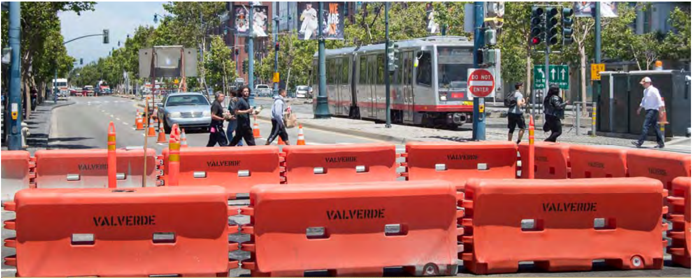
Triton barriers mark the outline of some utility relocation work being done at the intersection of King and 4th Street in SoMa.
