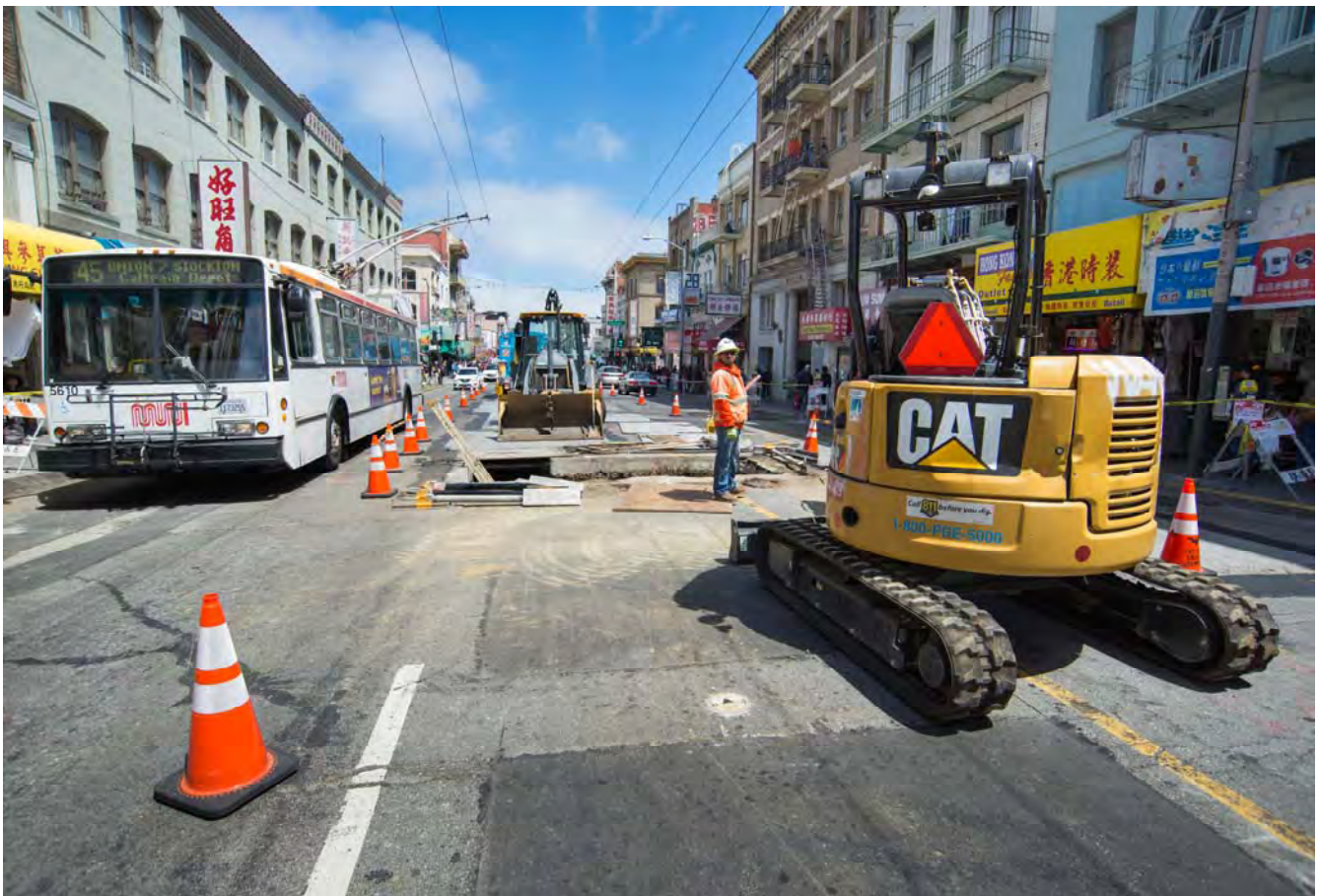
Prior to the excavation of an emergency access shaft halfway between Washington and Jackson on Stockton, work to relocate utilities is underway.
