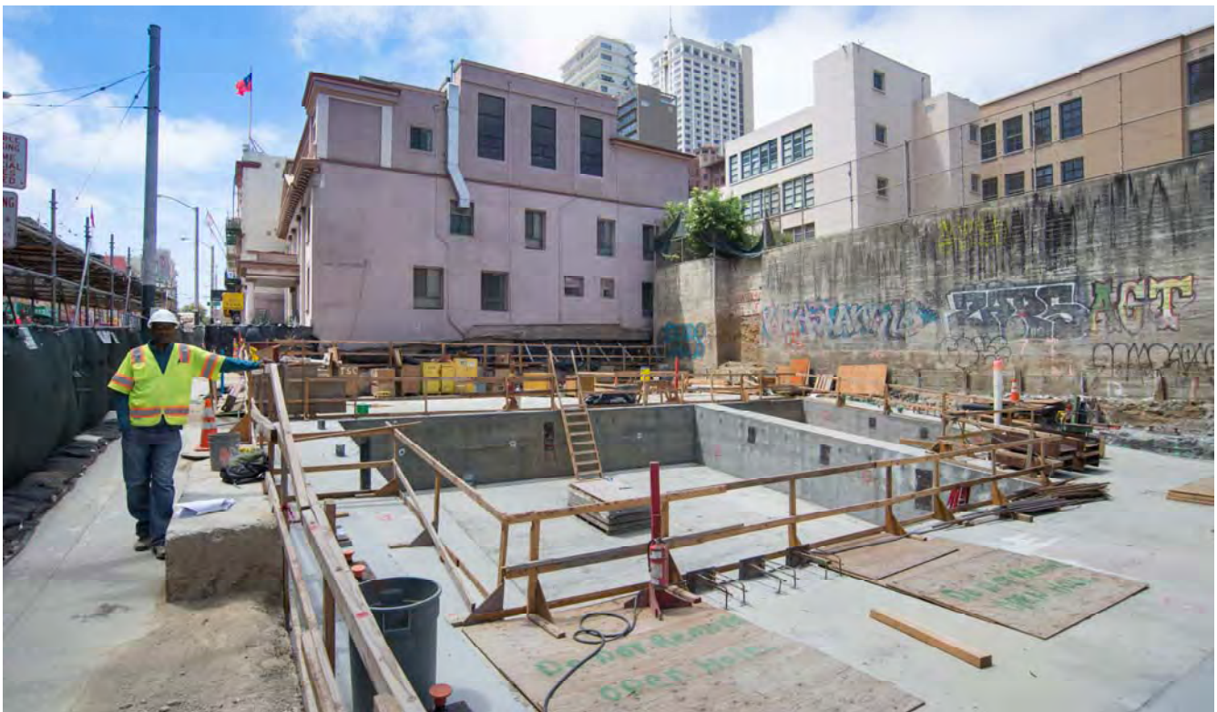
Workers will “break through” the temporary concrete slab constructed at the bottom of the access shaft shown here, when beginning excavation efforts.
