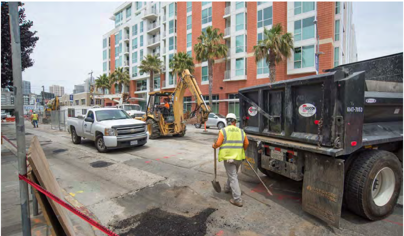
Workers have been conducting utility potholing, upgrading, and relocation activities along 4th Street, where the future surface alignment of the T Line will travel.
