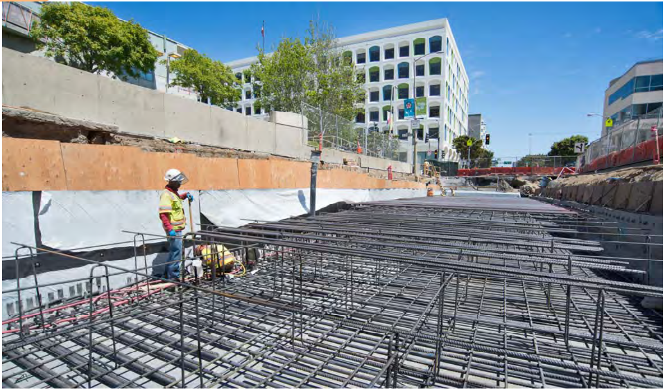
The roof of the Yerba Buena/Moscone Station is being constructed in phases. Work on the west side of 4th Street has been completed. Here work on the east side is underway.
