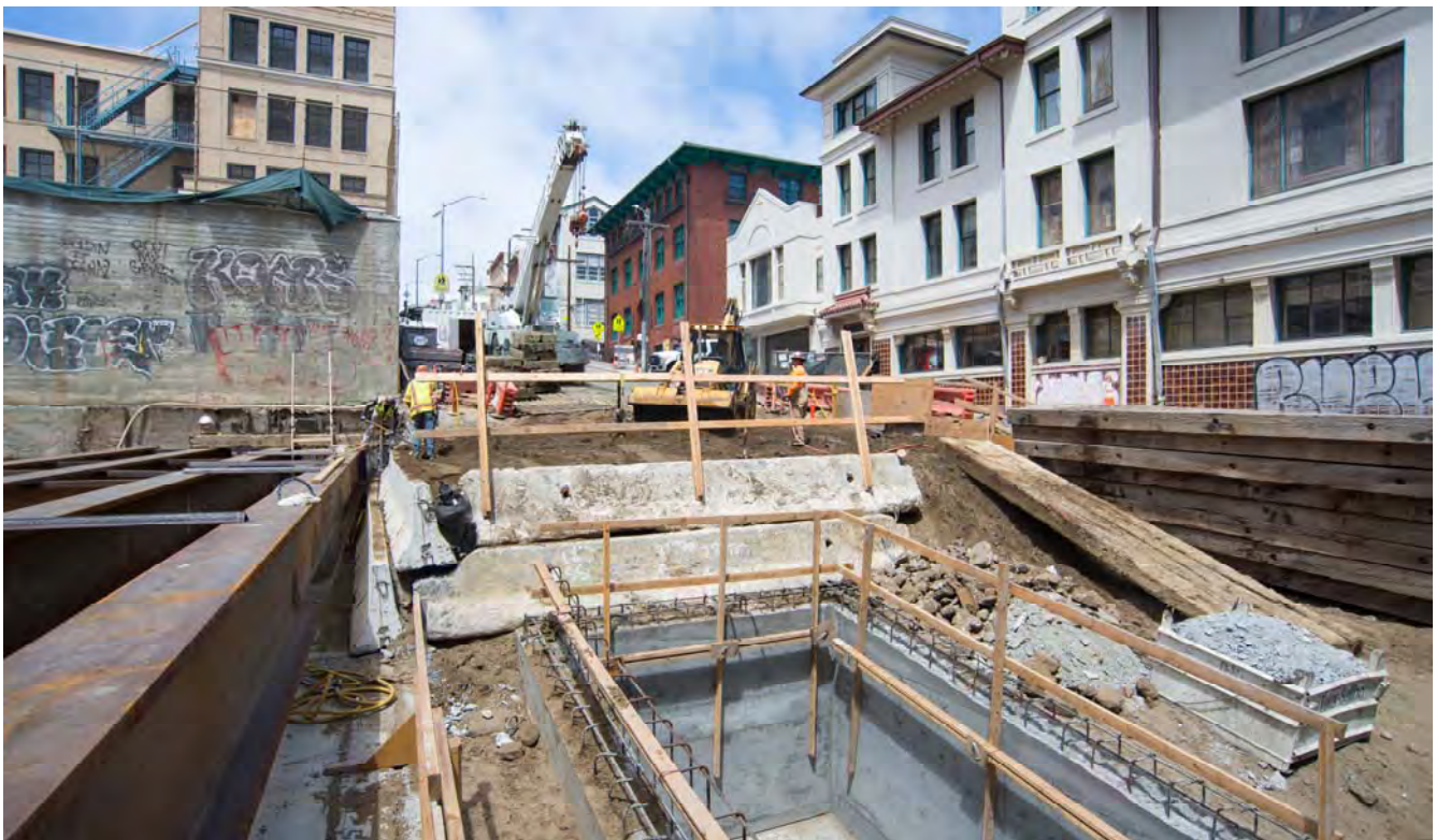
A future access shaft in the roof slab can be seen near a temporarily-backfilled portion of Washington Street.
