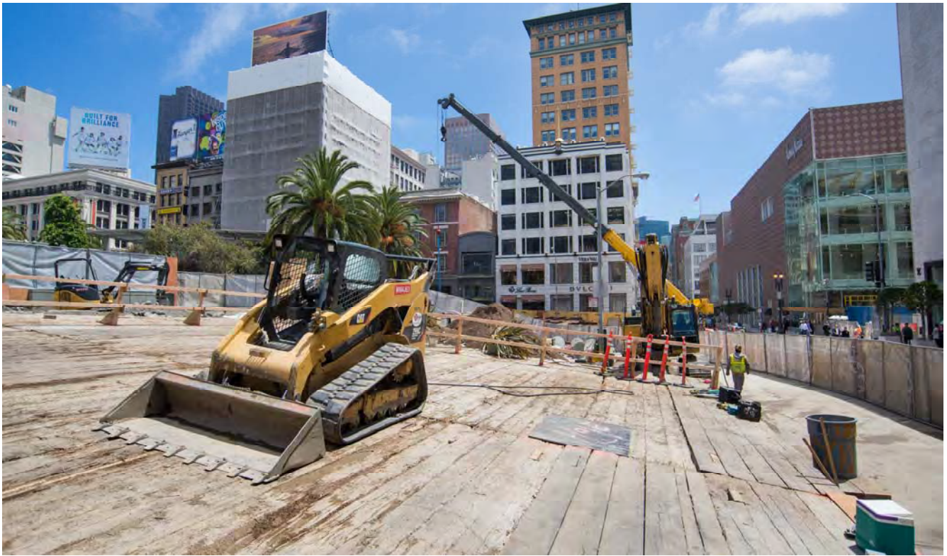
A temporary steel and wooden deck has been constructed over the future portion of the Union Square Garage that will be demolished prior to station entrance construction.
