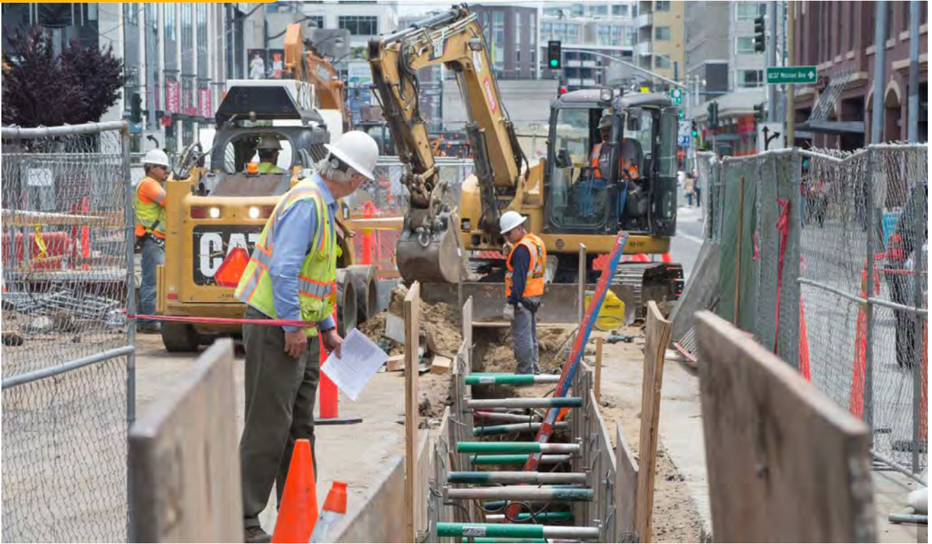
A worker inspects shoring at a trenching operation near Bluxome and 4th.
