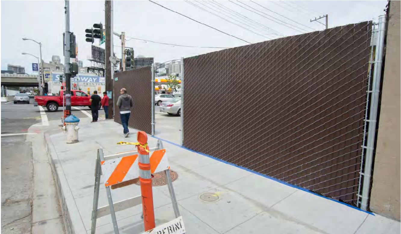
New fencing was installed outside local taqueria Chavo's. A new utility vault has been installed under the sidewalk, here.
