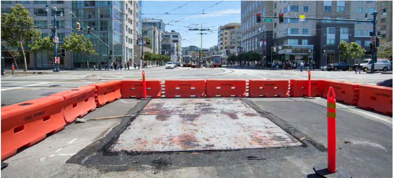
T Line trains arrive at the 4th and King surface station while utility relocation work is underway at the edge of the 4th and King intersection.
