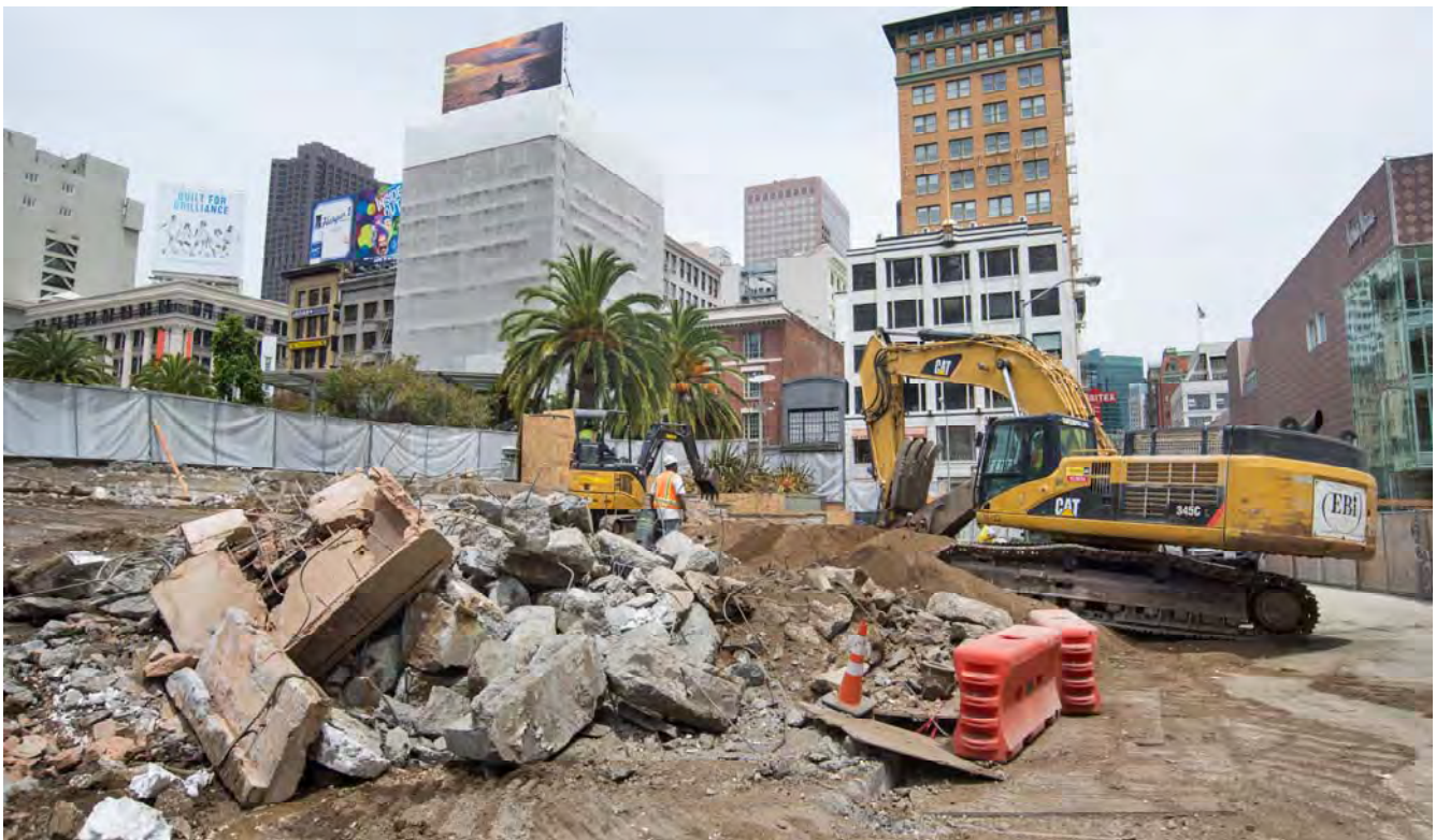
Rubble from benches and terrace walls is sorted by material before being removed off site.
