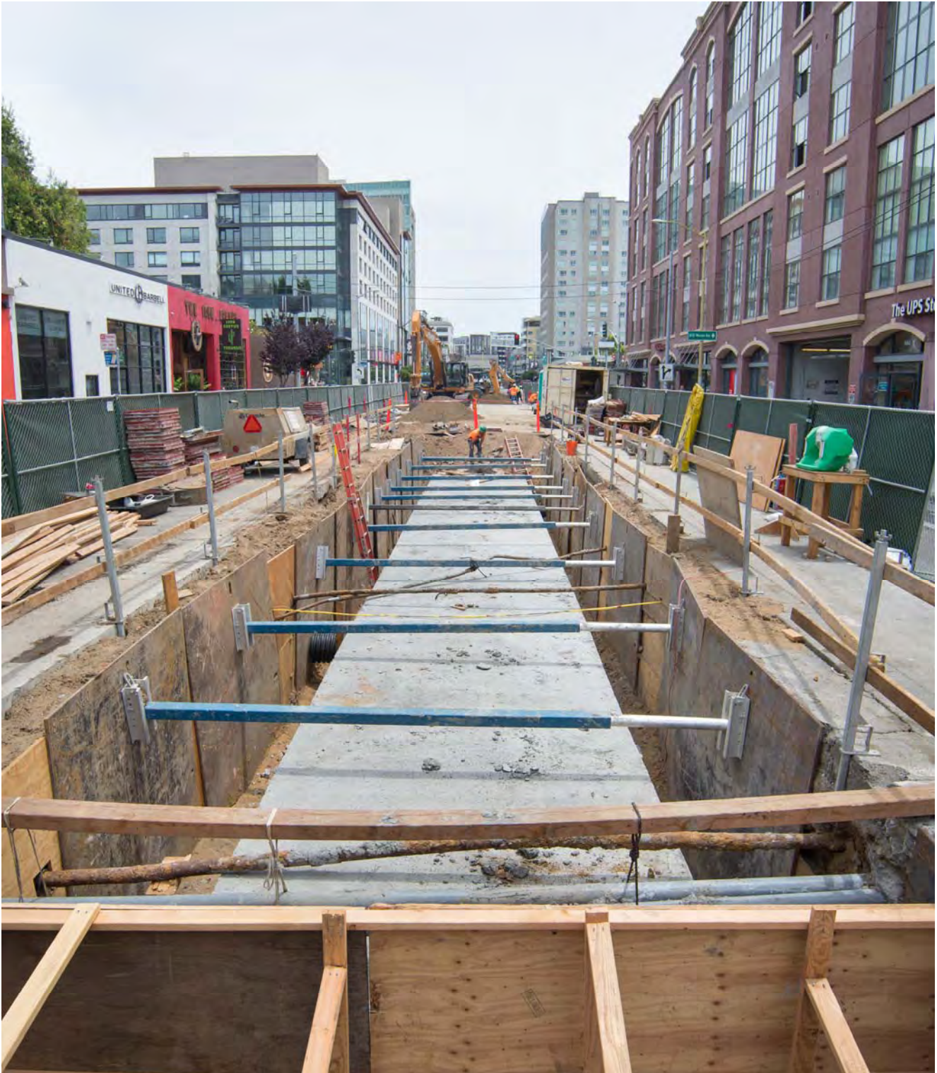
A finished section of reconstructed sewer roof just south of 4th and Bluxome. Once complete, this section will be backfilled and work will progress to the next section.
