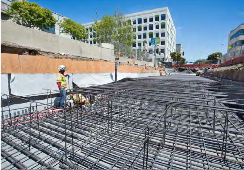
1 A gigantic rebar cage is assembled in place for each specific roof section
