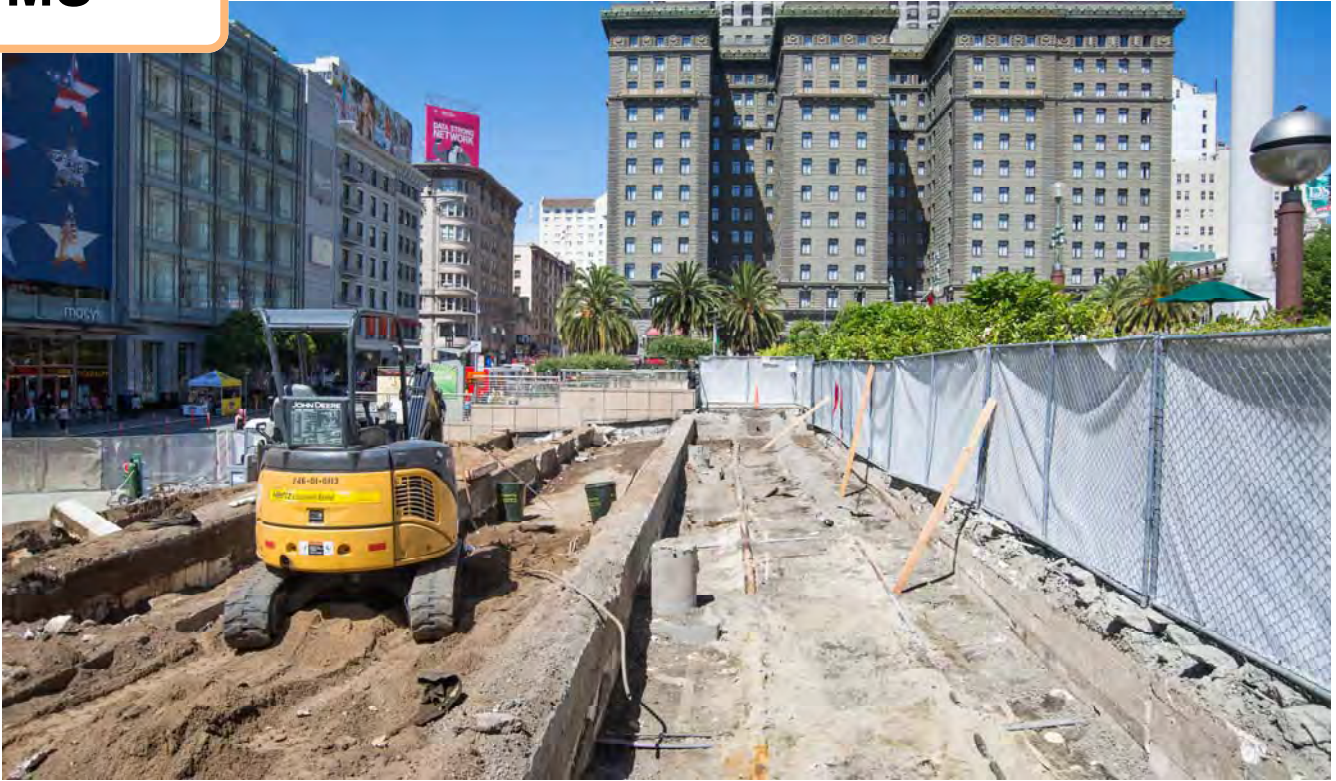
Terrace walls and other decorative elements have been removed from the future north entrance site to the Union Square/Market Street Station at the Union Square Garage.
