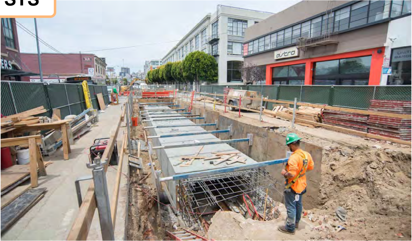
A new, reinforced sewer roof can be seen just south of Bluxome in SoMa.
