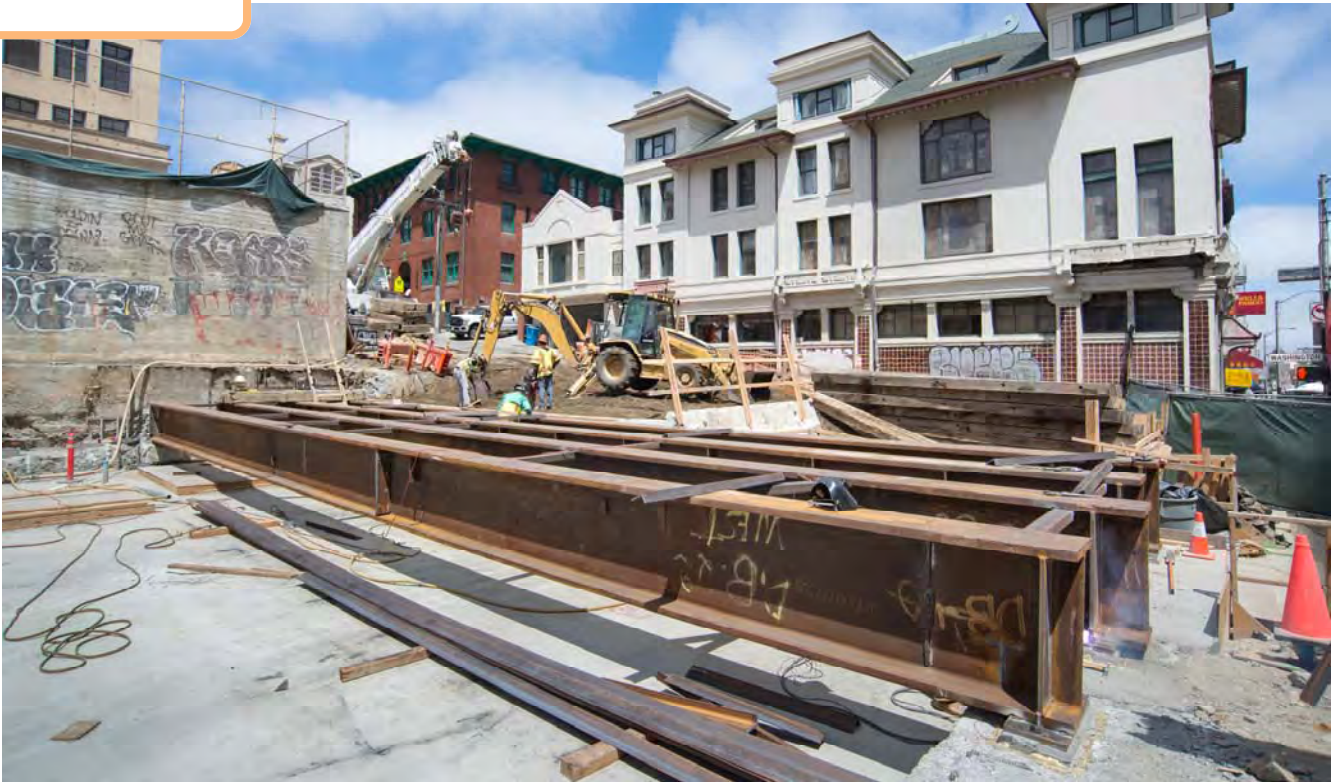
A temporary steel deck can be seen being erected over the finished roof slab of the station headhouse. This will prevent the roof slab from being damaged by vehicle tracks.
