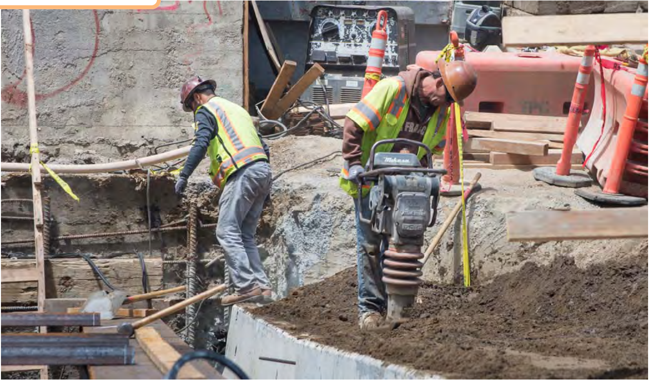
A worker compacts soil accumulated adjacent to a temporary deck being constructed for heavy machinery.
