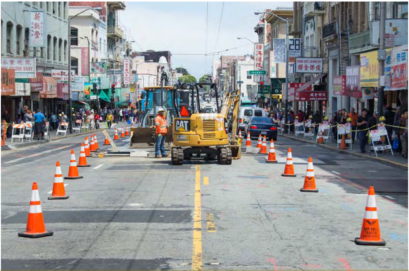
A mini excavator works to assist a crew performing utility relocation efforts on Stockton near Jackson.
