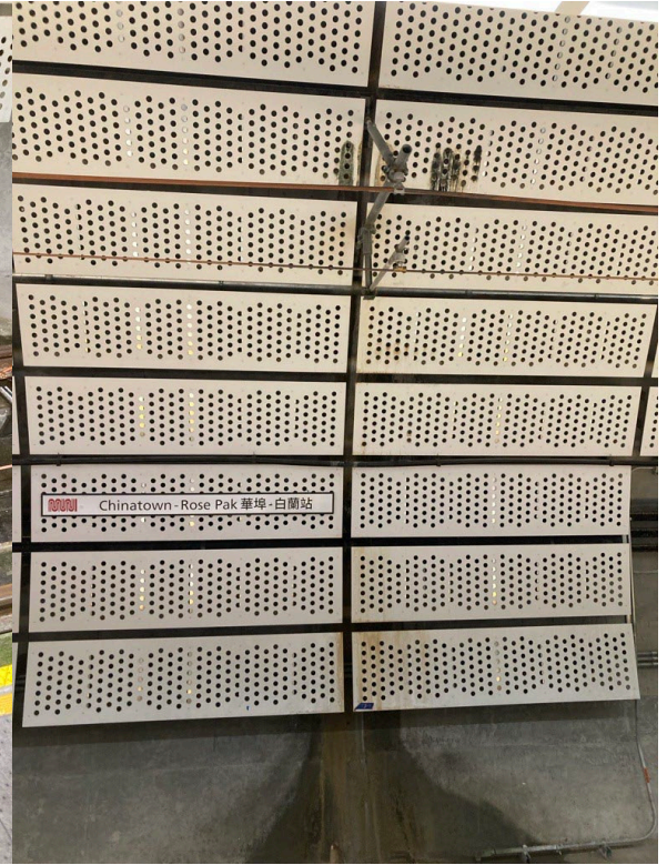
Water Damage on Panel and Fasteners
