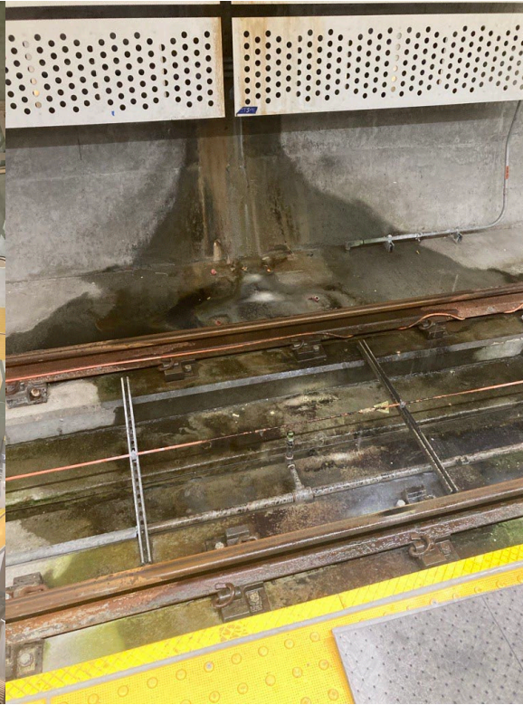
Water Seepage at Joint
