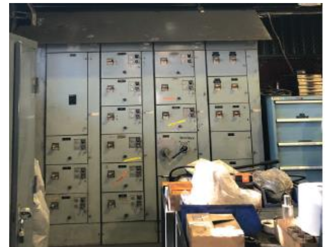
Motor Control Center (MCC)
