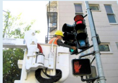
Traffic Signals and Signs
