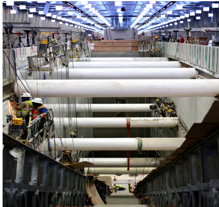
Workers hang from platforms to install panels to escalator walls going from the Concourse Level to the platform
