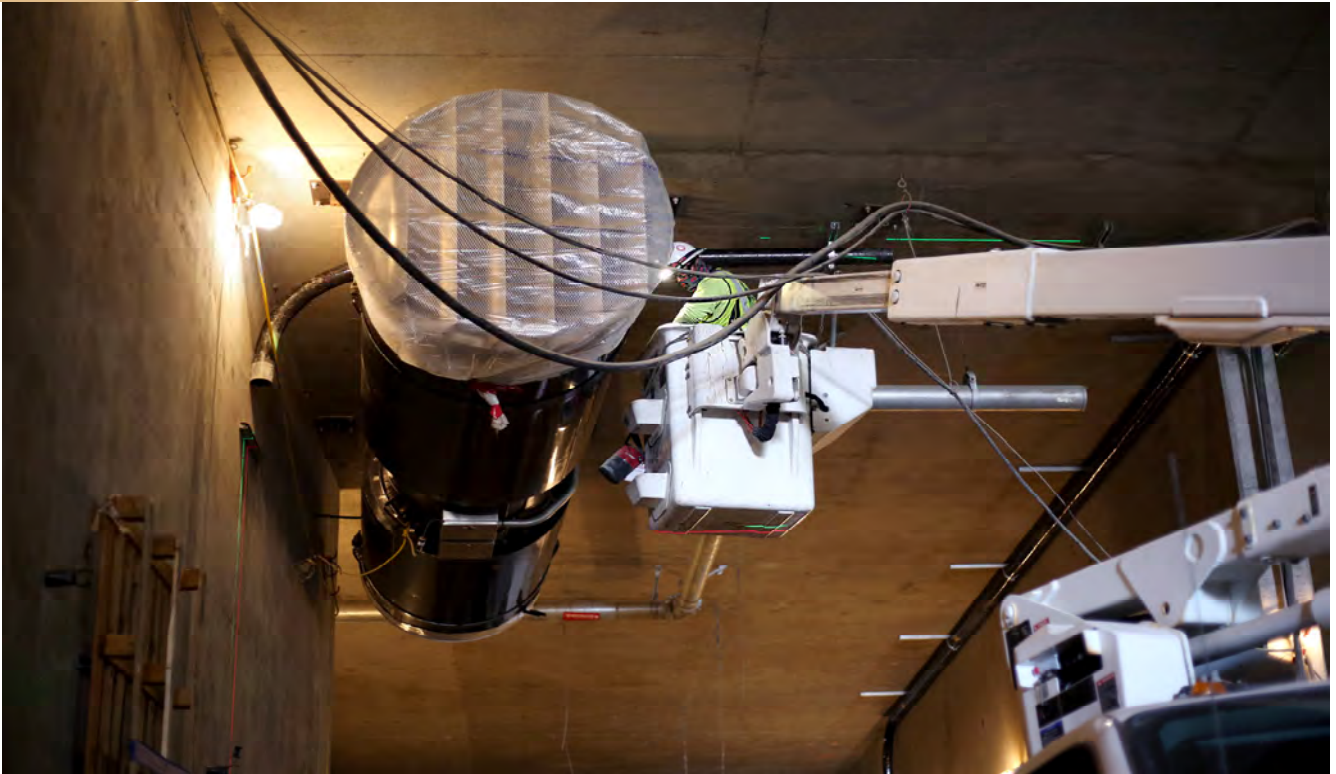
Ventilation jet fans, automatic train control system, OCS, traction power, radio system supports and tunnel signage continue to be installed at tunnel systems portal.
