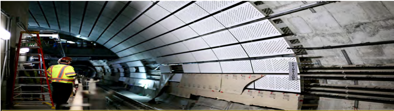
Workers overlook the installation of panels on the platform of Rose Pak-Chinatown Station
