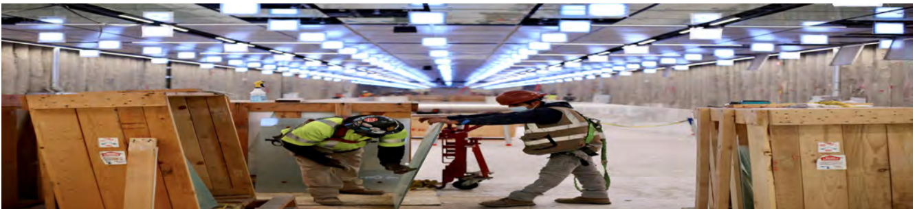
Glass and metal ceiling panels hide utility conduits inside the south concourse ceiling for Union Square/Market Street Station.
