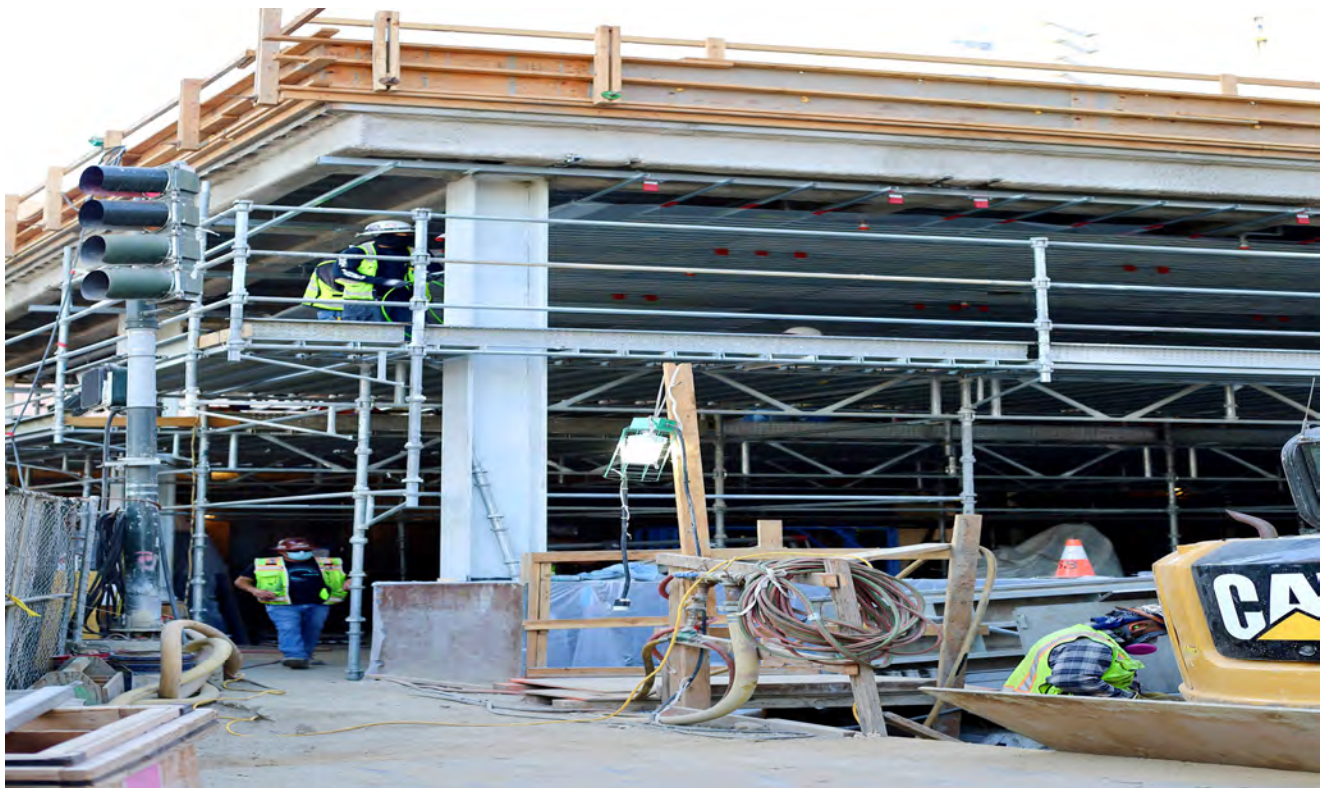
Ceiling panels being placed for the future Rose Pak-Chinatown Station rooftop plaza.
