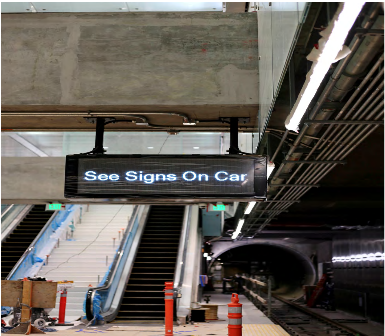
Sign being fixed on concrete structural beam on the north end of Union Square/Market Street Station, where the platform meets the southbound tunnel.
