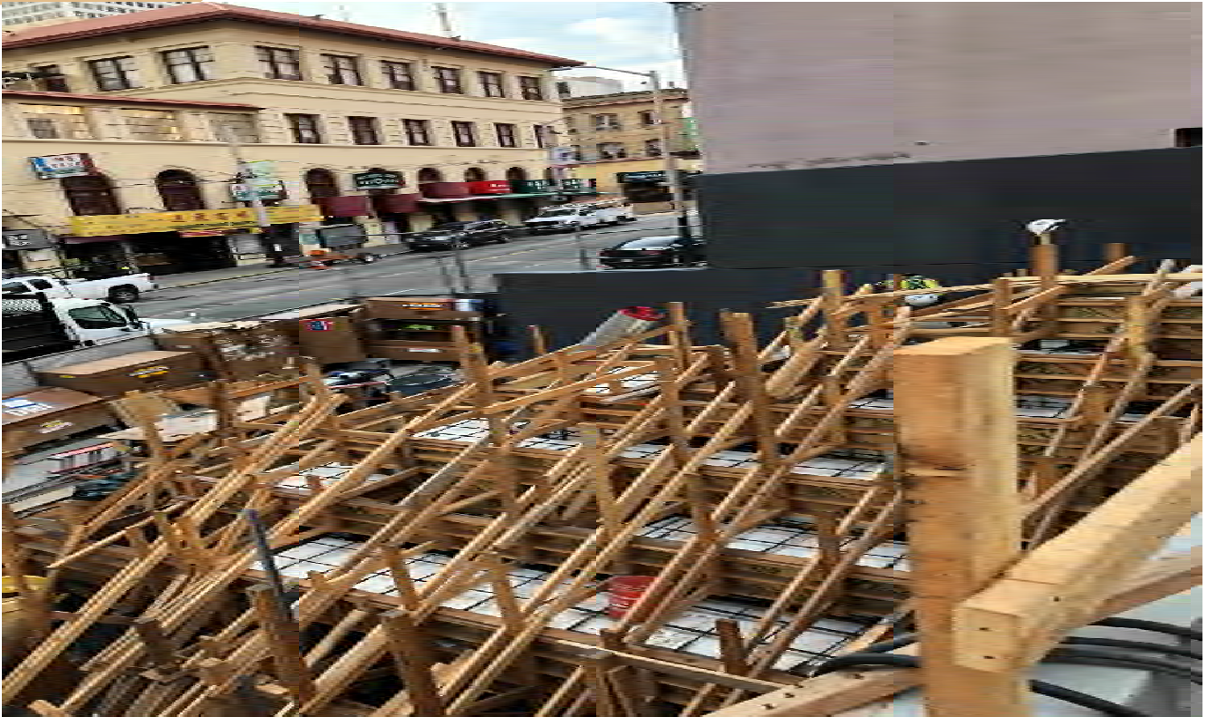
Formwork for the Monument Stairs on the surface of Stockton and Washington
