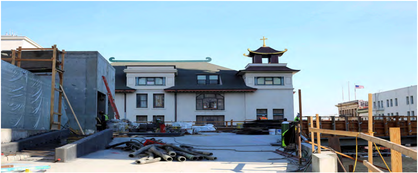
Deck for surface level for Rose Pak-Chinatown Station is being fitted with water proof membrane and being prepped for the concrete pour later that week.
