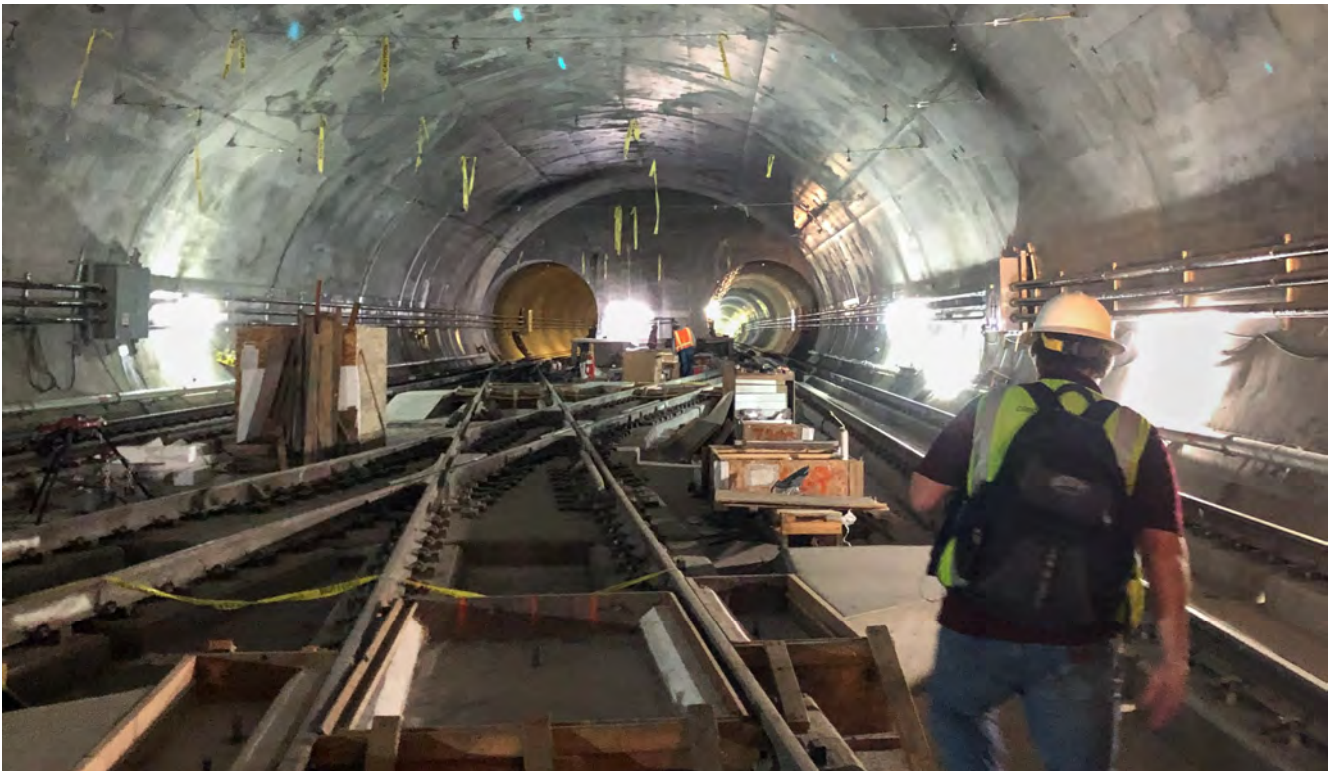
Crews continue building a raised walkway across the switchover tracks inside the cross-over cavern just south of Chinatown Station.
