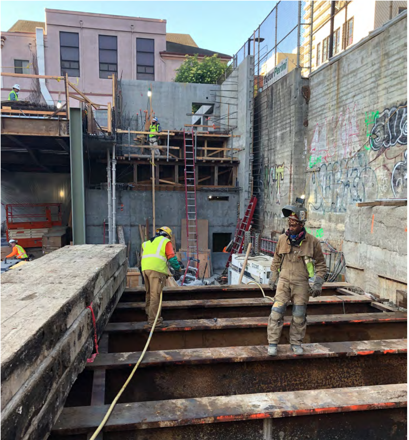
Steel reinforcing used to hold up the former temporary roof deck for Chinatown Station has been removed piece by piece to allow the next portion of the surface entrance structure to be built.
