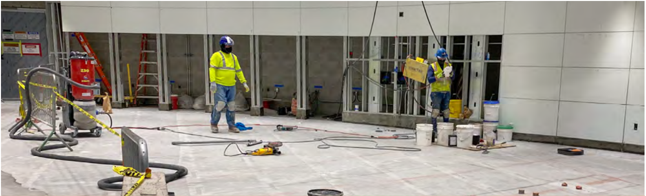
Adhesive matting has been rolled out and placed inside the Union Square/Market Street Station north concourse area ahead of pouring the first layer of terrazzo floor base.
