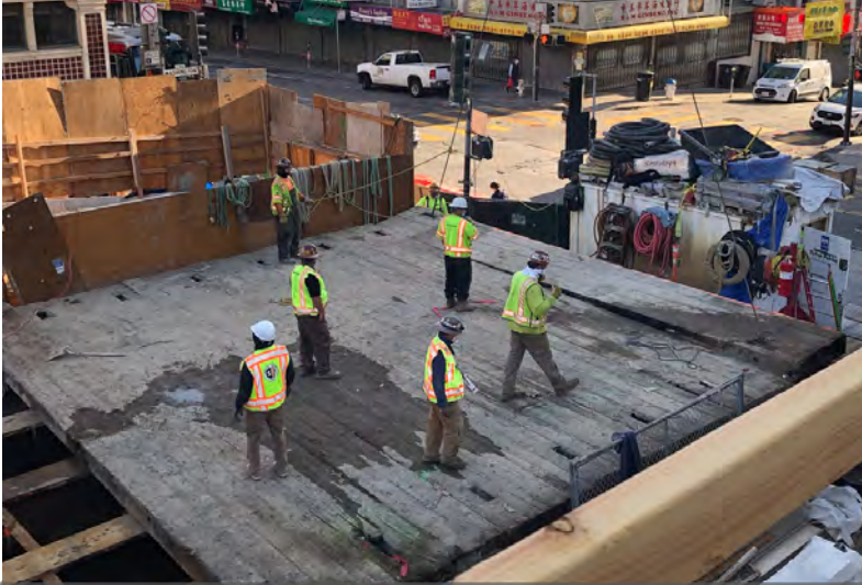
The area is cleared and sections of wood cribbing atop the structural beams are removed one piece at a time.
