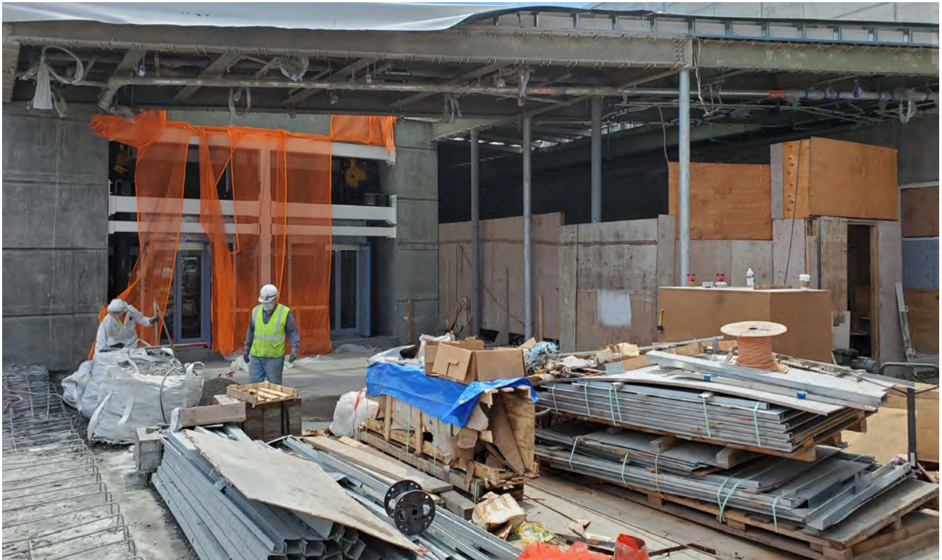
Framing, wall panels, and other materials slated for the station interior are staged in the future entrance plaza for Yerba Buena/Moscone Station.
