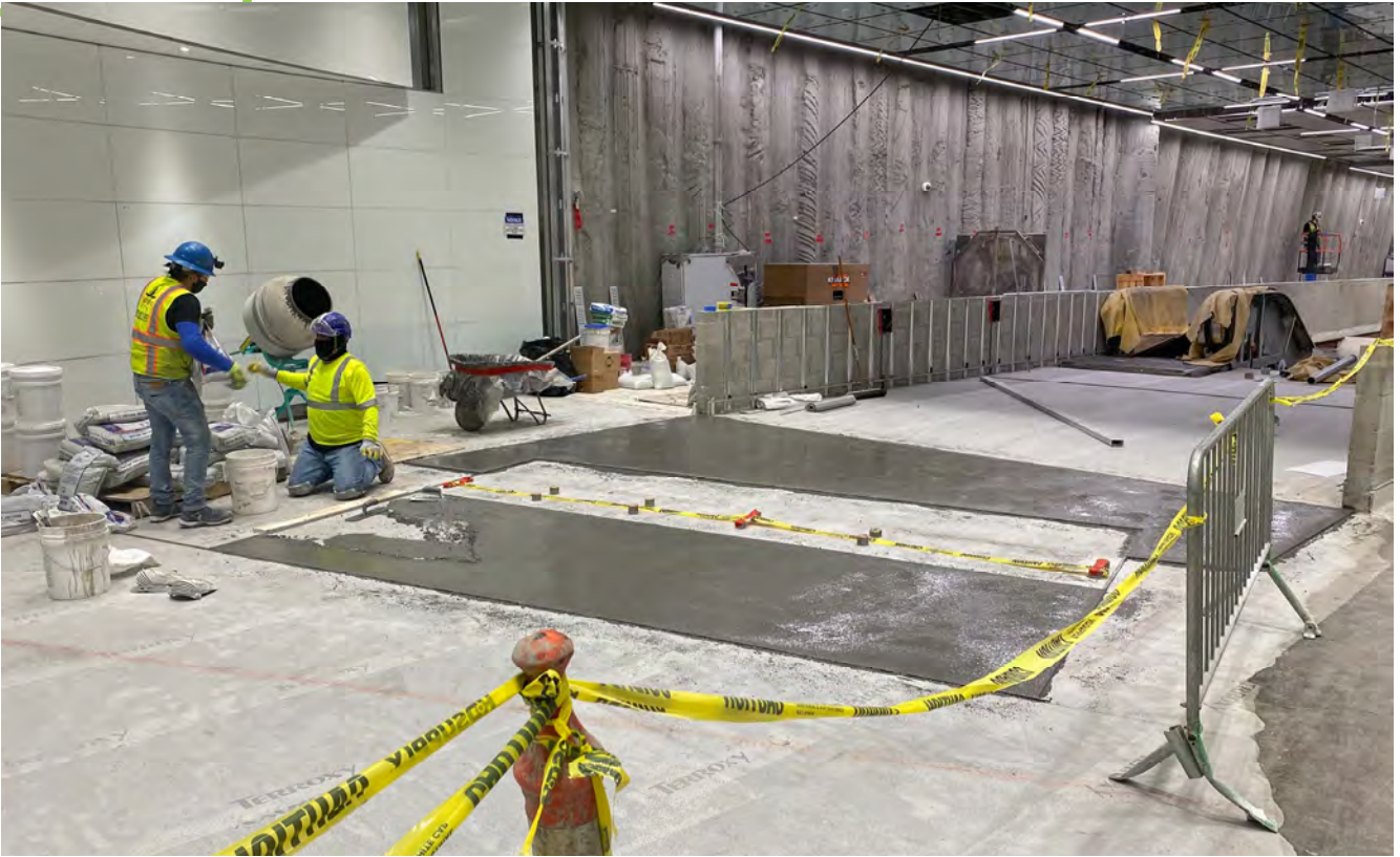
Alternating sections of dark floor shapes being poured will lead the way to the north escalators inside the Union Square/Market Street Station north concourse.
