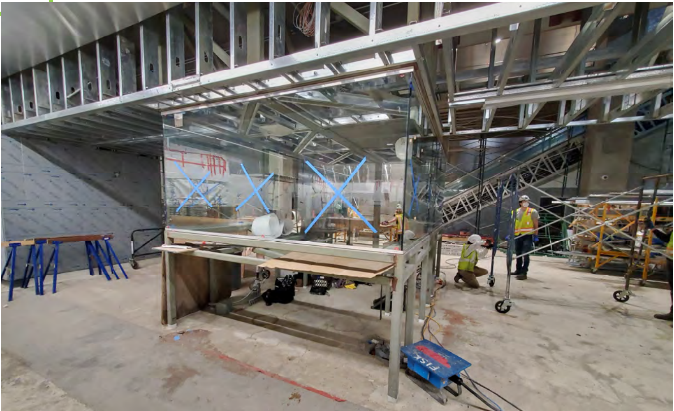
With steel framing and glass windows now in place, the future station attendant booth is coming together inside the Yerba Buena/Moscone Station concourse lobby.
