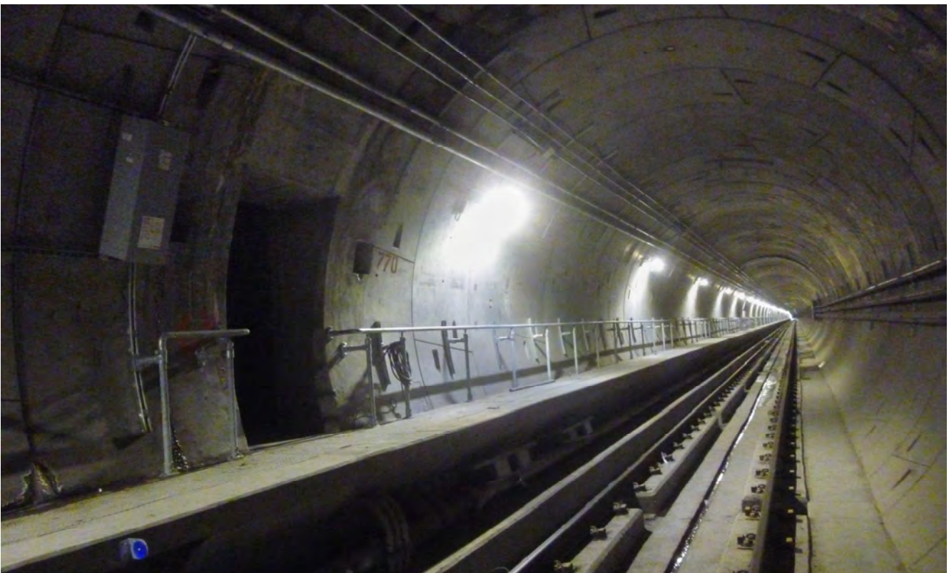
Steel railings have been installed along the raised walkway inside the northbound tunnel, seen here near a cross-passage just north of Union Square/Market Street Station.
