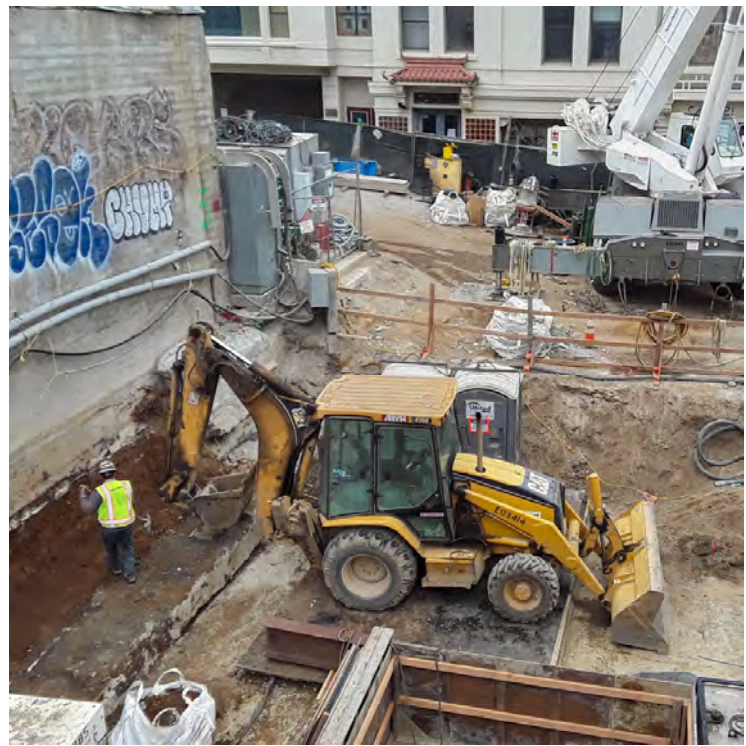
Additional materials are removed, the area is cleared, and the site is prepared to build the next section of the steel-level station entrance structure.
