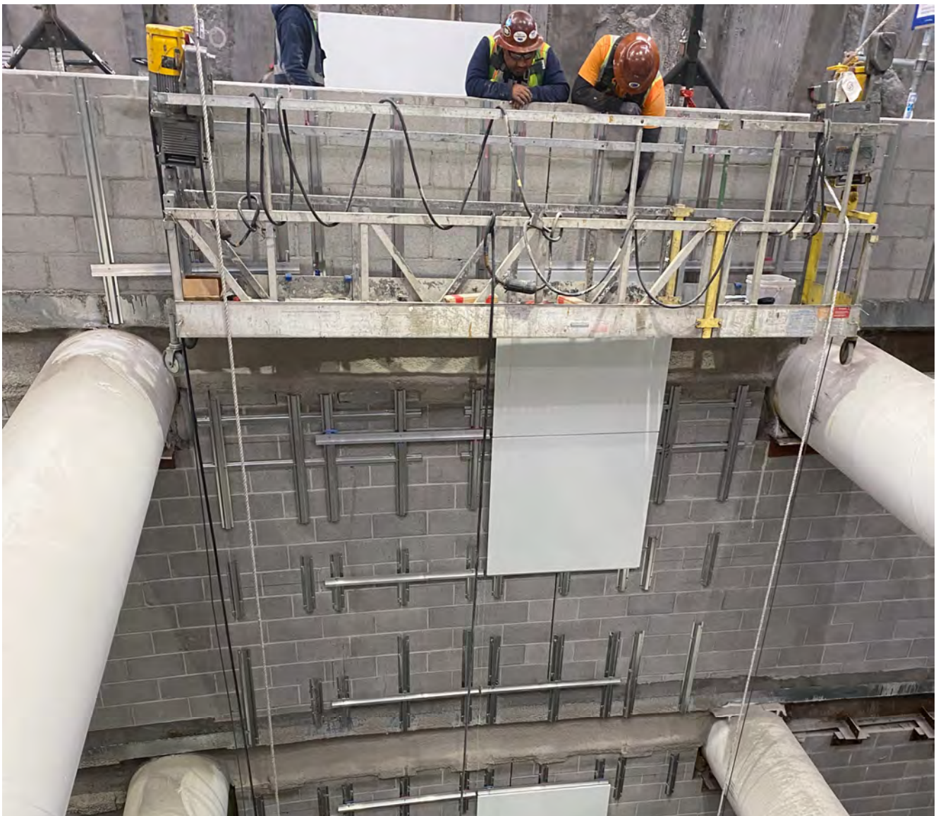
Mounting brackets and white wall panels have been going in surrounding the north stairs and escalators inside Union Square/Market Street Station.
