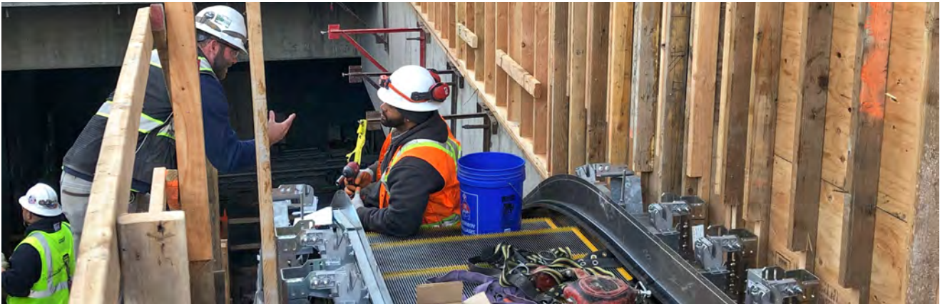
Workers discuss particulars during escalator assembly at the street level entrance for Chinatown Station.
