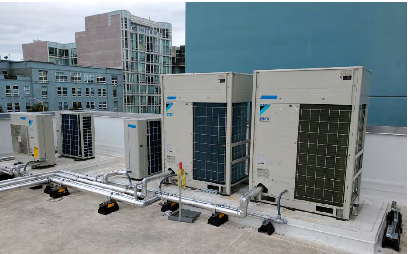
Air conditioners and other systems have now been installed, with these units placed atop the Yerba Buena/Moscone Station headhouse roof.
