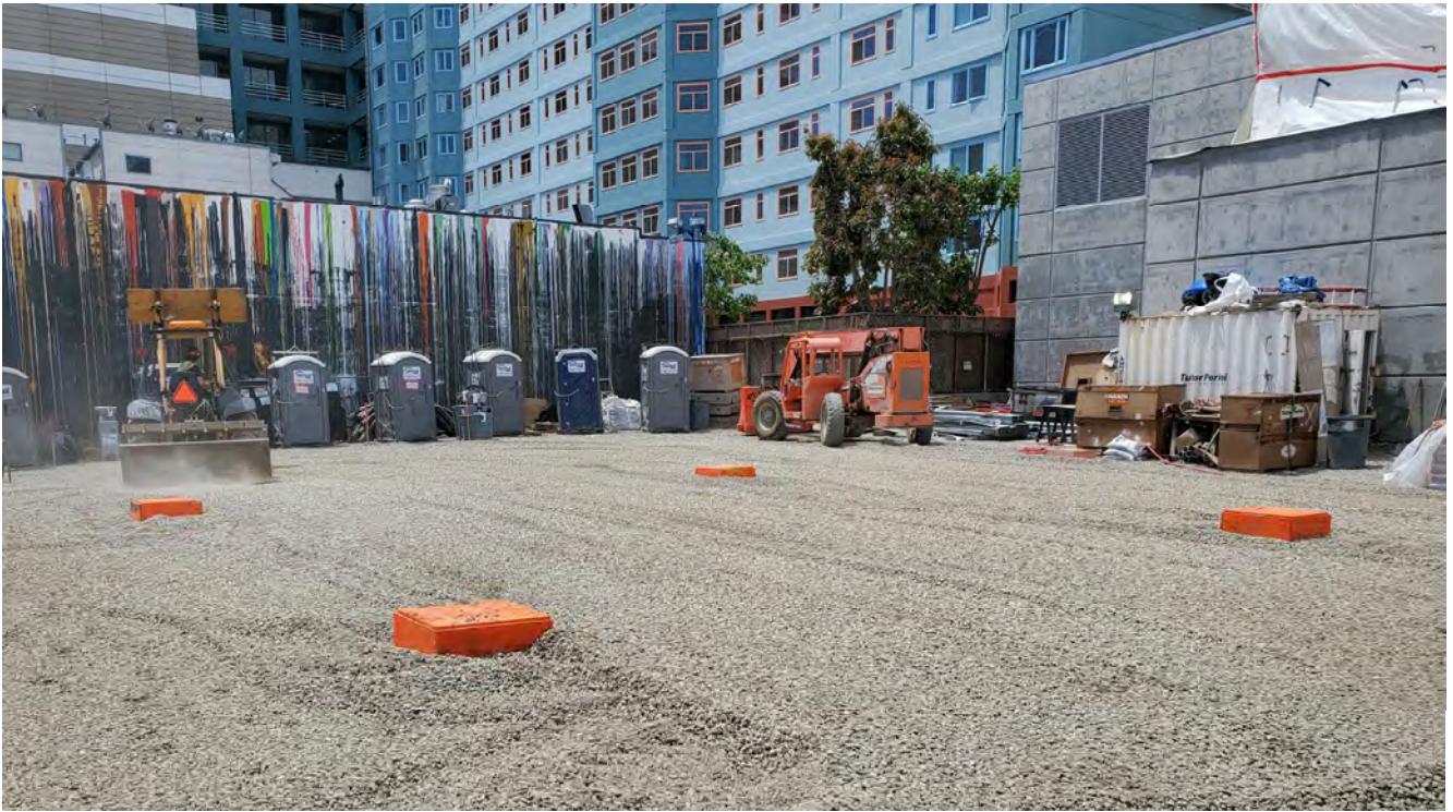
Supplies and equipment have been temporarily cleared from the site atop the southern half of the Yerba Buena/Moscone headhouse roof so crews can grade a layer of gravel.
