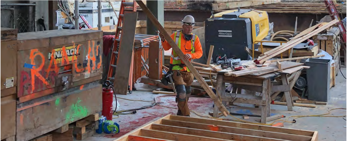
A carpenter assembles wood framing for a future concrete form atop the Chinatown Station headhouse.
