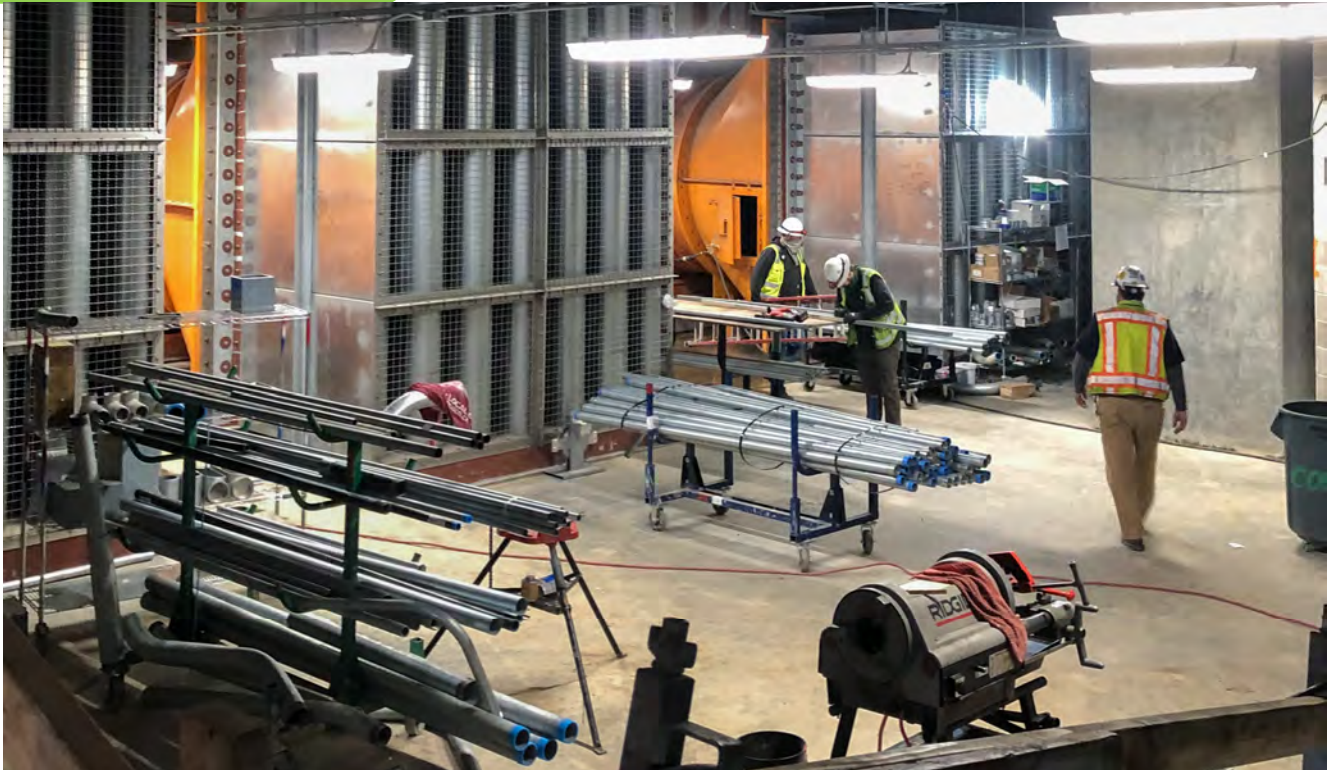
HVAC systems, large diameter conduits, and massive fans have been installed for inside the lower level of Chinatown Station's headhouse structure.
