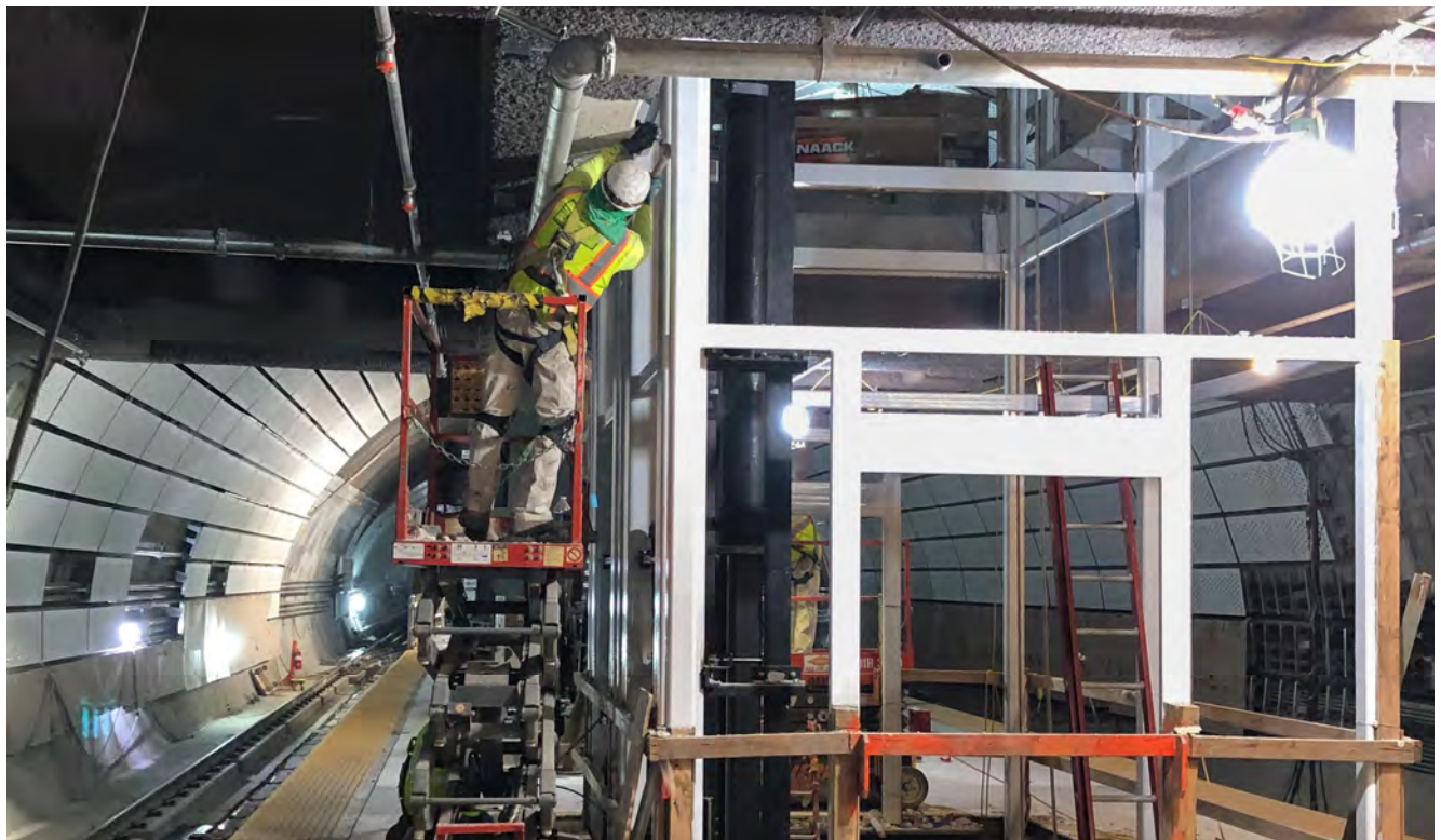
Steel framing for Chinatown Station's concourse-to-platform elevators has been constructed, and workers have begun building out the elevators themselves.
