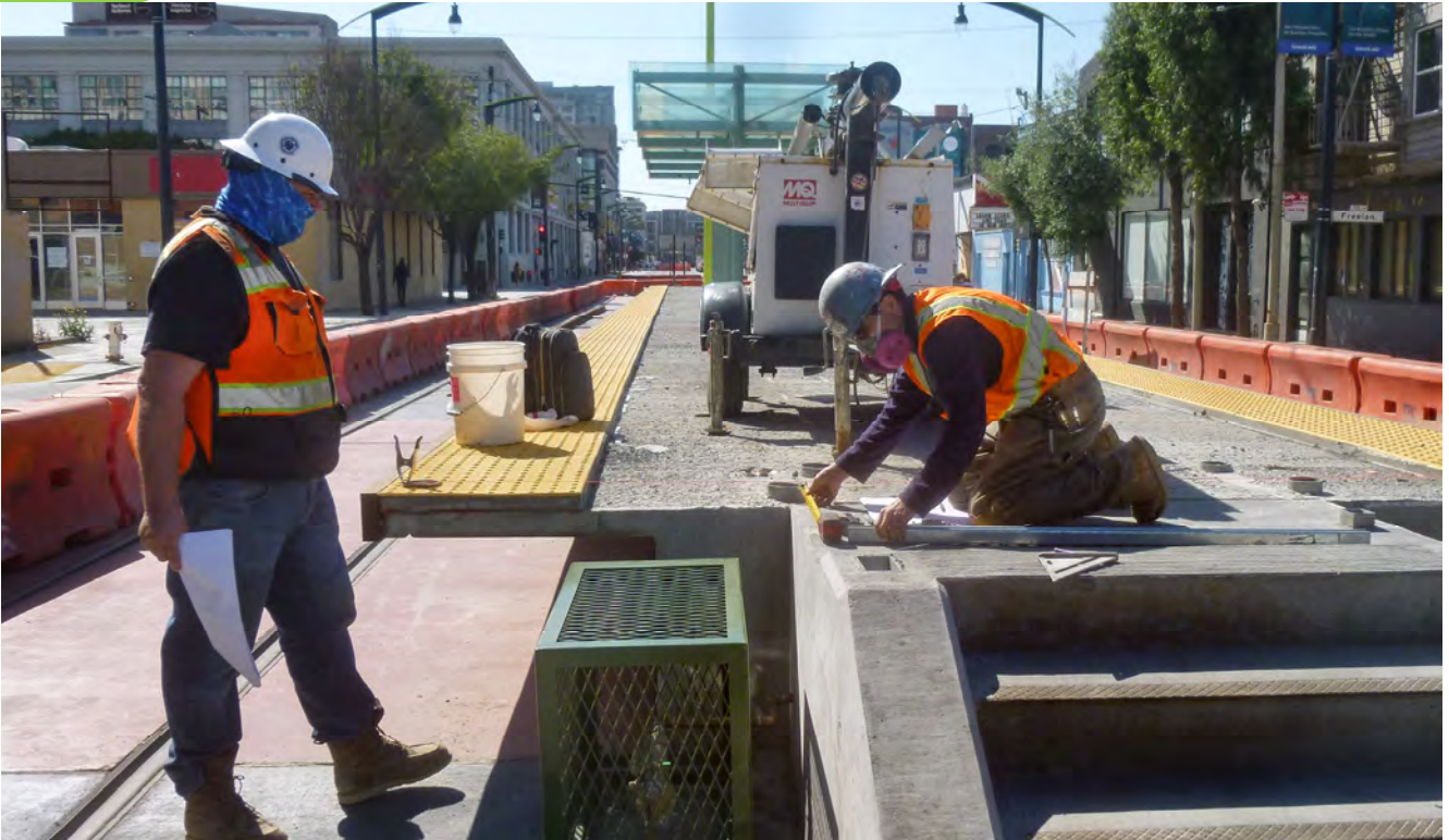
Two workers go over plans to build steel brackets for mounting utilities at the 4th and Brannan surface station platform.
