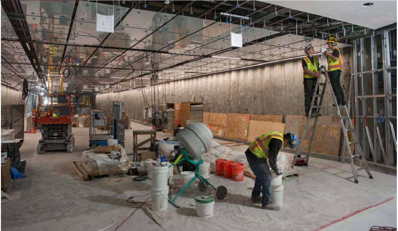
Glass ceiling panels and an LED array are being installed inside the south concourse for Union Square/Market Street Station. The LED panels will be a public art piece by Erwin Redl called Lucy in the Sky .
