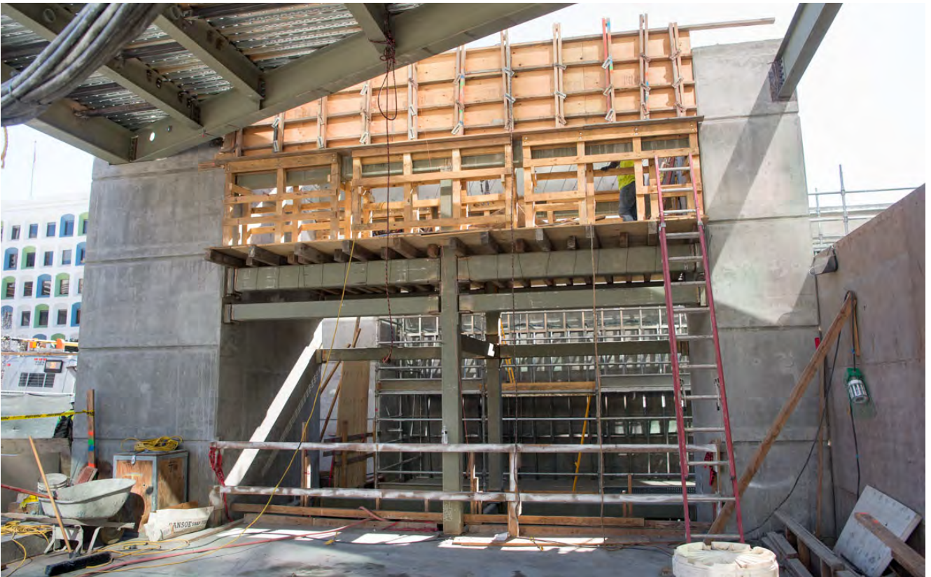
Steel framing and other structural elements are being installed as part of surface-to-concourse elevator shaft construction for Yerba Buena/Moscone Station.
