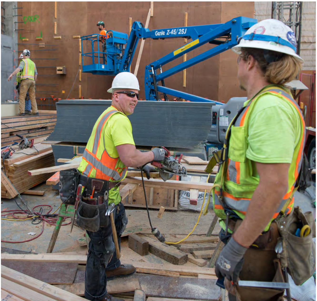
Carpenters build concrete forms near the south end of the Chinatown Station surface worksite.
