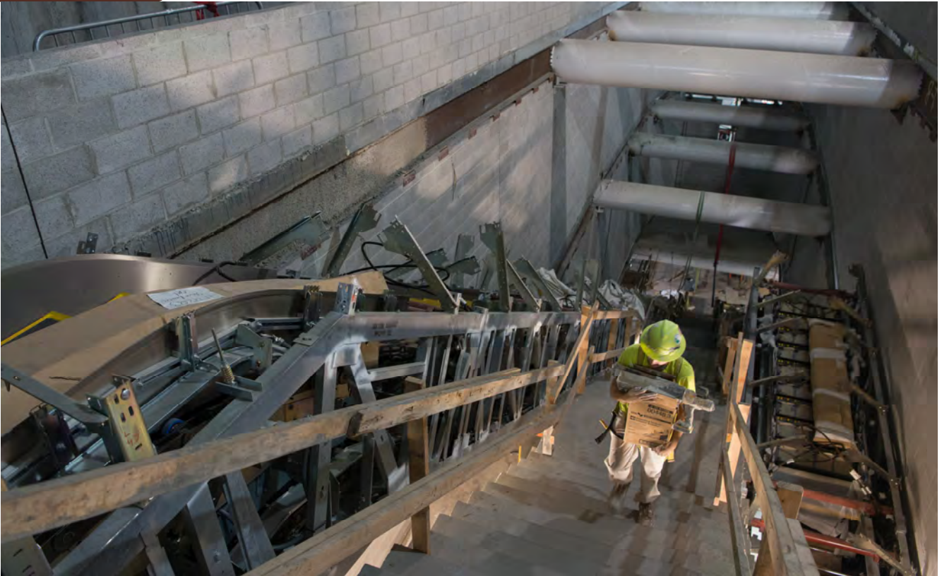
A worker carries supplies up the long flight of stairs at the north end of the Union Square/Market Street Station, where escalators are being installed.
