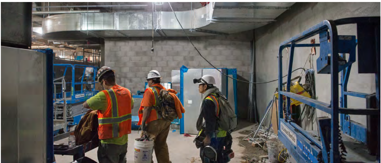
A crew carries gear and equipment past recently-installed HVAC ductwork on the platform level of the Chinatown Station headhouse.
