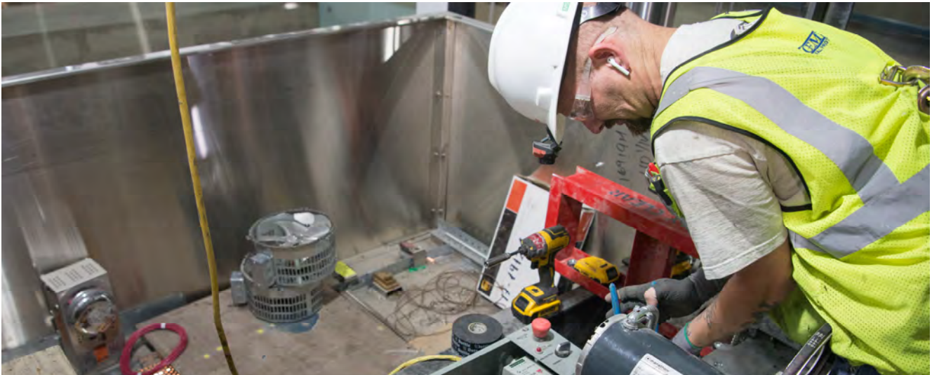
A technician works to assemble machinery for the north concourse-to-platform elevator inside Yerba Buena/Moscone Station.
