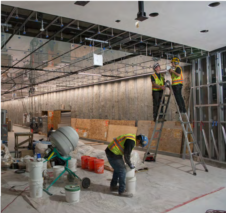
Workers attach glass panels and LED squares, part of the public art program.
