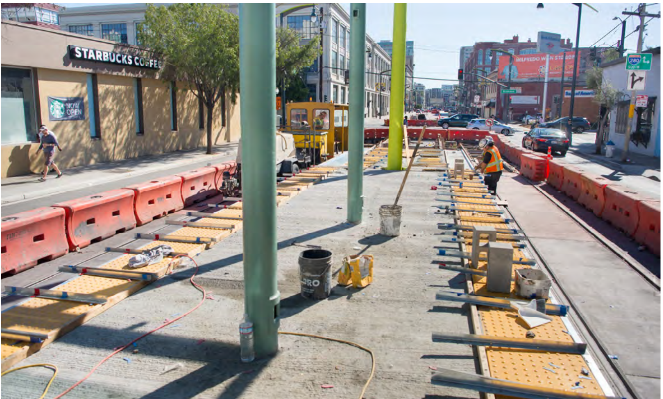
Crews have installed tactile paving tiles at the edges of the 4th and Brannan surface platform, to help the visually impaired know where the edge of the platform is.
