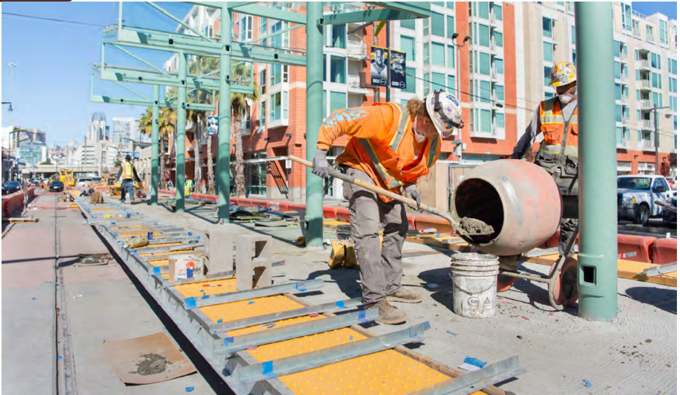
Concrete is mixed on site to build a small staircase at the north end of the 4th and Brannan surface platform, in addition to other structural work being finished there.
