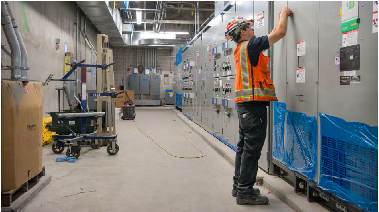
A worker tightens bolts on a panel inside the lowest level of Yerba Buena/Moscone Station, where many systems and utilities hum away.
