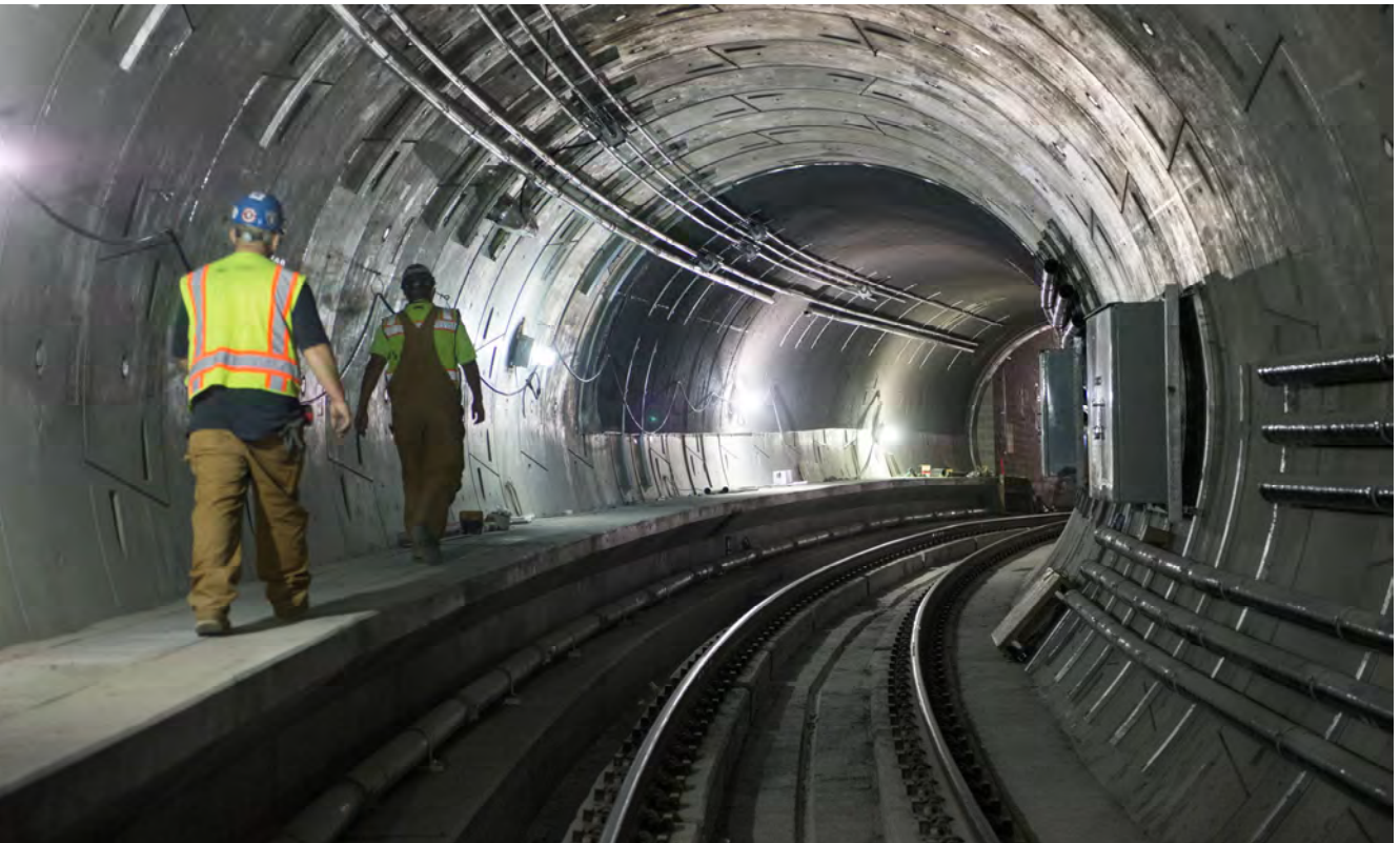
Workers walk north up the northbound tunnel S-curve underneath the Market Street Subway, where one can faintly hear BART trains pass overhead.
