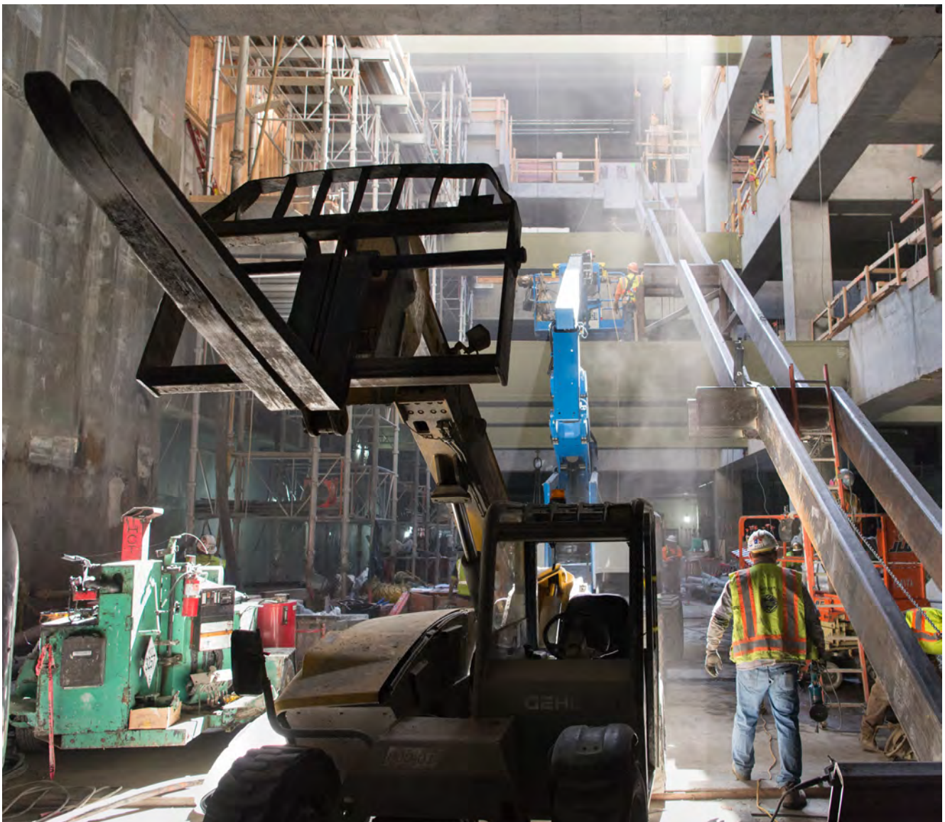
Looking south inside the concourse level for Chinatown Station's headhouse, light pours in the main access shaft adjacent to steel framing being assembled to reinforce a future staircase.
