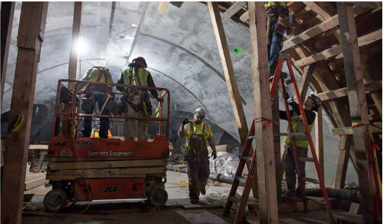
A crew builds massive, arched concrete forms at the entrance to the cross-cut cavern leading into the Chinatown Station platform cavern.
