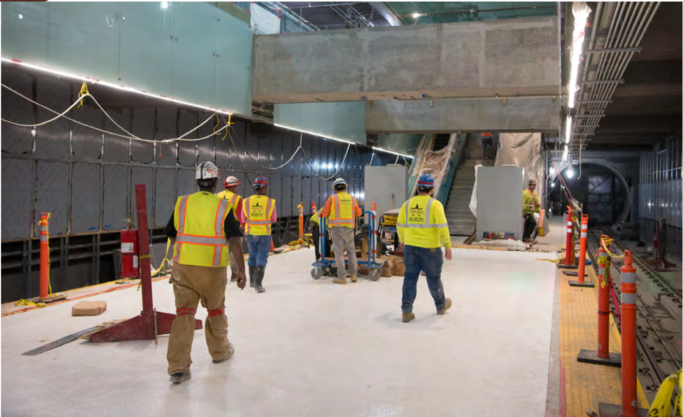
A layer of white terrazzo has been poured down the length of the platform for Yerba Buena/Moscone Station.
