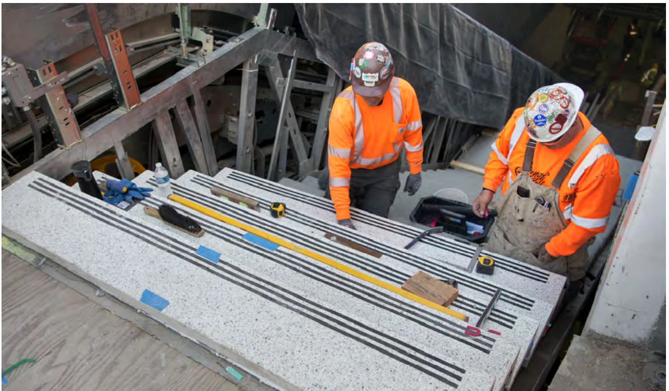
Slick-resistant terrazzo steps are being installed at the north entrance for Union Square/Market Street Station, inside the entrance structure nestled into the southeast corner of the square.
