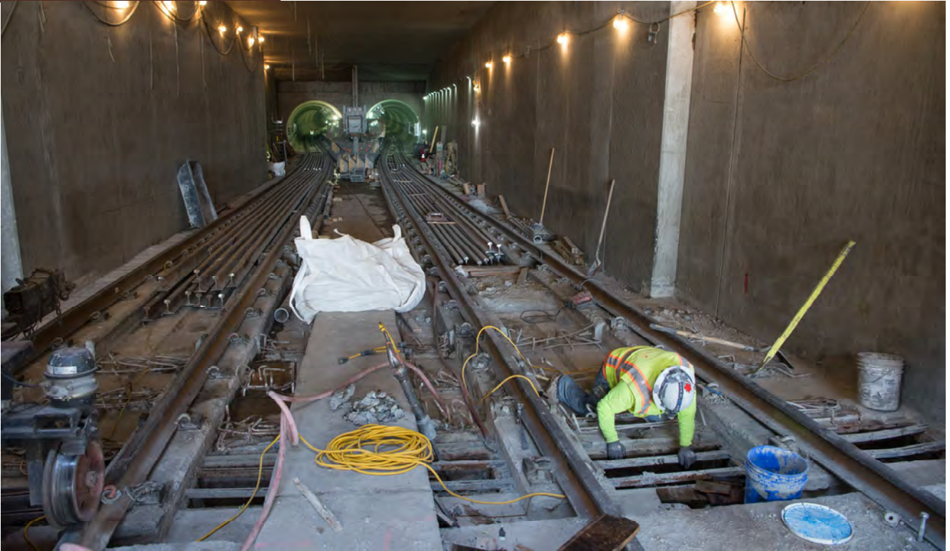
A trench at the entrance ramp of the 4th Street tunnel portal is looked over and cleaned out and rebuilt.
