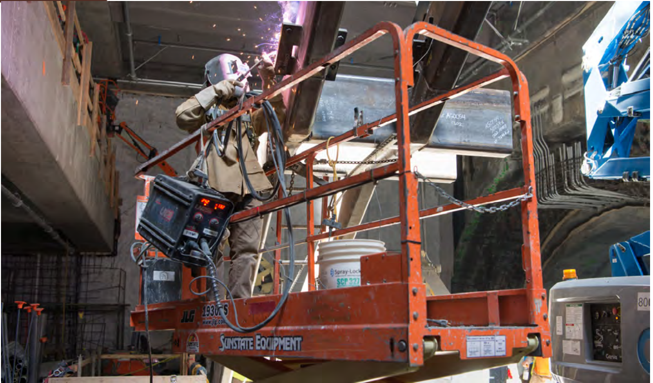
A welder attaches steel brackets to framing poised to carry the main staircase from the surface into the concourse level of Chinatown Station's headhouse.
