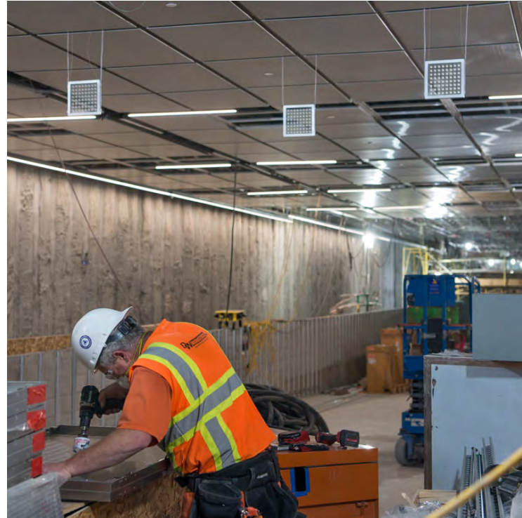
Electrical and communications systems are integrated into the public art installation.
