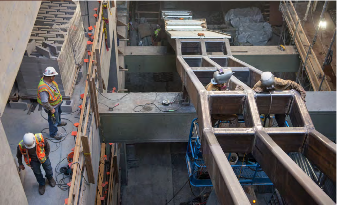
Heavy duty steel reinforcing is being welded in place to support a future staircase leading from the upper mezzanine level down to the future station lobby for Chinatown Station.
