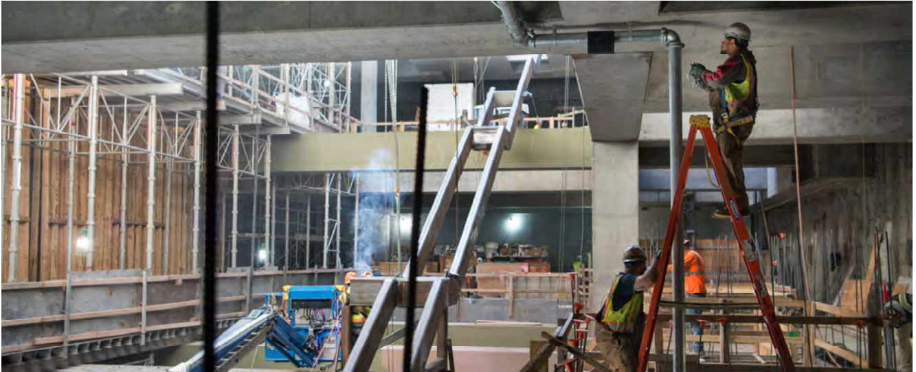
Workers install piping which will become part of a fire suppression system on level five above the concourse for Chinatown Station.
