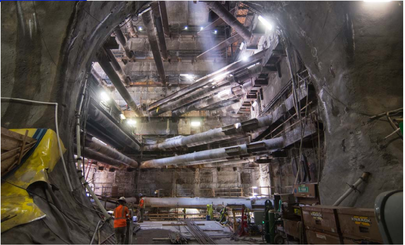
Light beams through a roof deck access shaft looking west from the cross-cut cavern into the Chinatown Station headhouse.
