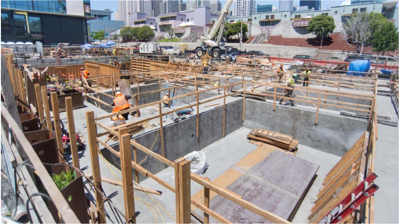
The southern half of the Yerba Buena/Moscone Station headhouse roof slab was recently poured, and concrete forms were removed soon after.
