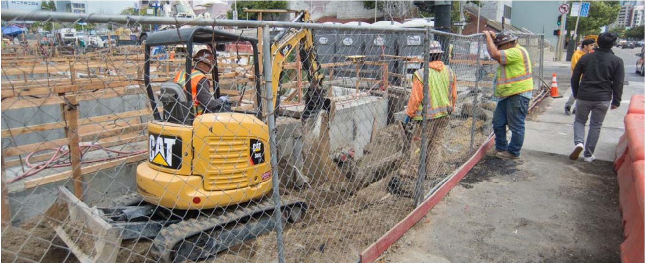
Workers remove unneeded formwork and reinforcing from along the southern edge of the Yerba Buena/ Moscone Station headhouse at Folsom and 4th.
