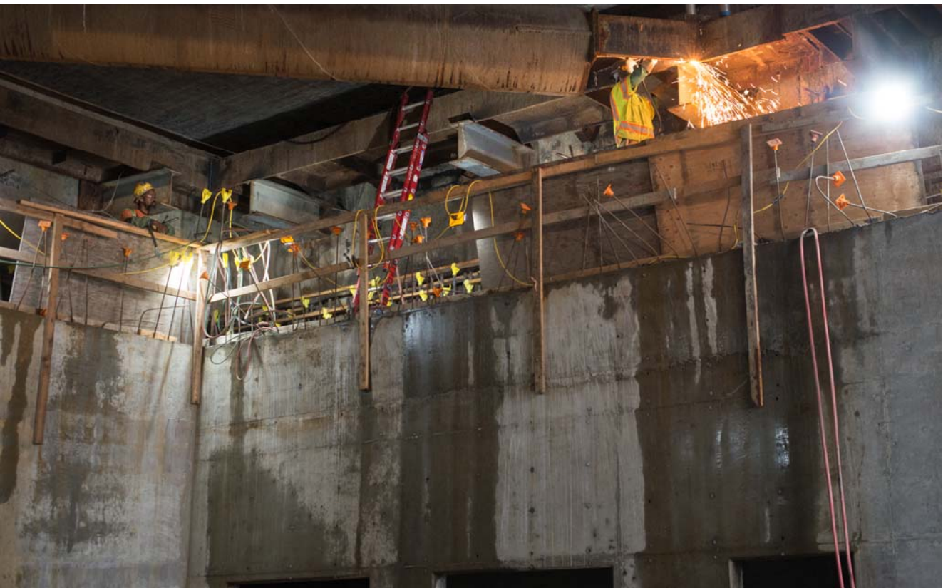
Now that the southern half of the Yerba Buena/Moscone Station headhouse roof slab has been constructed, temporary steel bracing at the south end of the headhouse can be removed.
