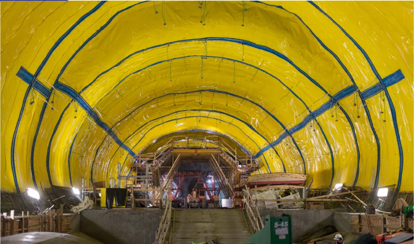
Yellow waterproofing and blue gasket strips line the length of the Chinatown track cross-over cavern, looking south.
