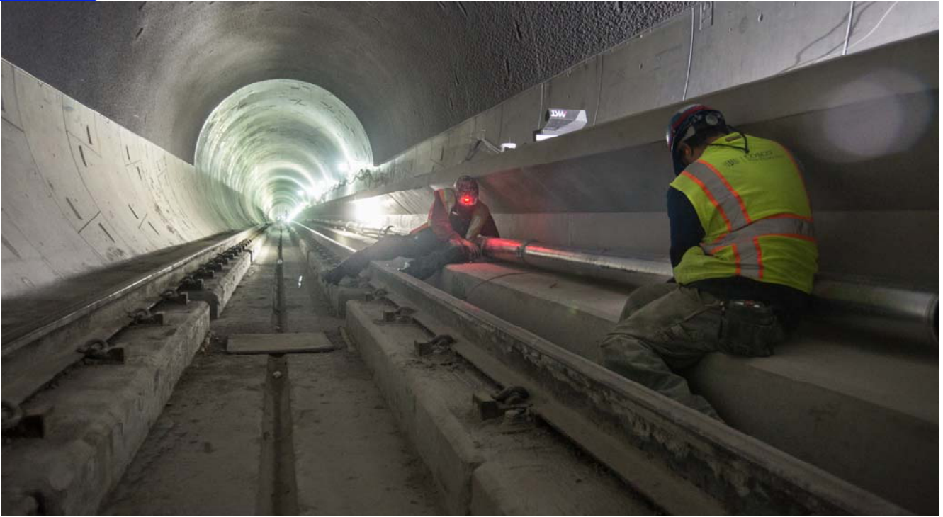
Two men attach a section of large utility conduit to the base of the tunnel emergency walkway inside the southbound tunnel.
