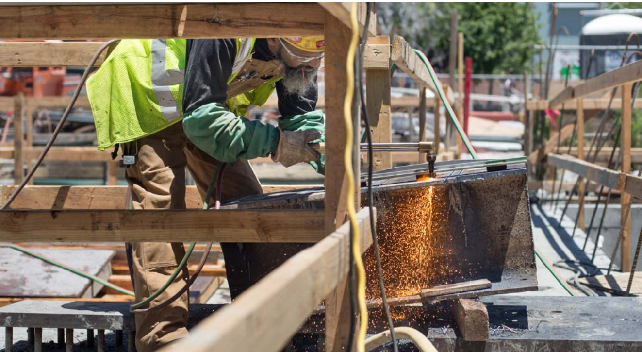
An ironworker uses a guide and cutting torch to fabricate brackets atop the Yerba Buena/Moscone Station headhouse roof slab.
