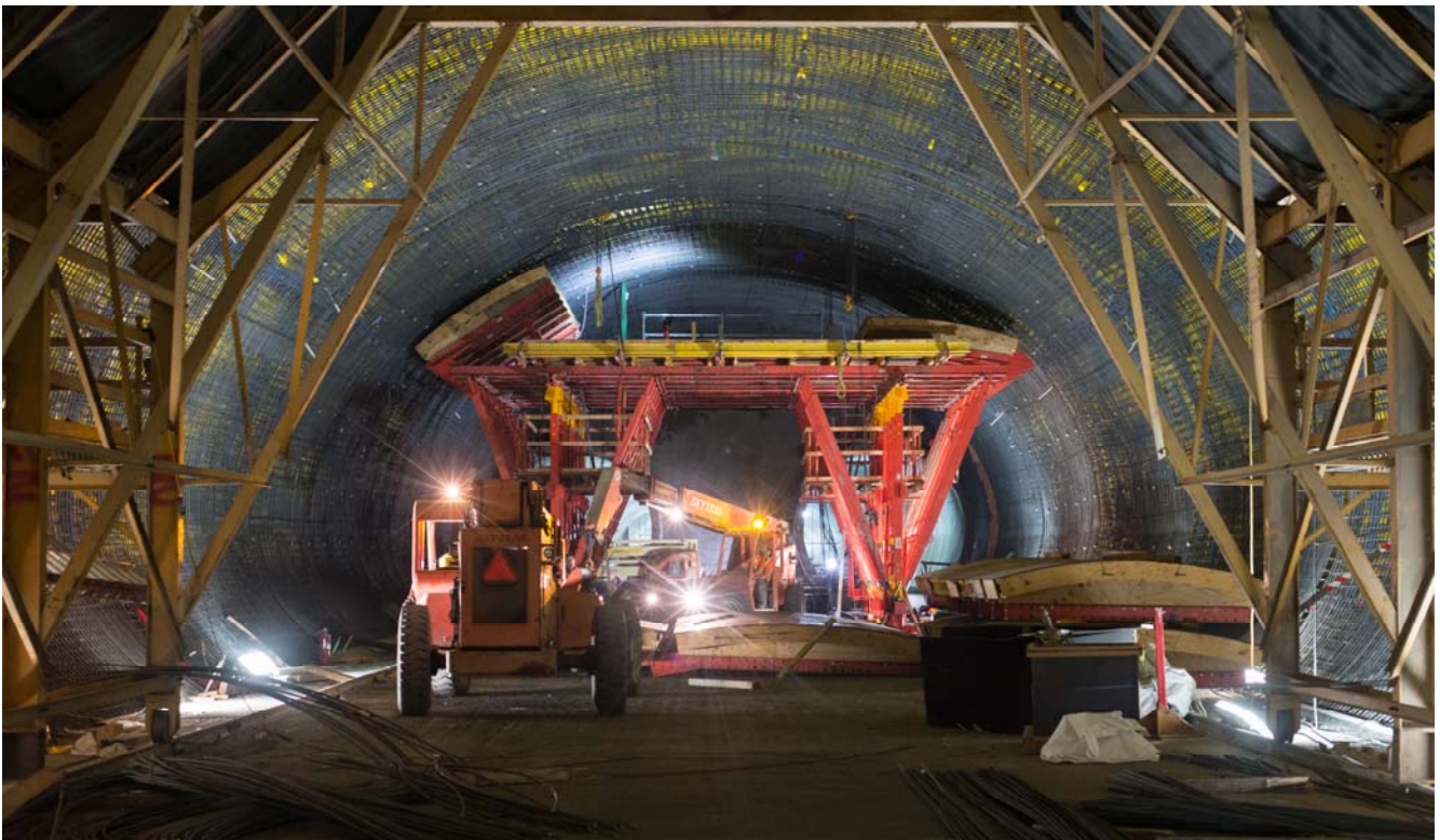
Looking south inside the Chinatown track crossover cavern, curved formwork can be seen partially installed in a huge, rolling truss structure prior to pumping in concrete to build the inner structural shell of the cavern.
