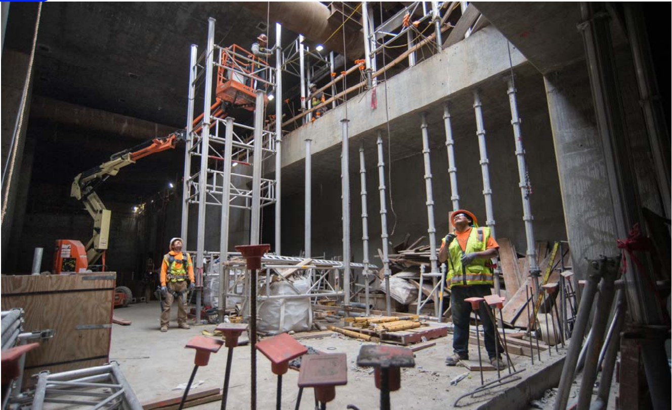
A crew inside the concourse level of the station headhouse coordinates by radio with a crane operator at the surface to receive a box of supplies.
