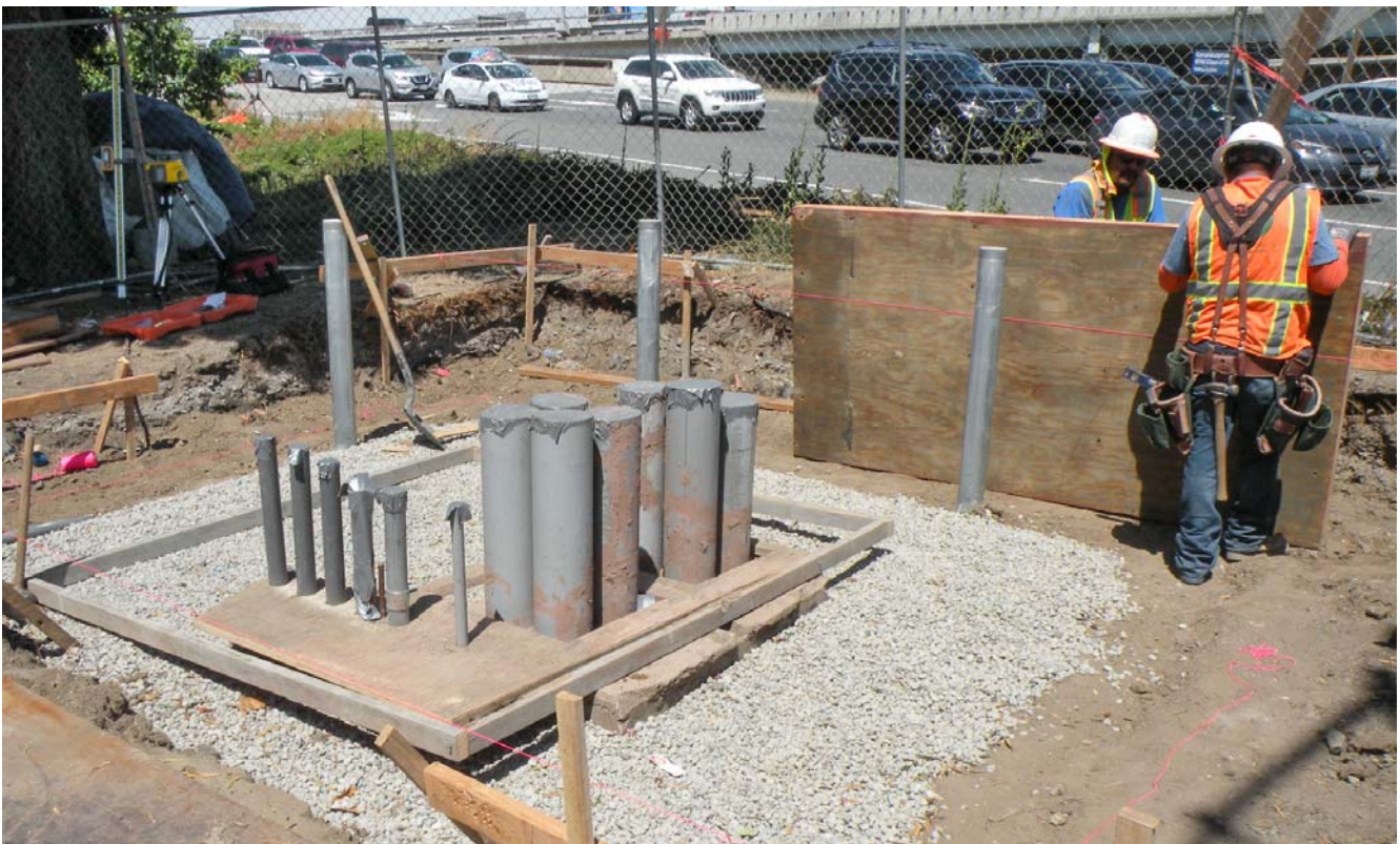
Workers construct concrete forms prior to pouring the slab of a sectionalizing breaker panel near the end of the 4th Street ramp of I-80.
