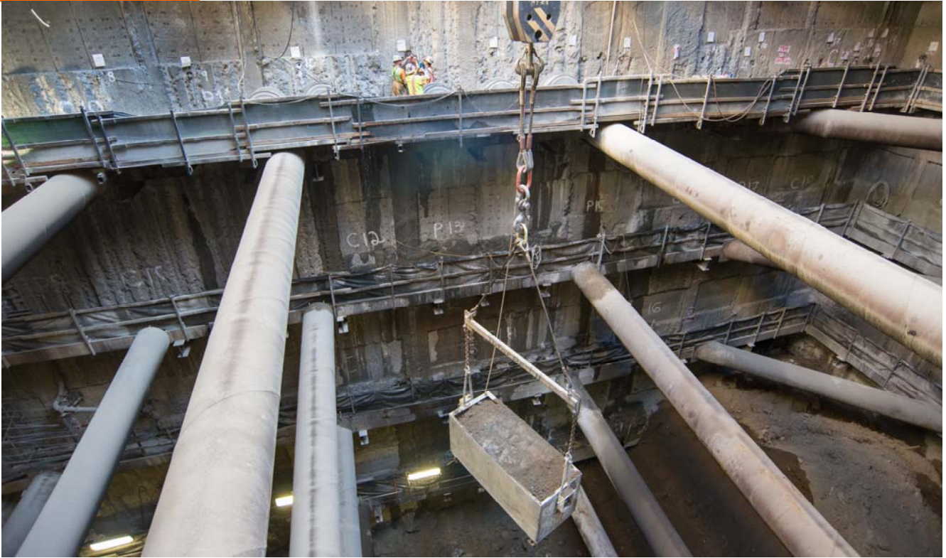
The massive steel bucket used to haul excavated material out of the Chinatown Station headhouse slowly makes its way to the surface.
