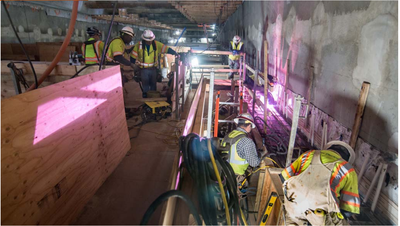
A rebar cage and concrete forms are constructed around existing walers on the west wall of the station box, prior to pouring concrete.
