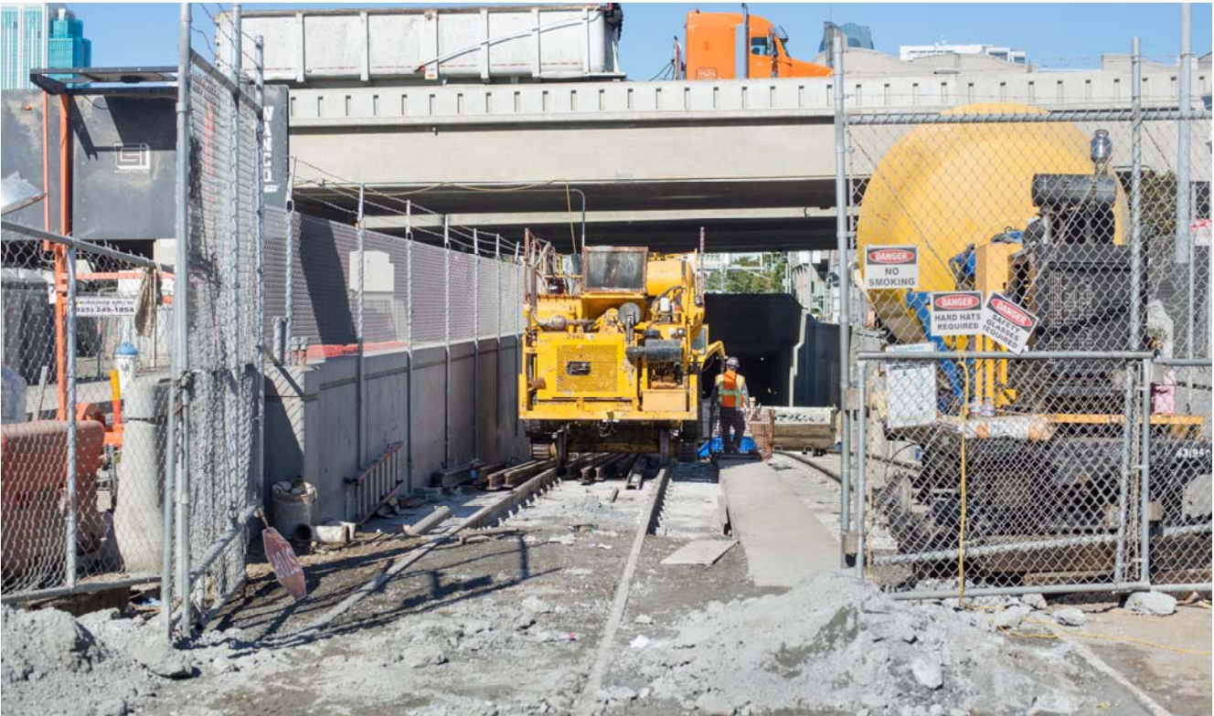
Specialized rail cars have been rolled onto existing tracks inside the tunnel portal structure, to aid rail installation and concrete pouring inside the tunnels further north.
