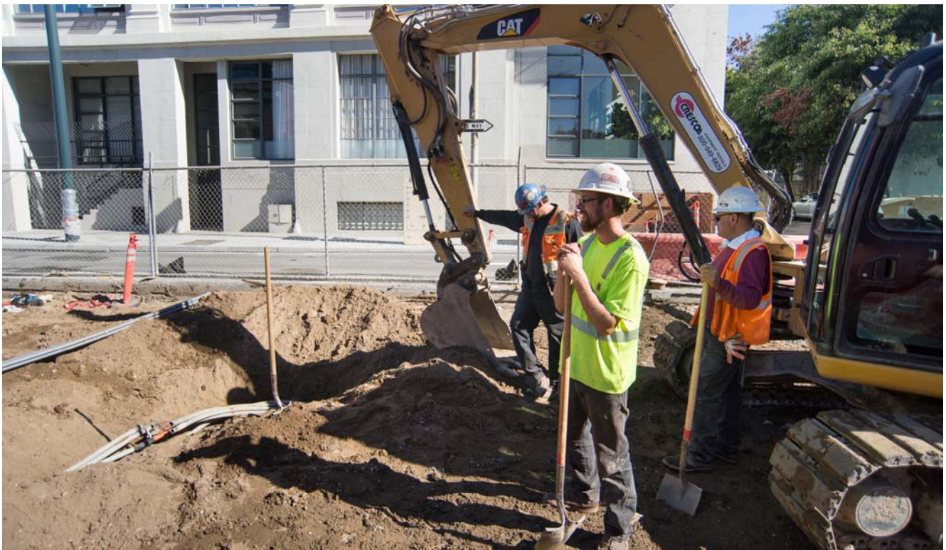
A crew pauses for a moment to wait for equipment to move during utility upgrade work near 4th and Bluxome.
