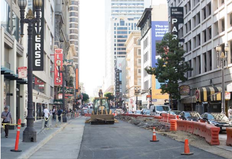
1 Traffic is moved to the north side of Ellis while the south side is rebuilt
