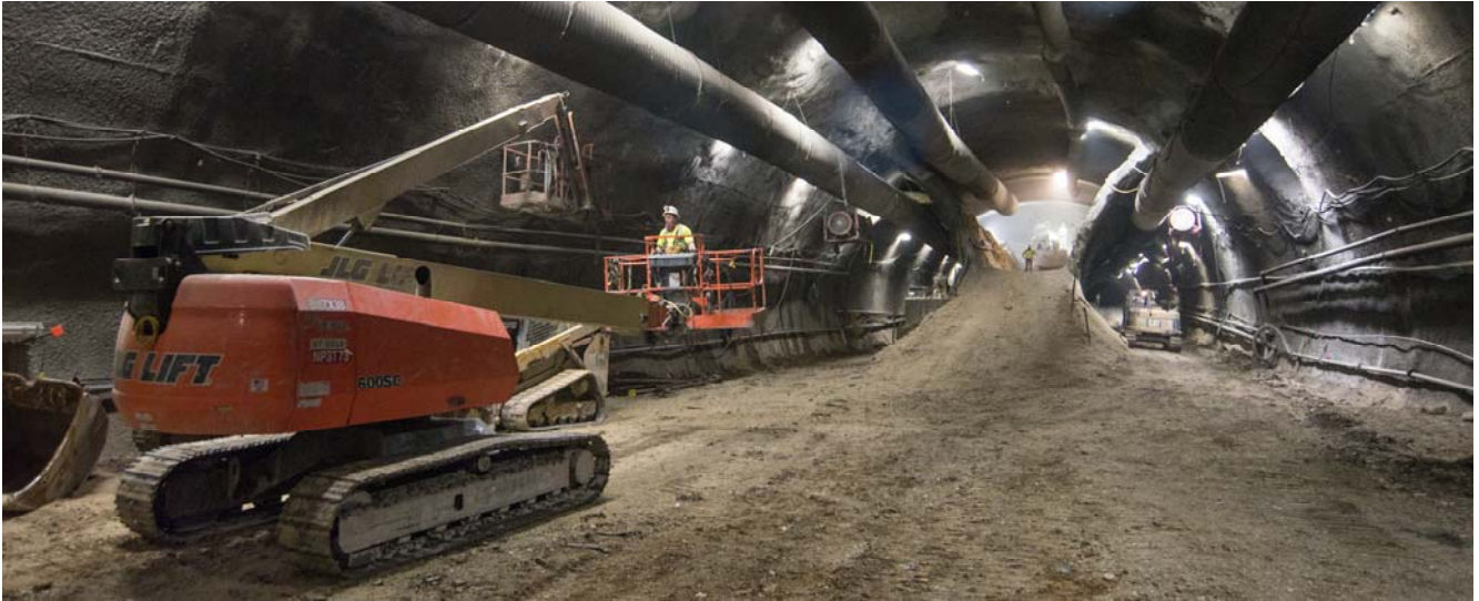
A man carefully maneuvers a boom lift down the south platform cavern for Chinatown Station., while shotcrete spraying is being done inside the top heading beyond.
