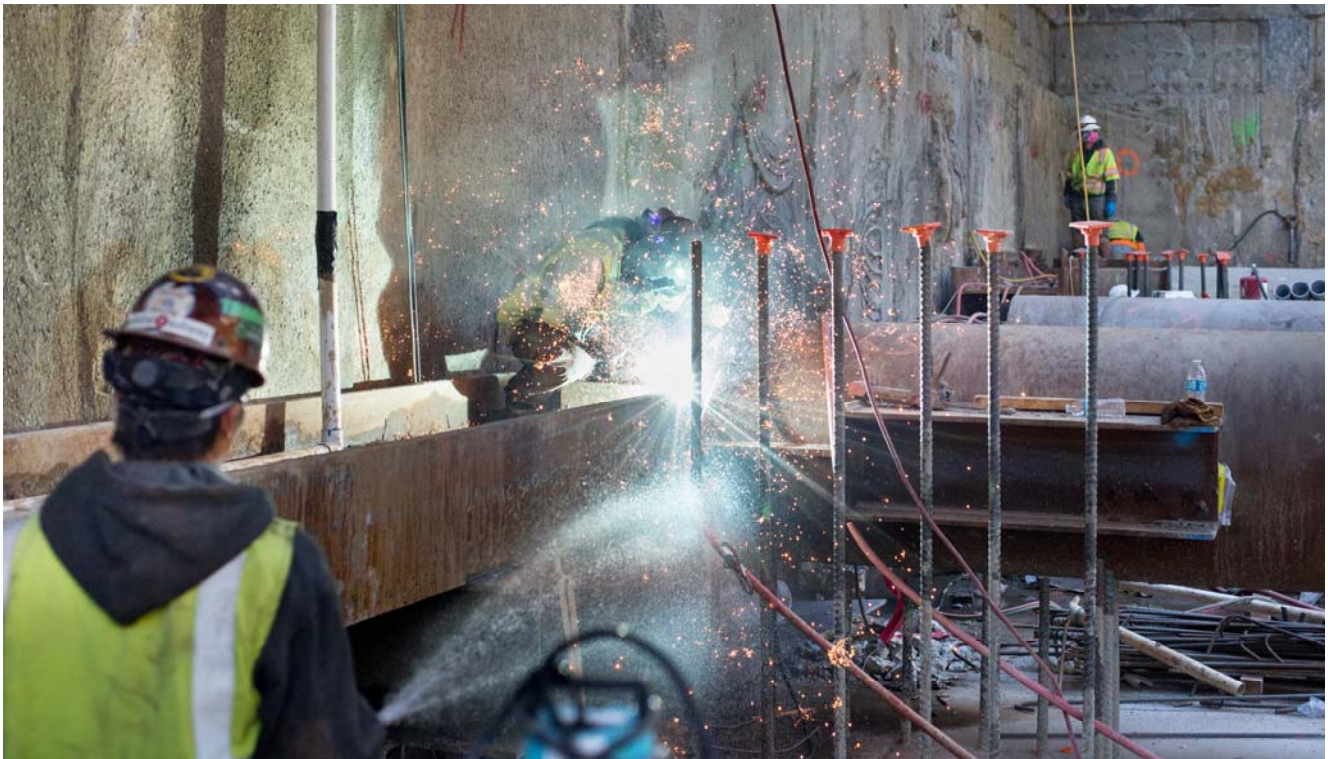
Two men work together at the western wall of the headhouse to keep the work area cool by spraying water while cutting portions of steel brackets slated for eventual removal.
