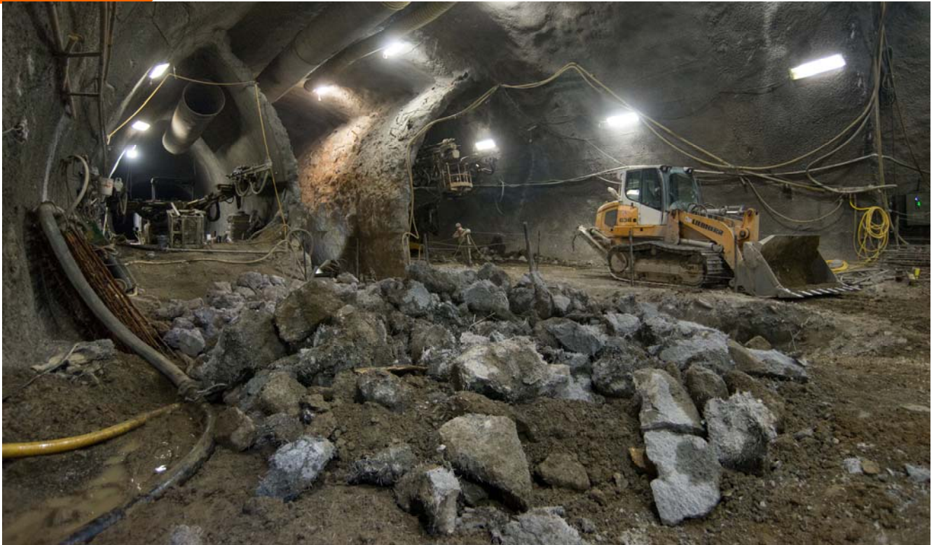
Chunks of demolished shotcrete wait to be broken down further where the platform cavern meets the cross-cut cavern entrance from the station headhouse.
