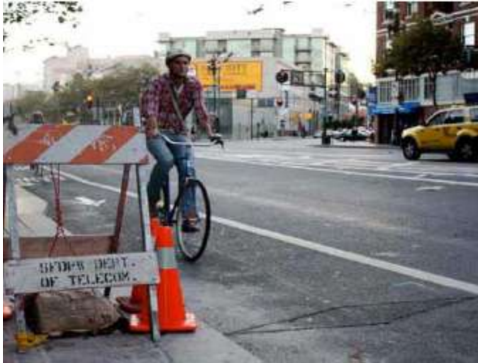
Image: Bicyclist approaching a newly installed loop detector.
