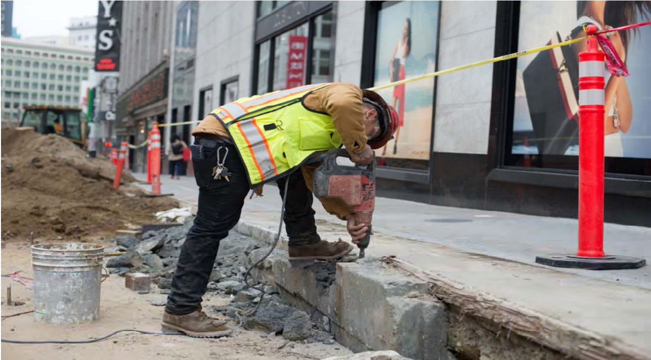
Site restoration work to prepare for the 2016 Winter Walk on Stockton, south of Geary.
