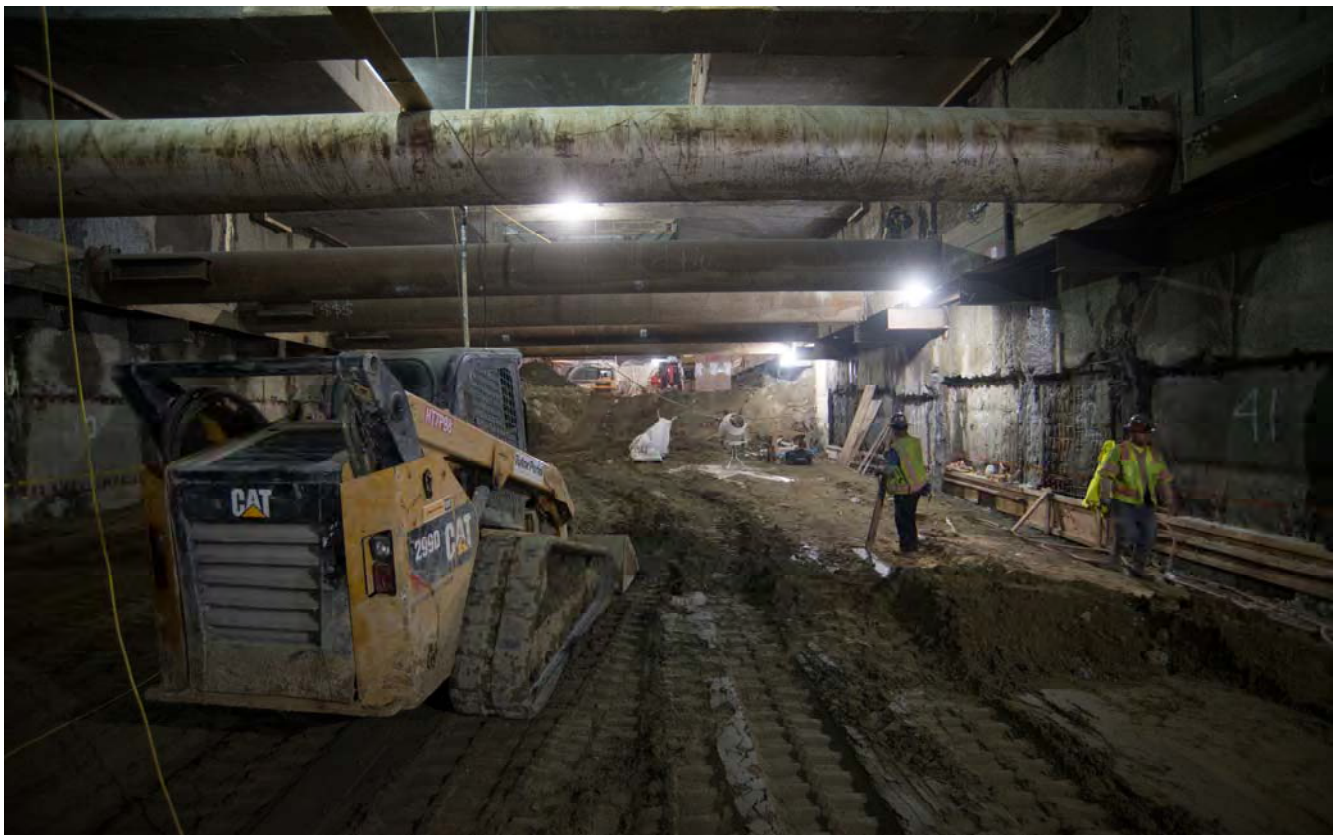
Workers install concrete forms at the base of the exterior slurry walls and grade the north end of the station box, to prepare for eventual invert slab construction.
