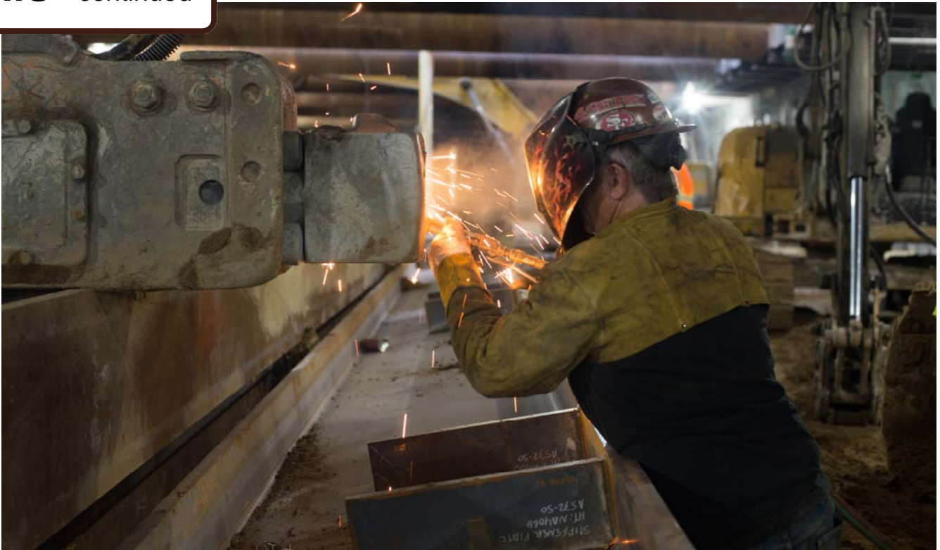
A mechanic fixes a large jackhammer used during excavation work inside the station box under Stockton.
