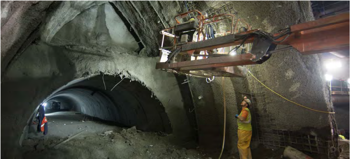
Workers inspect steel mesh and shotcrete installation work at the right side drift of the south station platform cavern.
