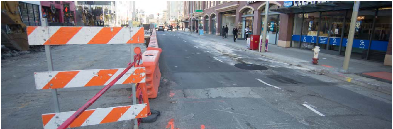
Crews on 4th Street in SoMa along the future surface portion of the alignment are conducting street restoration improvements one portion of the blocks at a time.
