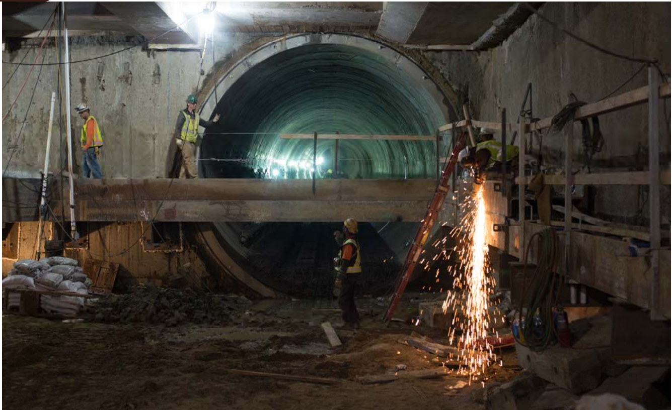
Sparks fly as workers install temporary steel bracing inside the station box under 4th Street in SoMa.
