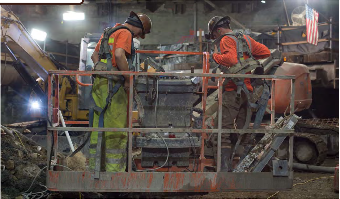
Workers suit-up with safety harnesses before being lifted toward the ceiling of the cross-cut cavern to inspect shotcrete reinforcing work.
