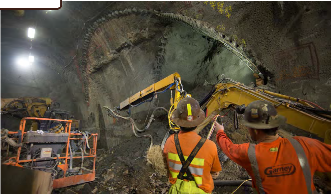
With the first phase of drilling and soil grouting complete, work to excavate the side drifts of the south platform cavern area has begun.
