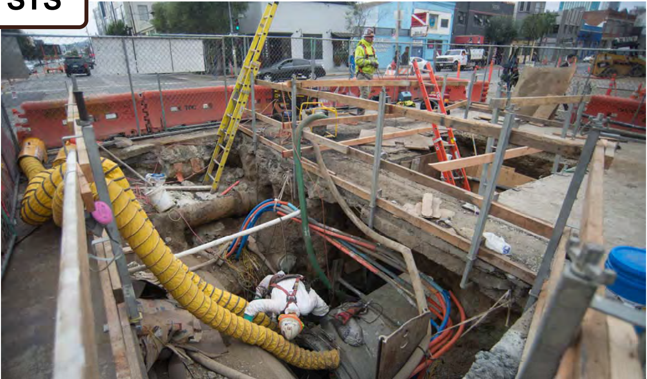
Workers have been conducting sewer reconstruction work at the 4th and Brannan intersection, where a new section of sewer is being fitted to the old.
