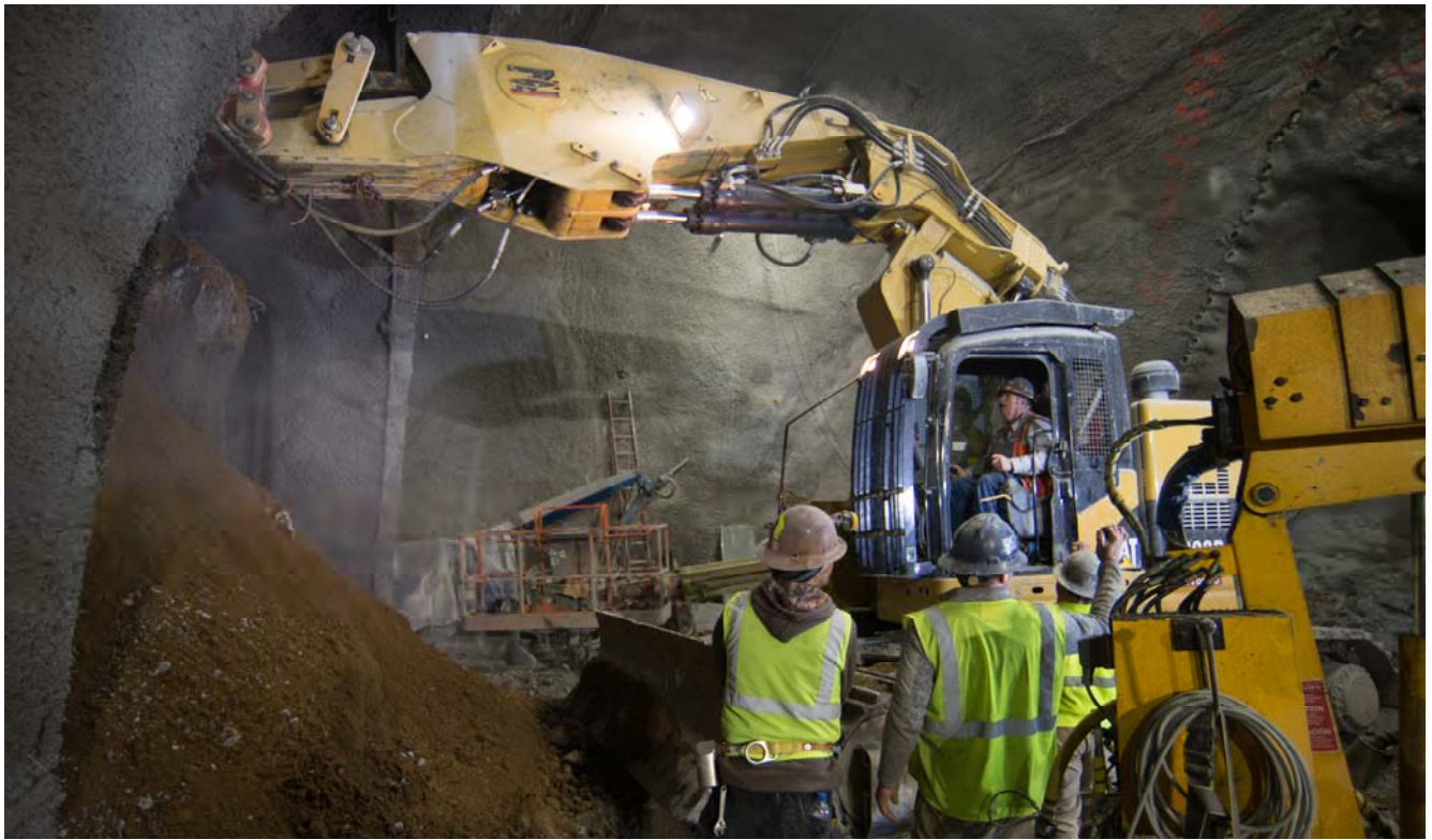
A large excavator fitted with a special grinding wheel slowly works its way through the previous excavation's shotcrete wall and the soil beyond.
