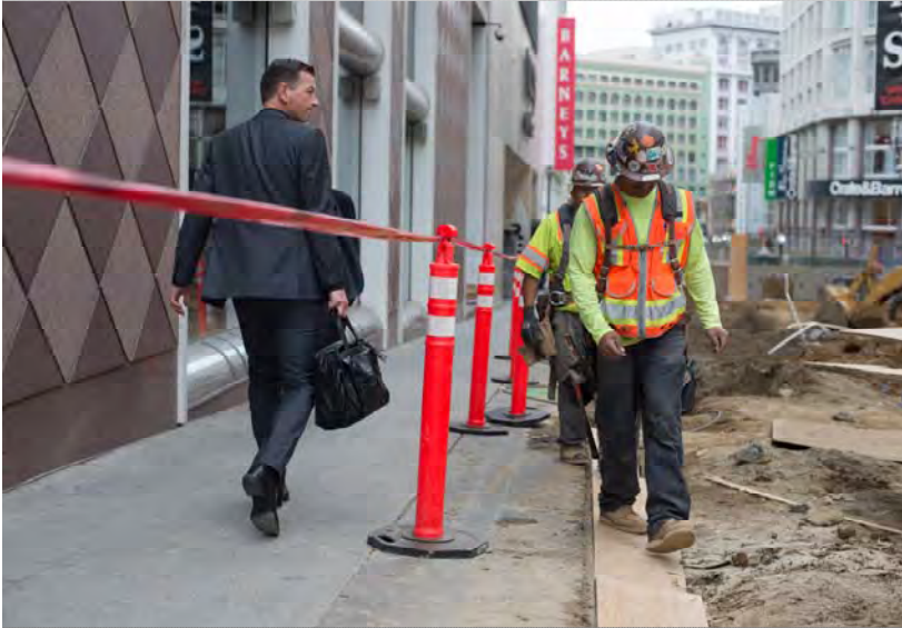
1 Crews clean up the work site, remove pedestrian barriers, and grade the site
