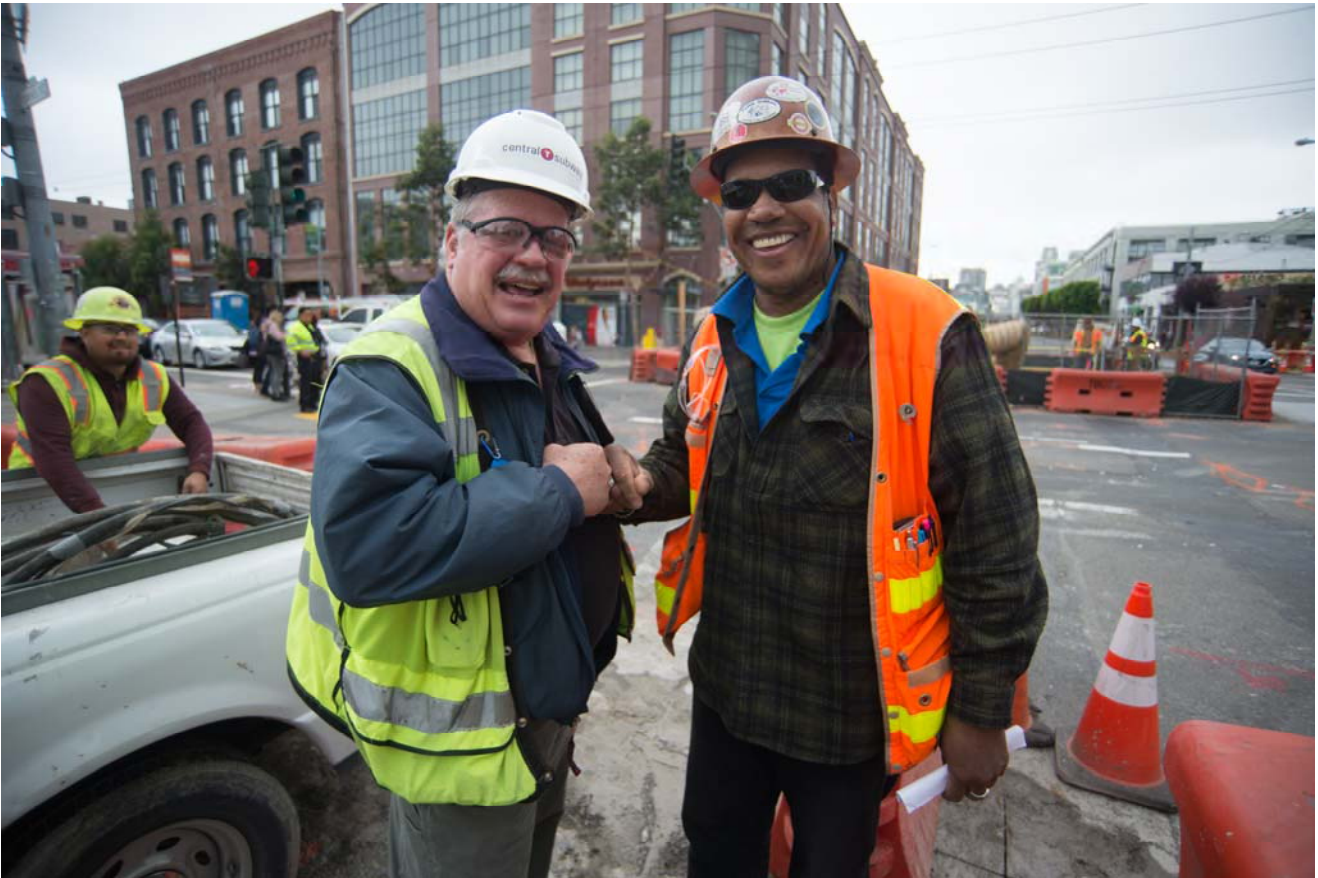
Project Safety officer Jeff Kraus greets TPC safety officer Gilbert Williams near street repaving work at 4th and Townsend.
