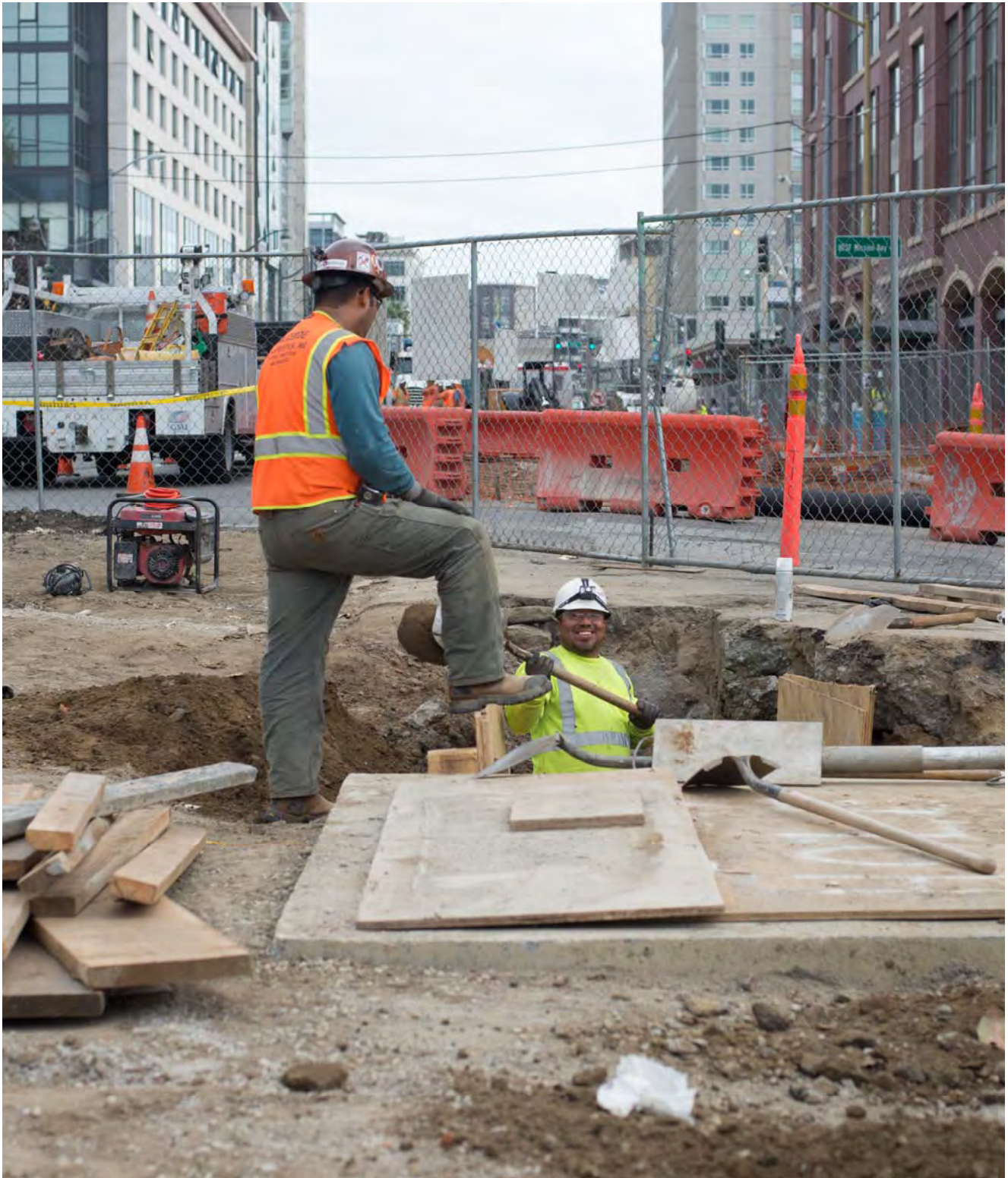
Two workers address a utility trench near a newly-constructed manhole structure on 4th, near Bluxome.
