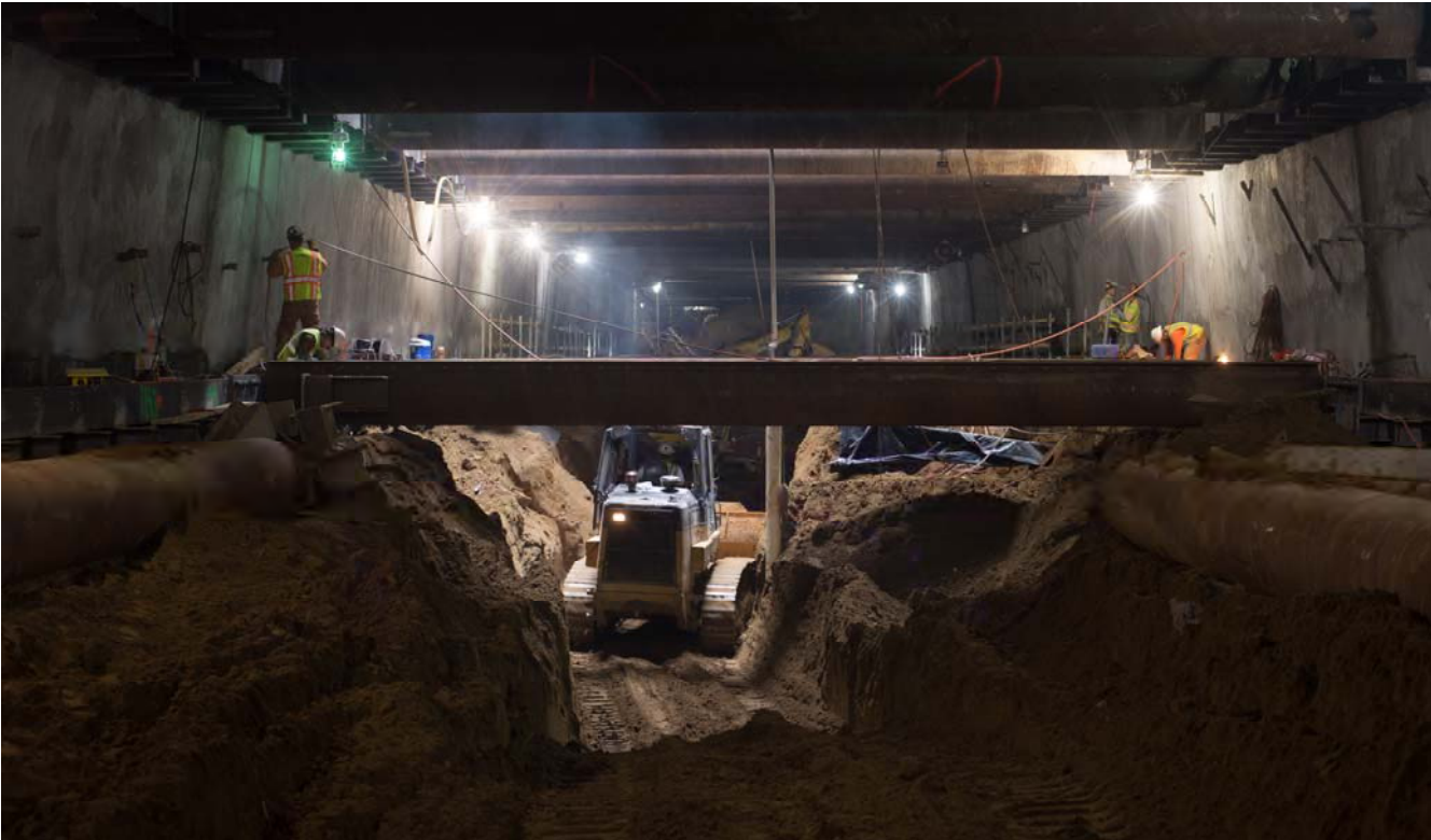
Work to excavate the next level of the station box has begun under Stockton Street. This work is carried out underneath the Winter Walk and soil is removed at night.
