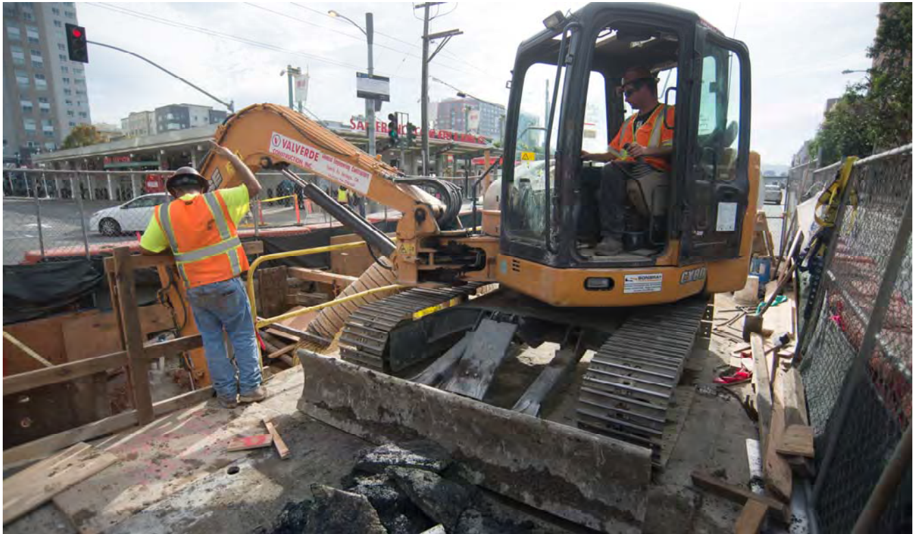
A large, reinforced concrete manhole cover is being constructed at the 4th and Townsend intersection.
