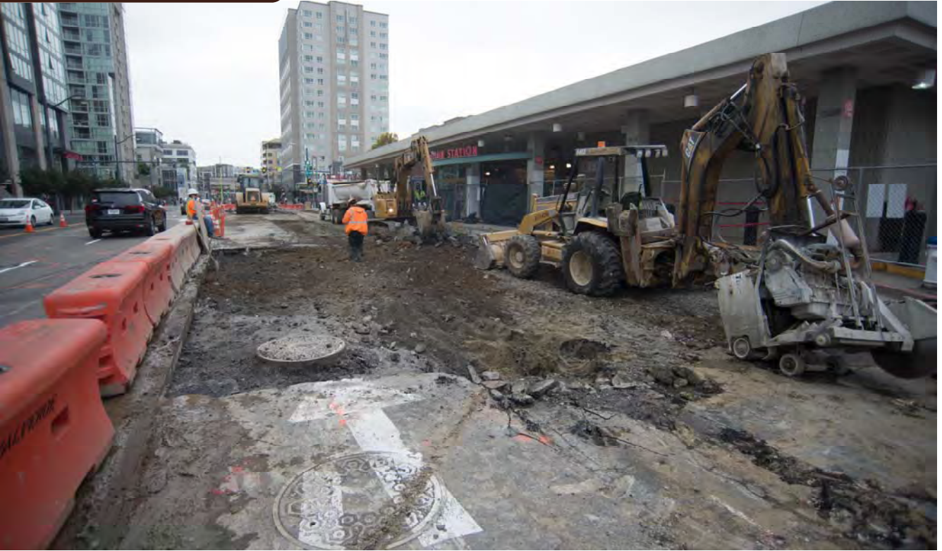
Workers have been resurfacing sections of 4th Street following the end of utility work in certain areas.
