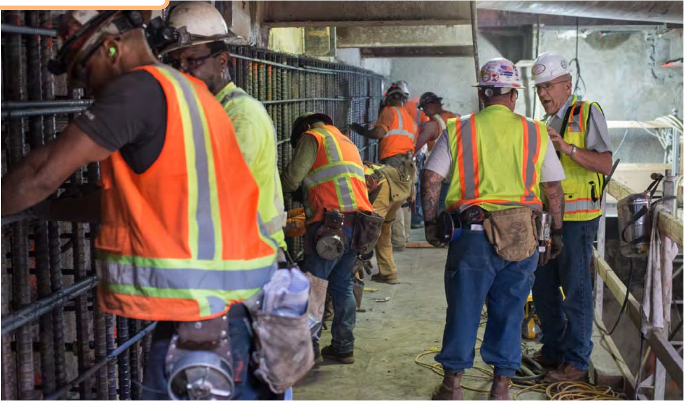
Workers construct a long rebar cage at the northwest corner of the headhouse site.
