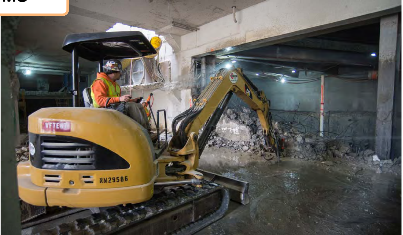
A small excavator fitted with a jackhammer breaks through the outer wall of the Union Square Garage, opening it up to the north station concourse.
