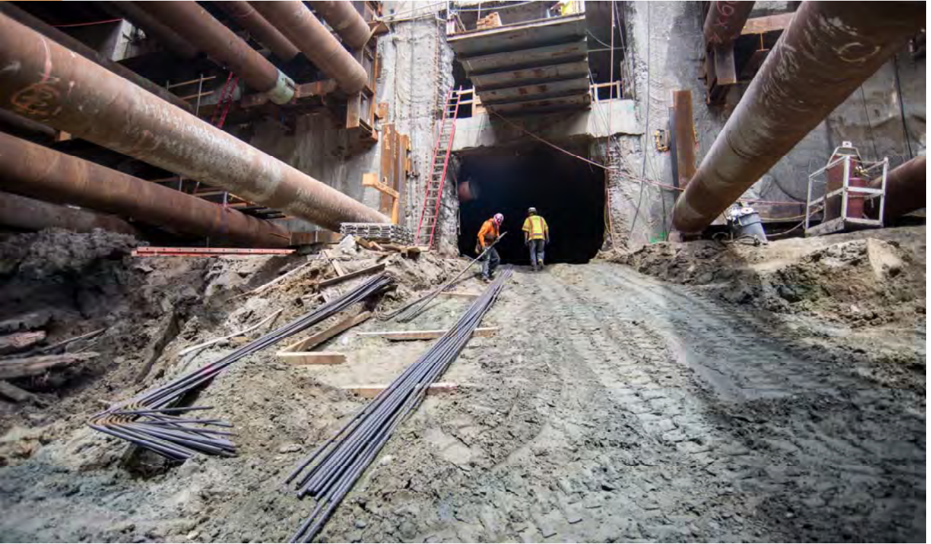
Long bundles of rebar are carried in one piece at a time during the assembly of rebar cages used in construction of the mezzanine floor slab.
