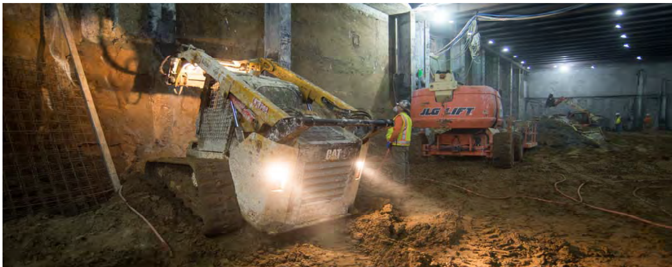
A bobcat fitted with a jackhammer removes concrete from around steel beams in the north concourse near where the entrance to the future north entrance will be located.
