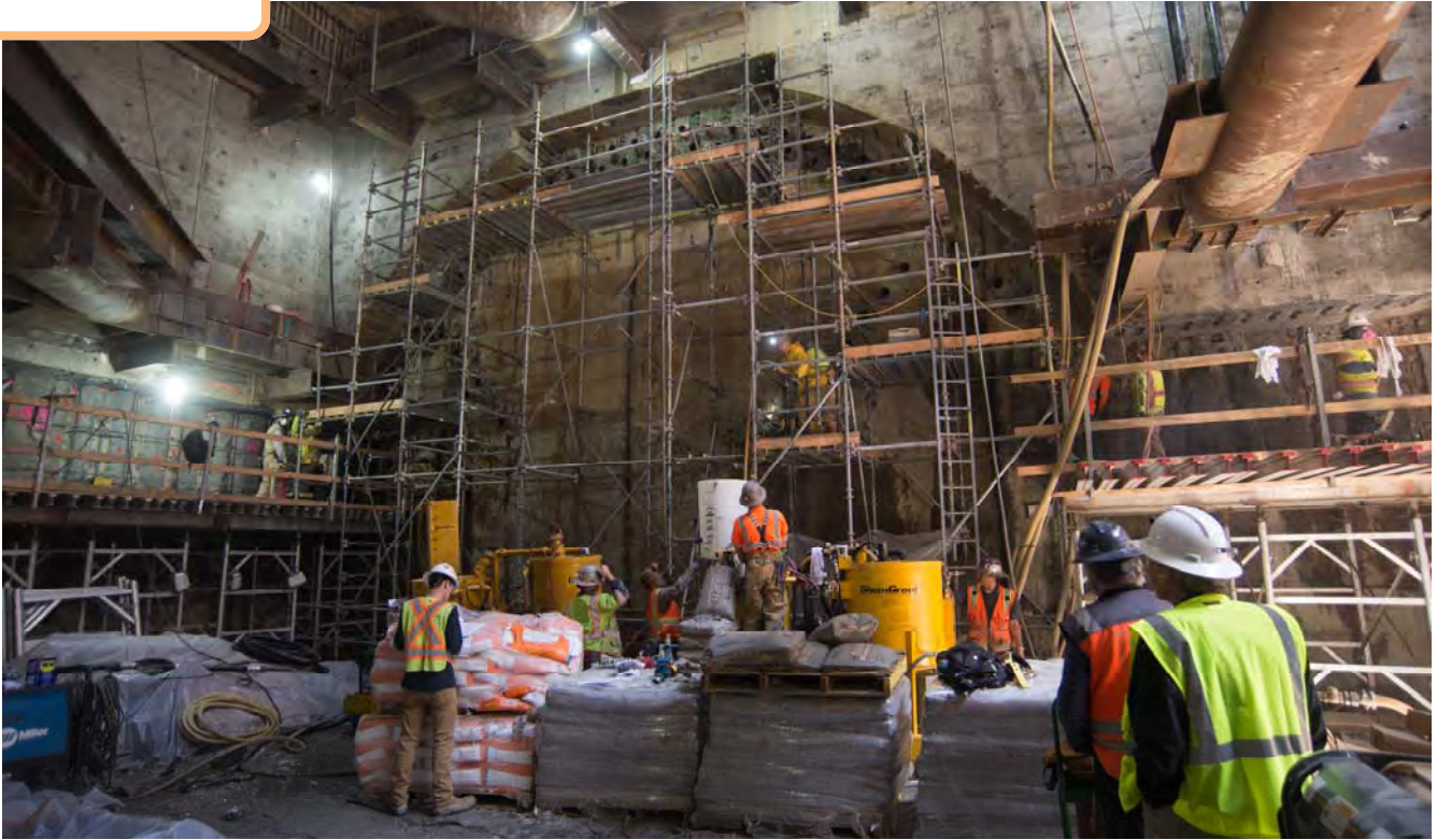
Veiled in scaffolding, the fare gate archway will eventually become the entrance to the station cavern, yet to be excavated.
