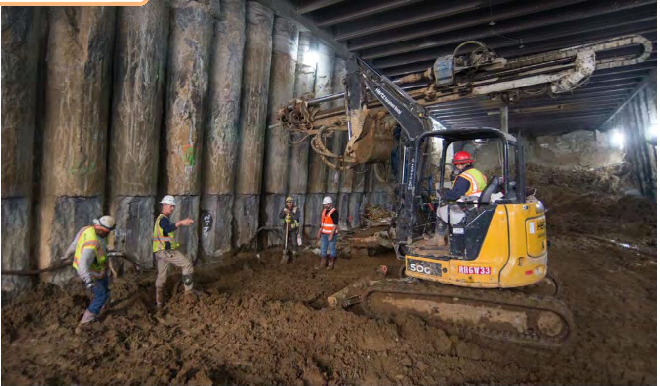
Workers are conducting drilling work inside the station box between Geary and O'Farrell.
