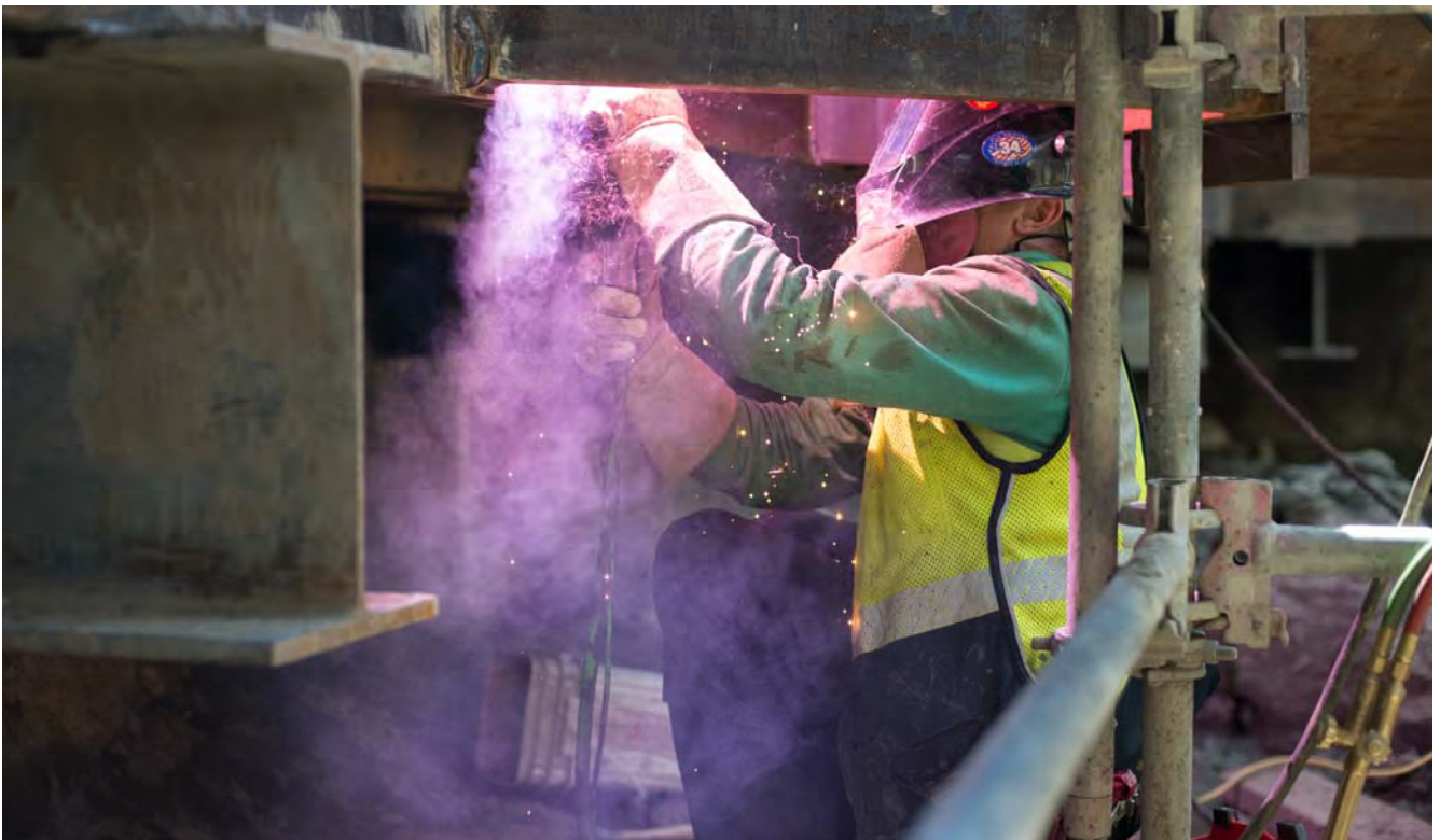
Smoke colored with violet light streams from under a large steel I-beam where a welder is attaching temporary supports on the east side of the headhouse.
