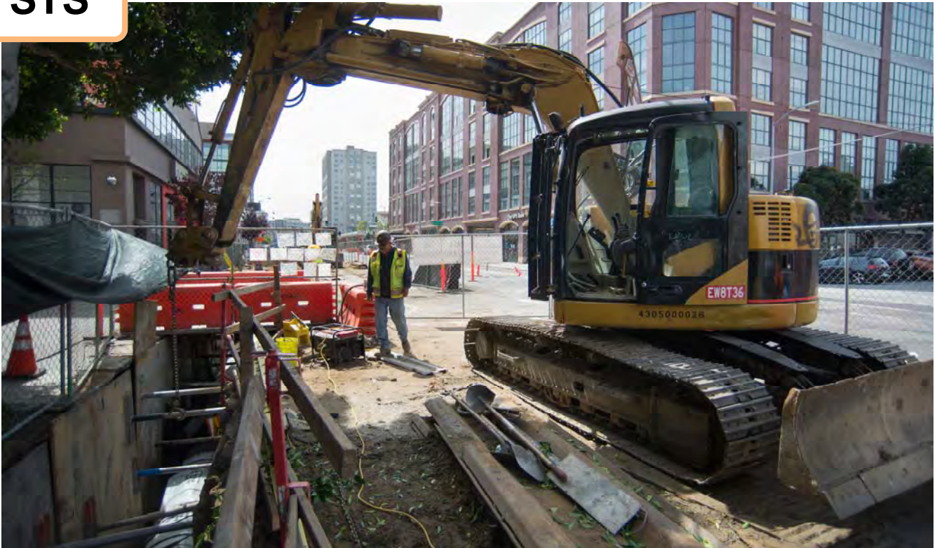
An excavator operator helps remove trench shields after a section of new sewer line has been installed north of Bluxome on the east side of 4th.
