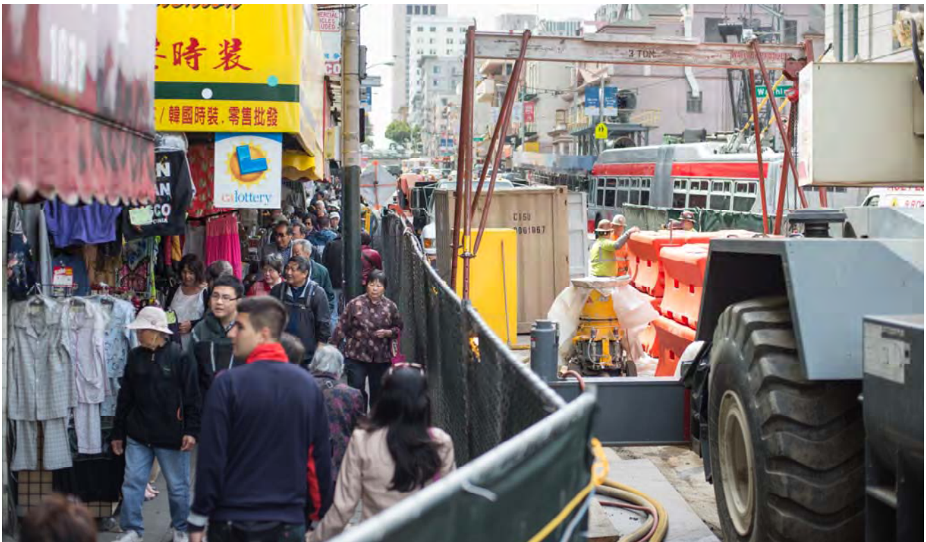
Workers set up a moveable gantry to move equipment around the north access shaft work site, while pedestrians and shoppers walk through the area nearby.
