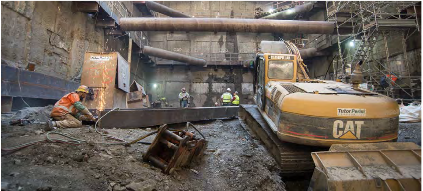
Looking south inside the station headhouse, where work to prepare temporary steel reinforcing beams for another round of excavation is underway.
