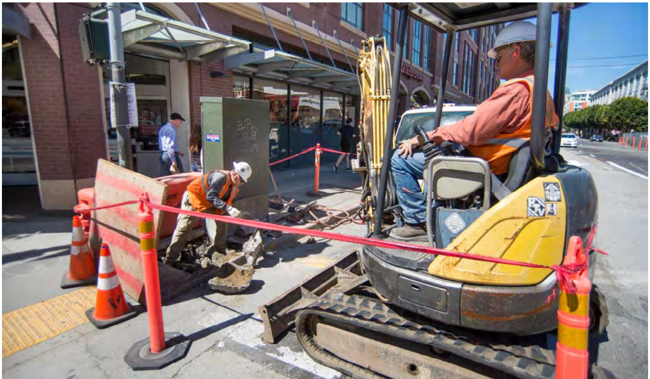
A worker removes debris from a hole in the sidewalk being dug at 4th and Townsend to install the foundation of an OCS pole.
