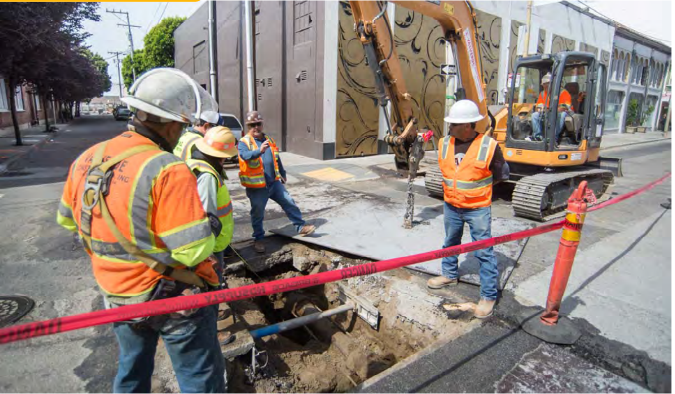
A crew discusses specifics utility excavation operations at 4th and Freelon. Lateral utilities are shown exposed in a recently-excavated trench.
