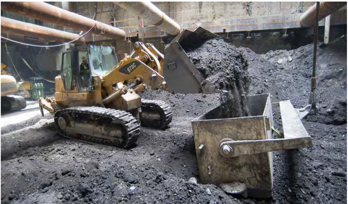
A bulldozer dumps a load of excavated material into the steel bucket used to remove it from inside the headhouse. This bucket is lifted to the surface by a large crane, and material is accumulated for loading onto waiting trucks.
