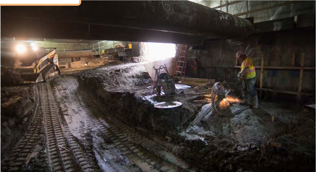
Before constructing concrete forms for the mezzanine level floor slab inside the station box, sections of tunnel roof must be cut out to make clearance for the forms.
