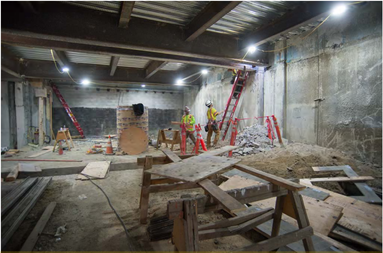
Corrugated steel decking covers the south concourse at Ellis and Stockton. Work to construct the roof of this portion of the station is ongoing.
