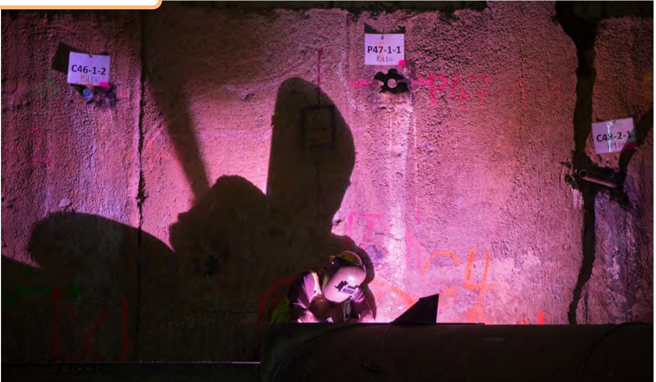
A violet shadow is cast on the headhouse slurry wall from a welder fashioning brackets for temporary steel supports.
