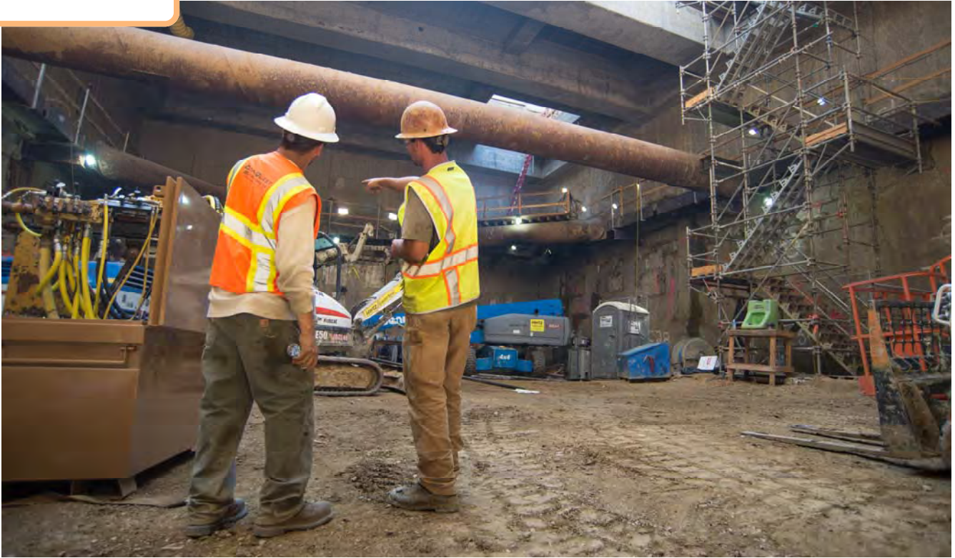
Inside the Chinatown Station headhouse structure, work to waterproof the exterior walls is conducted with each level of excavation completed.
