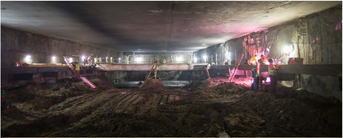
Welders attach steel reinforcing beams to the exterior slurry walls of the station box inside Yerba Buena/Moscone Station.
