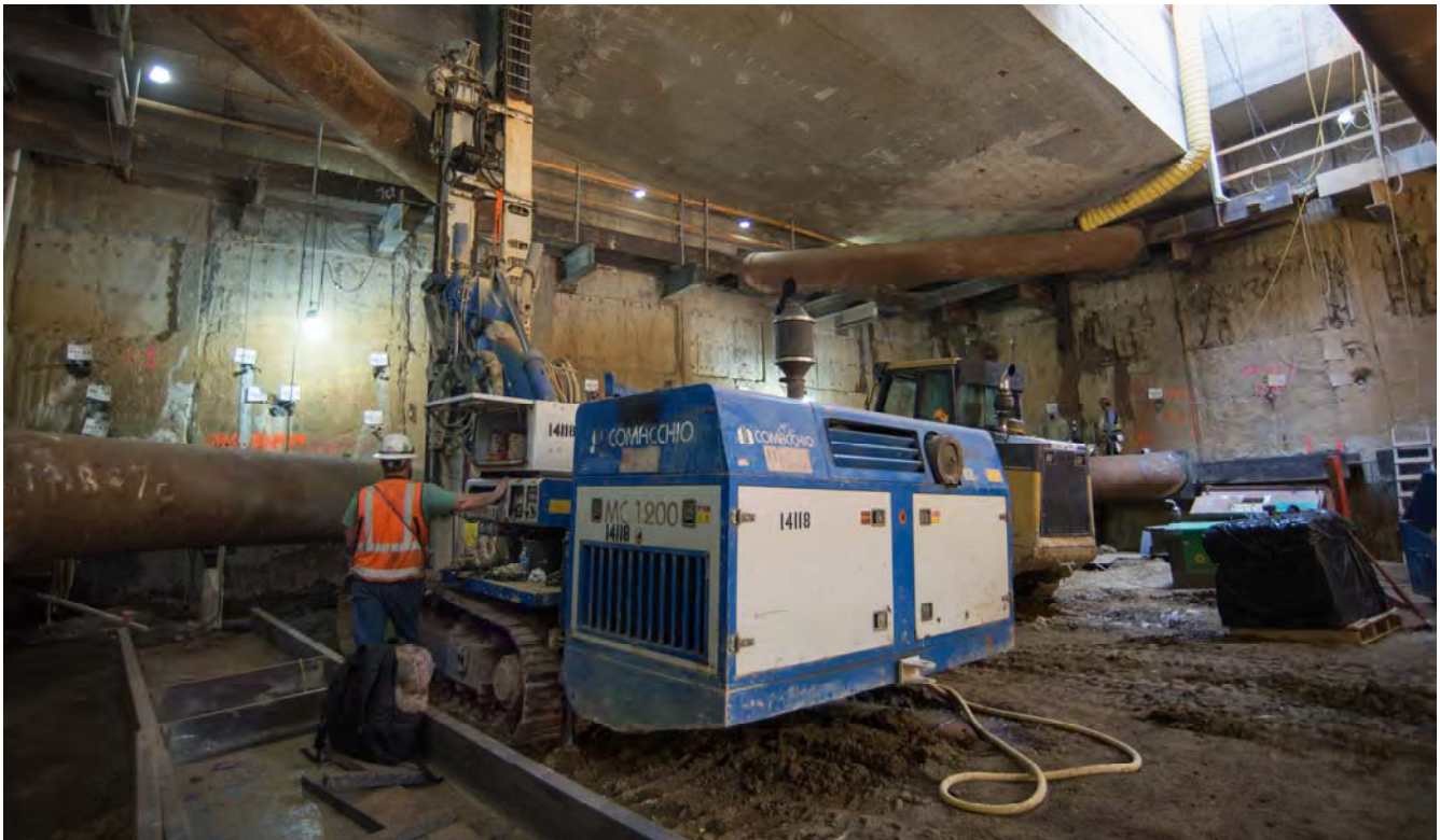
A drill rig is used to inject a grout-like solution into the surrounding soil, improving its stability and waterproofing the station entrance structure.
