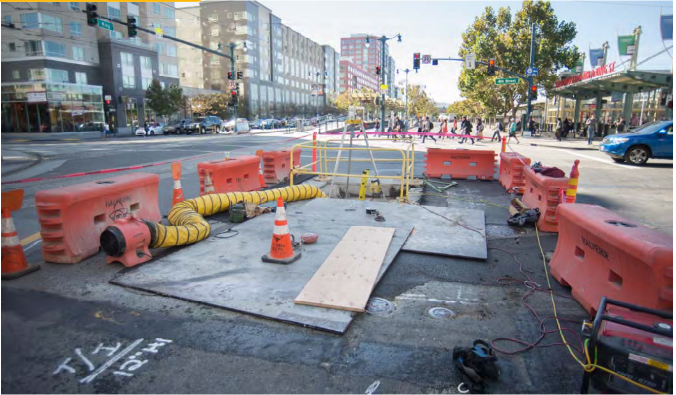
Safety barriers contain the work zone on the north side of the 4th and King intersection. Work to install new track configuration here will commence the week of Veterans Day.
