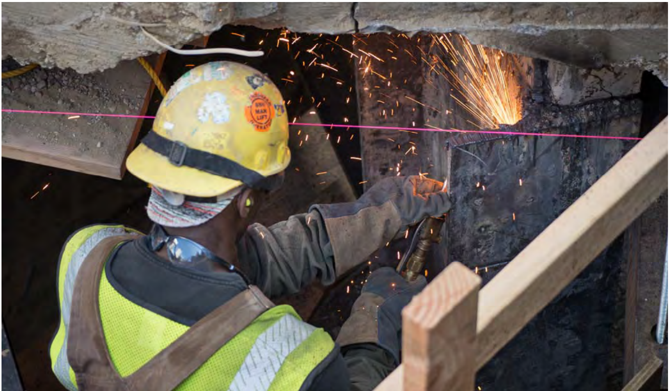
A metalworker cuts specific portions of a steel I-beam away to prepare it to be tied into additional structural elements.
