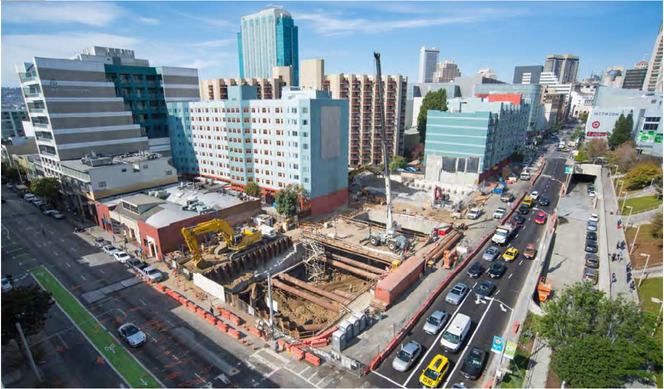
The site of the Yerba Buena/Moscone Station and headhouse structure as seen from the roof of a nearby building.
