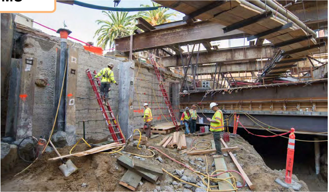
Inside the north concourse, work to build structural elements of the concourse roof is underway while live utilities are suspended overhead.
