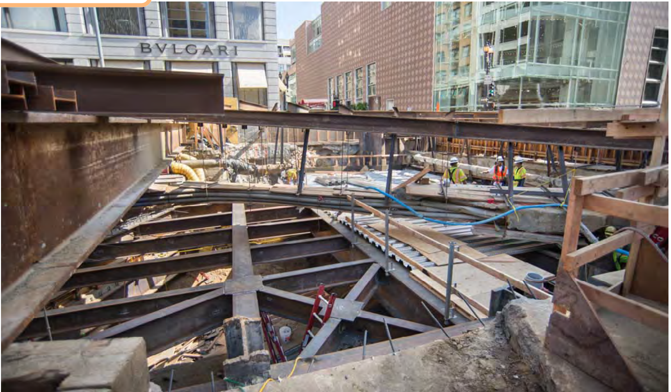
Exposed structural steel of the north concourse roof deck greets the sun prior to being covered over in corrugated decking, and later rebar and concrete.
