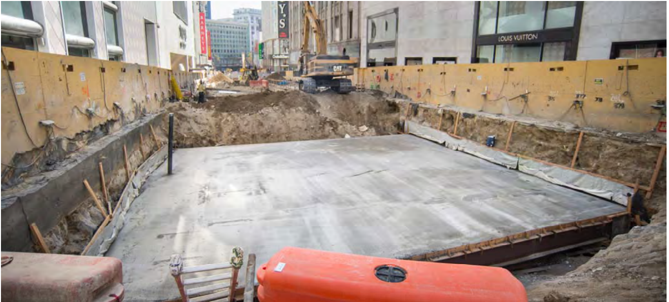
A newly-constructed section of roof slab is seen exposed between O'Farrell and Geary. After constructing each section of roof slab, workers backfill the section and move to the next.
