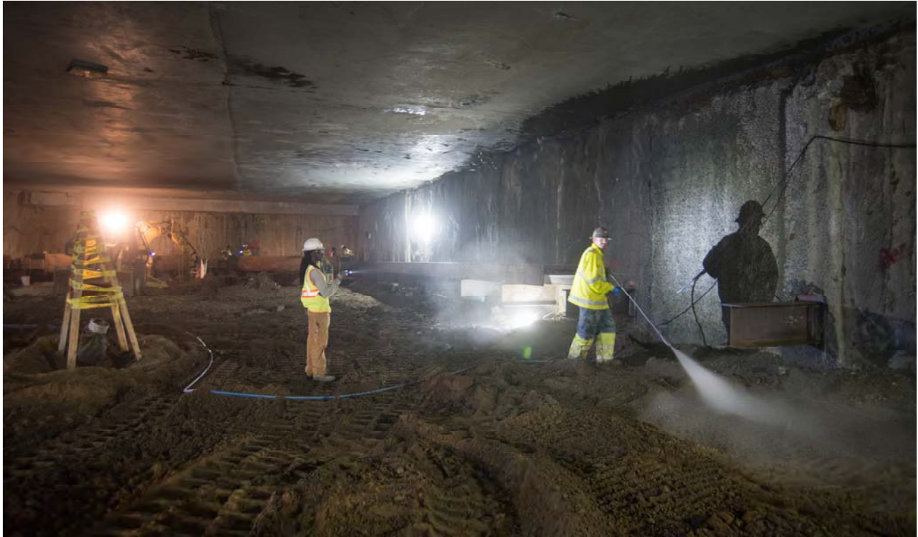
Inside the station box, a worker is seen using a high-pressure hose to remove loose material from the exterior slurry walls, and clean them ahead of reinforcing steel installation.
