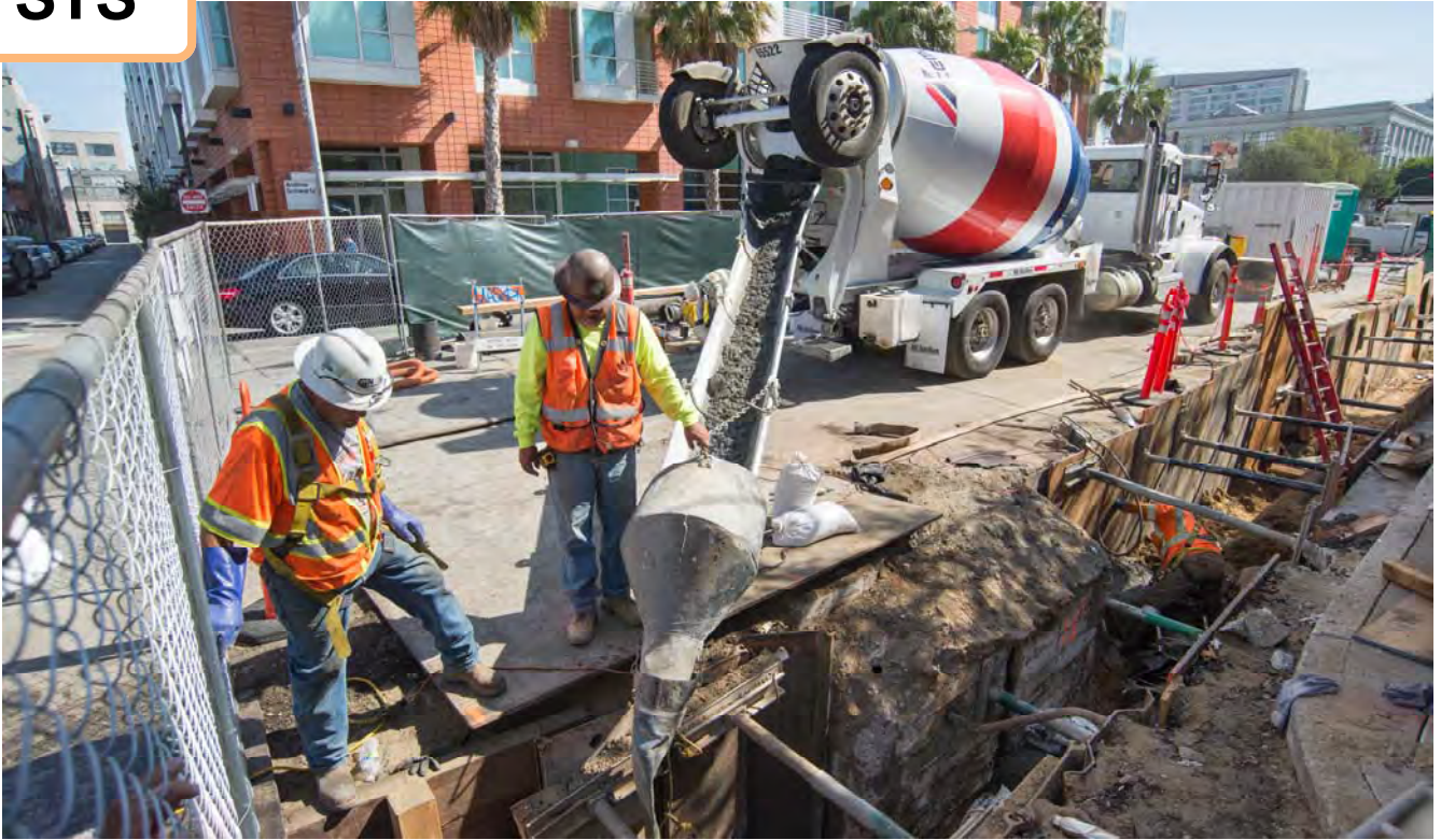
Workers carefully pour concrete in a trench to create a base slab for utilities to be installed here.
