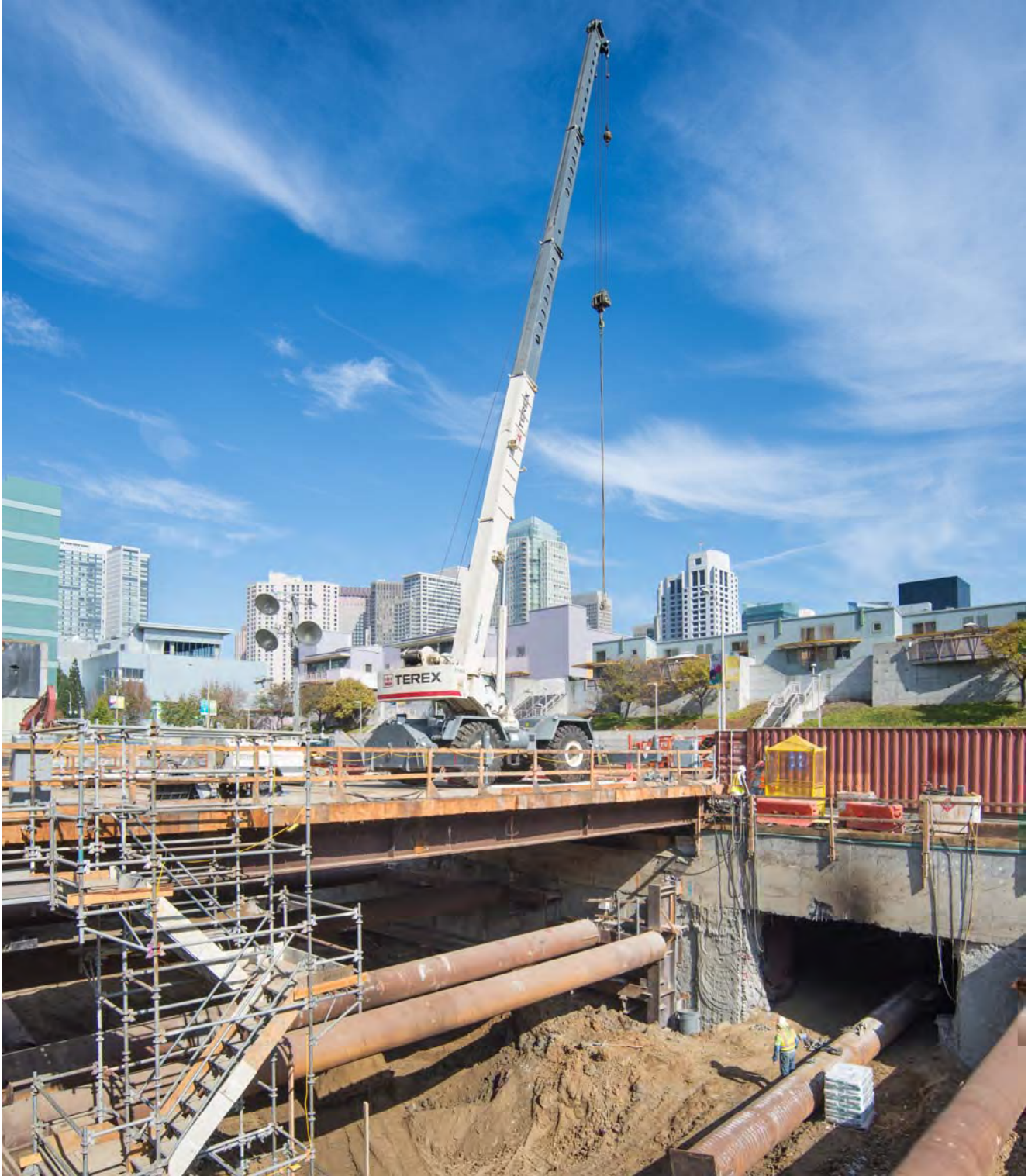
A large crane is used at the Yerba Buena/Moscone Station site to lift steel reinforcing members and other heavy equipment into the headhouse and station box interior.
