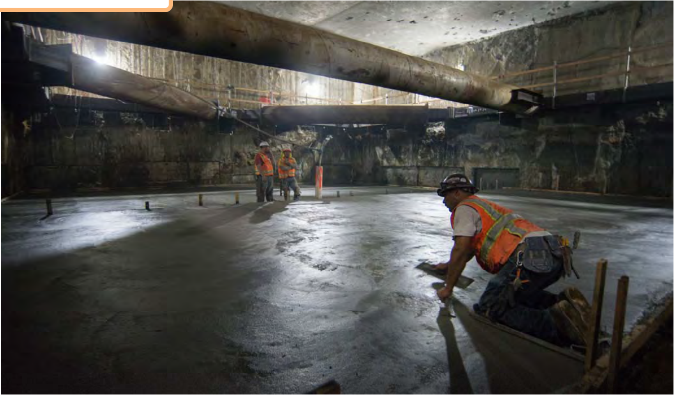
A temporary “rat slab” of concrete is installed as the base of a future concrete form.
