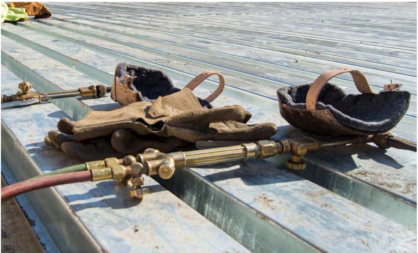
A cutting torch waits to be packed up at the former TBM retrieval shaft site. The site will soon be completely demobilized, and all equipment will be removed.
