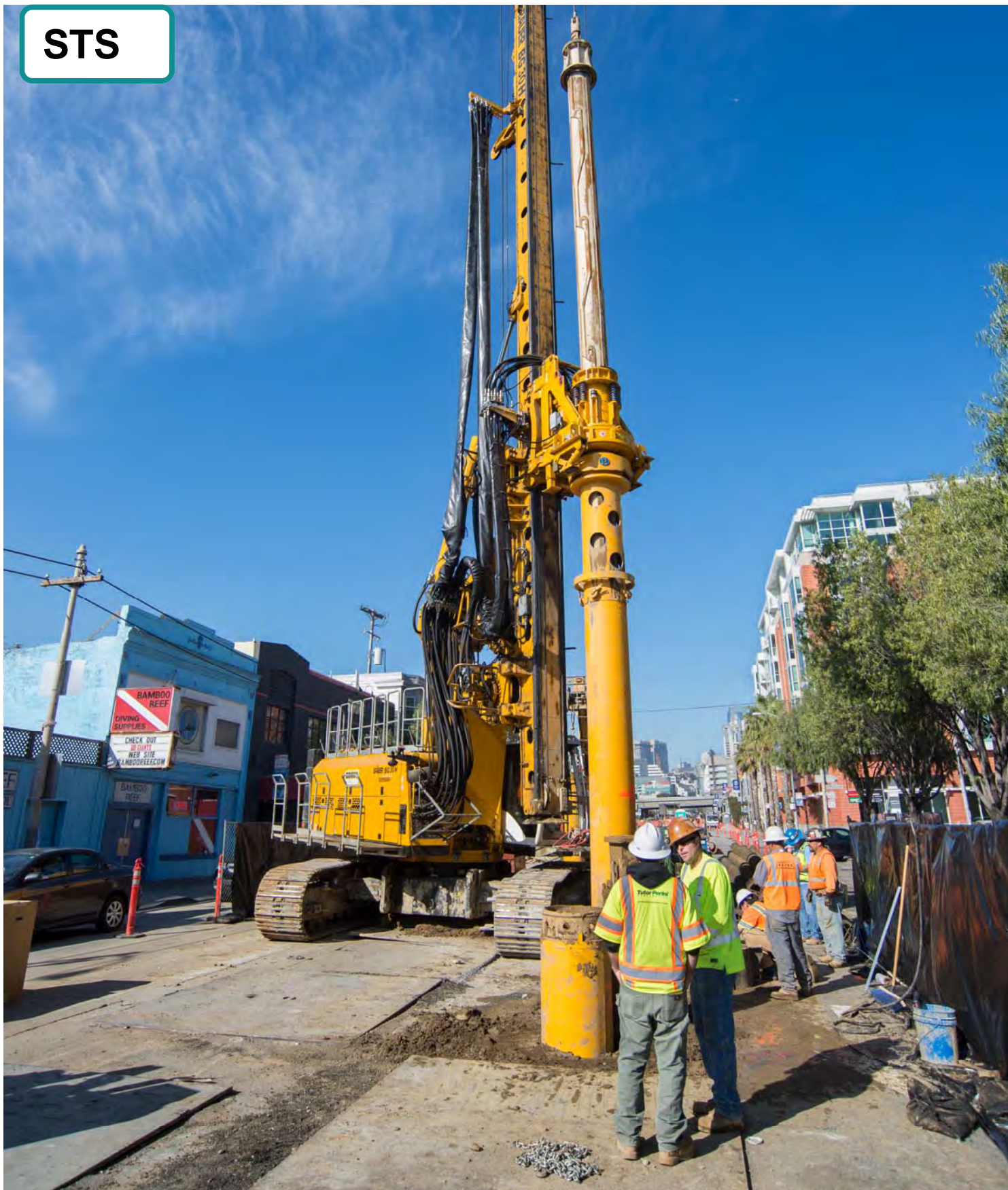
This machine, called a rotary drill rig, will aid in construction of the foundation of the future 4th and Brannan surface station.
