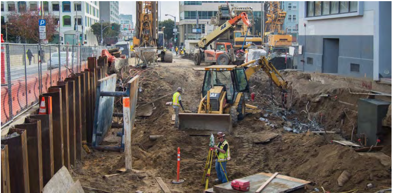
Work to excavate the interior of the station has begun at the Yerba Buena/Moscone Station site.
