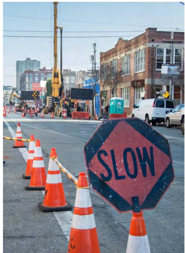
Utilities are being relocated and upgraded ahead of foundation work and surface track construction.
