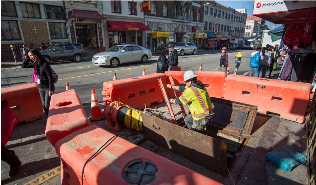
Workers have been accessing the basement of a building at the corner of Washington and Stockton to install the necessary plumbing for a high-pressure fire hydrant nearby.
