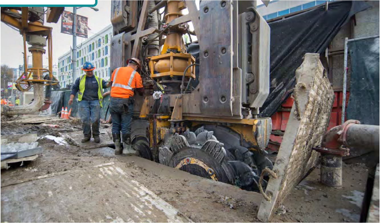
This device, called a hydromill, excavates vertical wall sections which, joined together, will comprise the future station's structural walls.
