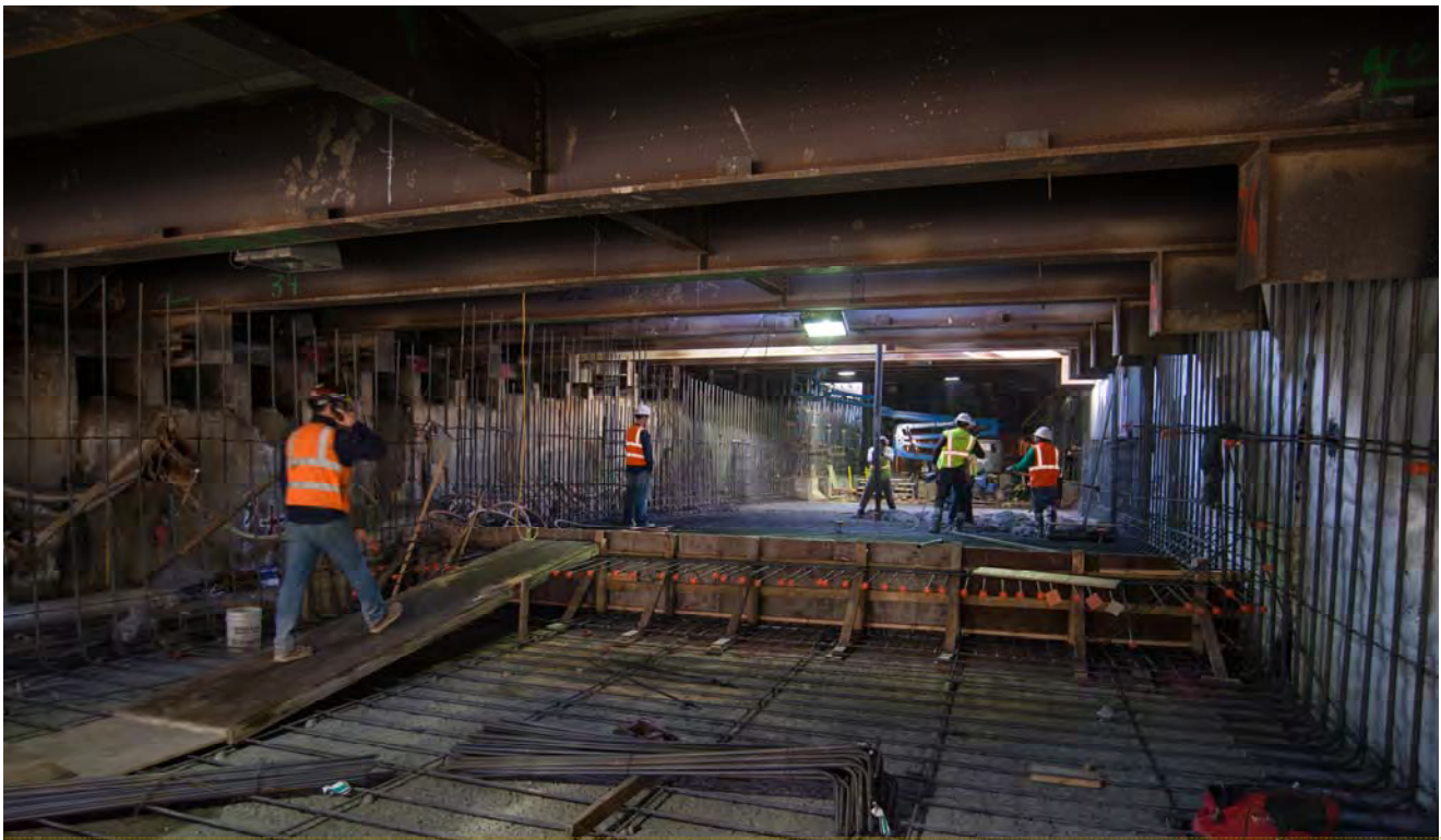
Construction of the tunnel portal continues in phases. The floor slab is being constructed in sections while rebar goes into place for future interior walls.
