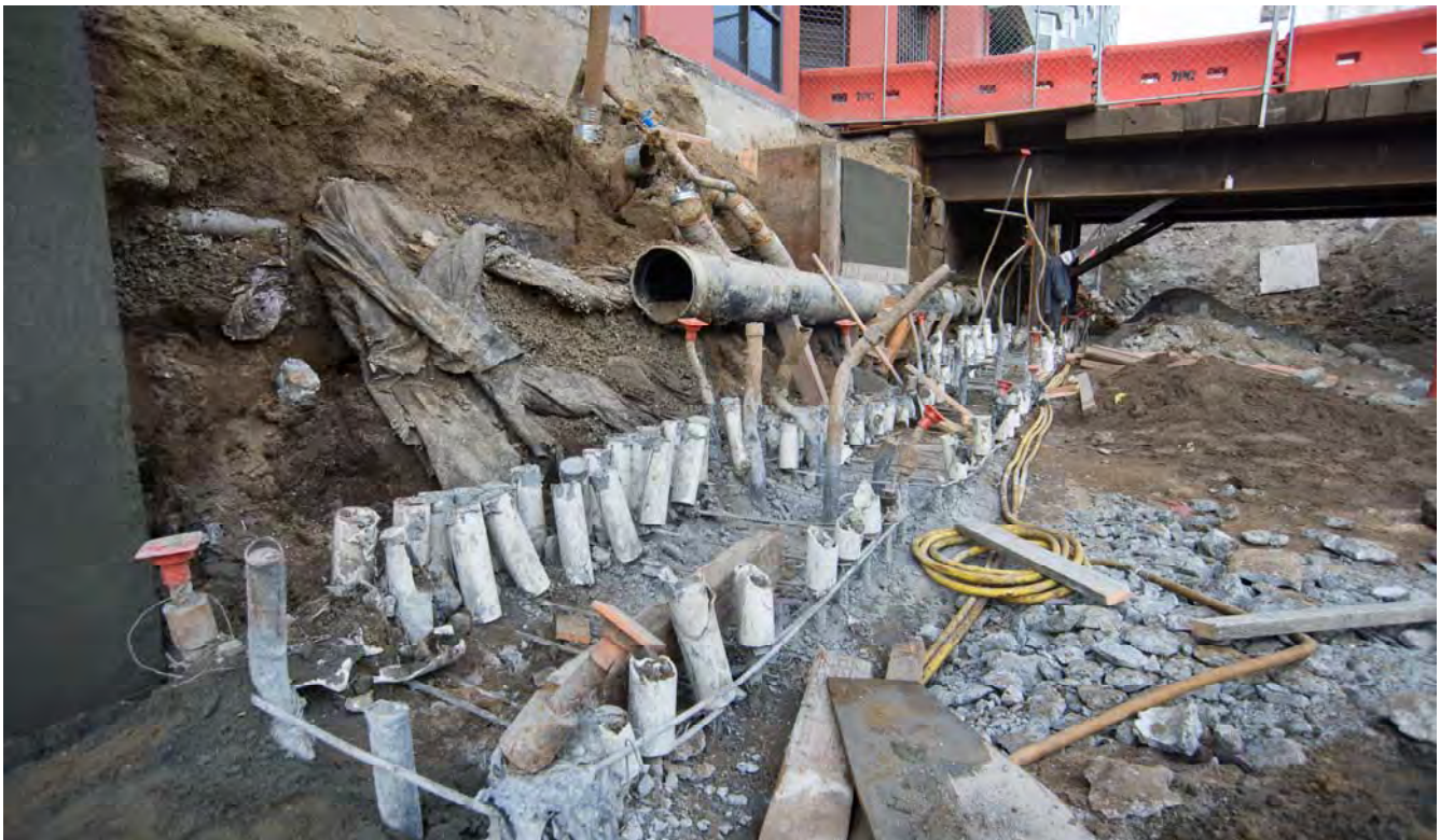
The tops of completed underground wall sections can be seen here on the east side of 4th Street. They are being exposed to attach them to the future roof slab.
