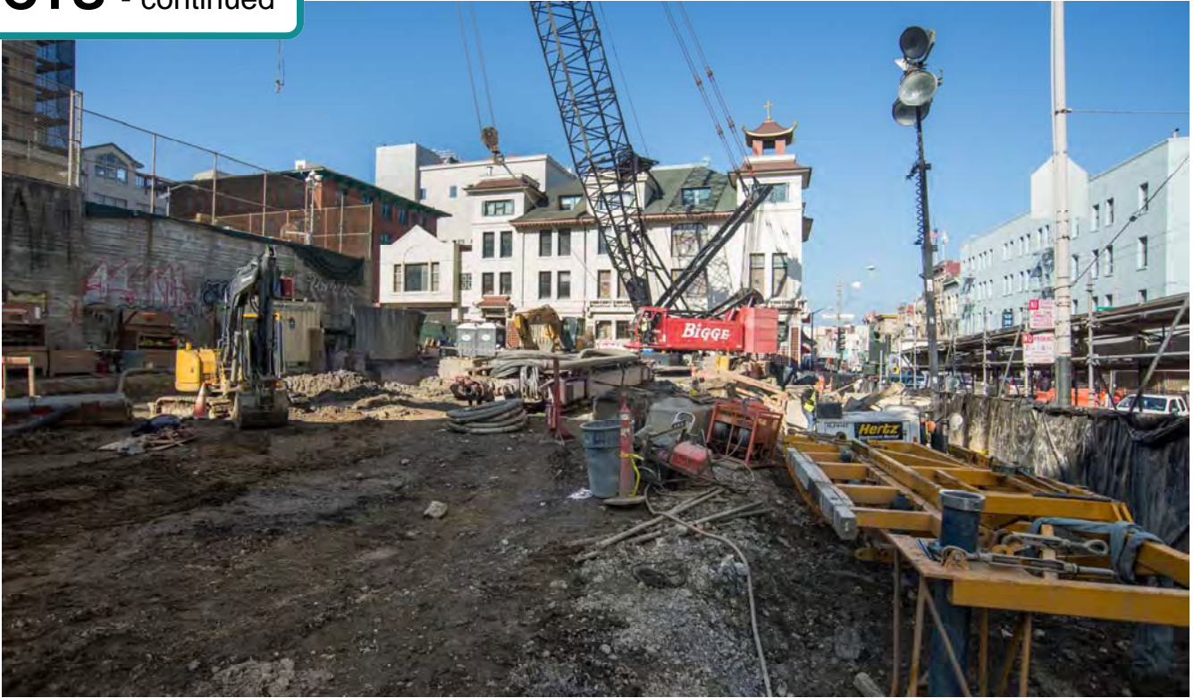
All slurry wall support equipment has now been removed at the Chinatown Station site, and work will begin to transition to station excavation.
