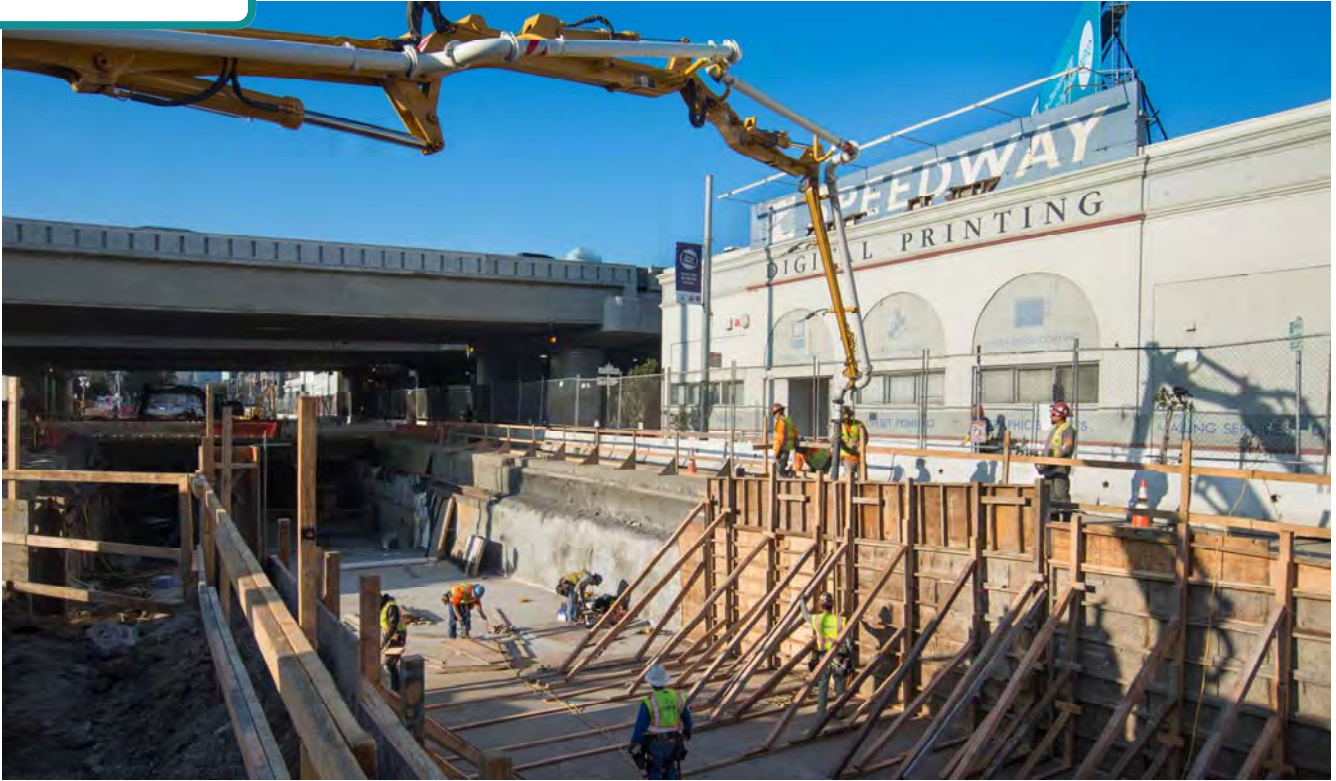
Temporary shoring walls are being poured at the end of the future tunnel portal ramp. These walls will hold back the soil while the structural ramp elements are constructed.
