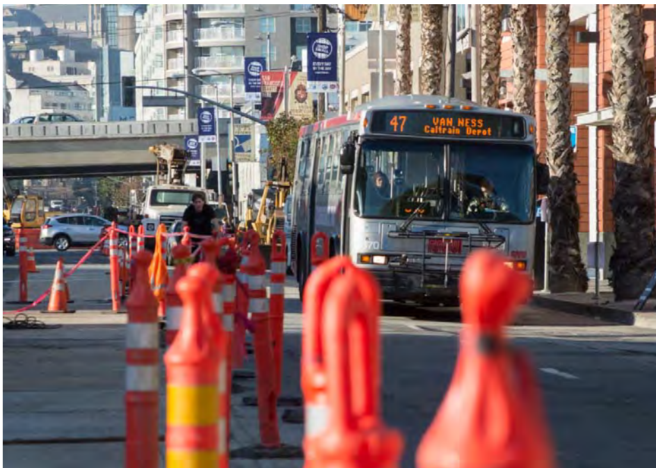
A 47 bus approaches the future 4th and Brannan surface station location, where foundation pile construction is underway.
