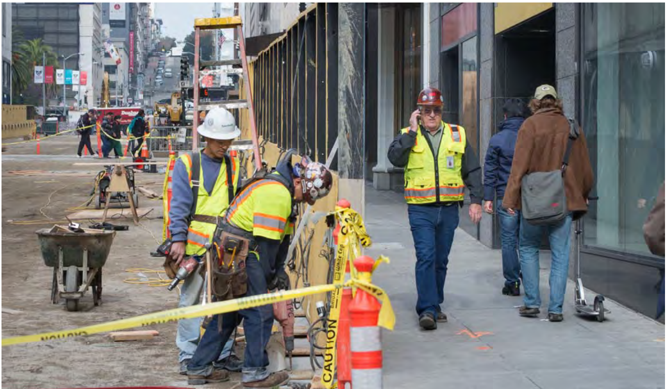
This safety barrier protects passing pedestrians from construction activity.
