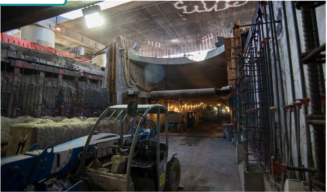
The partially-completed tunnel portal begins to take shape, with the roof opening up to a “C” shape under the I-80 overpass.
