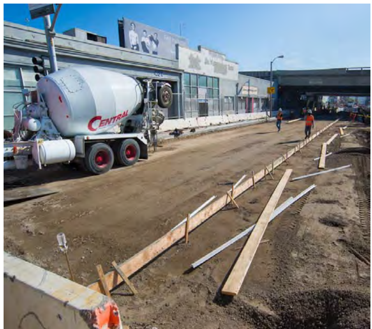
3 The surface is graded and a new road slab is poured - see pgs. 43 -44
