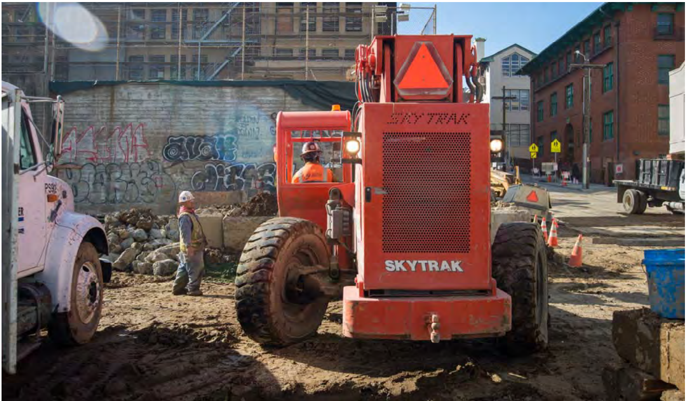
This skytrak driver moves equipment around the site to aid in the demobilization of slurry wall operations.
