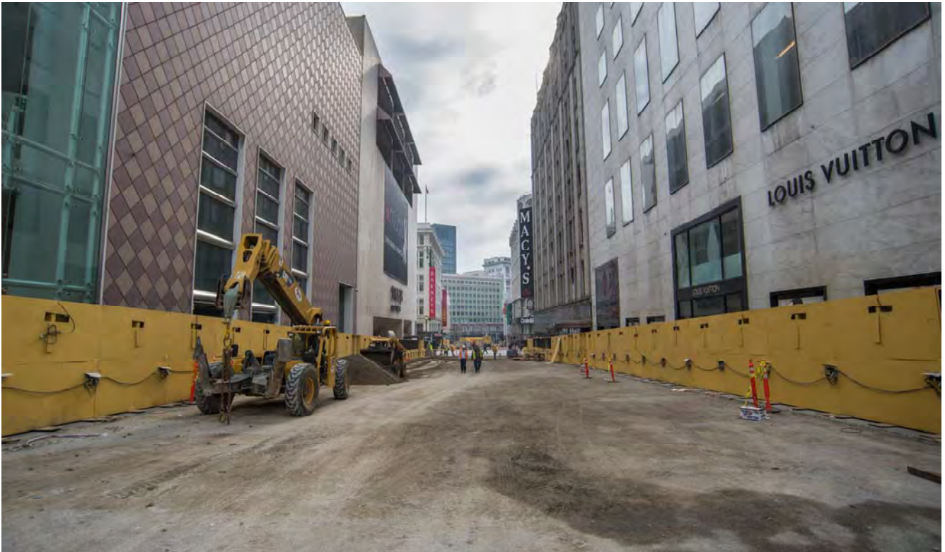
With the end of the holiday season also came the end of the 2014 Winter Walk. The green turf has been removed, and the contractor has re-erected safety barriers.
