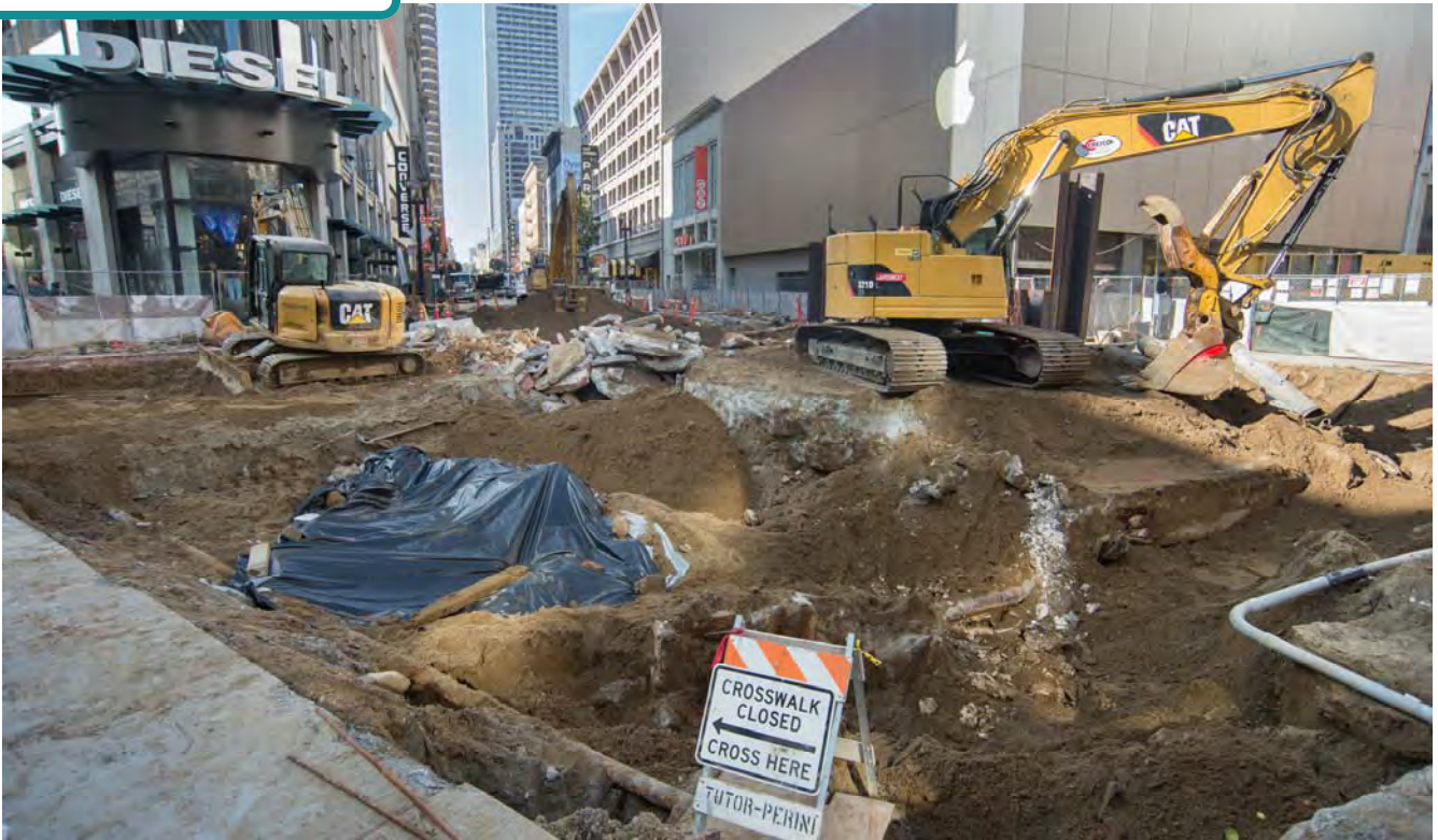
At the intersection of Ellis and Stockton, work to excavate soil and remove the former ground improvement shaft used during tunneling operations is underway.
