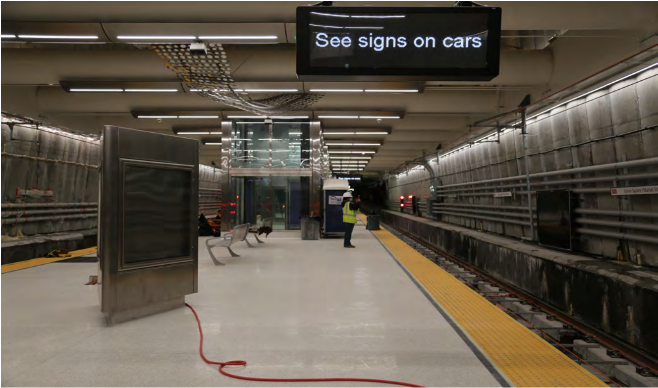
UMS Platform Elevator and Signage
