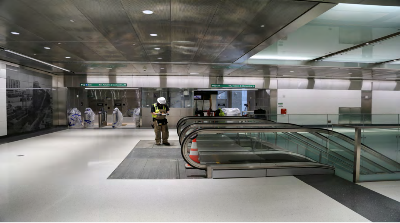
YBM Concourse escalators
