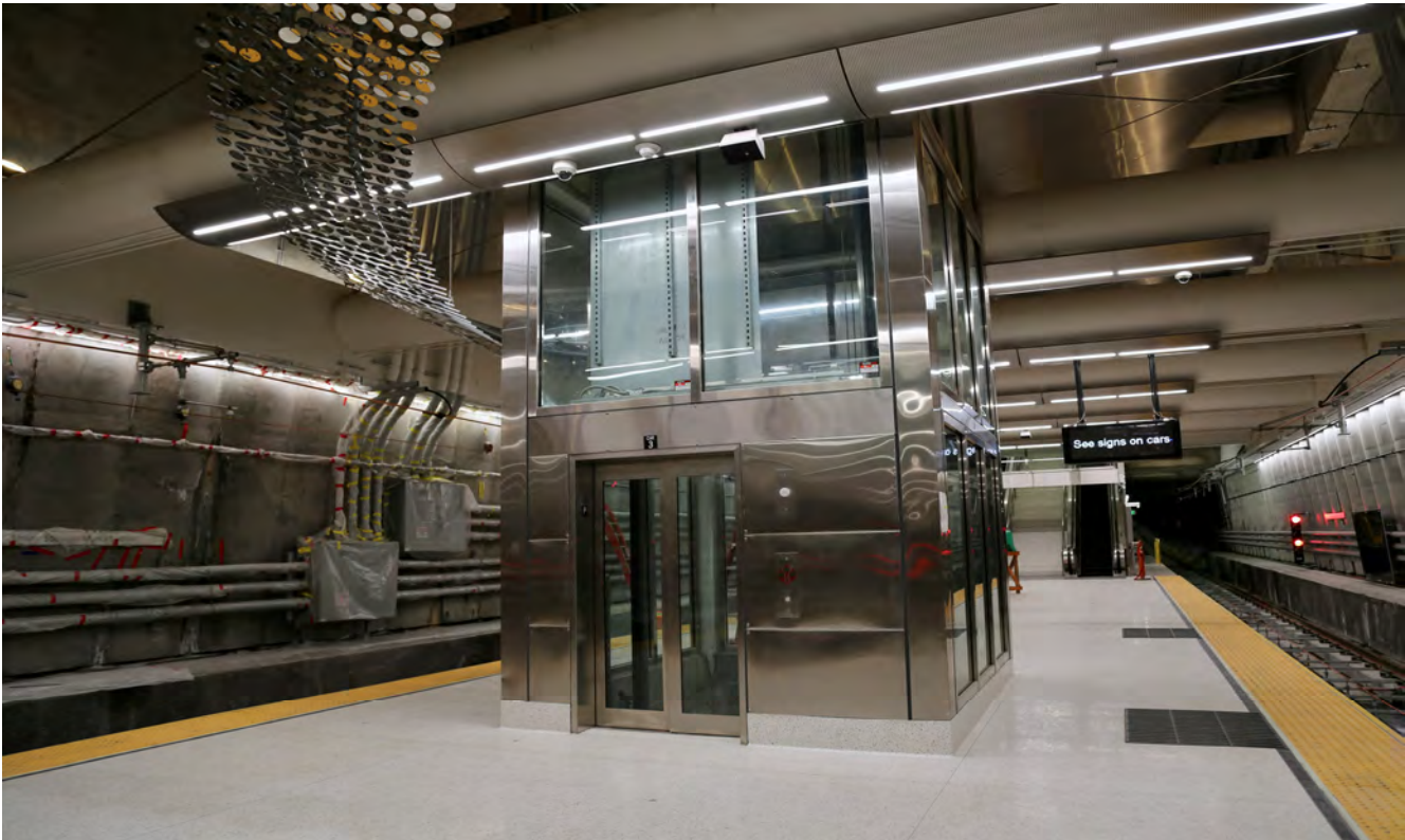
UMS Platform Elevator finishes
