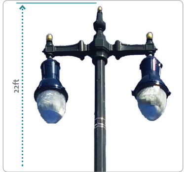
Existing Holophane Memphis 22ft Tall Pole + Double Teardrop Fixtures
