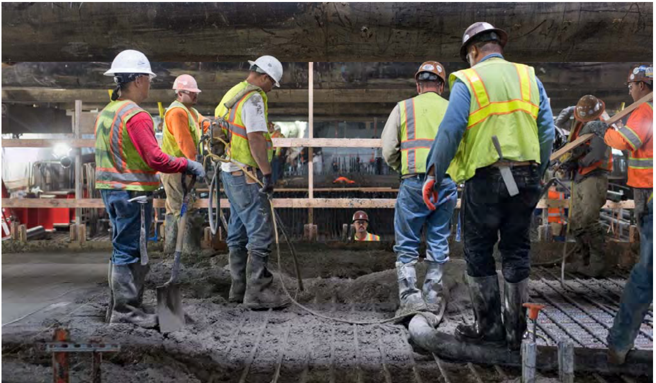
A crew works to distribute and smooth concrete to construct a new section of station box invert slab.
