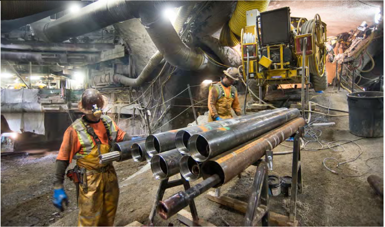
Two men ready a section of drill casing before lifting it up the ramp to the drill rig positioned as part of grouting work for the north platform cavern.
