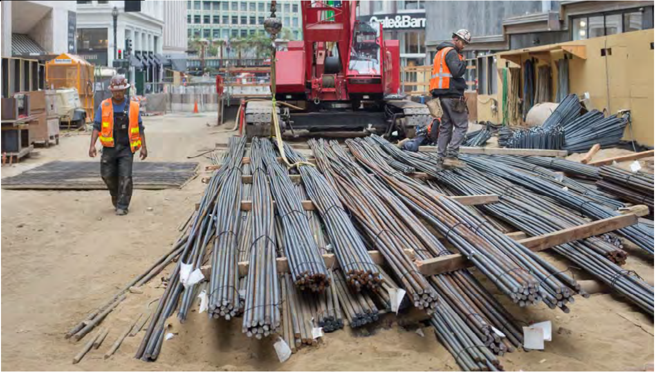
Prepared strands of rebar wait at the surface worksite just north of O'Farrell to be lowered into the station box as part of invert slab construction.
