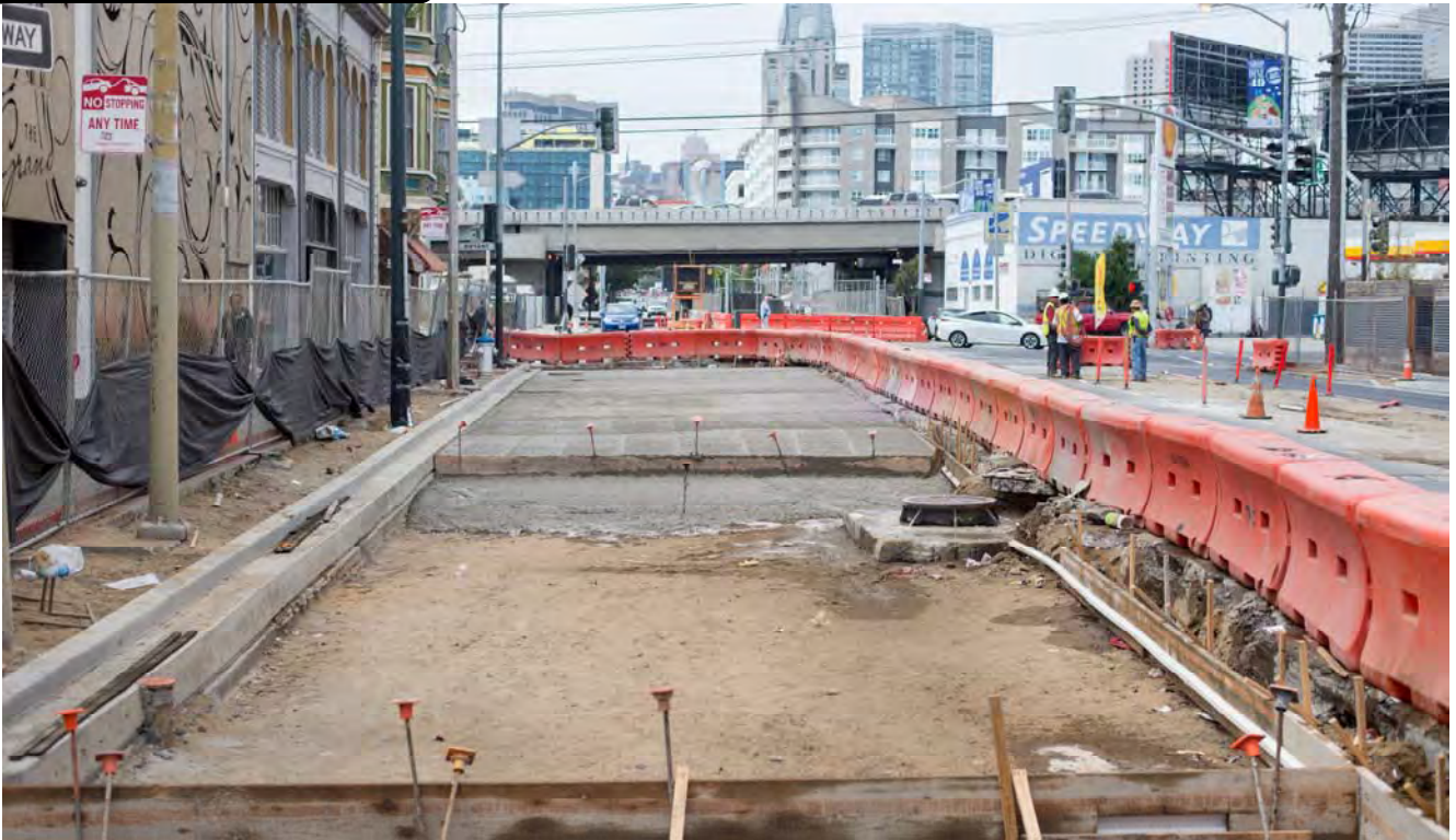
The concrete foundation of the roadway can be seen partially completed on the west side of 4th between Welsh and Brannan.
