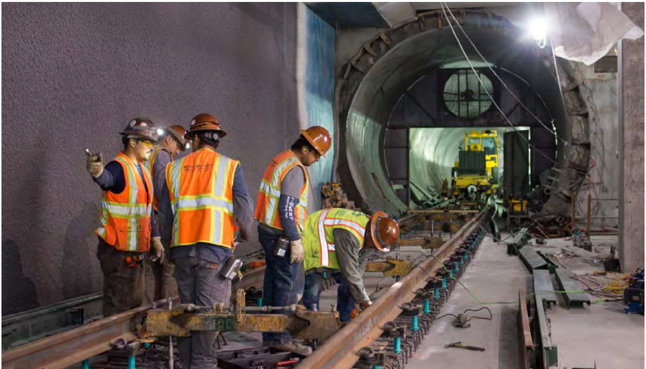
Sections of rail inside the station platform area are adjusted atop spacers and rebar which will eventually become plinths, or track foundations.
