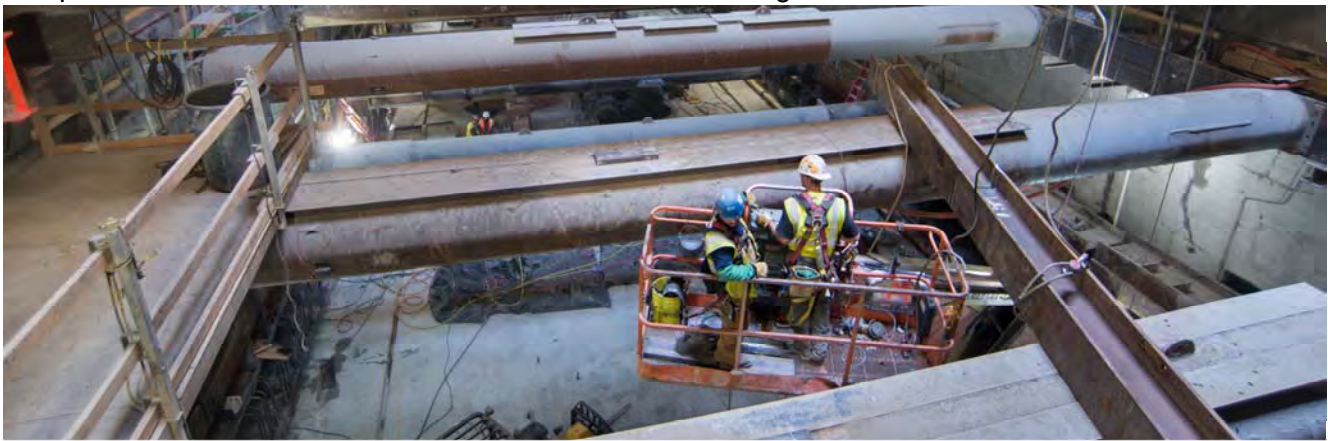
Looking south from the north Union Square/Market Street Station headwall, two men position a steel beam as part of temporary bracing for work platforms inside the station box.
