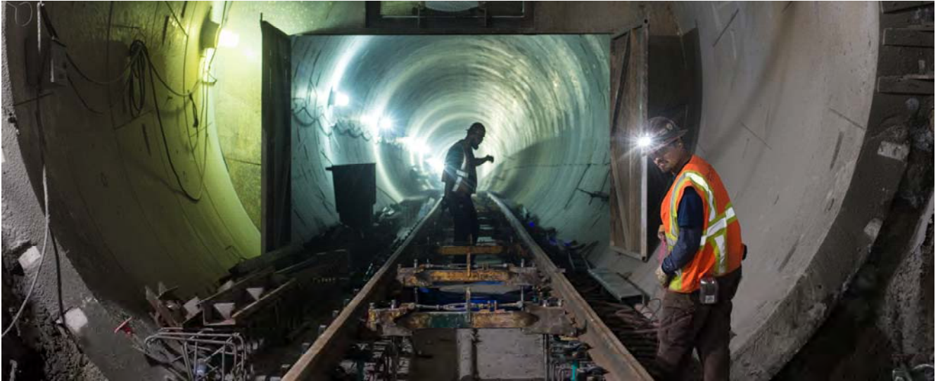
Tracks and track foundations are being installed inside the Yerba Buena/Moscone Station.
