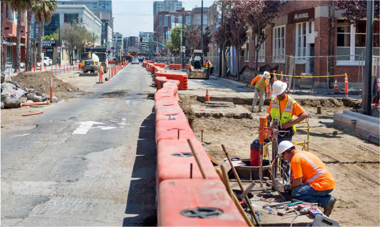
Looking south near Bryant, lanes of traffic along 4th Street have been altered and rerouted depending on street restoration and utility installation work.
