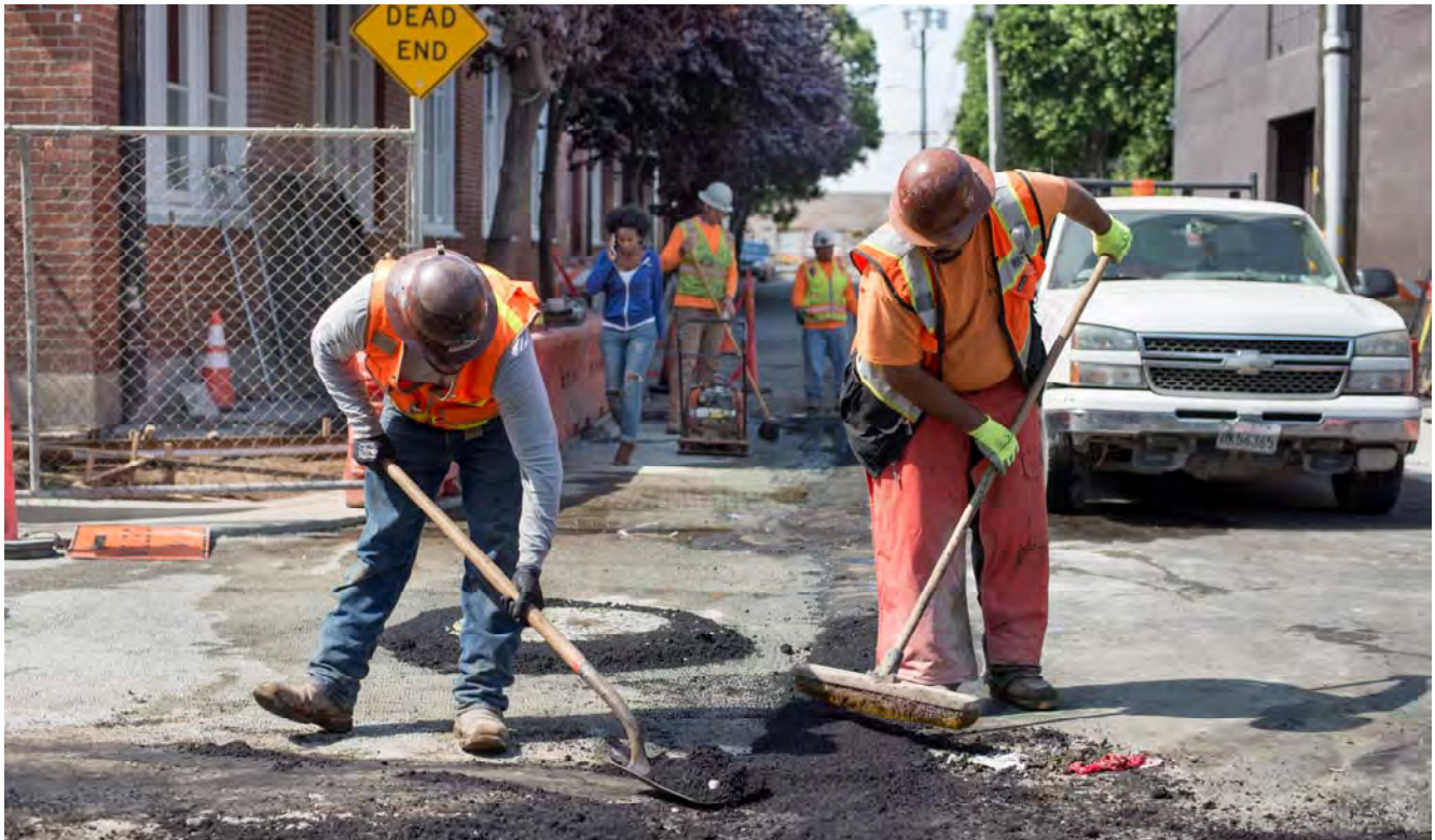
Workers spread asphalt around the edges of steel plates and a manhole during street restoration work at 4th and Welsh.
