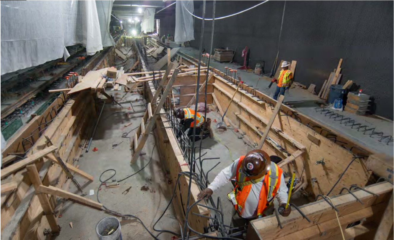
Carpenters work to assemble rebar cages and concrete forms as part of station platform construction inside the station box.
