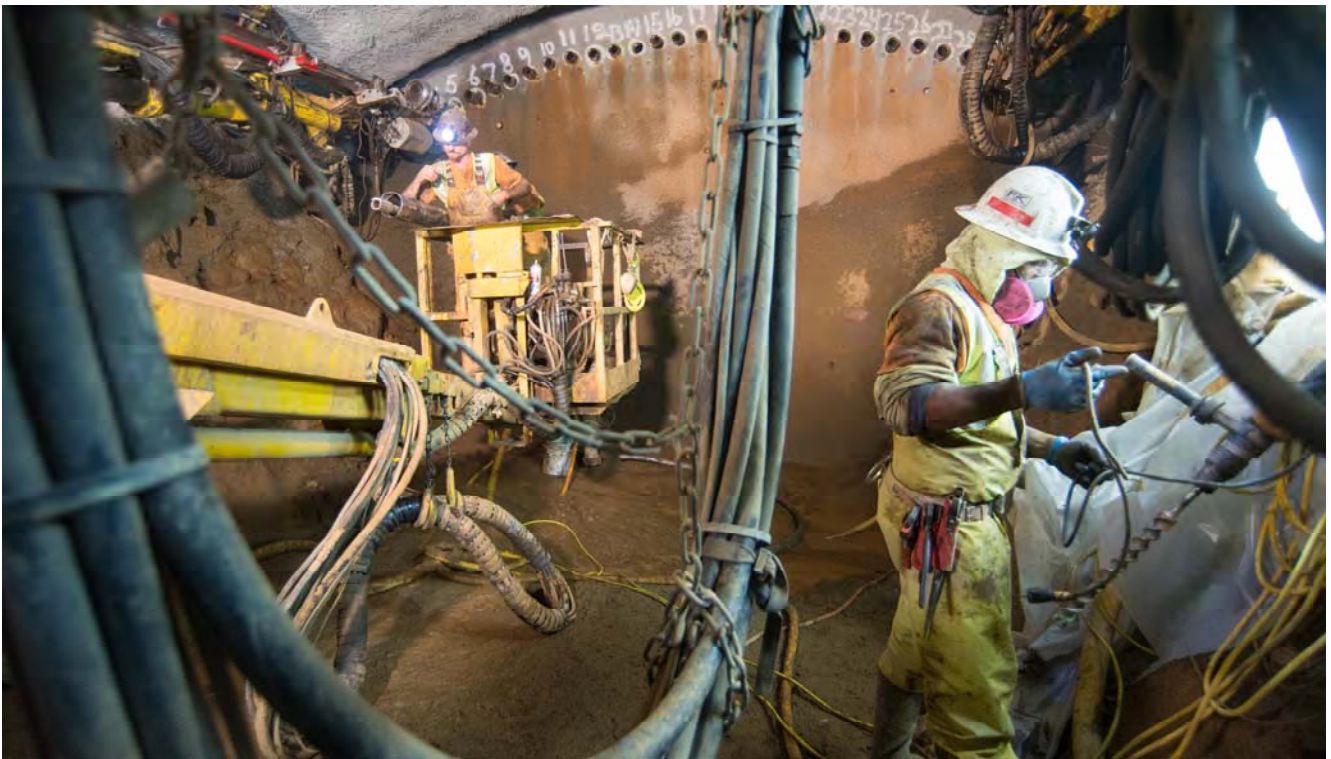
Hydraulic lines and high-pressure slurry and water lines criss-cross an already challenging work area where soil hardening work is ongoing for the central portion of the north platform cavern's ceiling archway.
