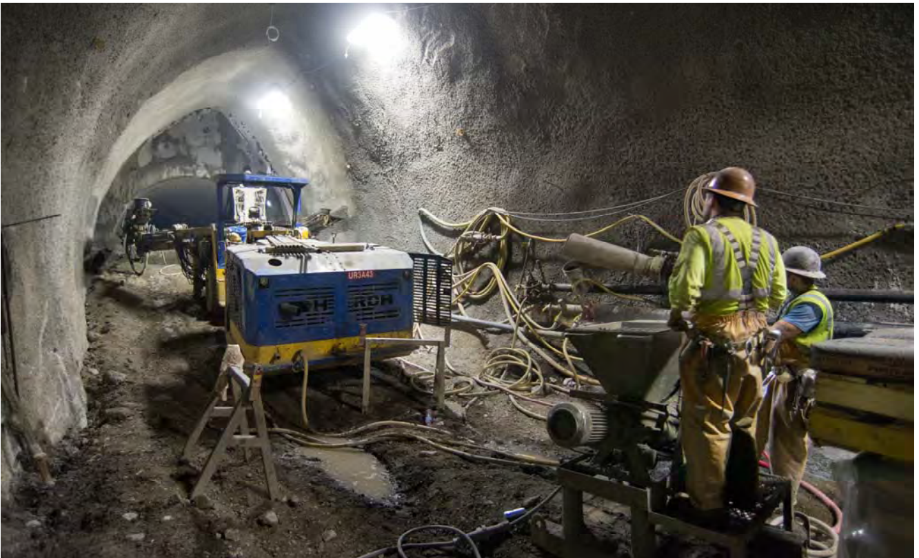
Workers on a drill rig crew hold back at a concrete pump hopper while conditions are reviewed at the end of the side drift excavation area.
