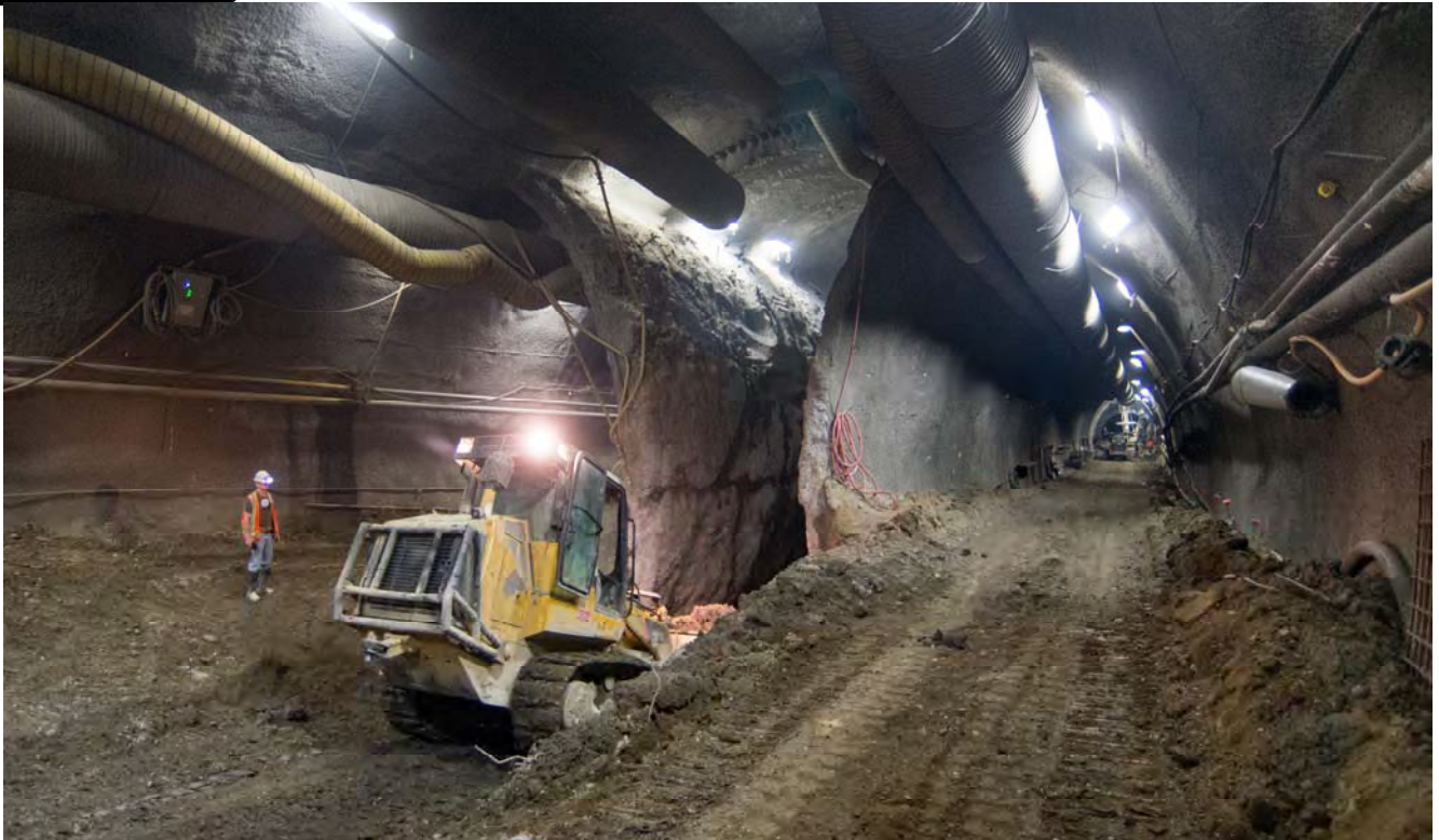
Looking south into the southern portion of the station platform cavern, a large bulldozer dives into the invert area of the center drift to remove material during excavation.
