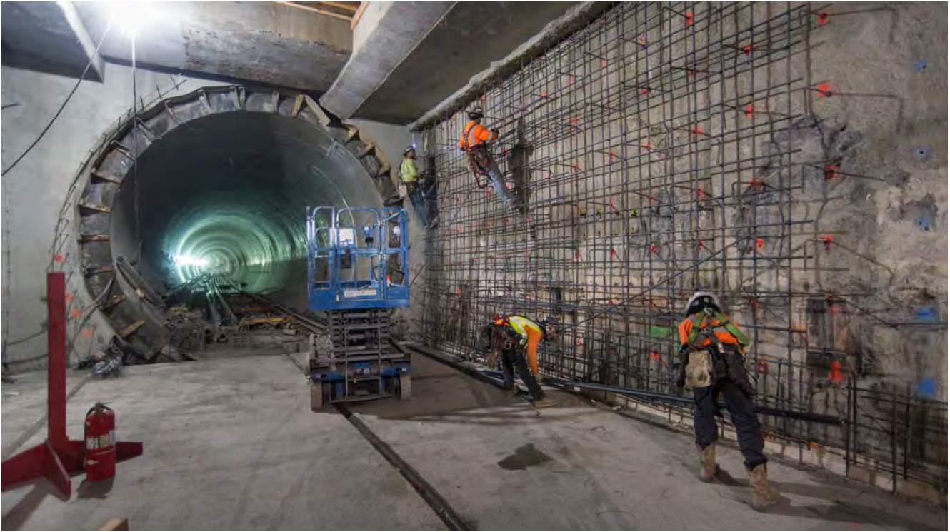
Workers hang from harnesses while assembling a large rebar cage along the west wall of the station box's south end.
