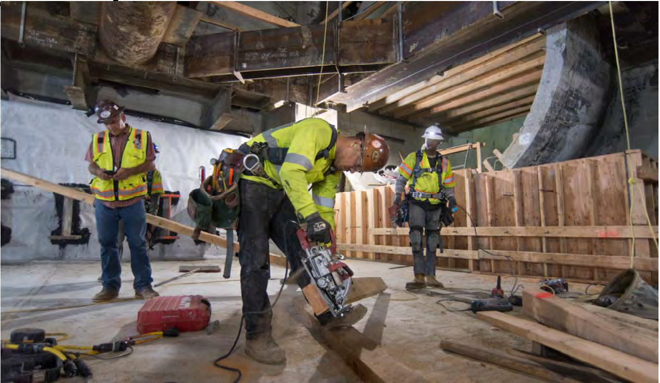
Carpenters cut boards to assemble cross-bracing as part of concrete form construction at the south headwall of the station box.
