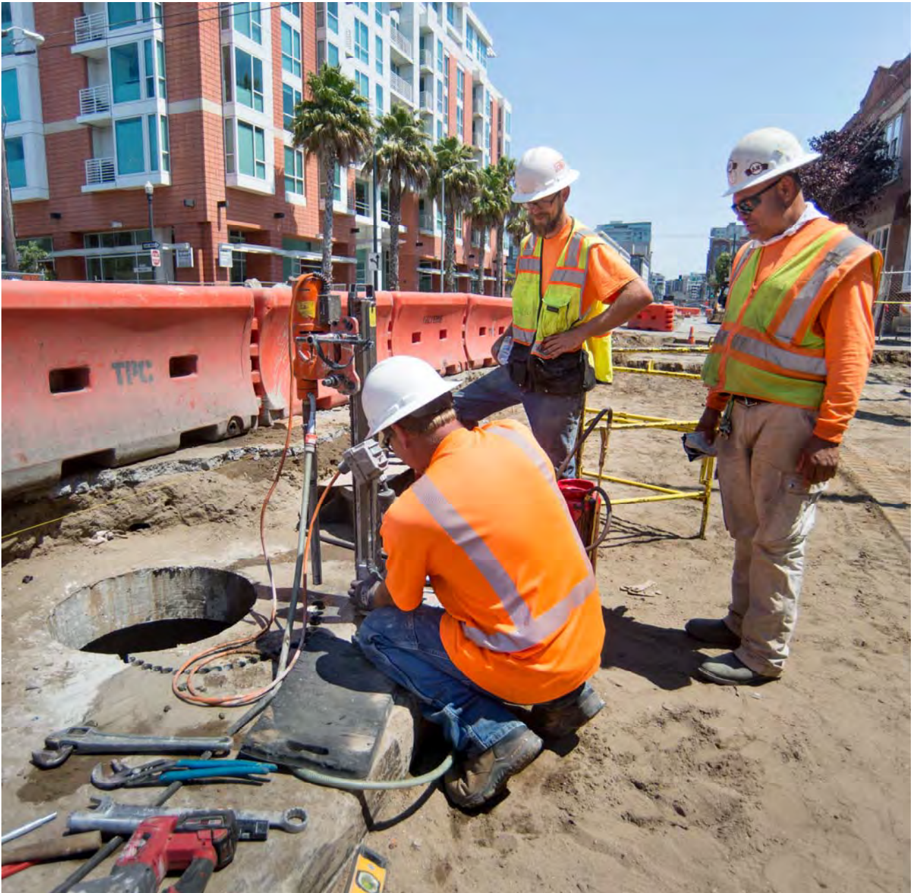
A crew works to relocate a manhole opening atop a utility vault near 4th and Welsh.
