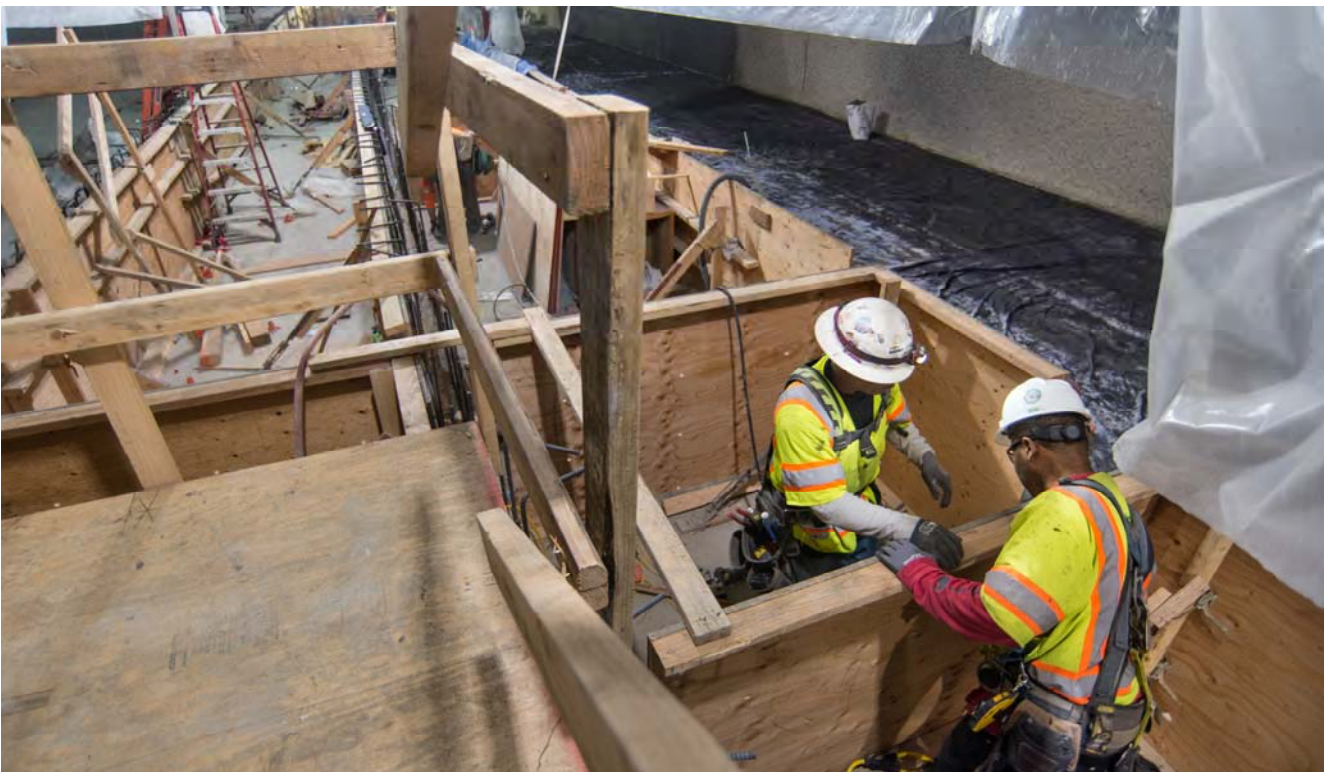
Two men place sections of concrete forms into place as part of station platform work toward the north end of the Yerba Buena/Moscone station box.
