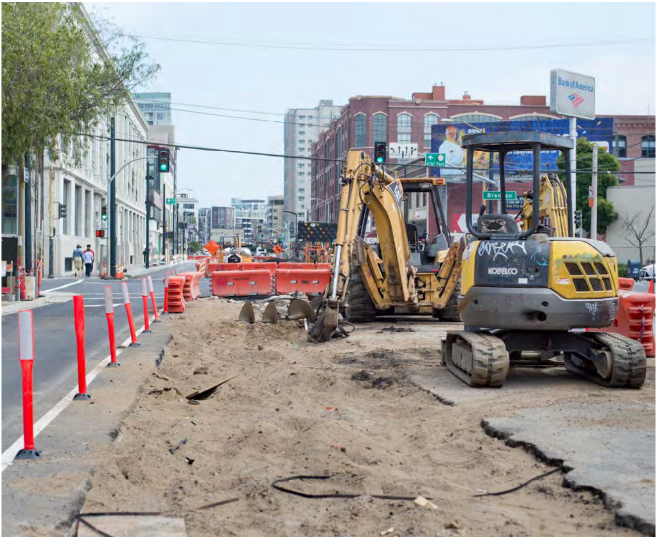
Excavation equipment rests just north of the 4th and Brannan intersection, where the surface station platform will eventually be located.
