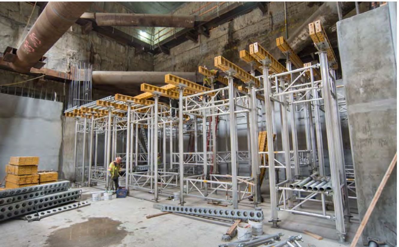
A lattice of struts and beams at the north end of the headhouse is assembled to carry the weight of concrete forms, rebar, and concrete which will be used to build the floor of the concourse level above.
