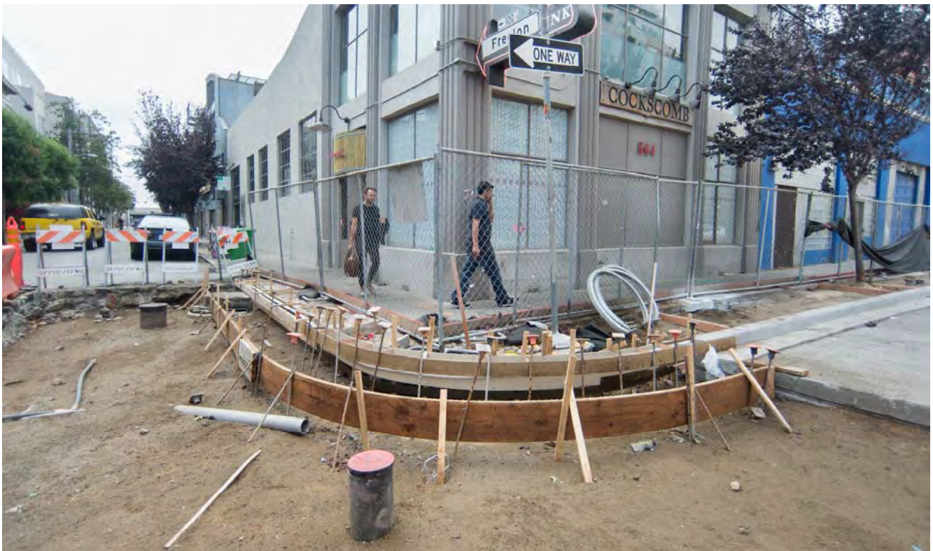
Curved concrete forms mark future curbs and gutters at 4th and Freelon.
