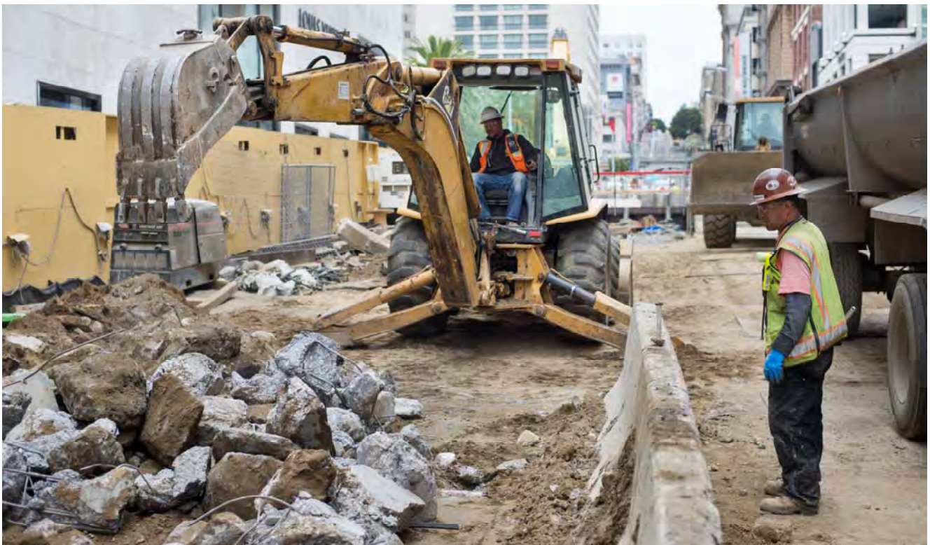
Pieces of demolished tunnel lining segments are sorted in a collection area near the truck loading zone atop the surface work site between O'Farrell and Geary.
