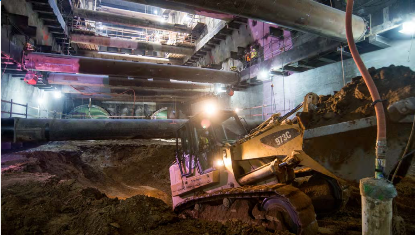
A bulldozer scales the incline leading from the invert level of the station box, as excavation of the lowest level of the station has begun.
