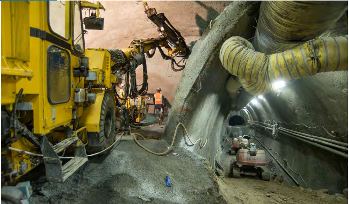
Crews install drill pipe casings as part of soil grouting work before excavating out portions of the south cavern top header.
