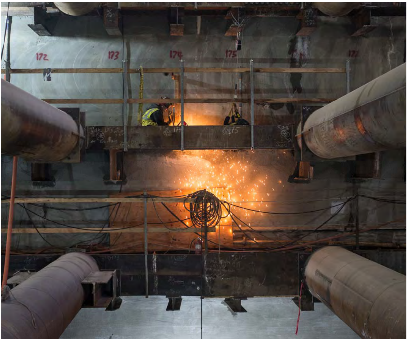
A welder cuts brackets atop a waler against the west wall of the station box, as part of temporary bracing work.
