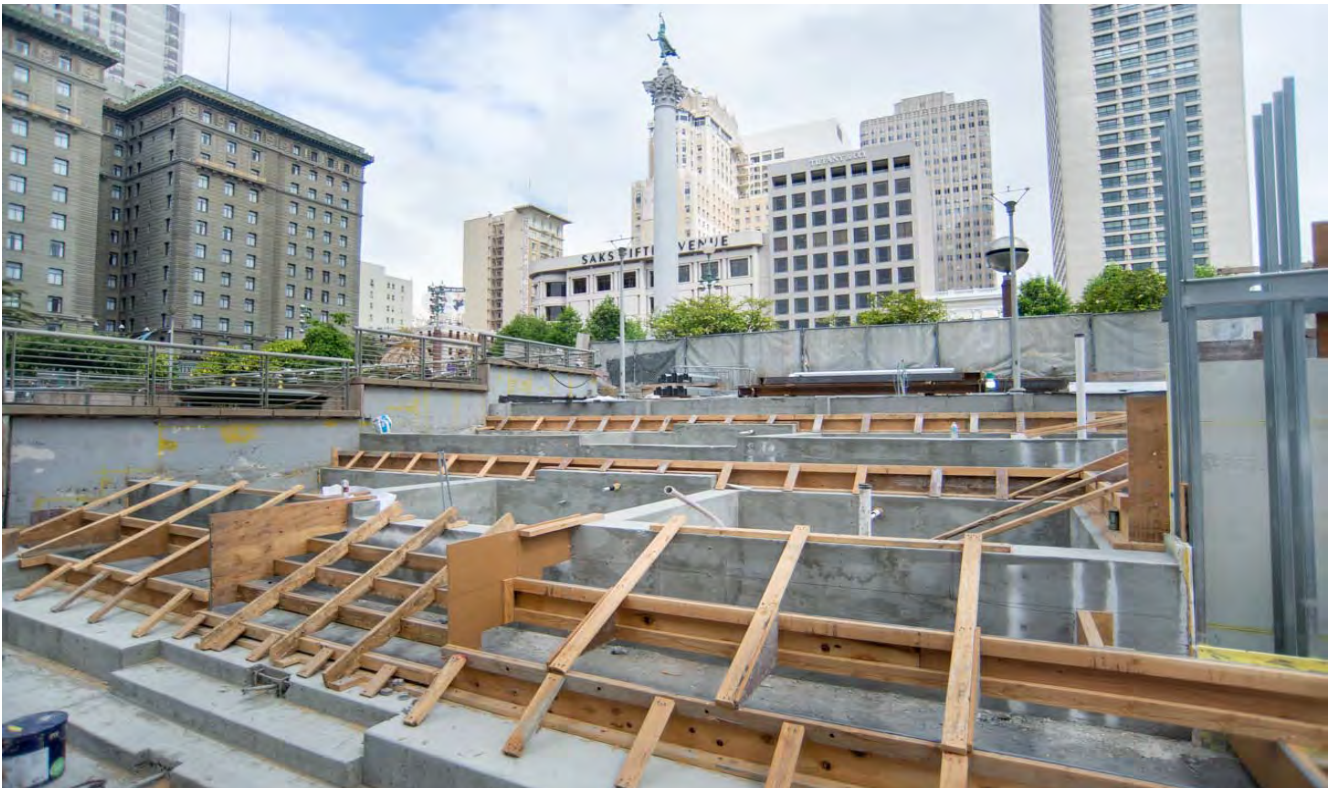
Concrete forms installed against recently-constructed terrace planter basins help prepare work for the next phase of terrace construction.
