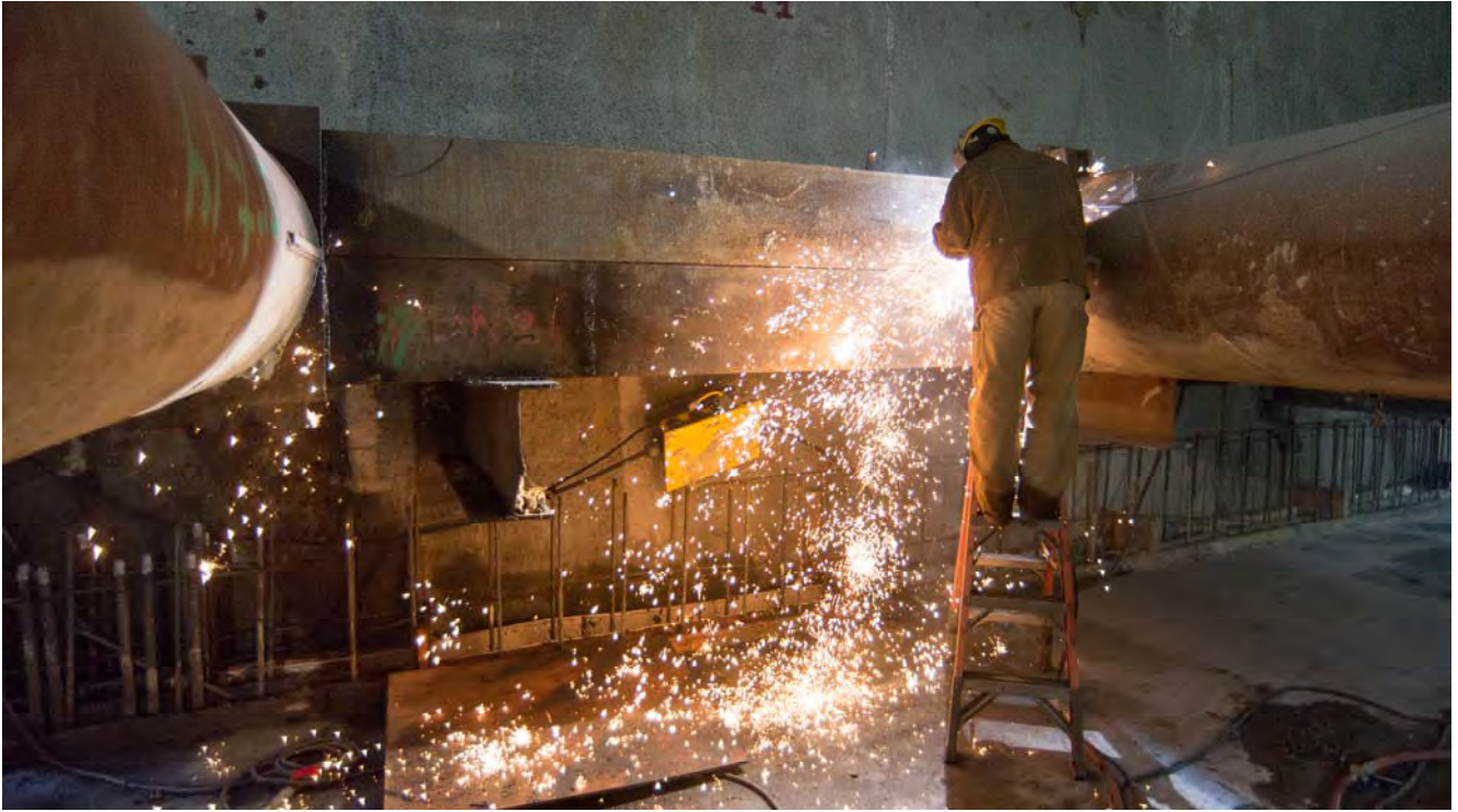
A shower of sparks on the west wall of the platform level jets from temporary bracing being removed following the completion of the station box and headhouse invert slabs.
