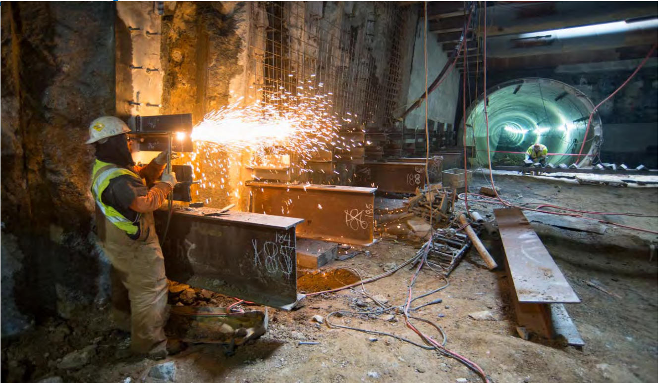
Sparks fly as a welder cuts steel brackets to proper dimensions as part of temporary bracing installation work inside the station box near the north headwall.
