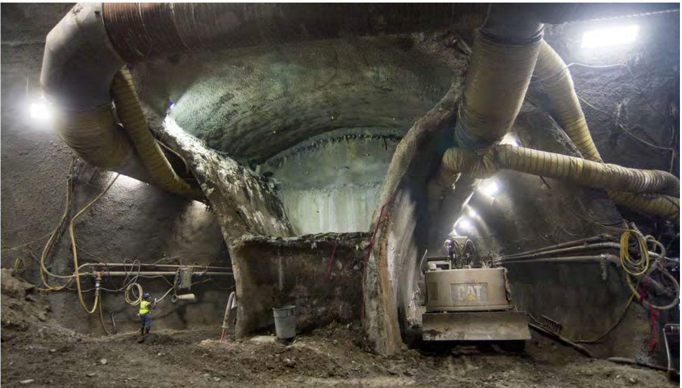
Looking south inside the cross-cut cavern, the right and left side drifts of the south platform cavern are clearly visible, separated by the top header and bench below (center).
