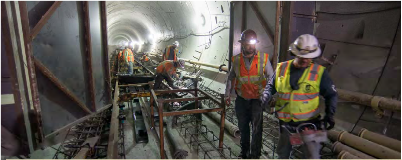
A crew finishes up following the end of a concrete pour inside the northbound tunnel, just south of the Yerba Buena/Moscone station platform area.
