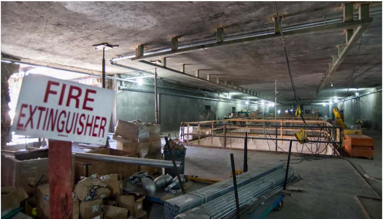
View looking north inside the concourse level of the station box under 4th Street, where internal structural elements and utilities are being installed.
