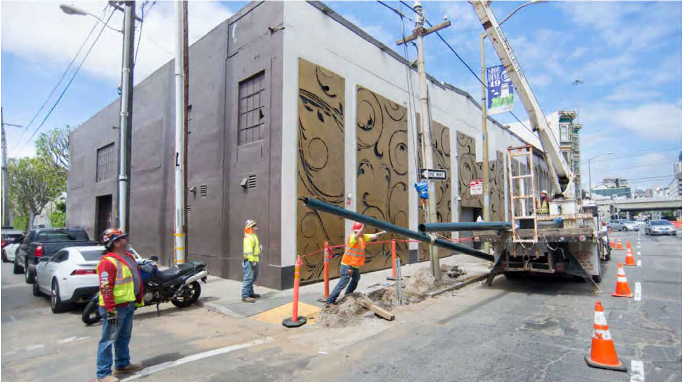
Crews have been installing new poles on 4th Street for the overhead catenary system (OCS) which will power light rail vehicles up and down the surface alignment.
