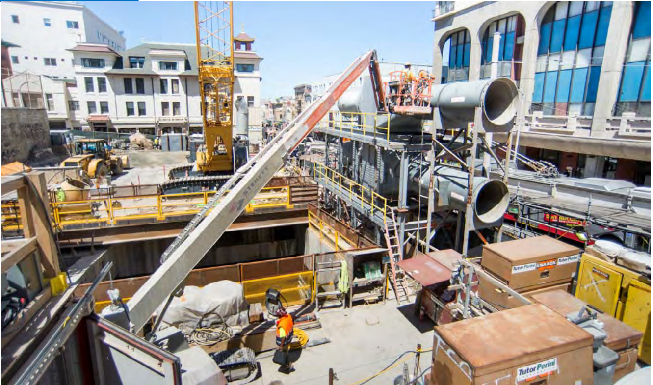
A large air-blowing system used as part of station interior ventilation is being disassembled on the east side of the work site.
