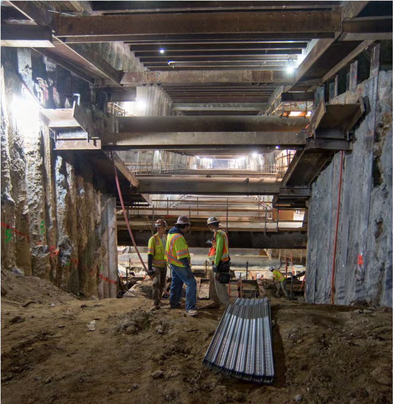
Workers scope out grading work at the south headwall, where stairs and escalators will eventually bring passengers to and from the station platform.
