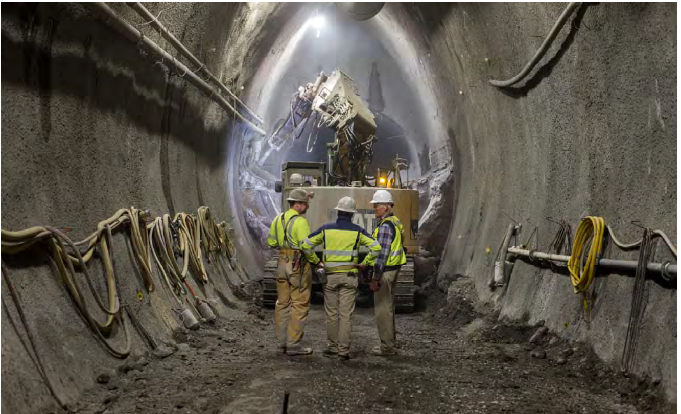
Station and tunneling engineers discuss the status of operations inside the left side drift of the south platform cavern, while an excavator removes shotcrete.
