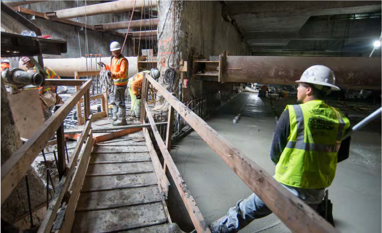
Workers finish smoothing the concrete surface of the last section of station box invert slab, at the access portal leading to the headhouse.
