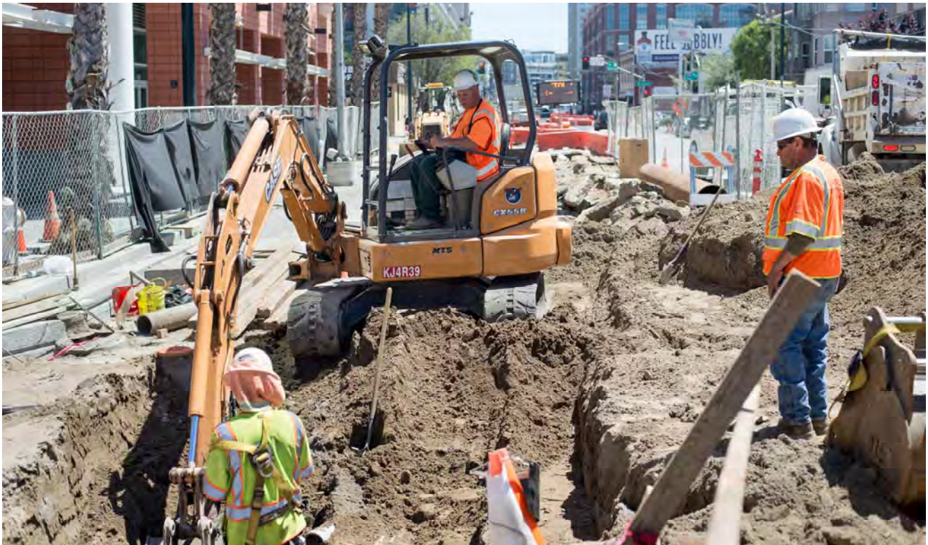
A crew digs a utility trench at 4th and Welsh, where water line and other utility work is being conducted.
