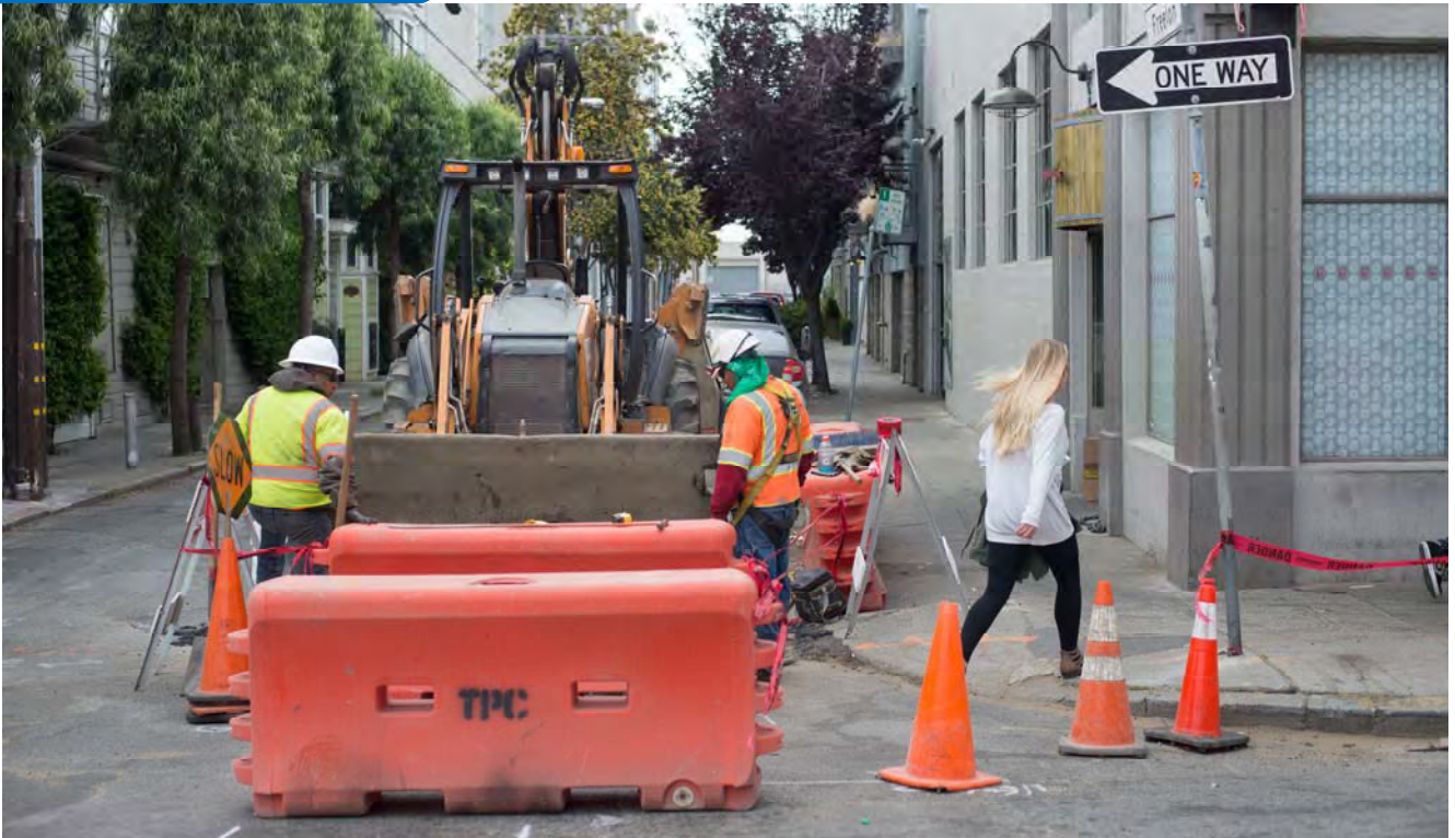
A crew conducts water line potholing work on the west side of 4th at Freelon.
