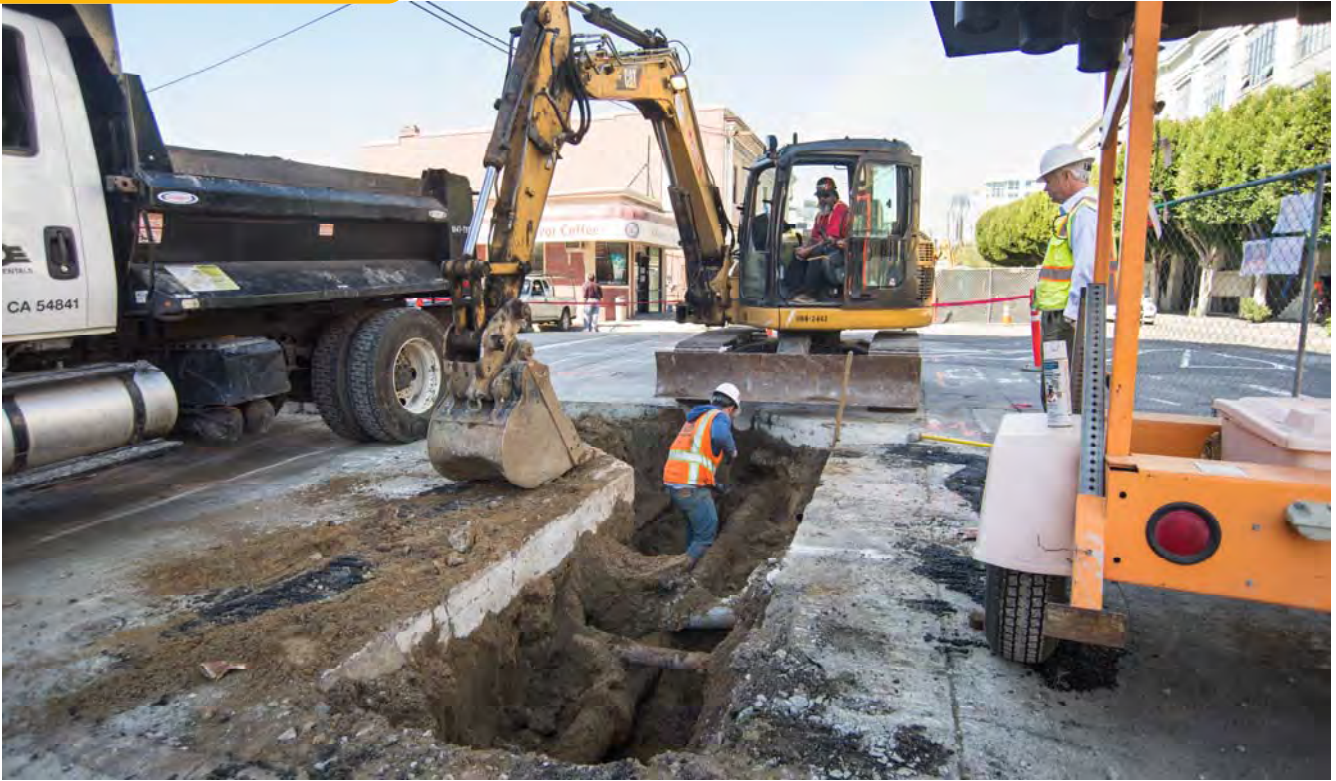
A crew works to uncover a utility pipe near Bluxome on 4th Street. Crews are working to relocate and reinforce existing utilities.
