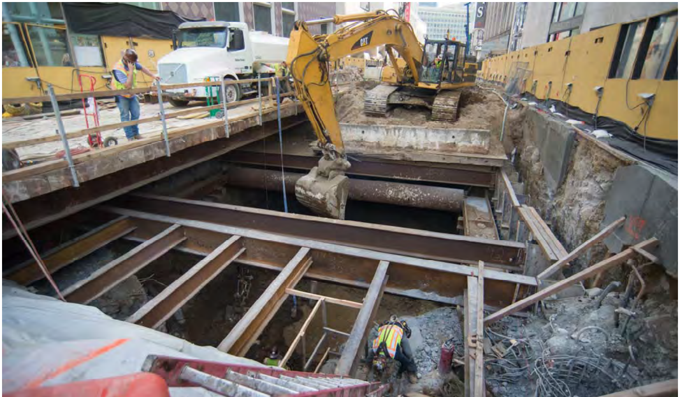
Just south of Geary on Stockton, a small access shaft has been created to a large excavator to lift excavated material to the surface, where it is loaded onto waiting trucks.
