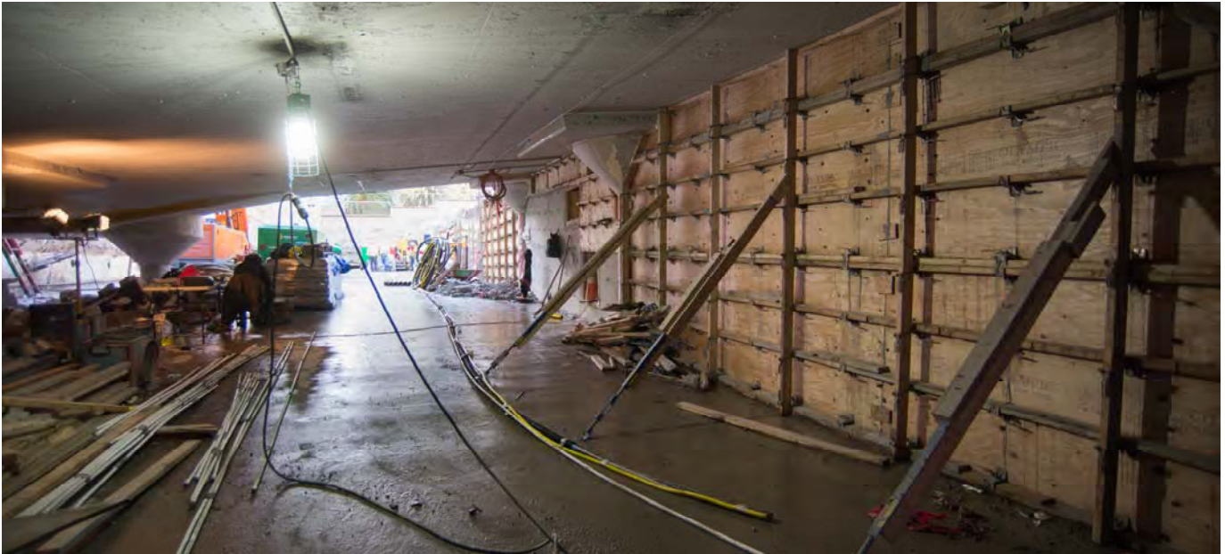
Concrete forms are in place both inside and outside the work area at the southeast corner of the Union Square Garage, where work to refit the garage with the north station entrance is underway.
