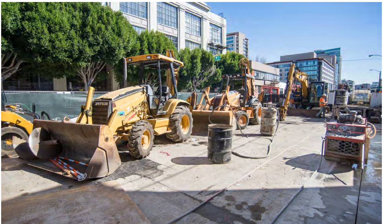
Equipment storage area and sawcutting machine for trenching operations between Brannan and Bluxome.
