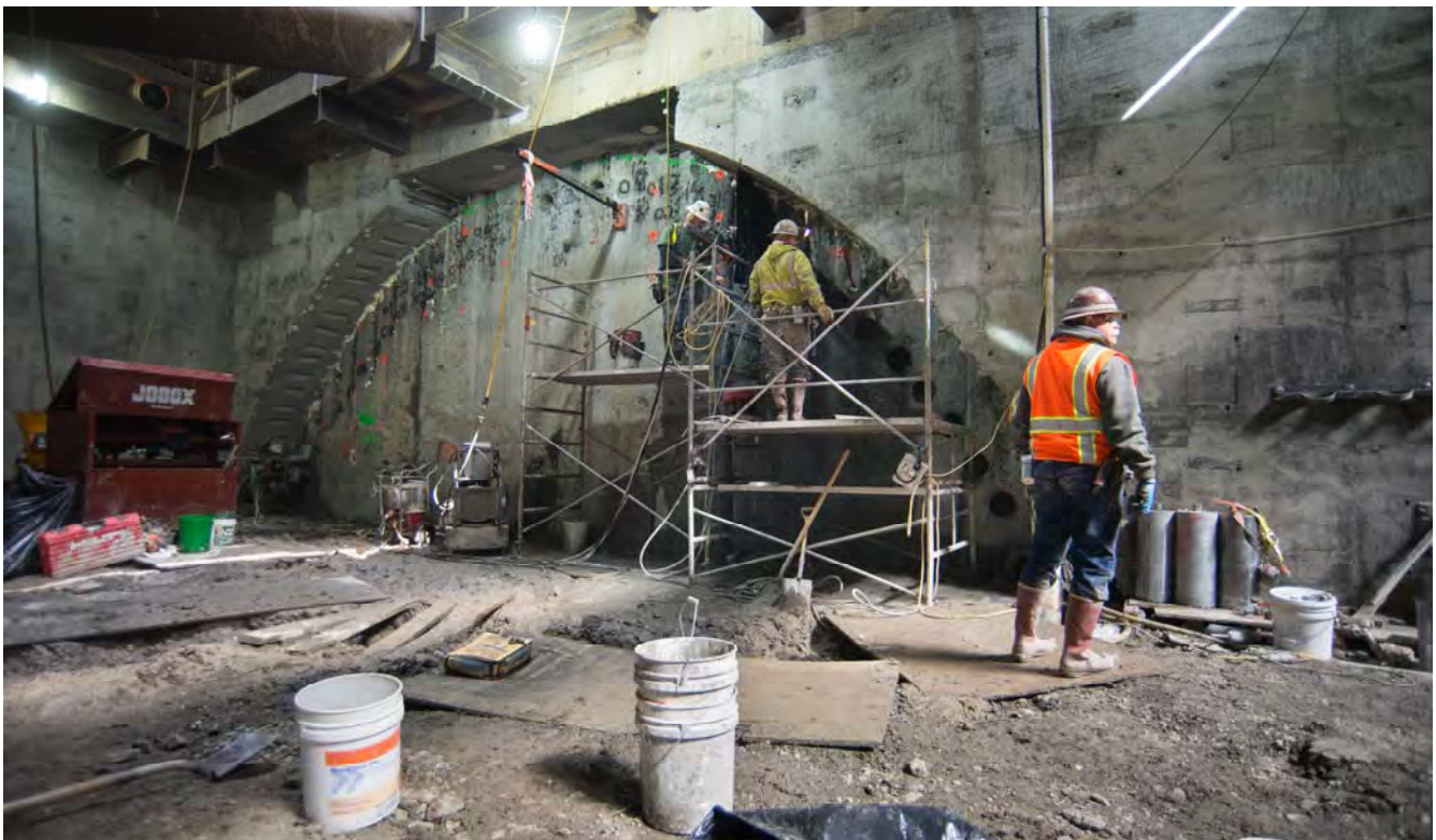
The entry archway to the station cavern is taking shape. Crews have constructed a reinforced concrete wall which will become part of the permanent station structure.
