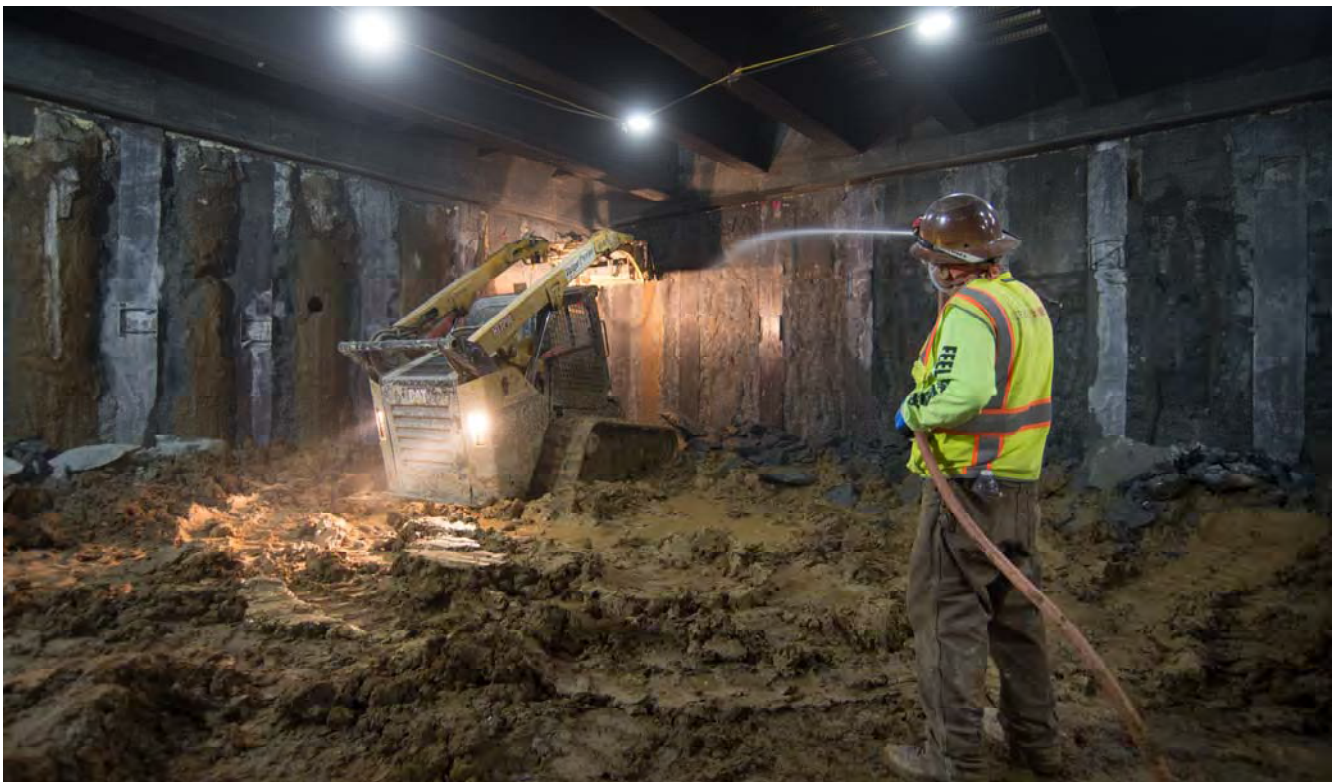
A bobcat operator uses a small jackhammer to remove loose material along the east wall at the northern end of the north concourse, while an associate keeps the dust down.
