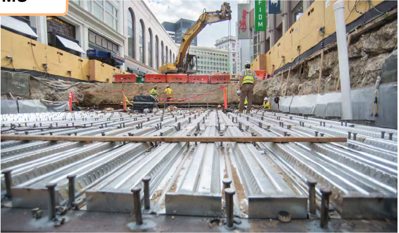
Steel pegs are installed intervals on top of the corrugated steel sheeting of the station box roof deck, prior to installing rebar and pouring concrete.
