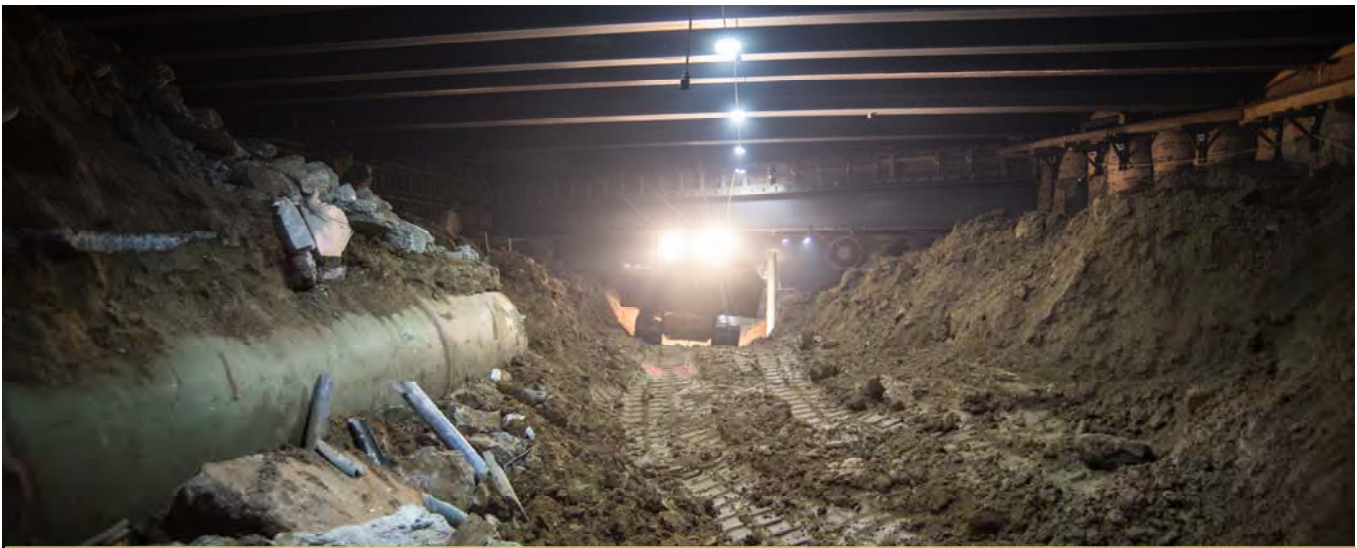
Lights from a bobcat illuminate the underside of Stockton at Geary, where excavation of the north station concourse is underway for the Union Square/Market Street Station.
