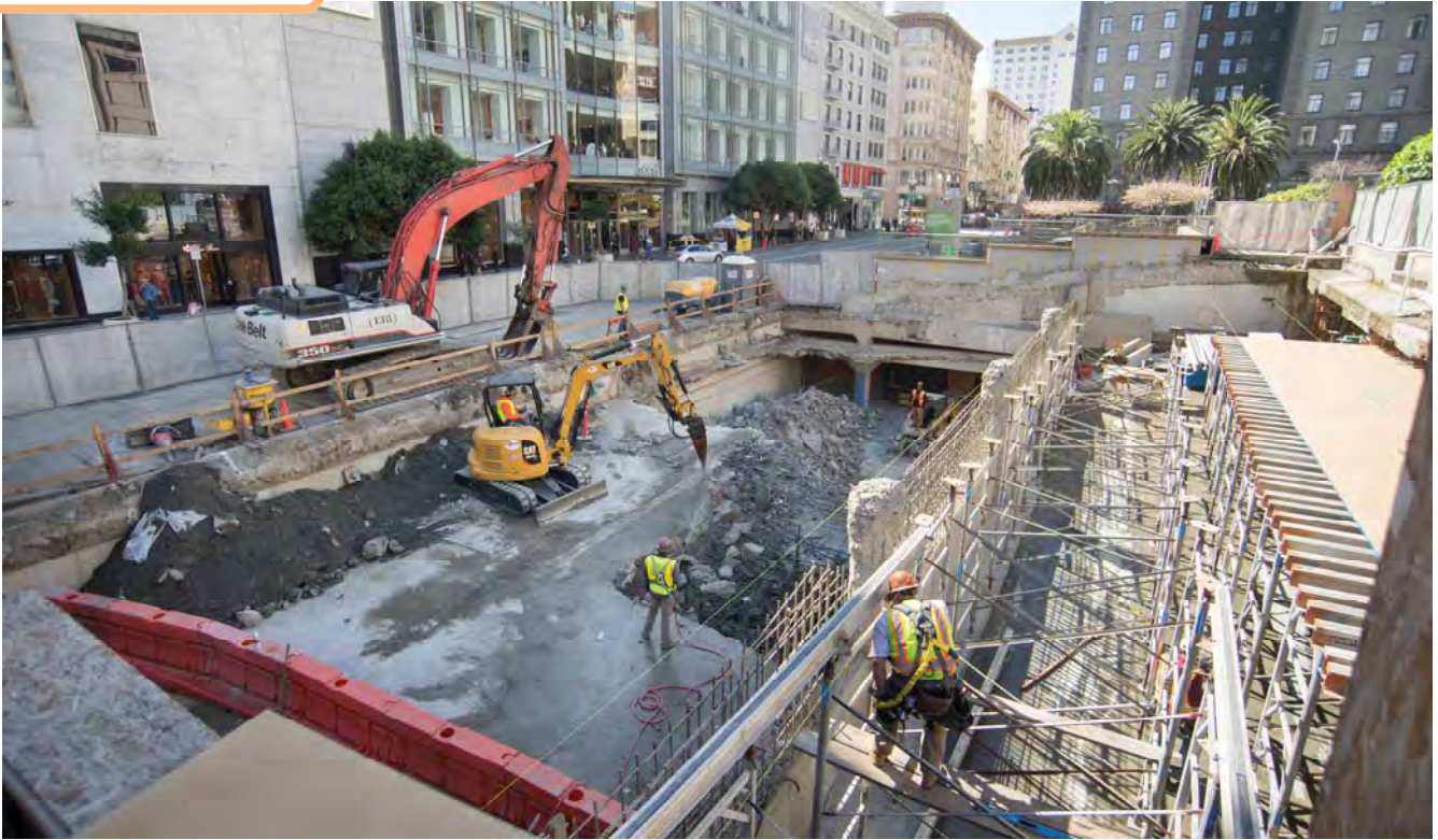
A worker aligns scaffolding for concrete forms on a newly-rebuilt ramp of the Union Square Garage alongside demolition work to prepare for construction of the north station entrance.
