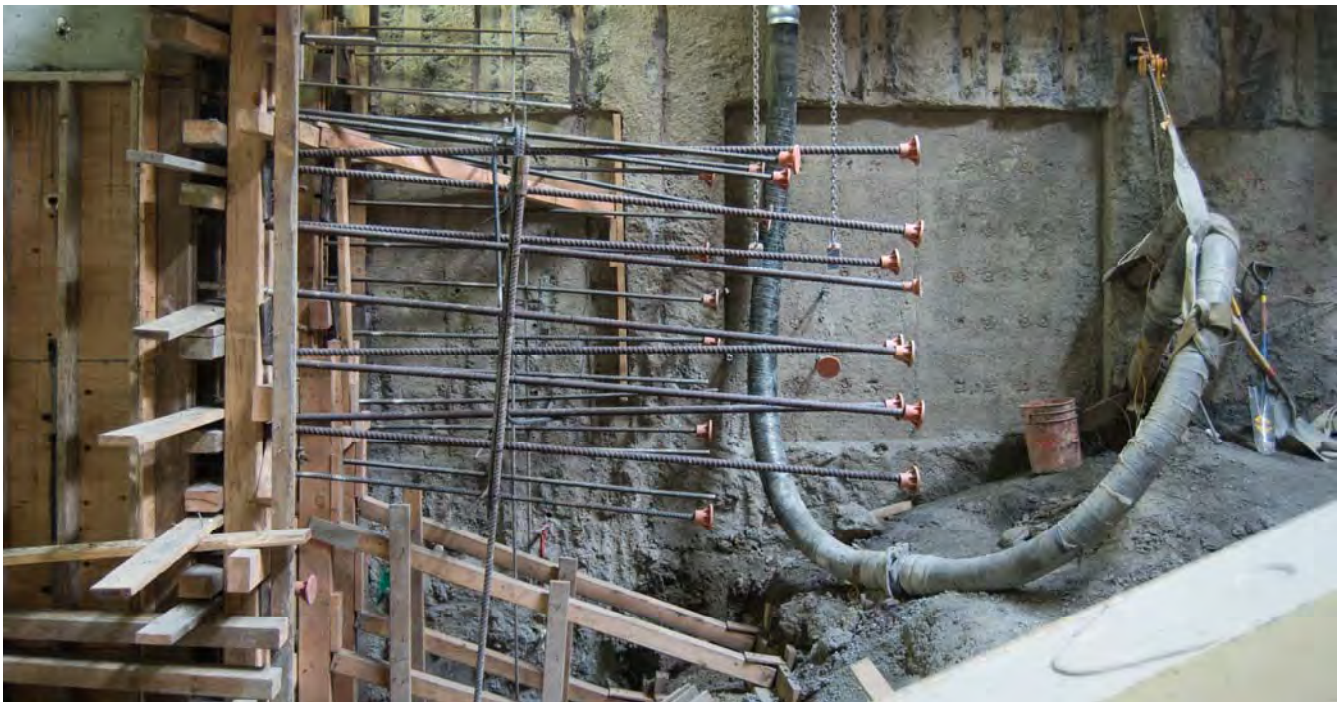
Rebar sticks out of the side of a finish wall being constructed against the exterior slurry walls at the bottom of the Chinatown Station headhouse.
