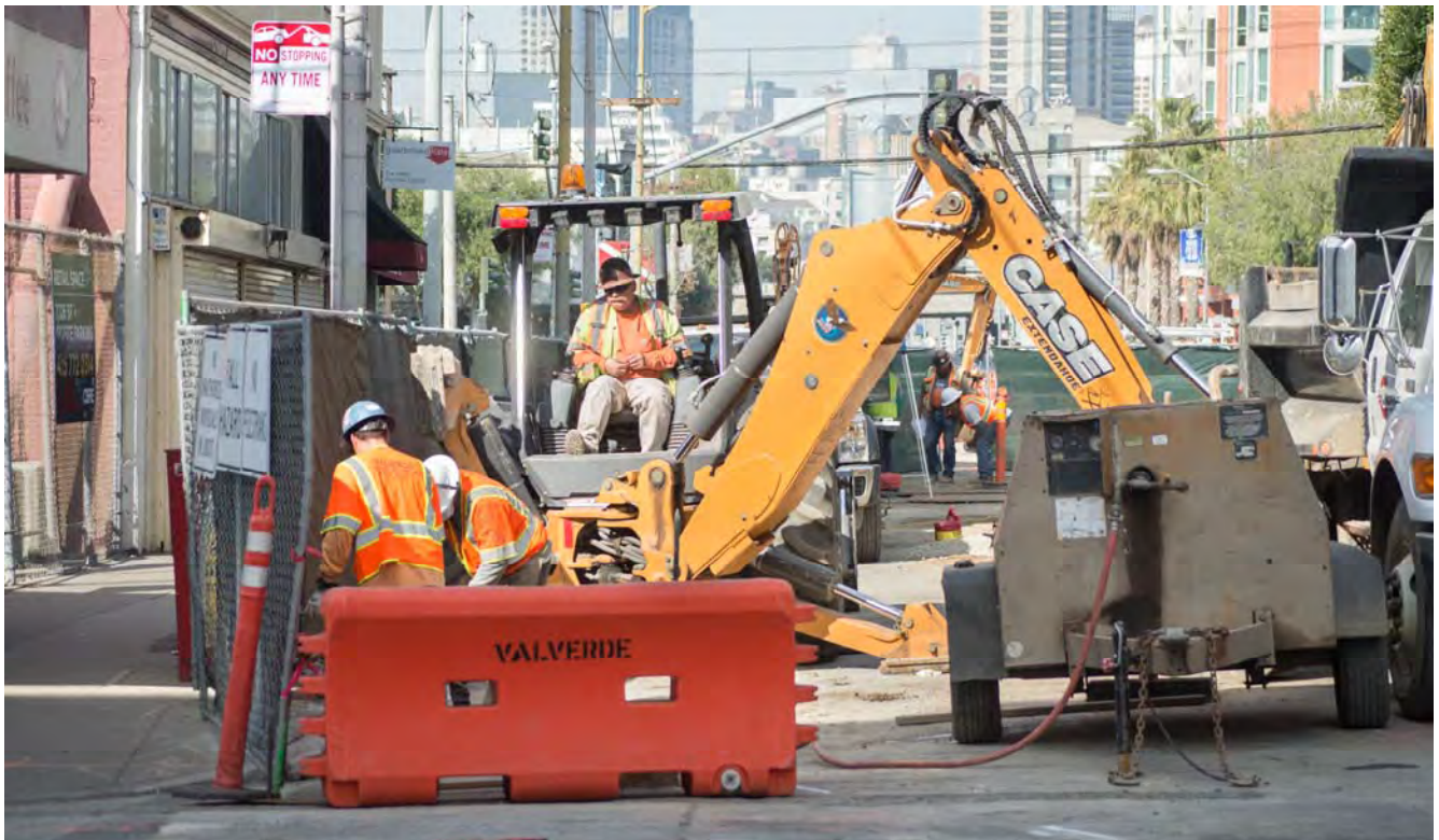
An excavator operator observes backfilling work on 4th Street just north of Bluxome.
