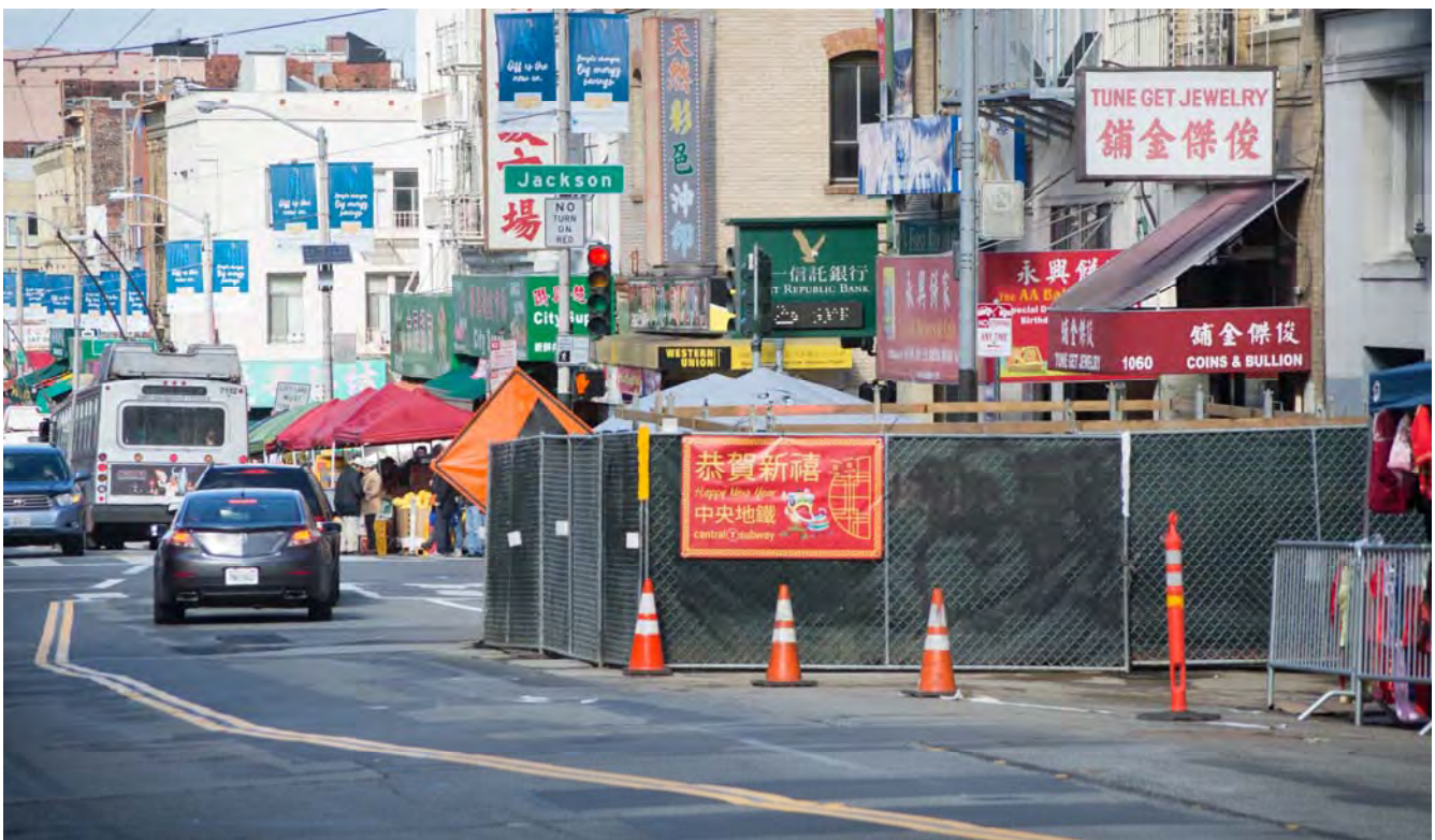
Work at the north access shaft between Washington and Jackson is currently on pause for the Chinese New Year.
