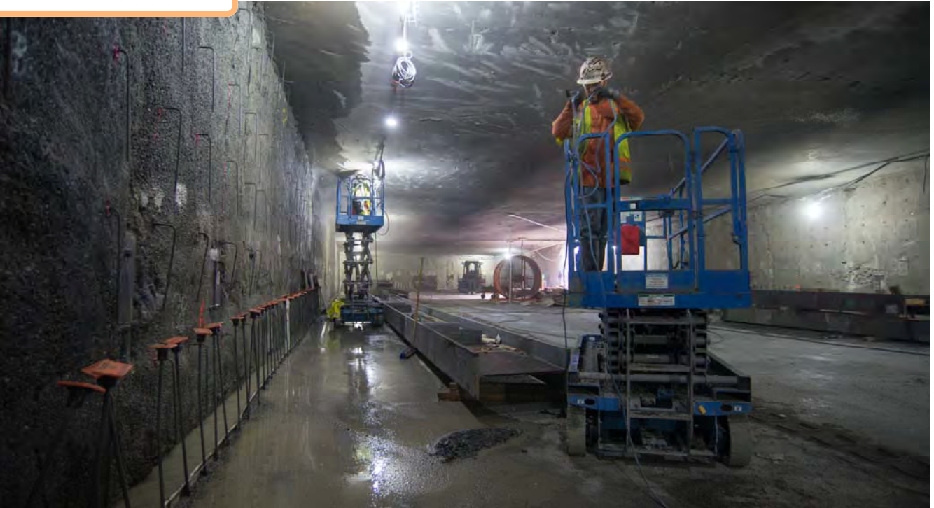
Inside the upper level of the station box, workers use high-pressure water jets to clean surfaces and remove any loose debris before installing rebar and building a finished wall.
