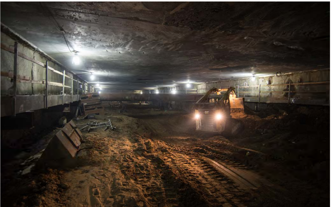
A bobcat dumps material at a transfer point inside the station box, where workers are grading the north end to begin installing concrete forms for the mezzanine floor slab.
