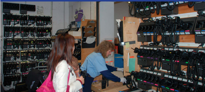
Interior of equipment room at 505 7th St.
