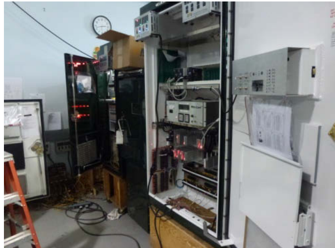
Traffic Signal Cabinet in the Programming Area
