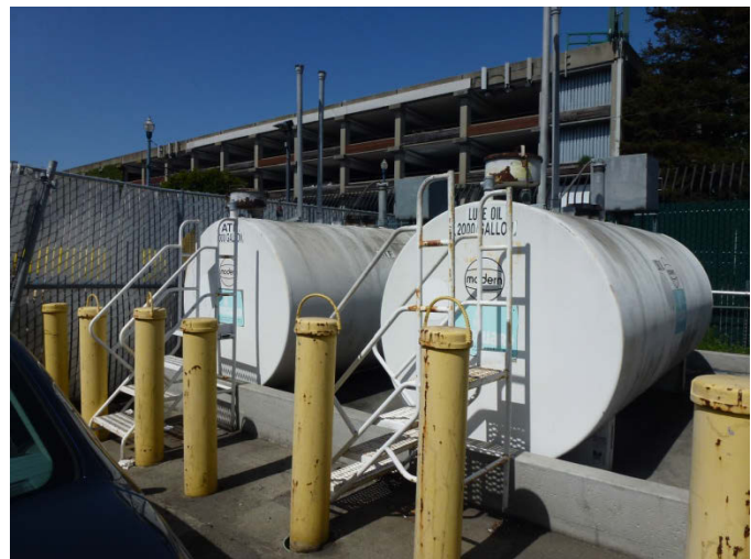
Lube Storage Tanks
