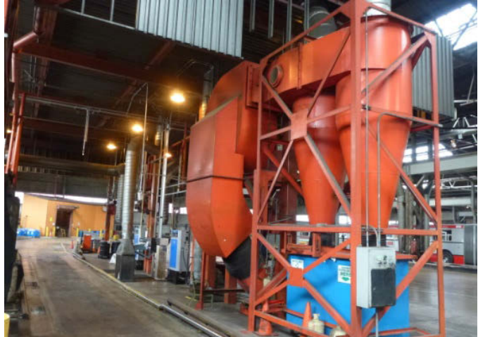
Bus Fuel Lane and Vacuum System
