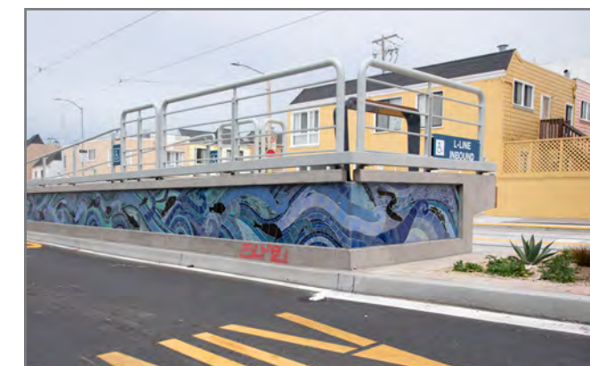
Mosaics and greenery: The project incorporated numerous features to enhance the streetscape and reflect the local character, including thematic mosaic tiles on wheelchair ramps, landscaping on boarding islands and new street trees.
