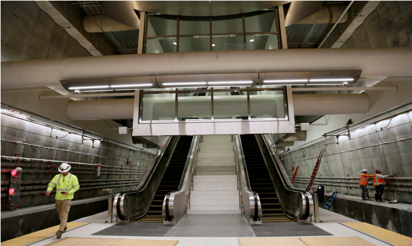
UMS escalators leading to Platform Level
