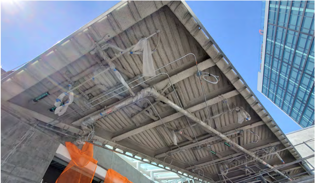
A fireproofing material has been sprayed against the underside of the station entrance roof near the street-level elevator entrances for Yerba Buena/Moscone Station.
