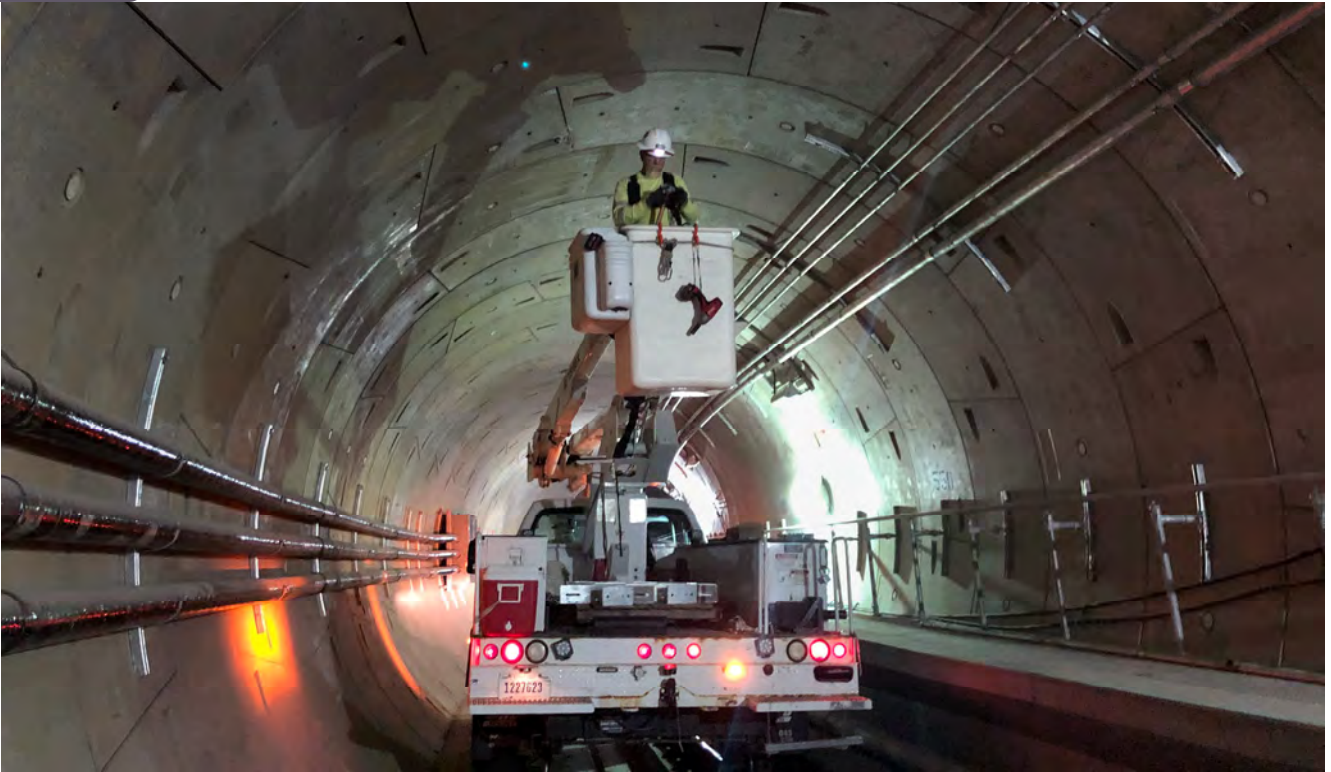
A crew in a work truck positions itself to begin installation of a mounting bracket for the overhead catenary wire.
