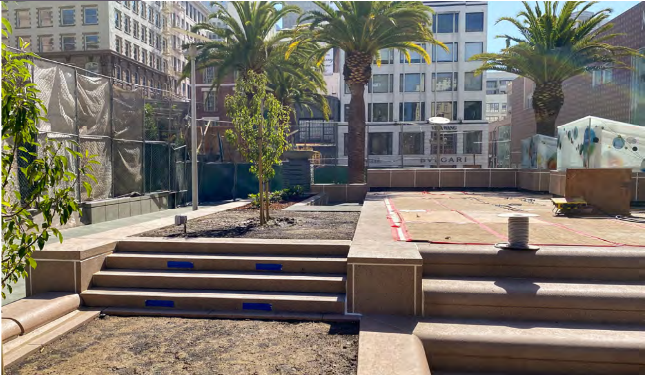
Soil and trees are being placed as part of Union Square/Market Street Station's north entrance roof construction, and Union Square terrace restoration.
