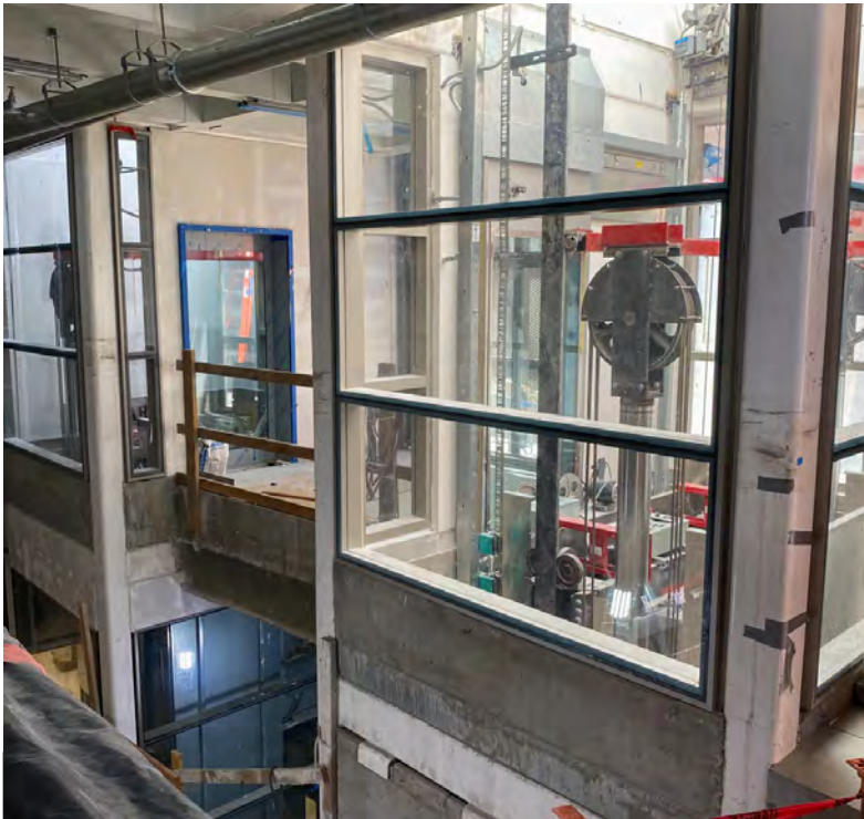
Below, mechanical systems and utilities for the station entrance are being fitted out.
