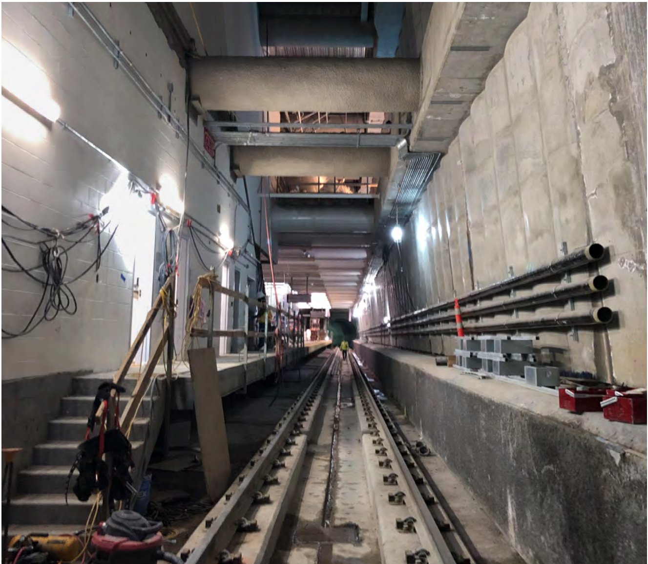
Utilities, conduits, and permanent lighting are being extended from the north end of Union Square/Market Street Station, where the platform meets the southbound tunnel.
