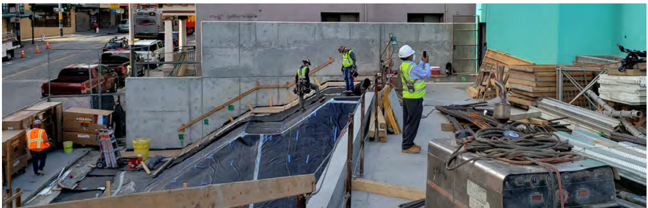
A crew lays out rolls of waterproofing membrane where future stairs will be built leading to the rooftop plaza at Rose Pak-Chinatown Station.
