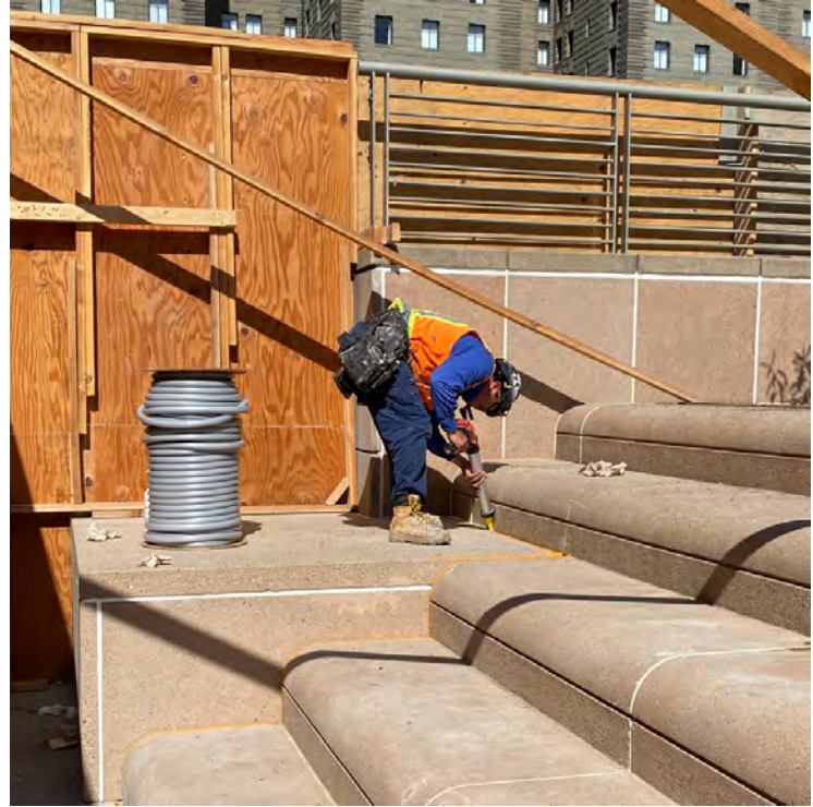
Workers put the finishing touches on sealing the terrace blocks, adding lighting, and other systems.
