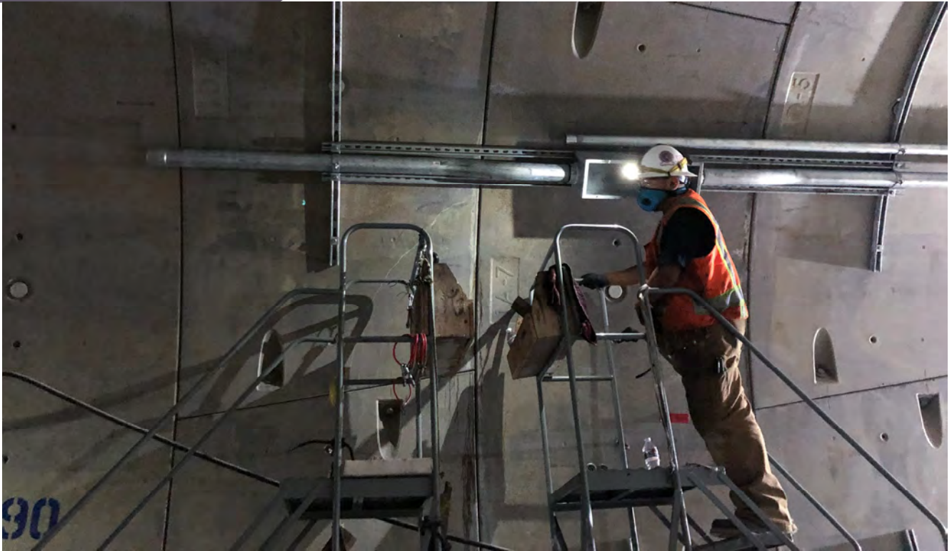
A technician prepares to install portions of a permanent lighting assembly inside one of the subway tunnels.
