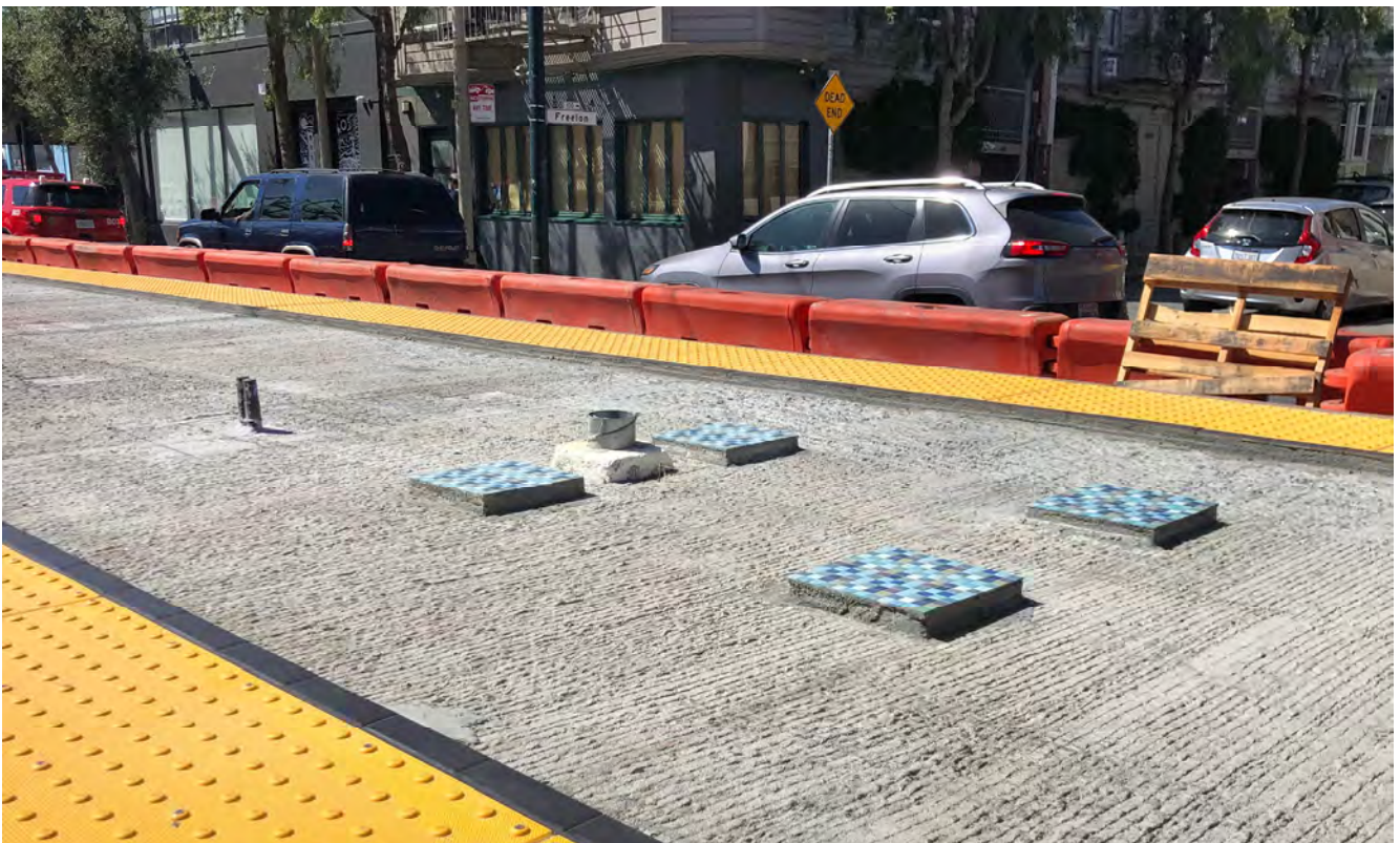
Colorful, decorative tile mosaics have been added to the face of the 4th and Brannan surface station, prior to pouring and smoothing the finished terrazzo platform surface around them.
