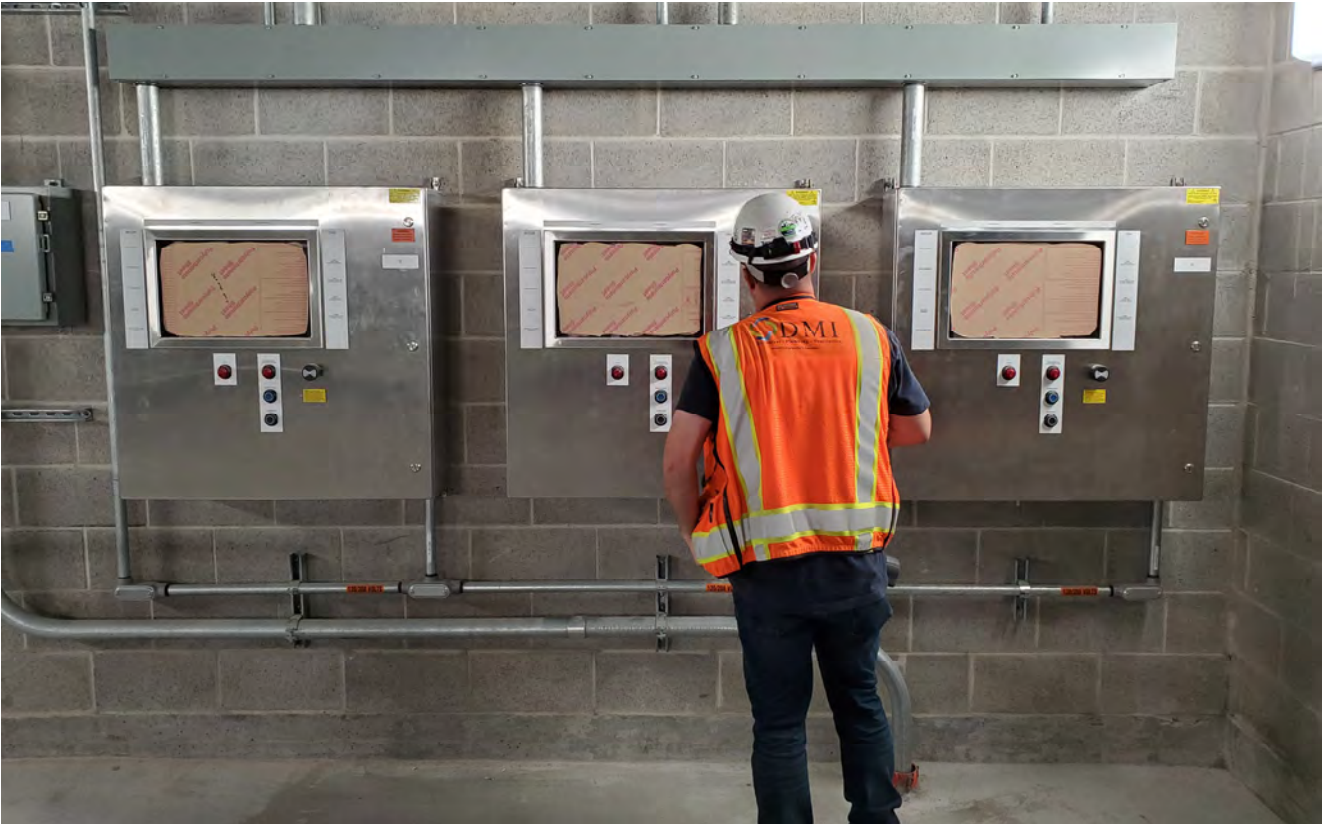
A technician inspects future fan control panels inside Yerba Buena/Moscone Station.
