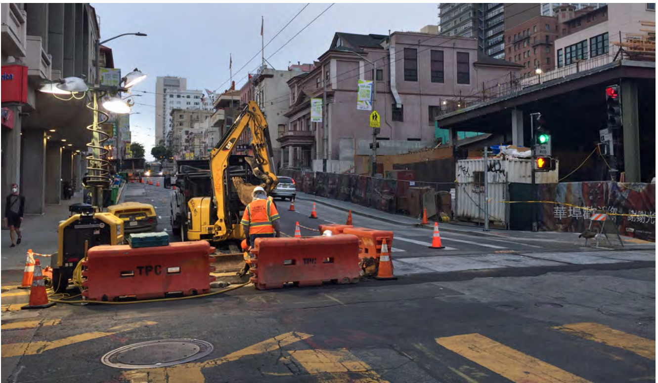
A crew sets up a light stand for night work to connect station utilities to city lines at the intersection of Stockton and Washington.
