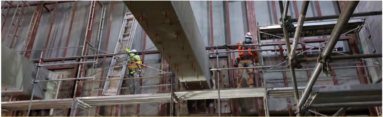
Steel framing has been furred out from the east wall of the concourse lobby for the installation of utilities behind and wall panels against it.
