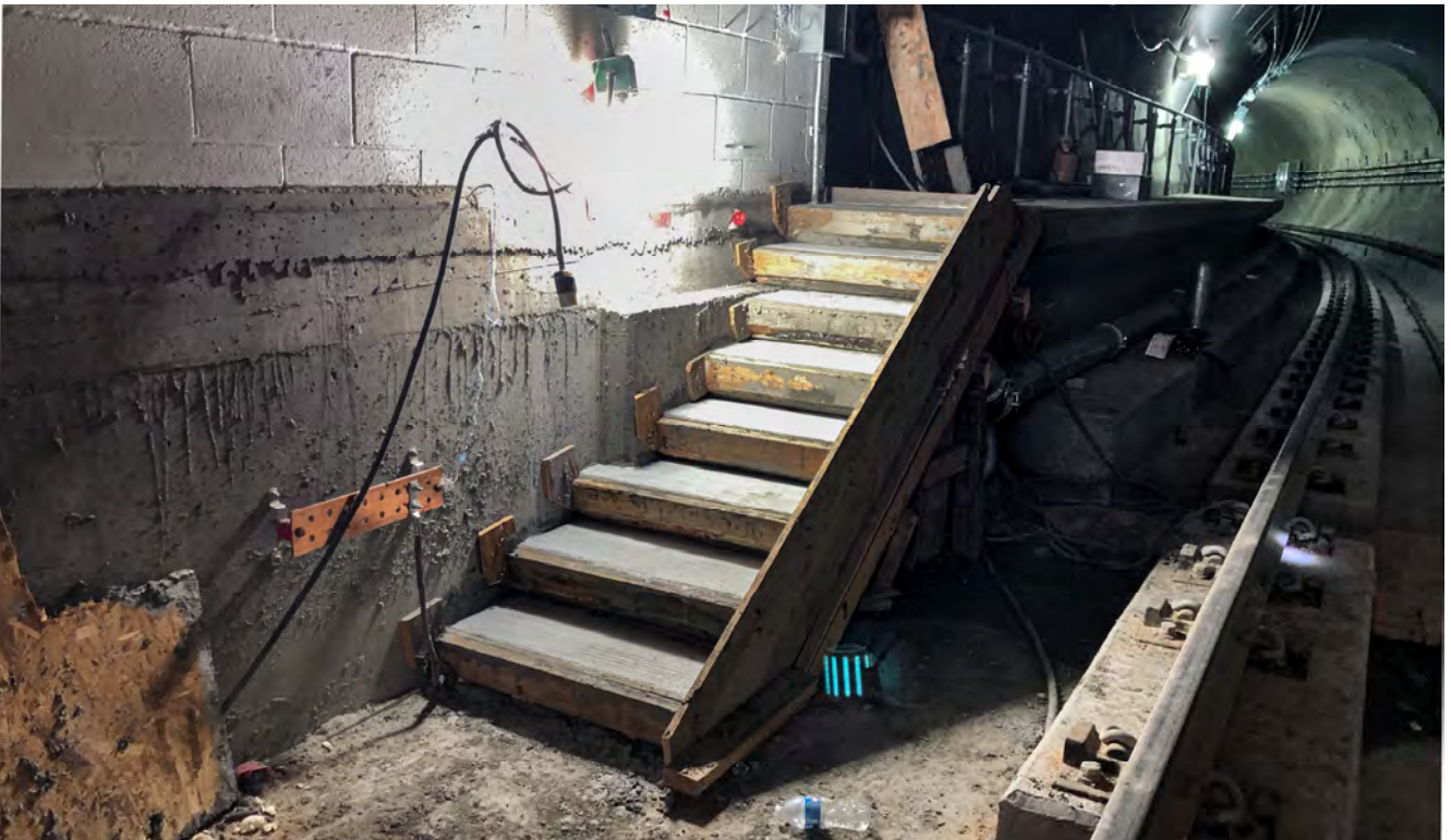
A new tunnel walkway staircase has been constructed where the of Union Square/Market Street Station platform transitions into the southbound tunnel.
