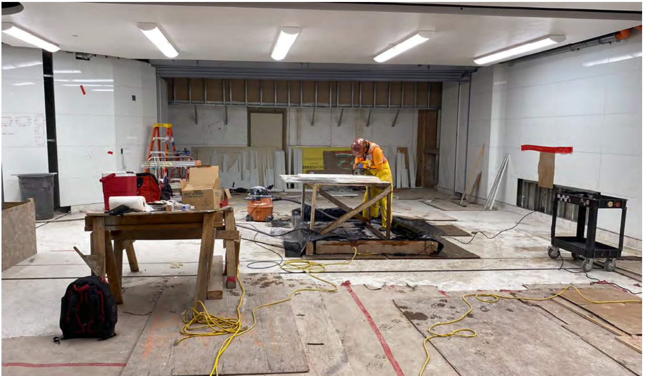
A worker shapes a piece of wall paneling near where the station concourse for Union Square/Market Street Station will open up into Powell Station under Market Street.
