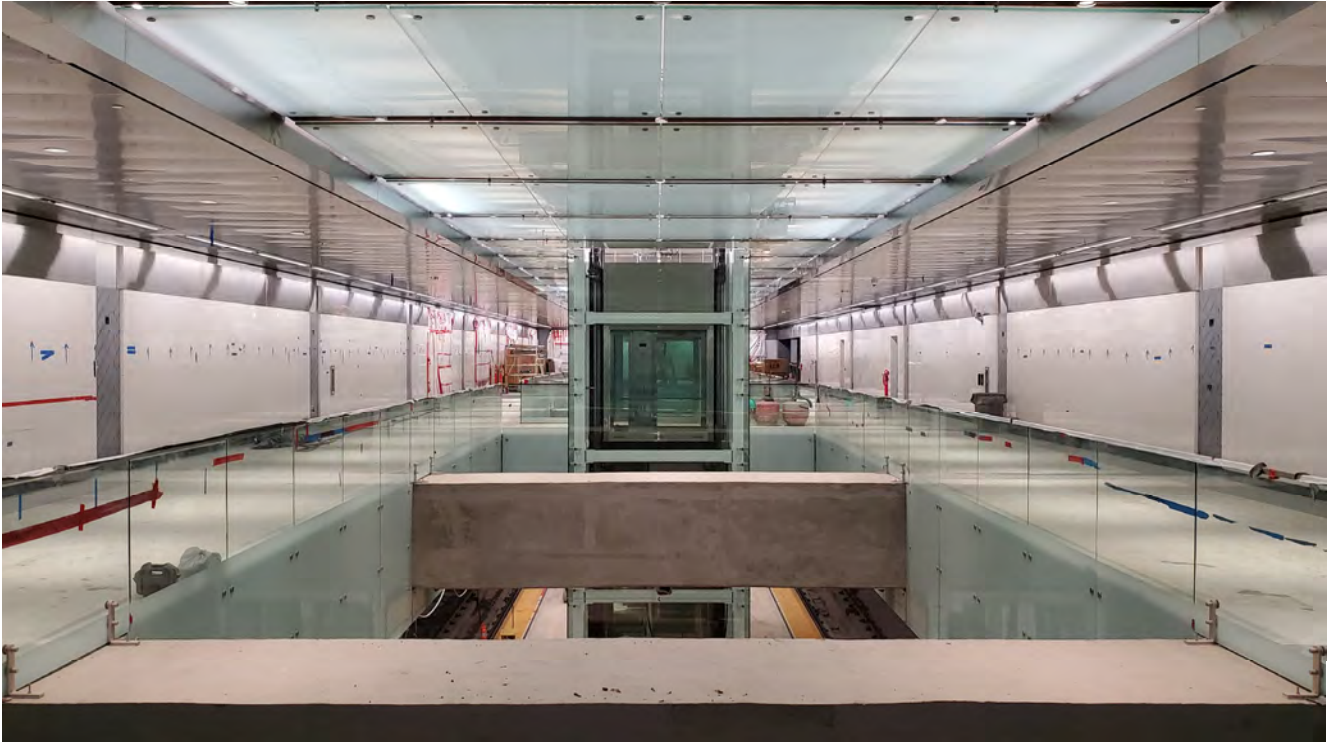
Gleaming, lit glass and stainless steel panels adorn the interior of the concourse level for Yerba Buena/Moscone Station.
