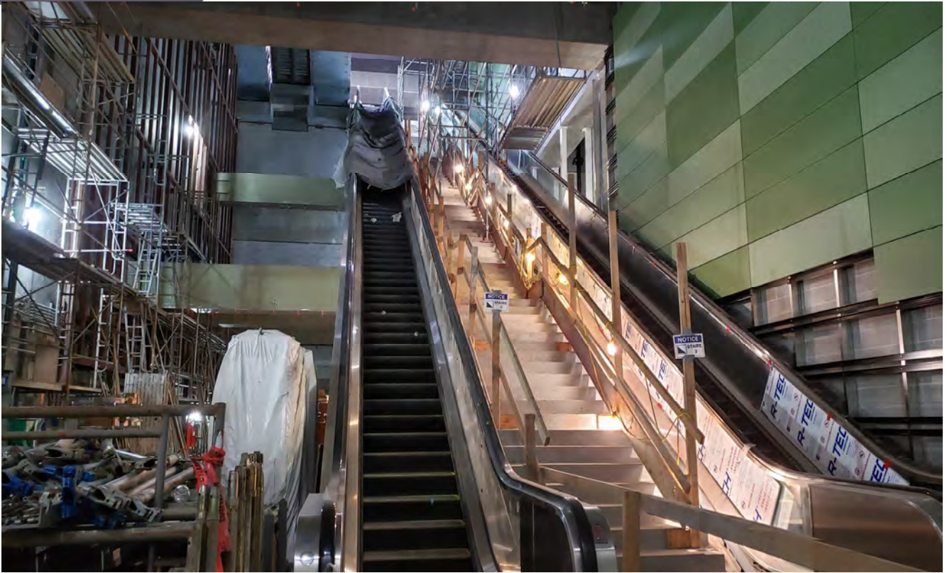
Varied jade-colored wall panels are being placed to create finished interior walls at the base of the dual escalators and entrance staircase for Rose Pak-Chinatown Station.
