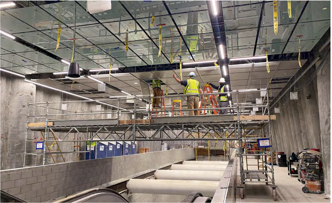
A long, rolling scaffolding assembly helps workers easily install utilities ceiling panels, and permanent lighting near the north end of the Union Square/Market Street Station concourse.
