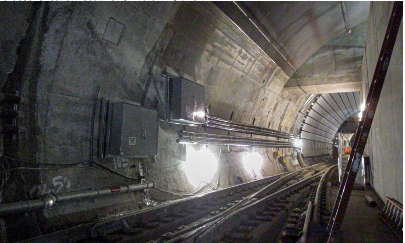
Electrical systems are being installed along the southbound track where it transitions from the Chinatown Station platform area to the track crossover cavern.
