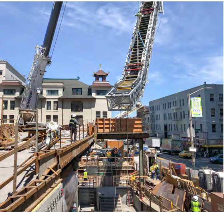
The right angle and approach are worked out, and the crew moves it into place very slowly and carefully.
