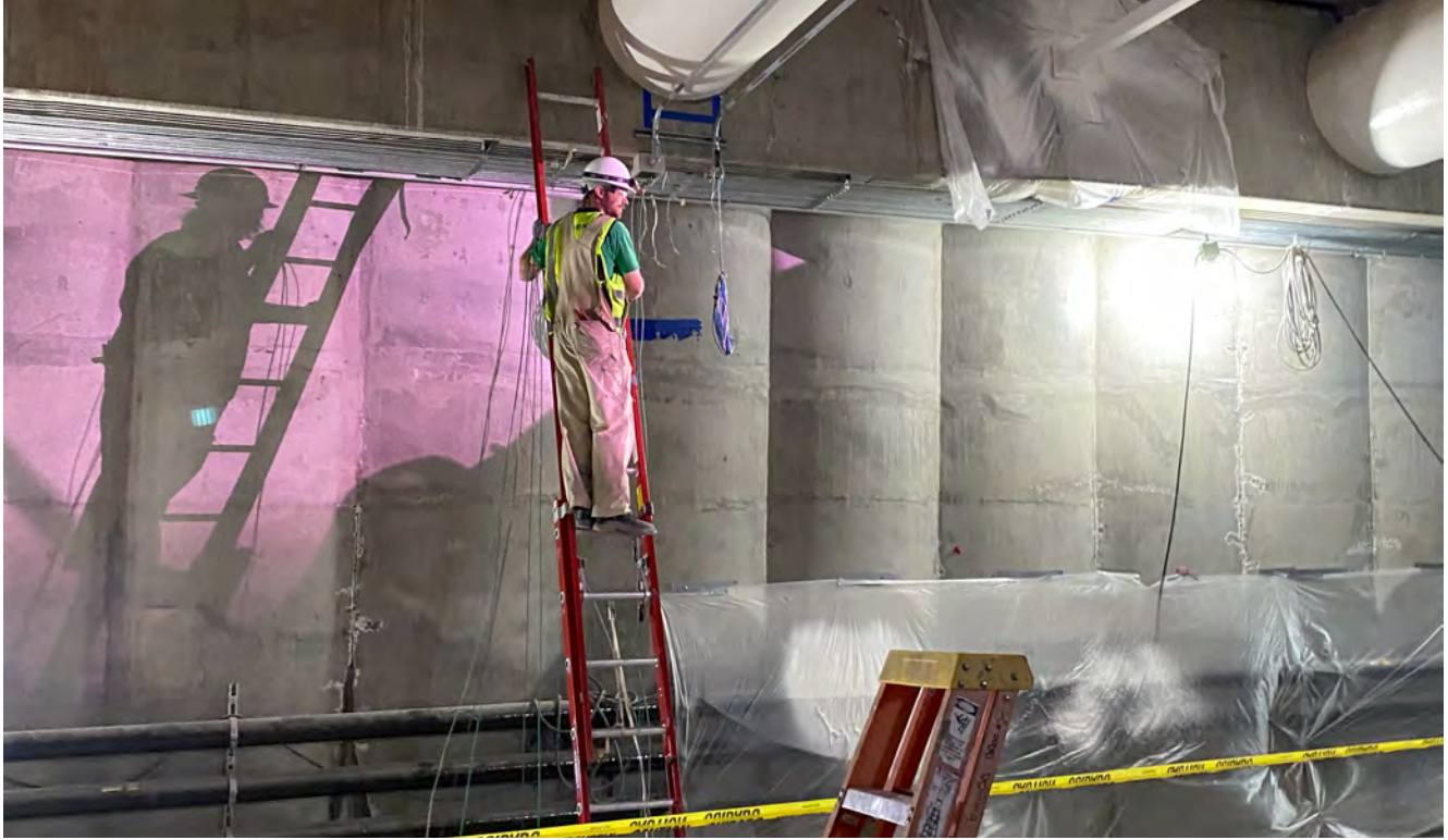
Arc welding highlights the shadow of a worker installing electrical systems for lighting and other interior elements adjacent to the Union Square/Market Street Station platform.
