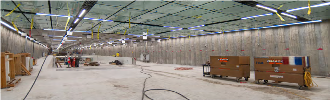
Lighting and glass ceiling panels have been installed inside the south concourse for Union Square/Market Street Station.
