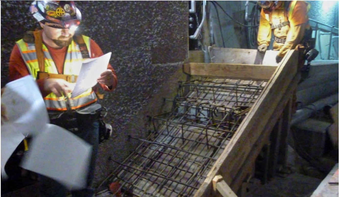
Workers review design details during construction of a staircase leading up to the north-bound tunnel walkway from Yerba Buena/Moscone Station.
