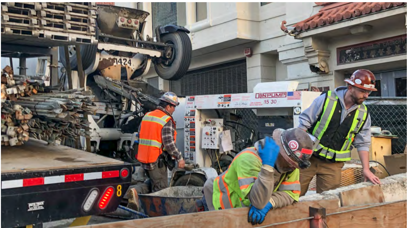
Scaffolding is bundled and loaded onto a flatbed following the completion of specific interior wall work, as two workers observe operations below from an access shaft on Washington Street.
