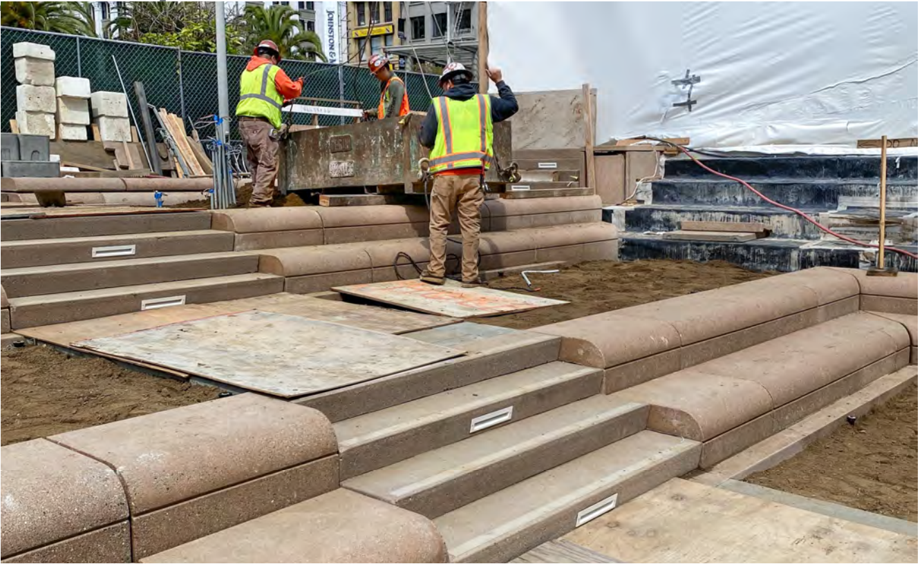
Next to the future north entrance for Union Square/Market Street Station, concrete stairs and terrace blocks have been placed, with soil now being added to the planters as part of work to restore this section of the square.
