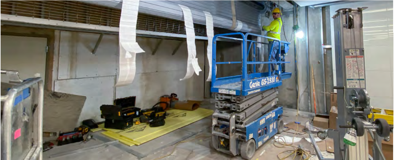
A roll-up steel gate is being installed and tested where the south concourse for Union Square/Market Street Station transitions into the concourse for Powell BART/Muni Station.
