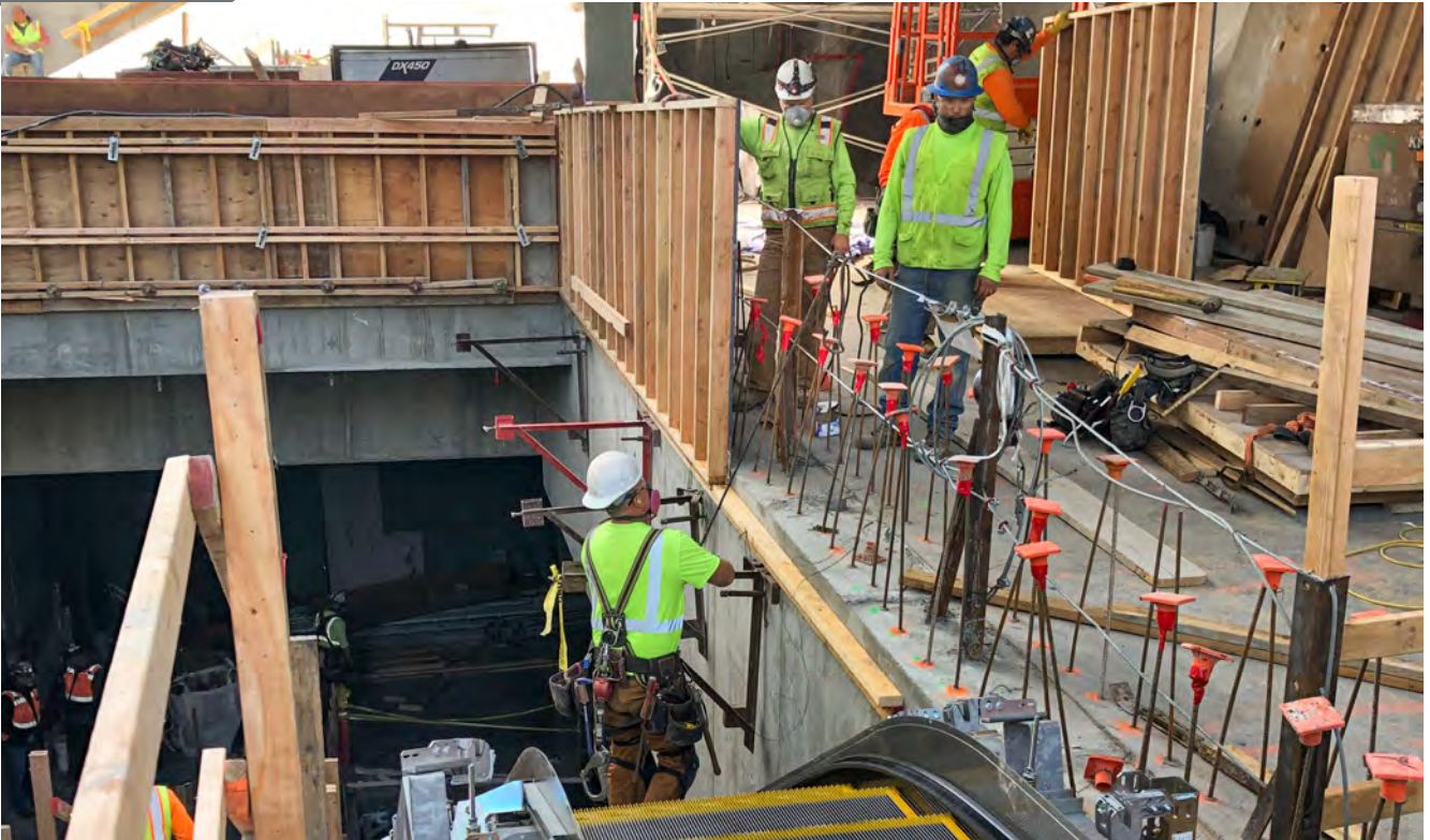
Now lowered into place, the first in a set of escalators leading to and from the street level entrance for Chinatown Station will be built out one piece at a time.
