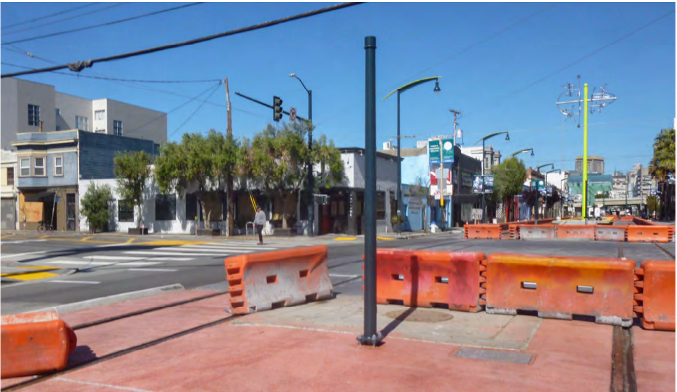
Poles for future signage and signaling equipment have been installed at a number of locations along the 4th Street surface alignment.
