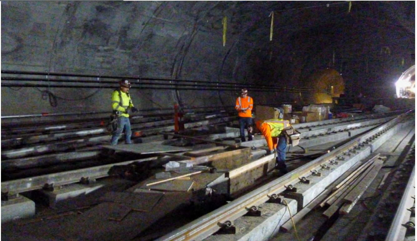
With recently-installed catenary system wires spanning overhead, a crew builds concrete forms for a raised walkway to ferry future heavy equipment across the tracks inside the crossover cavern south of Chinatown Station.
