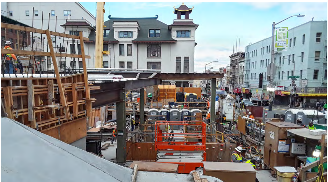
Steel framing for the Rose Pak-Chinatown Station's street level entrance structure and roof plaza is going up at Stockton and Washington.
