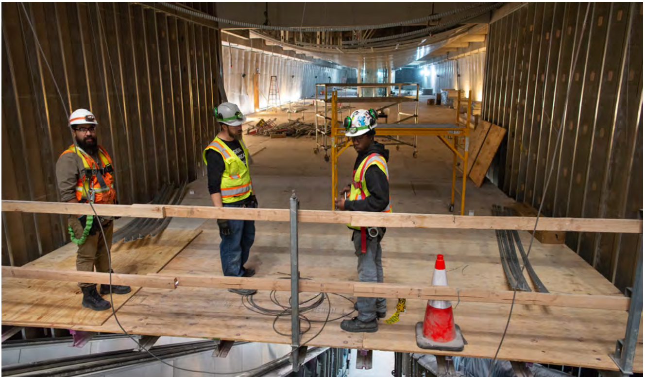
Workers discuss operations at the south end of Union Square/Market Street Station, where a temporary floor is in place to support work for a curved, ceiling-mounted interior design element.
