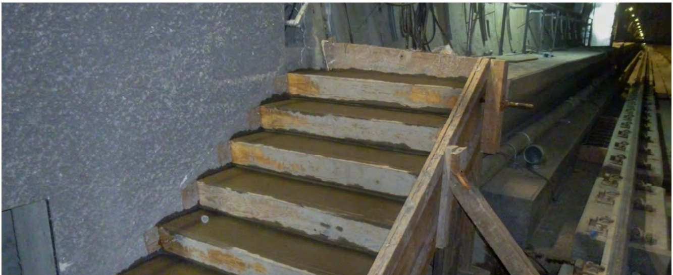
Reinforced concrete stairs leading up to the tunnel walkway have been poured at the north end of Yerba Buena/Moscone Station.
