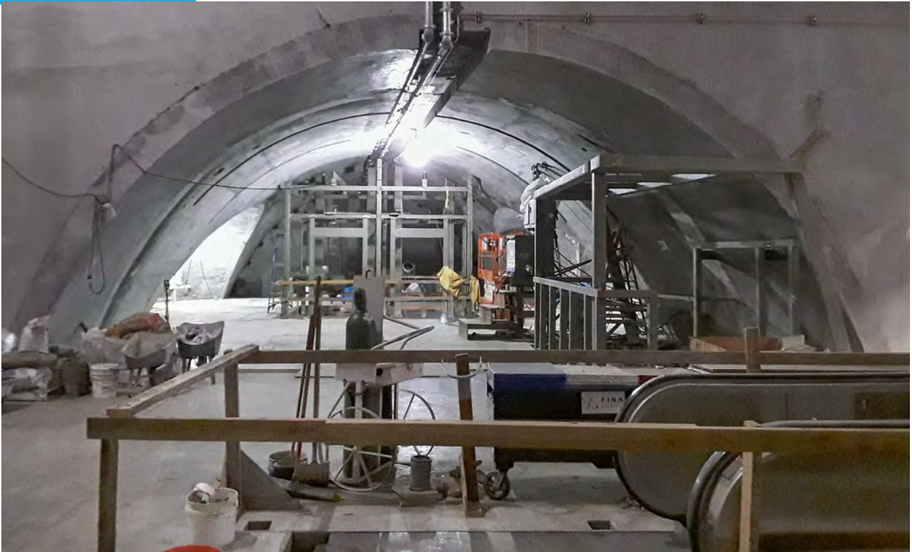
Steel framing for the future station agent booth and elevators is going in, inside the cross-cut cavern archway for Rose Pak-Chinatown Station.
