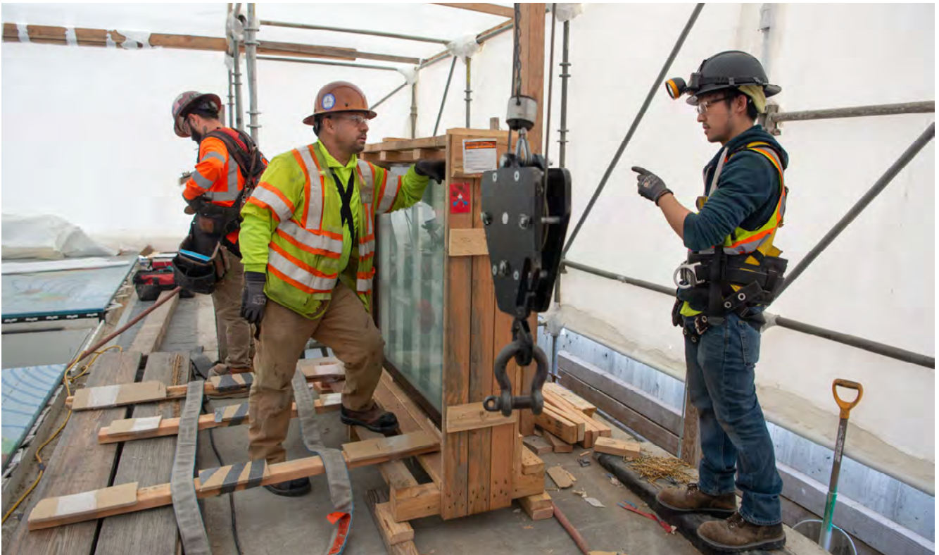
Two workers prepare to carefully lower and place another section of decorative glass roof deck atop the north entrance structure for Union Square/Market Street Station.
