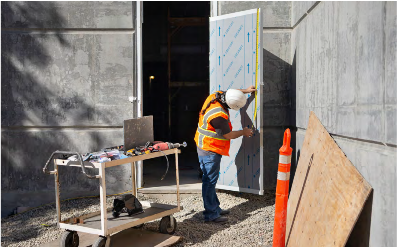
A worker checks measurements on a steel door, recently installed as part of the ventilation and utilities area for Yerba Buena/Moscone Station's surface level entrance structure.
