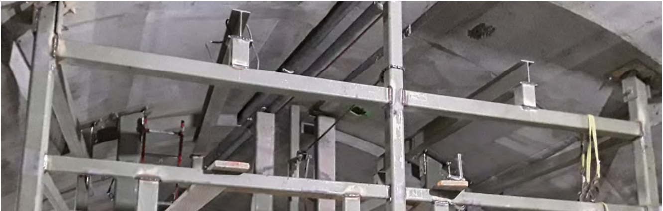
Steel framing for future concourse-to-platform level elevators is being constructed inside the cross-cut cavern leading into the Rose Pak-Chinatown Station platform cavern.
