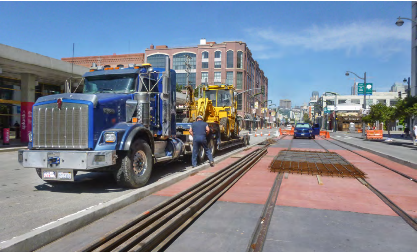
Steel reinforcing and rails wait inside the work area between Townsend and King Streets on 4th, as preparation for rail installation at the 4th and King intersection ramps up.
