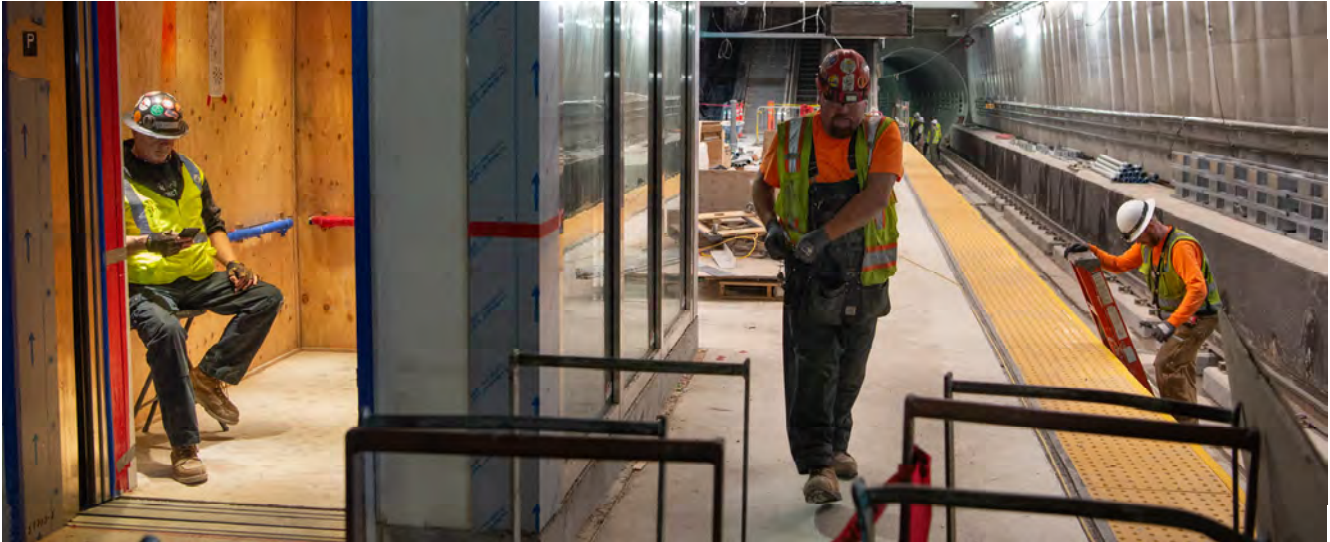
A crew collects at an elevator being tested, at the start of the mid-shift lunch break along the south-bound track side of Union Square/Market Street Station.
