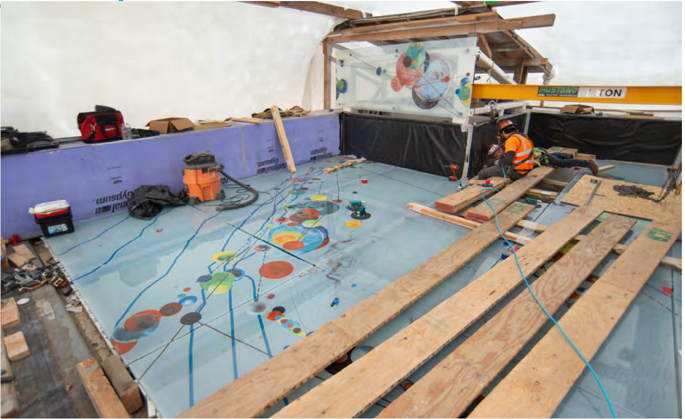
Sections of decorative glass roof deck are being installed atop the north entrance for Union Square/Market Street Station. These panels are designed by artists Amanda Huguen and Jennifer Starkweather.
