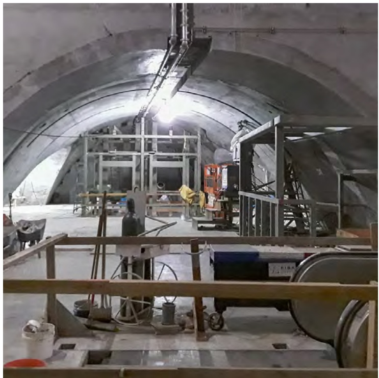
Next up will be the two sets of elevators, both from the surface to the concourse lobby, and from the concourse to platform level.
