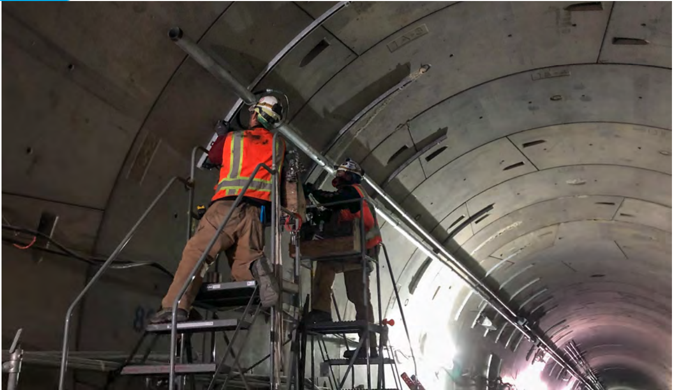
Steel mounting brackets, conduits, and pipes are being installed inside the twin subway tunnels for lighting, signaling, and other utility systems.
