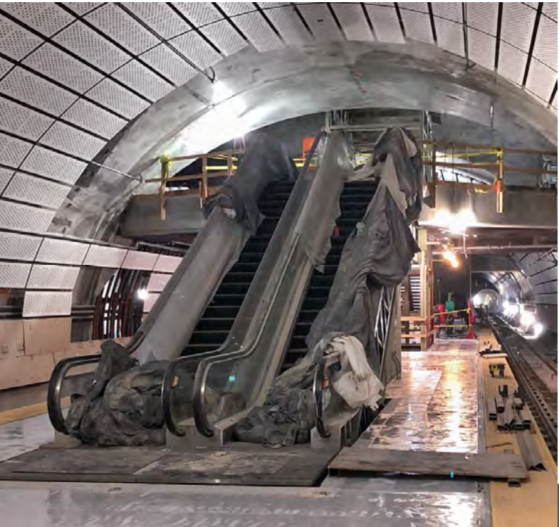
All three sets of escalators from the surface down to the station platform are now being fitted out.
