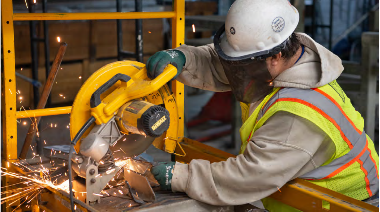
Small sections of steel beams are custom-cut and fit to assemble framing for the future fare gate area of Yerba Buena/Moscone Station.
