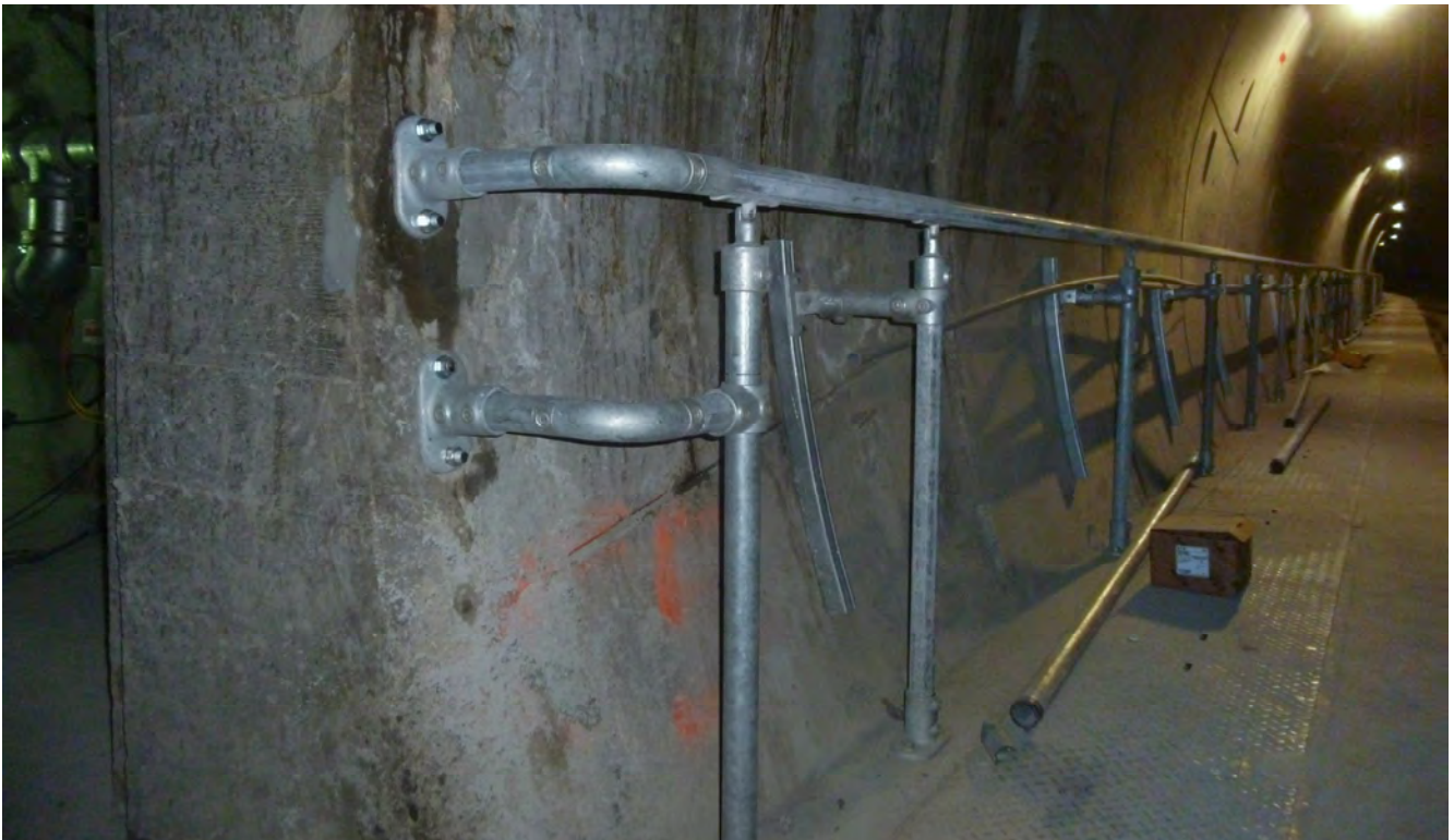
Railings have been added to the pedestrian walkway inside the northbound tunnel seen here near cross-passage 5.
