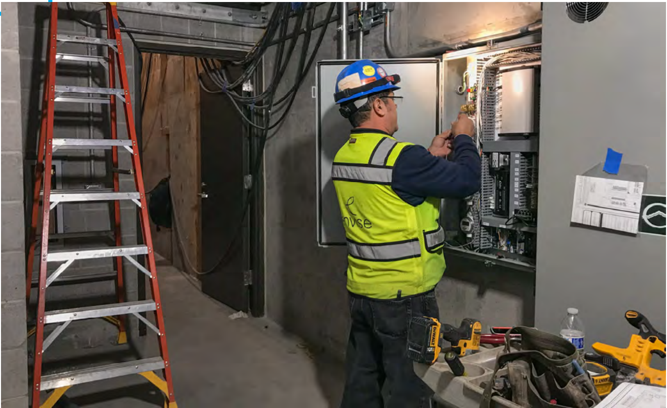
A technician installs communications equipment inside the mezzanine level of the Yerba Buena/Moscone Station headhouse.
