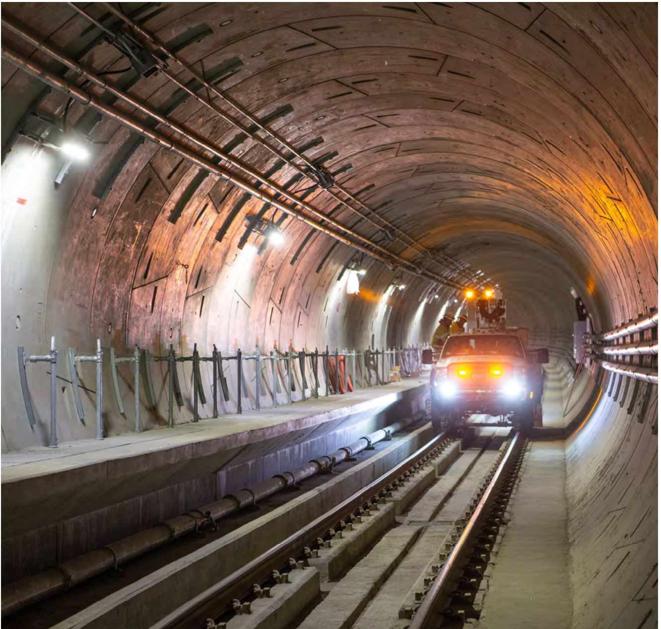
A work crew carefully makes their way south inside the northbound tunnel, following testing work near the S-curve under the Market Street Subway.
