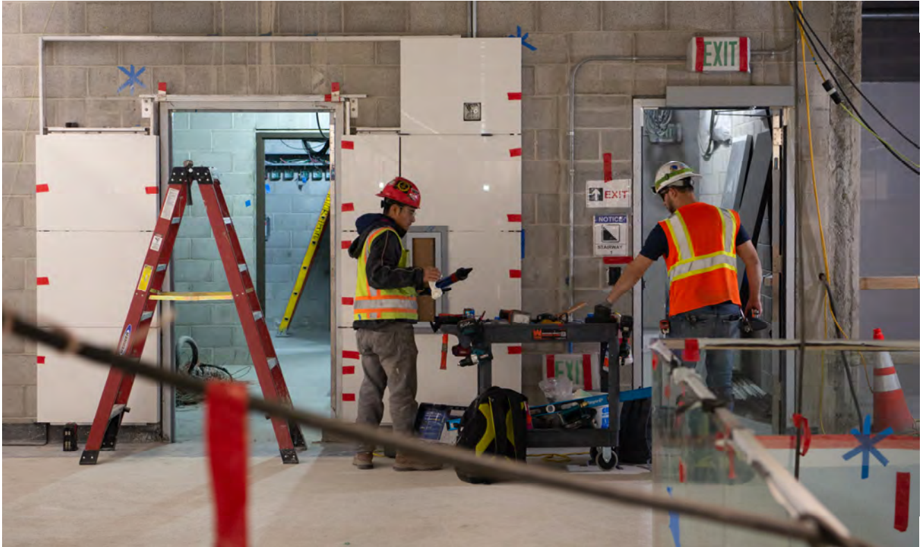
Workers at the south end of the concourse level for Yerba Buena/Moscone Station carefully install glossy wall panels around a doorway.
