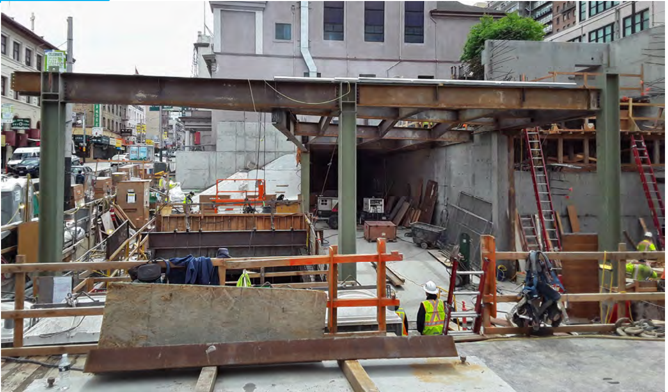
Looking into the future street-level entrance area for Rose Pak-Chinatown Station, where escalators will take passengers to and from the station cavern below.
