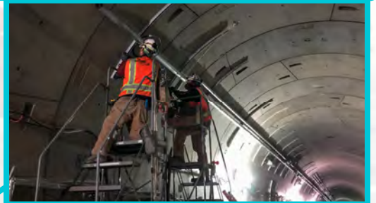
4th St. Surface Track, Systems (STS)
