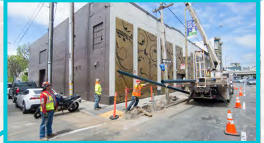
4th St. Surface Track, Systems (STS)
