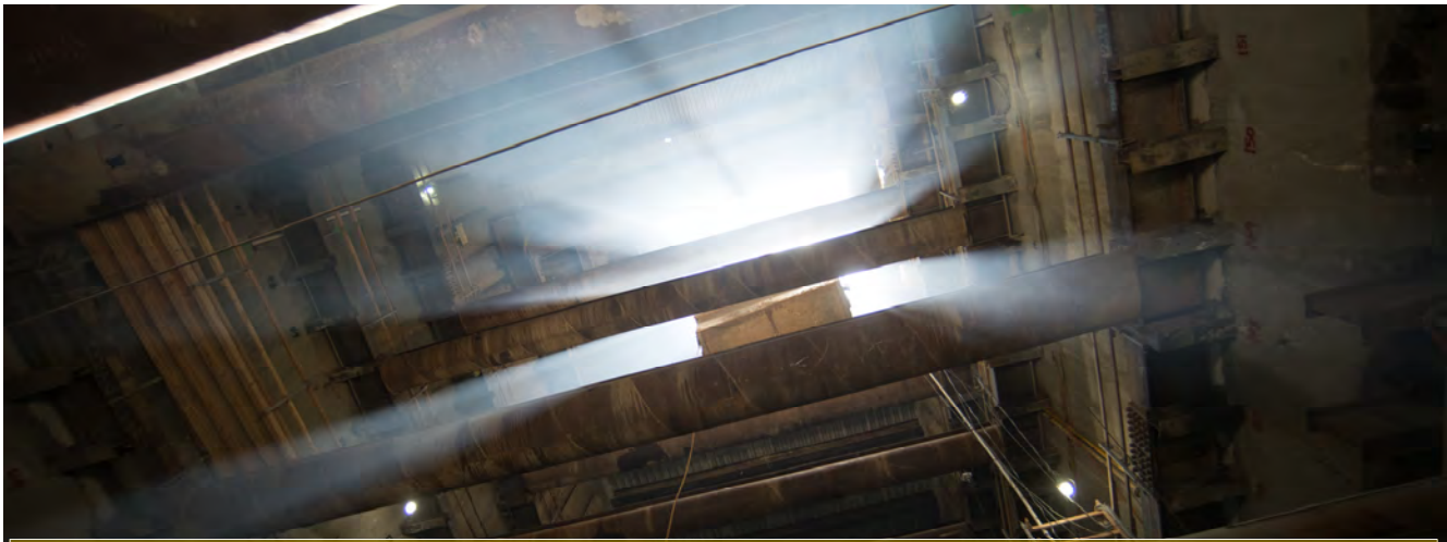
Light streams in an access shaft at UMS as a large steel bucket used to haul out excavated material is lowered carefully between temporary steel struts.
