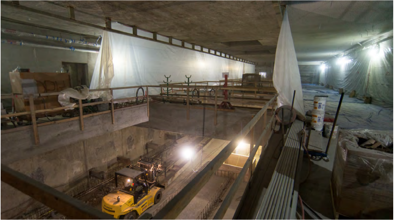
Plastic sheeting masks off areas where soundproofing material is being sprayed to walls and ceilings inside the station box.
