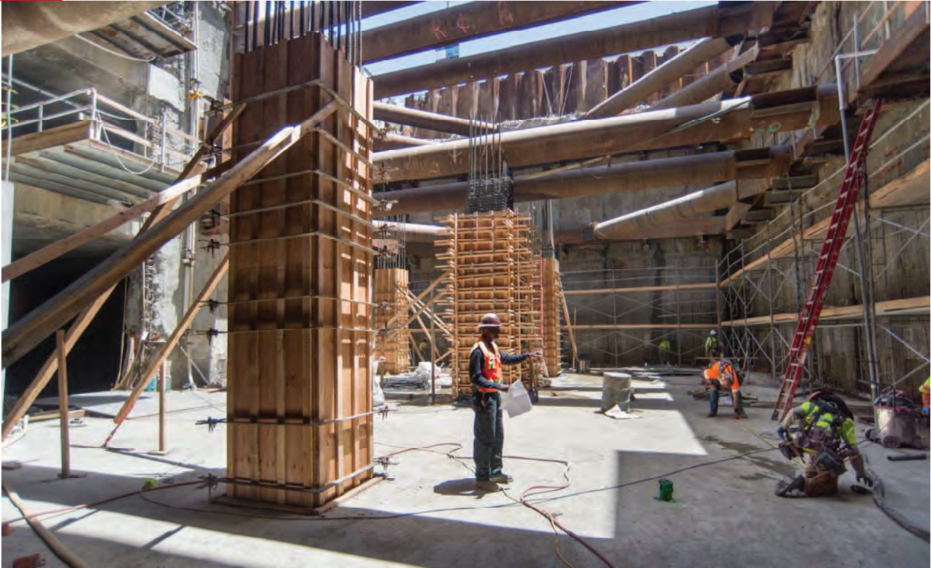
Large concrete forms are carefully leveled and reinforced as part of vertical column construction inside the station headhouse.
