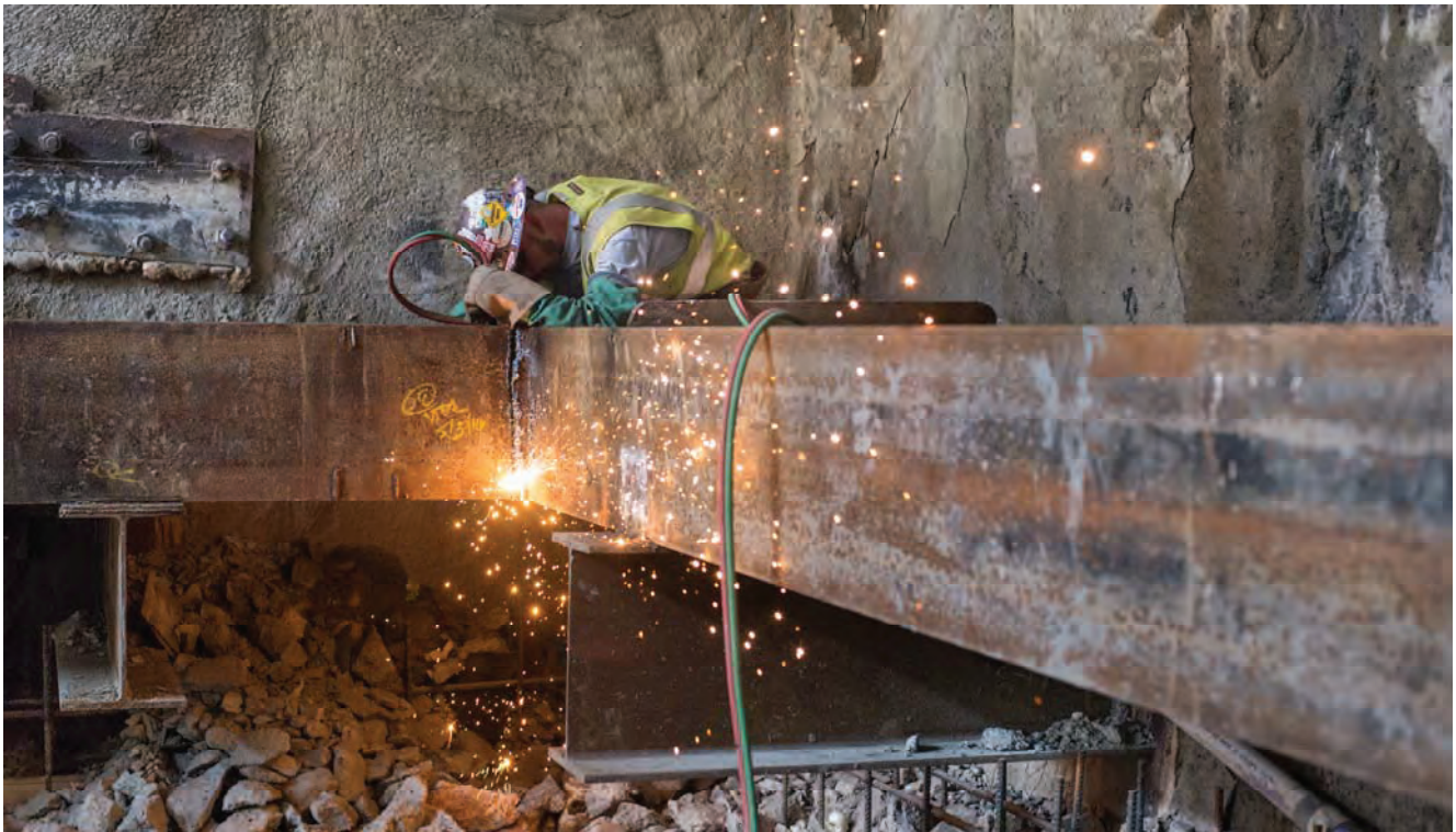
Sparks fly as a worker uses a cutting torch to separate massive steel I-beams which were used as part of temporary reinforcing inside the headhouse.
