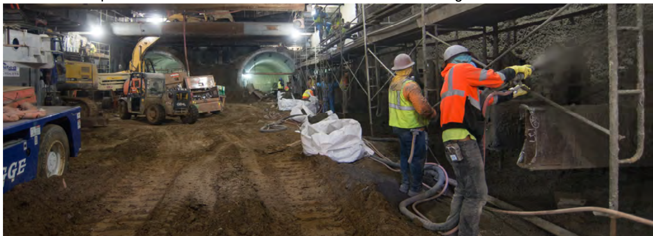
Workers spray shotcrete on steel mesh on the west wall of the Union Square/Market Street Station.
