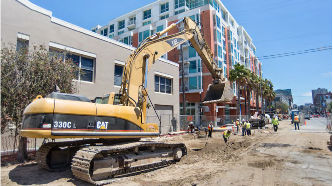
A large excavator stands north of Welsh on 4th, helping to grade the road bed ahead of street restoration work.
