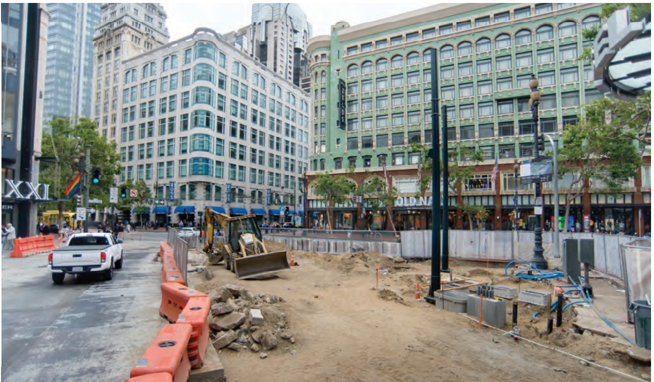
Utility boxes and OCS poles have been installed at the southwest corner of Stockton and Ellis, where street restoration work is underway.
