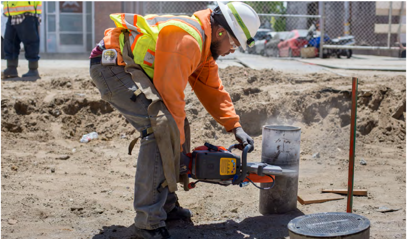
A worker cuts a section of vertical pipe to length, to match it with the level of the future paved roadway.
