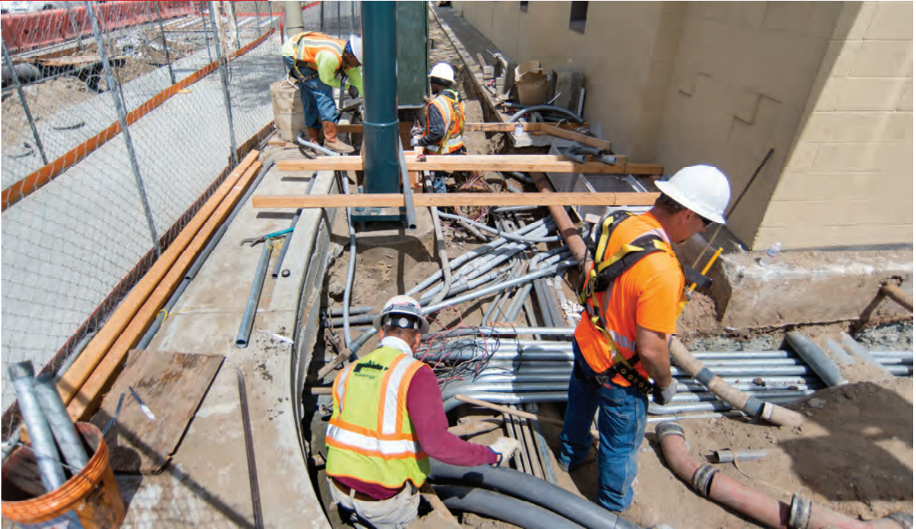
Seemingly endless rows of conduits and other utility works cross atop each other in the sidewalk area on the east side of 4th north of Brannan.
