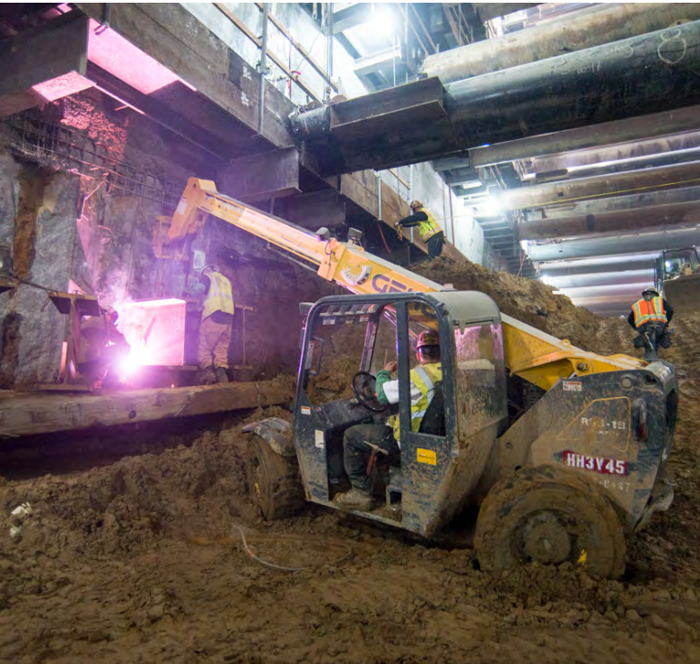
2 Temporary reinforcing is installed, as well as brackets for the invert slab rebar
