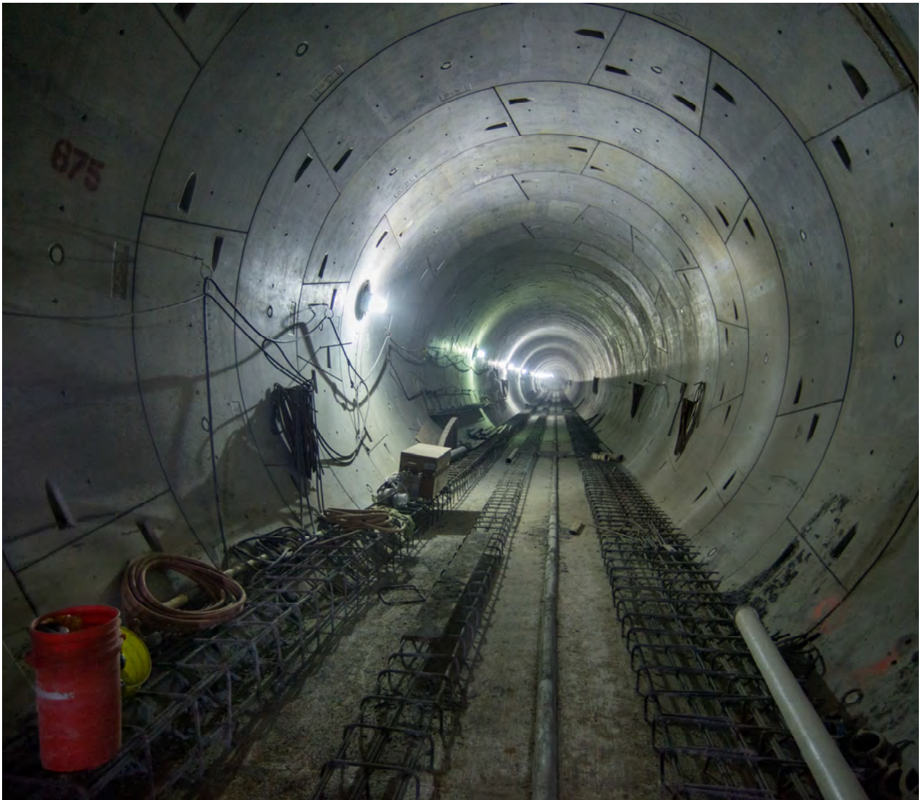
The northbound tunnel spans off into the distance, as seen from where it leaves the north end of the Union Square/Market Street Station.
