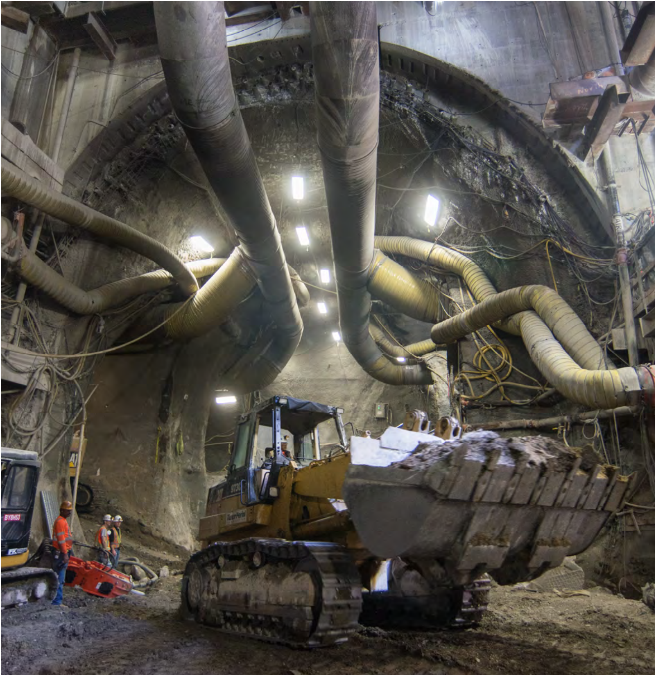
A bulldozer operator emerges from the arched cross-cut cavern, which will later become the entrance to the Chinatown station cavern from the station headhouse.
