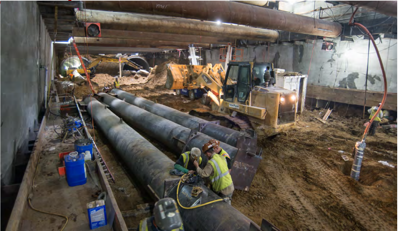
Large steel tubes called struts wait to be installed along the east wall of the station box, while removal of tunnel lining segments and excavation work continues just to the south.
