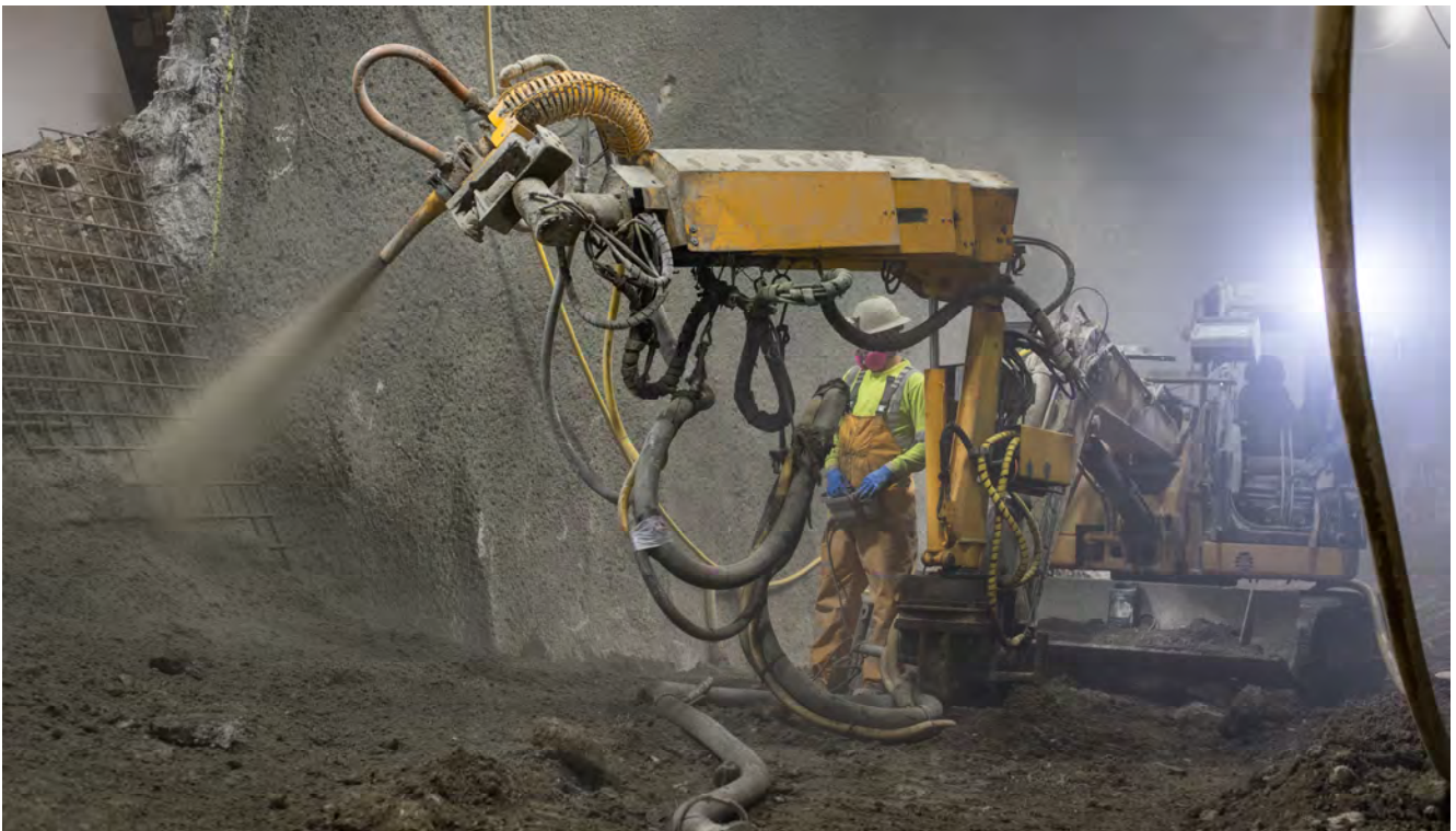
A shotcrete sprayer operator reinforces a small section of wall at the entrance to the right side drift of the south platform cavern.
