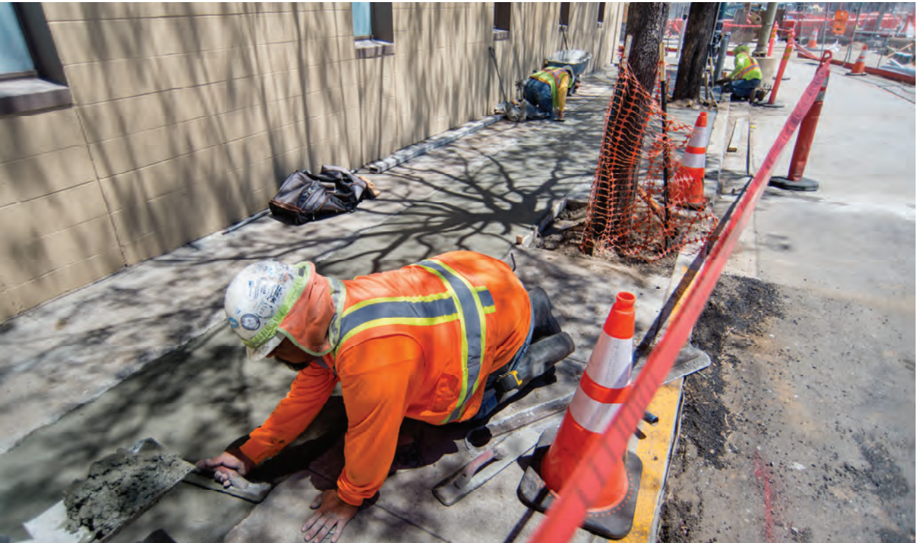
A crew smooths fresh concrete, poured on top of recently-upgraded and relocated utilities under the sidewalk north of Brannan.
