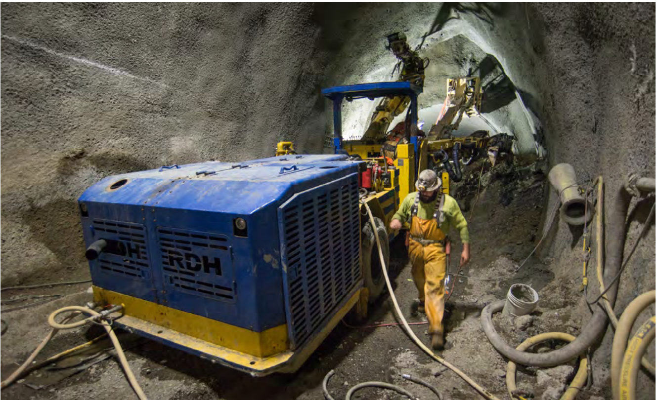
A crew conducts maintenance on a drill rig used to reinforce the ceiling arch of the platform cavern.
