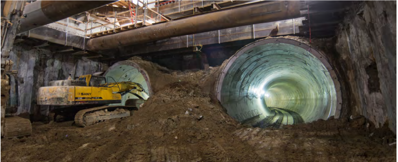
As will future trains leaving Union Square/Market Street Station, the southbound tunnel curves under market Street where it intersects with Stockton and Ellis, to move down 4th to Yerba Buena/Moscone.
