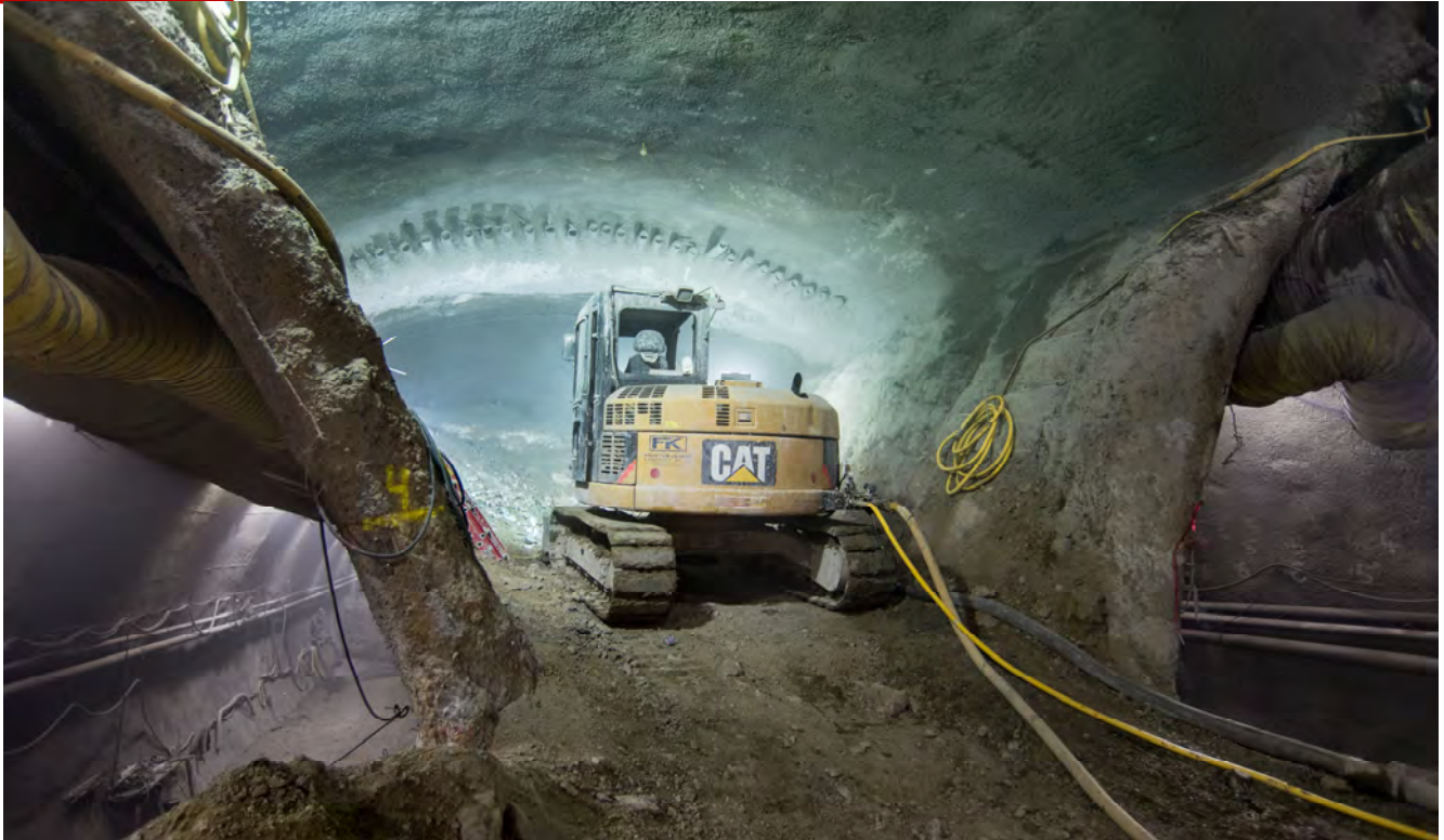
An excavator fitted with shotcrete spraying machinery sits inside the top header of the south platform cavern, which is currently being excavated.
