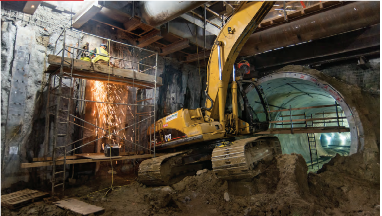
A worker cleans up the steel surface of a vertical reinforcing beam at the southeast corner of the station box, where the northbound tunnel opens into the future platform area.
