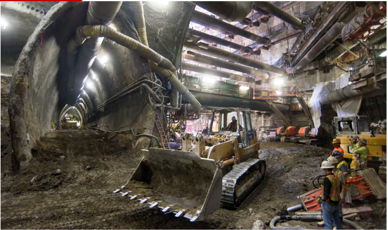
Bulldozers remove excavated material from inside the south platform cavern, and ferry it to collection areas inside the headhouse where it is sorted before removal to the surface.
