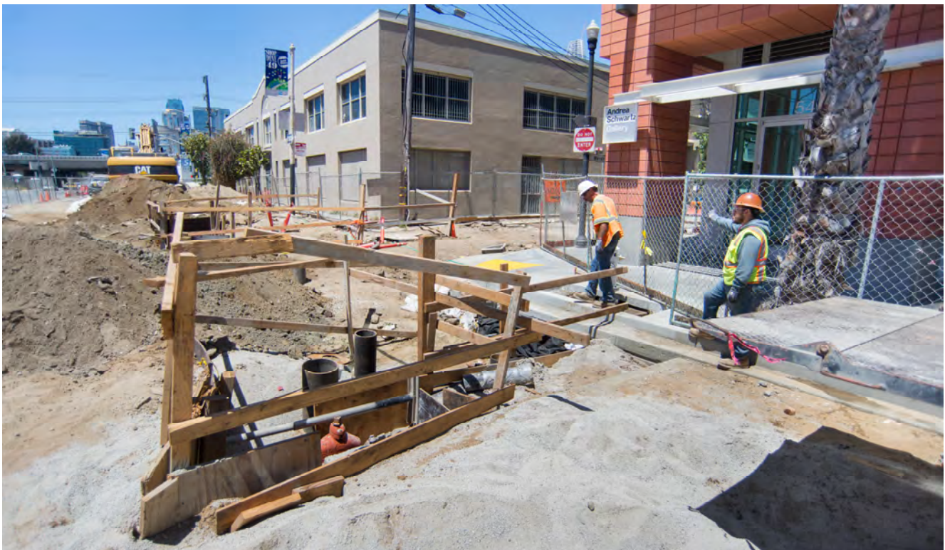
Upgraded high-pressure water pipes and valves wait for inspection at 4th and Welsh.
