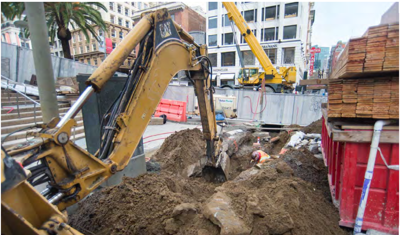
A utility trench is being dug on the north side of stockton, inside the north station entrance's worksite.
