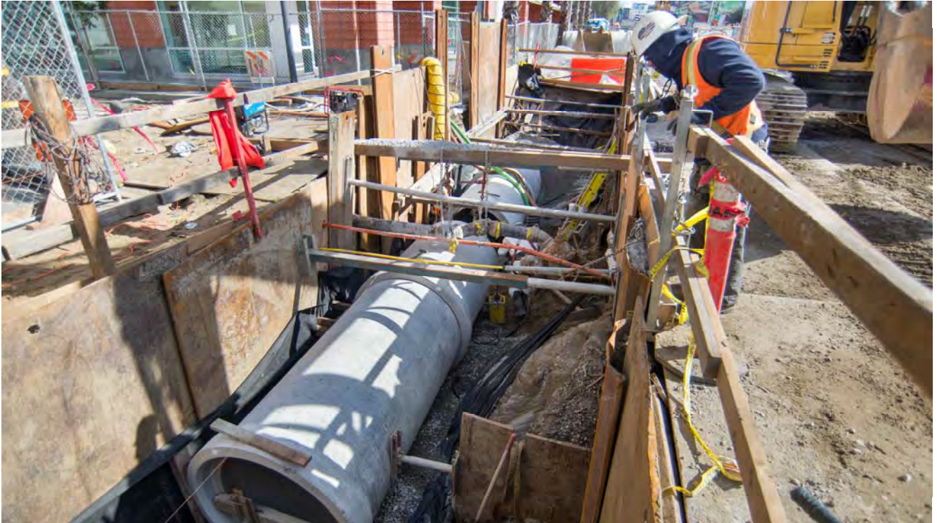
New sections of concrete sewer pipe and other utilities are being installed at the intersection of 4th and Welsh.
