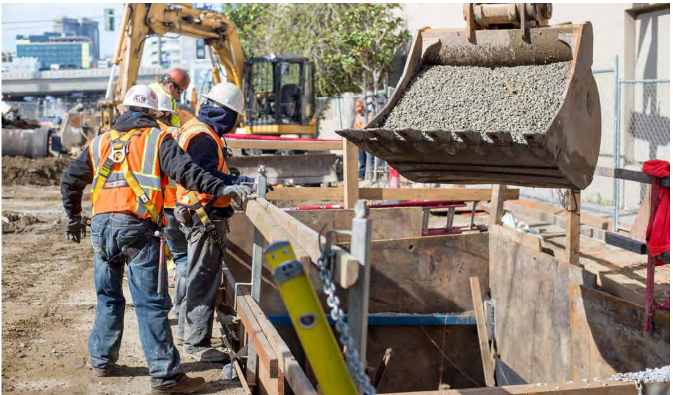
The bucket of an excavator is carefully positioned to dump gravel into part of a utility trench at 4th and Welsh as part of backfilling operations.
