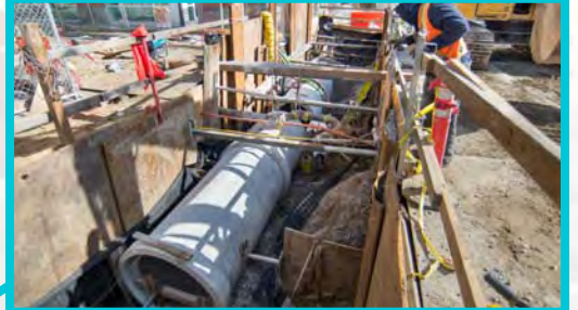
4th St. Surface Track, Systems (STS)
