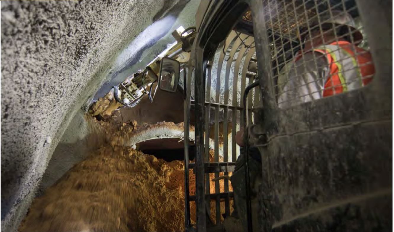
A wheel grinds away at soil inside the left side drift of the north platform cavern.
