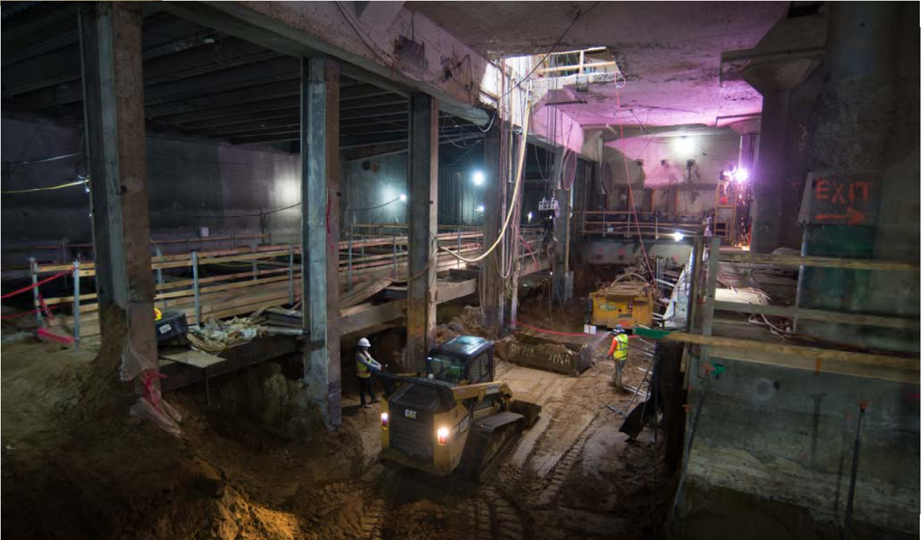
Work to remove excavated material inside the north concourse is done using a bobcat and steel bucket lifted through the access portal to Stockton.
