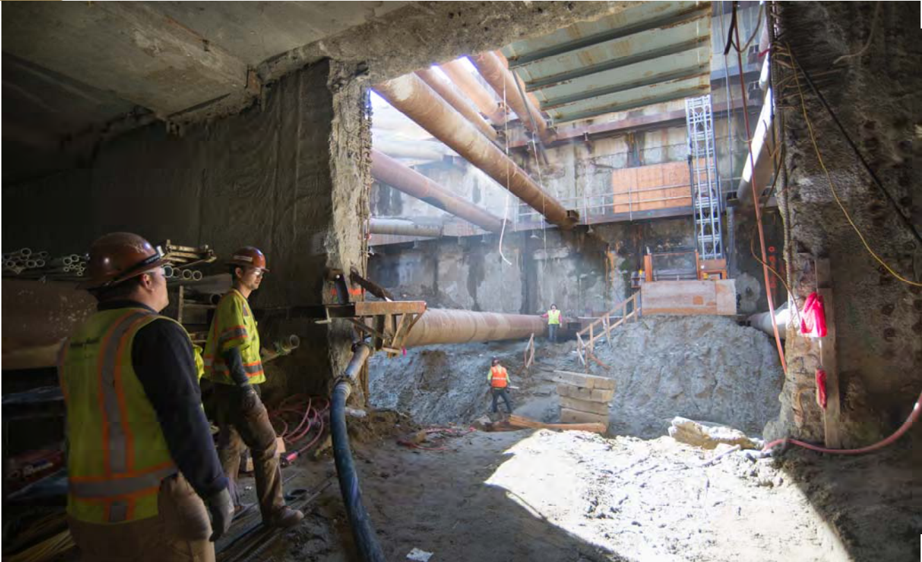
Workers prepare to bring materials in the station box from the headhouse portal opening following a crane lift.
