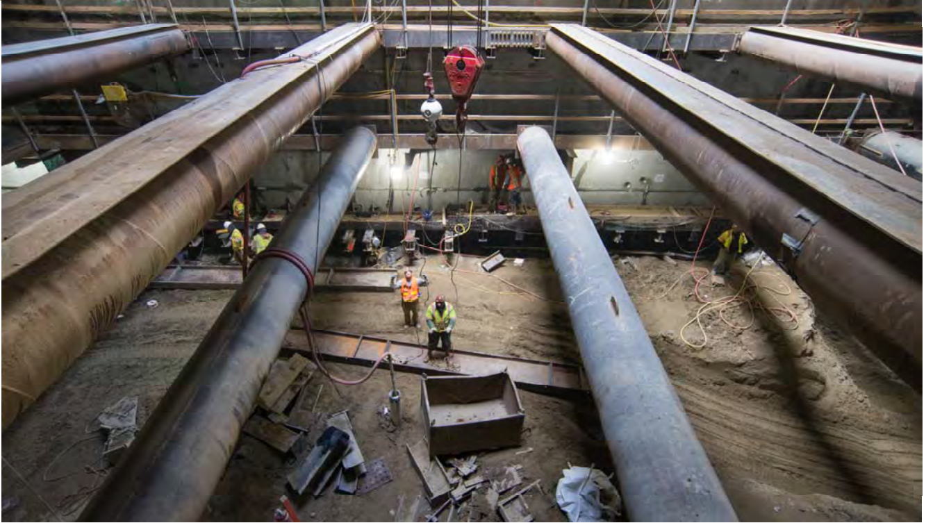
Workers detach a large steel beam used in temporary reinforcing from a crane hook, lowered in through the access shaft just north of O'Farrell.
