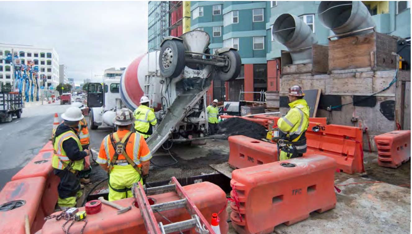
Concrete is poured into a utility trench mid-block between Howard and Folsom, on the west side of 4th, adjacent to the temporary station box ventilation structure.
