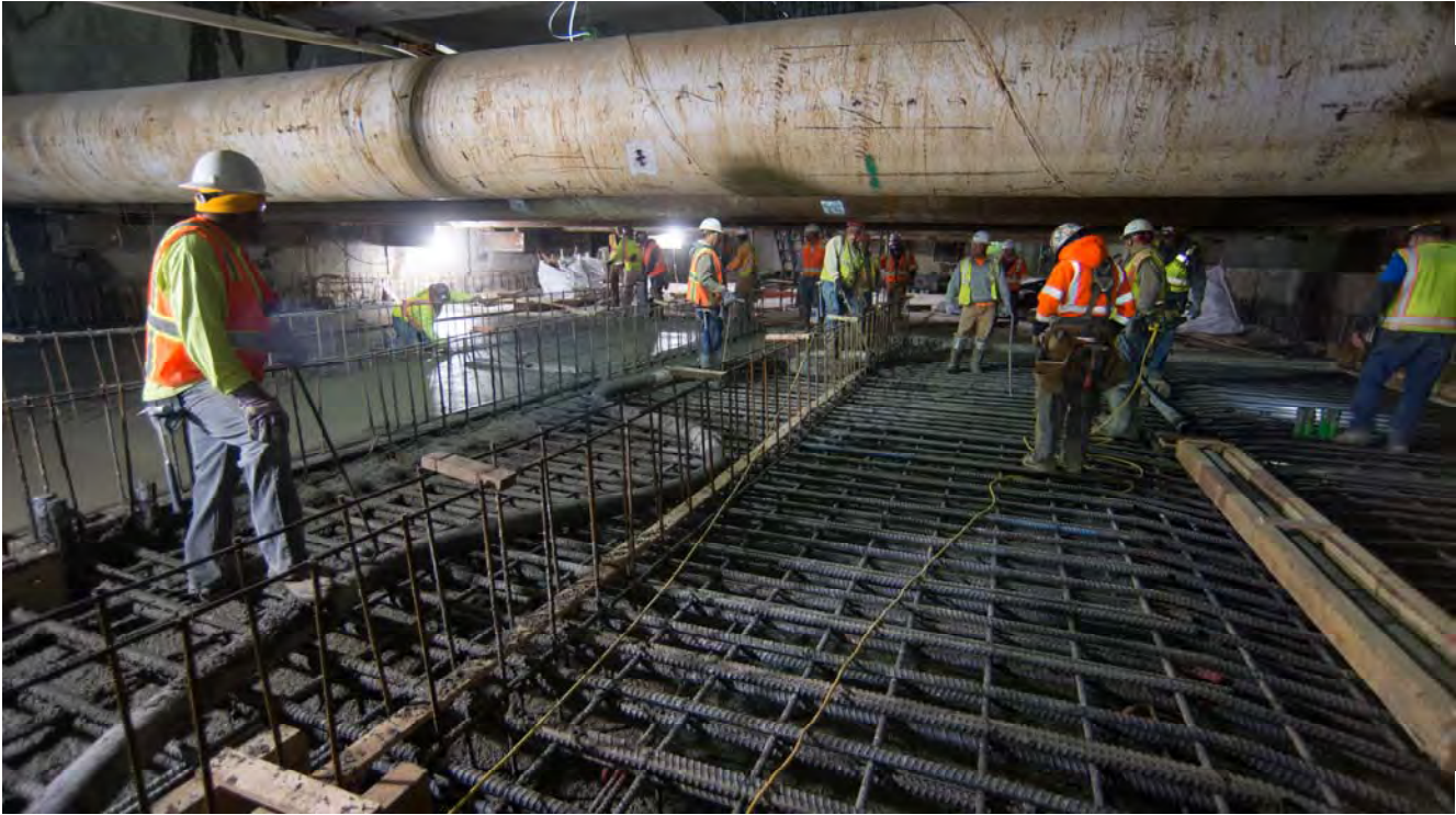
A hose is extended from a concrete pump on the surface, so workers can bring wet concrete where it's needed during a pour of another section of the invert slab.
