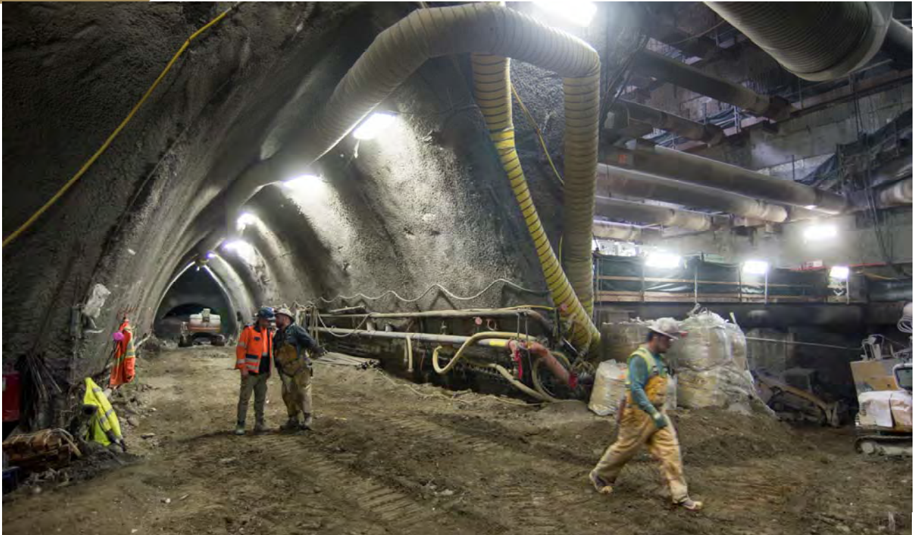
The entrance to the right side drift excavation of the south platform cavern, adjacent to the entrance archway to and from the station headhouse.
