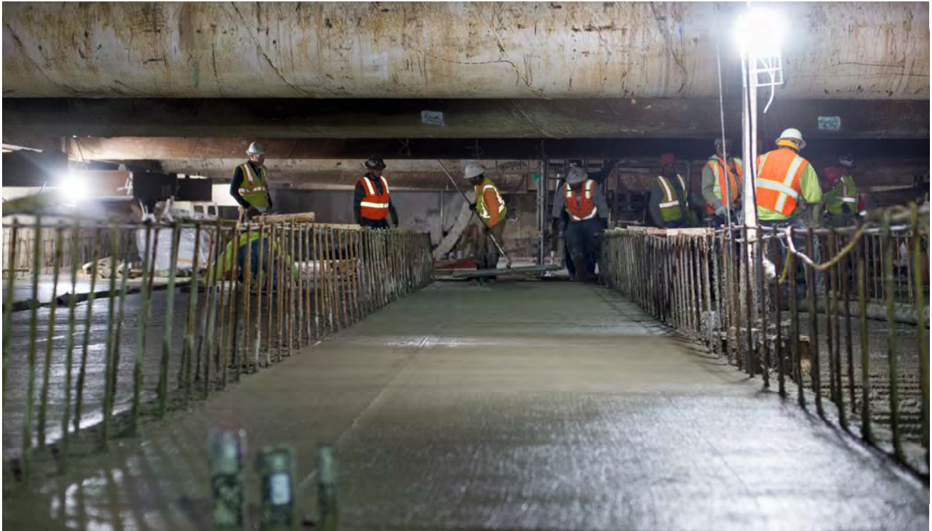
Workers smooth fresh concrete in the section section of the invert slab to be poured inside the station box.
