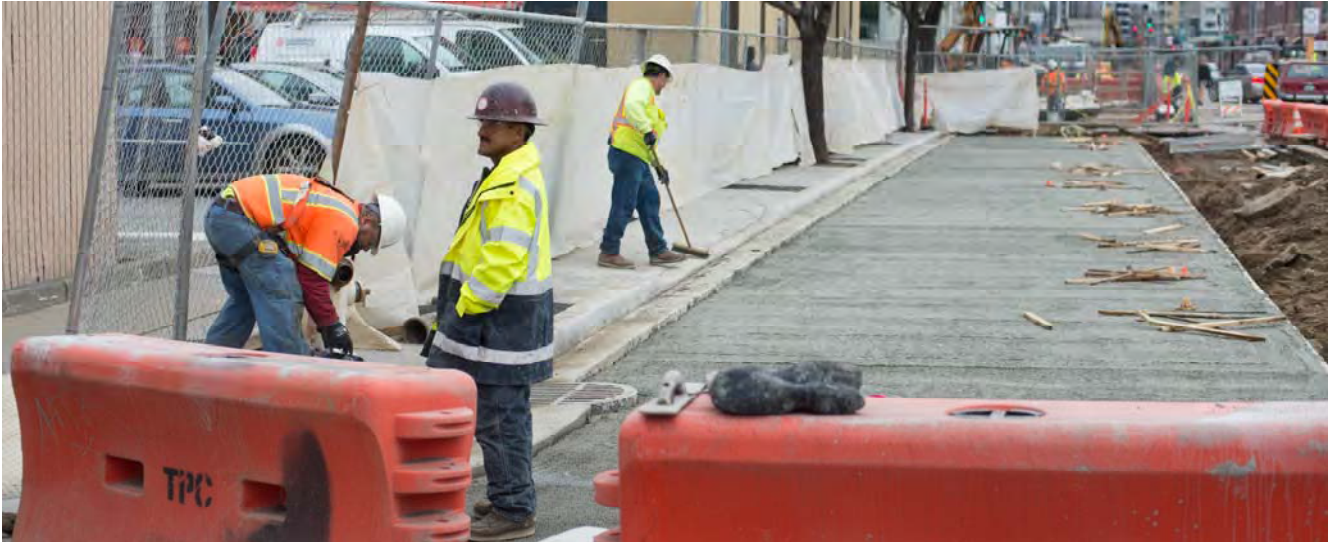
The easternmost section of the road slab has been constructed on 4th between Freelon and Brannan. Here, workers clean up the work site after removing pieces of concrete forms.
