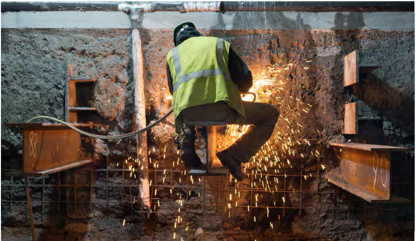
A welder sitting atop a steel I-beam bracket cuts vertical brackets to precise measurements before walers are installed.
