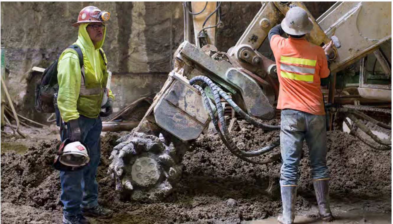
One worker pauses as another checks connections on the arm of an excavator inside the station headhouse.
