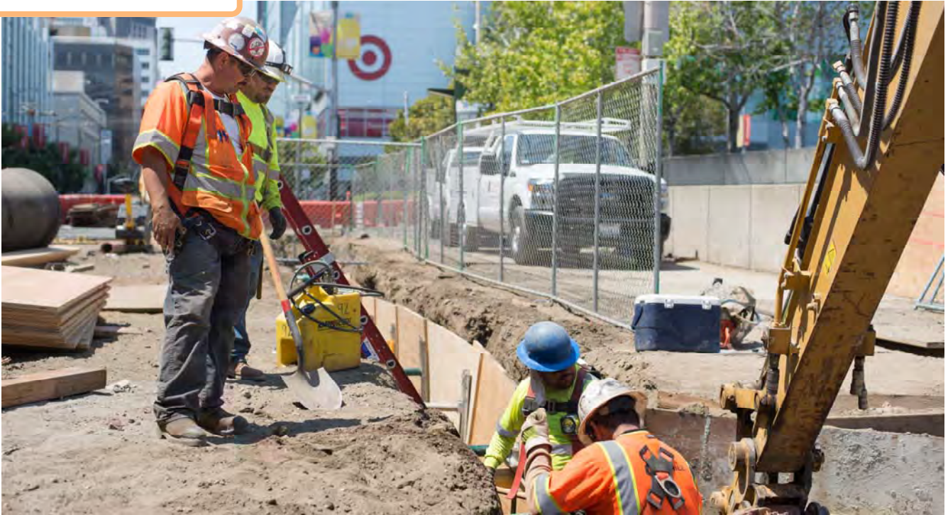
A utility trench spans the east side of 4th south of Howard, where utilities are being installed.
