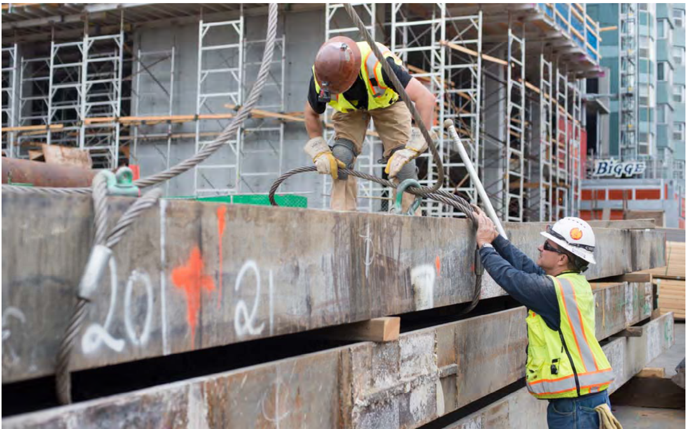
Two workers carefully thread steel cabling around a large beam prior to lifting it into the station headhouse site.
