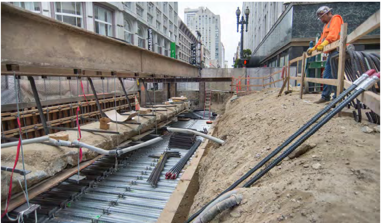
A worker looks down on corrugated steel panels being installed as part of construction of a new section of station roof decking, with a live utility duct bank spanning above, suspended from a steel truss system.
