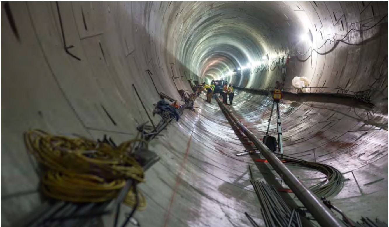
Looking south inside the northbound tunnel, north of the Union Square area, where the tunnel invert is being built.
