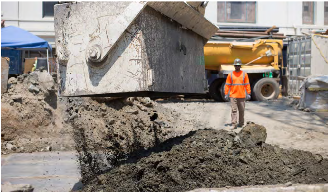
A crane operator unloads the large steel bucket used to remove excavated material from inside the station headhouse, as a dump truck waits in the background to be loaded.
