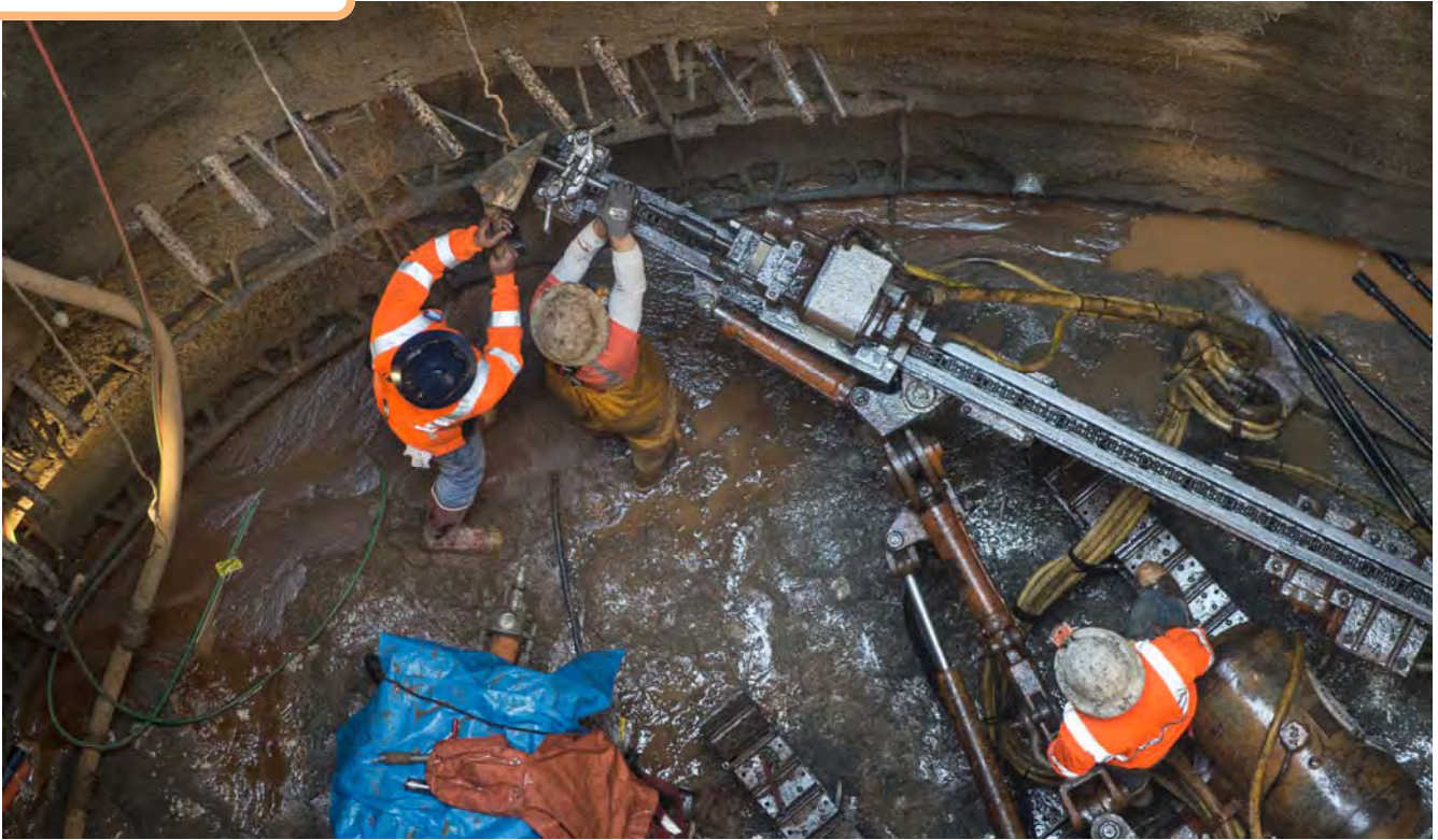
Workers drill through the shotcrete walls at the bottom of the north access shaft south of Jackson, to improve soil conditions ahead of excavating a lateral tunnel which will connect the shaft with the eventual station cavern nearby.
