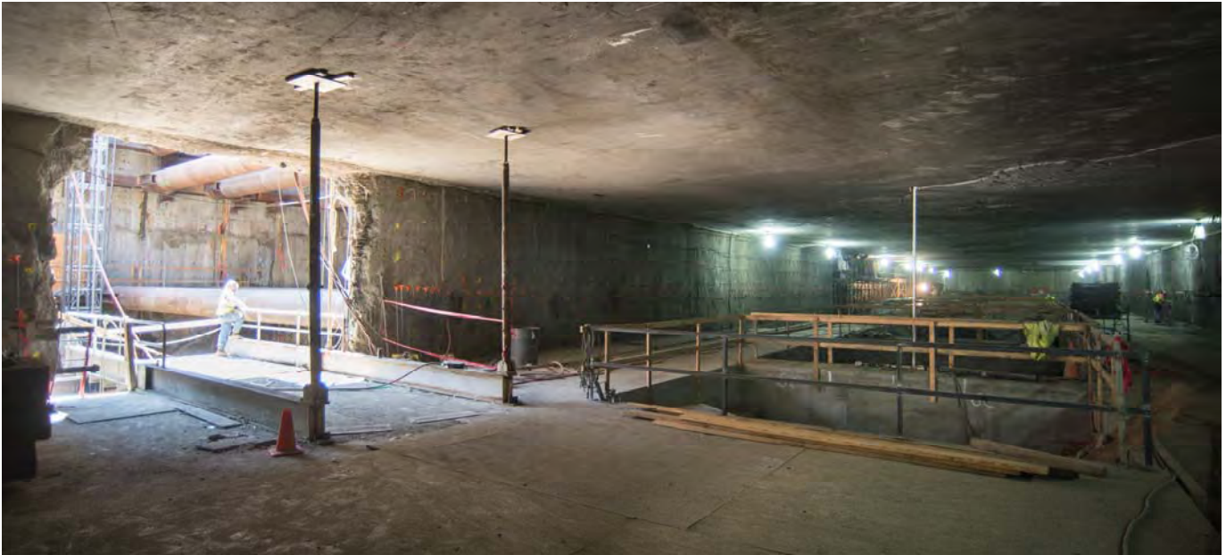
Light shines in the main access portal for the mezzanine level of the station box, where workers are preparing exposed sections of slurry wall for the installation of waterproofing.
