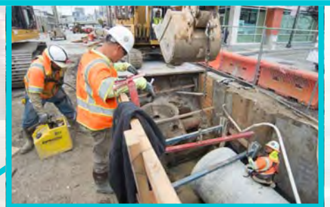
4th St. Surface Track, Systems (STS)
