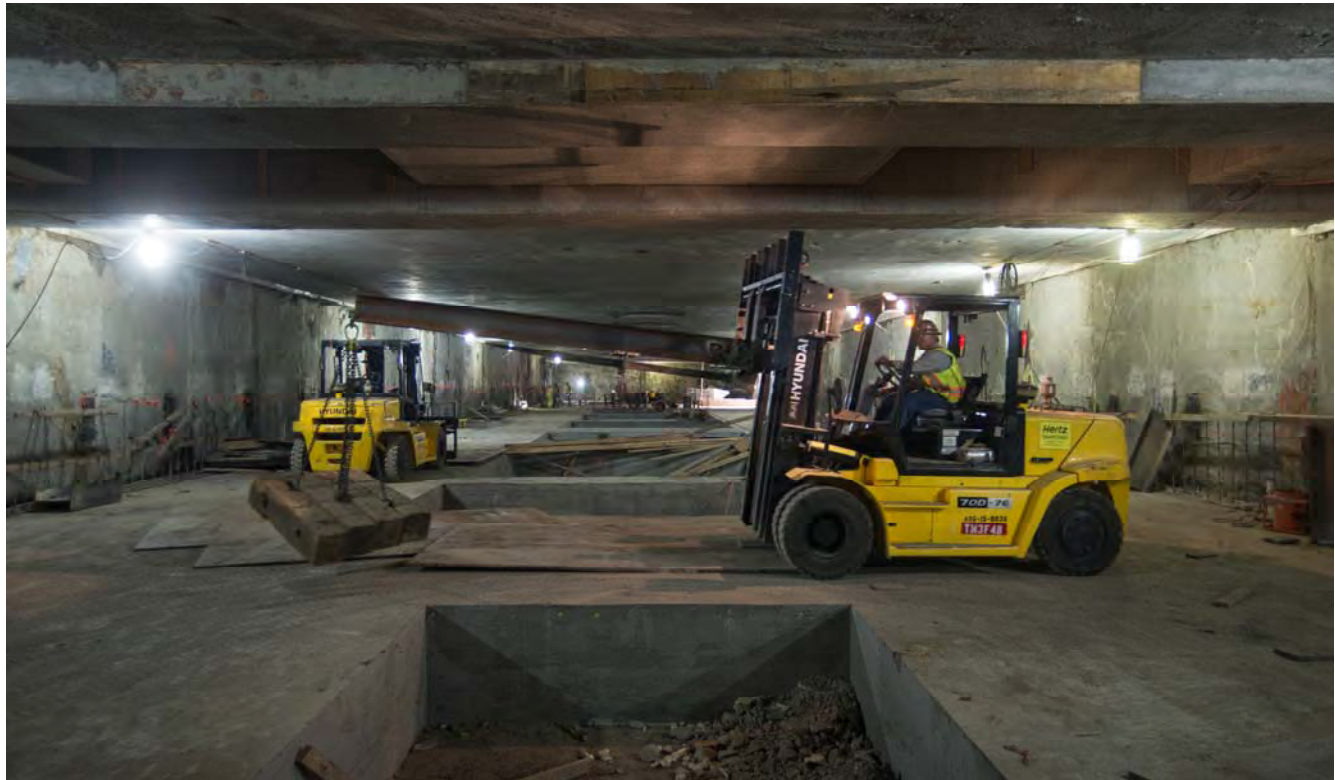
A large forklift moves cribbing materials at the north end of the station box, where work to clear out temporary reinforcing is almost finished.
