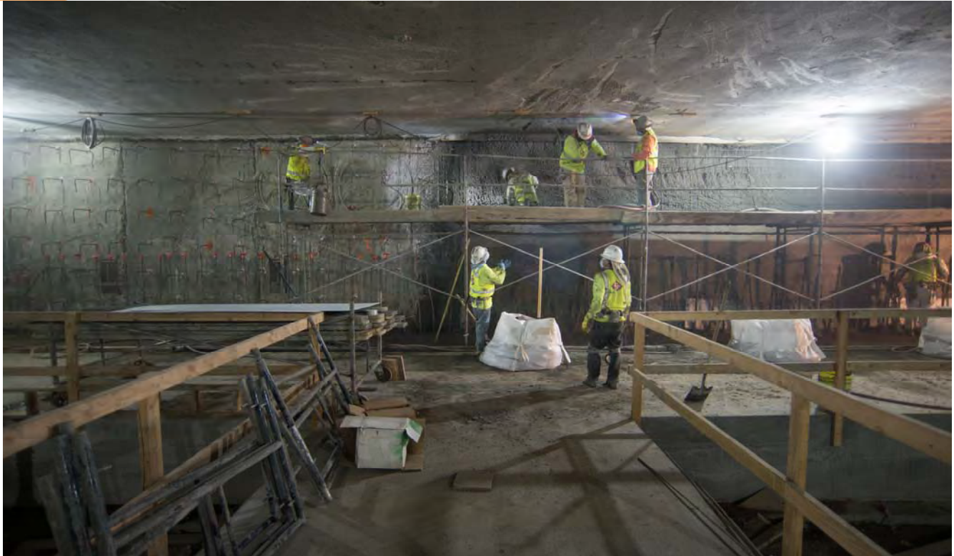
Workers prepare the outer walls of the station box for installation of rebar, shotcrete, and waterproofing, ahead of building a smooth "finish" wall.
