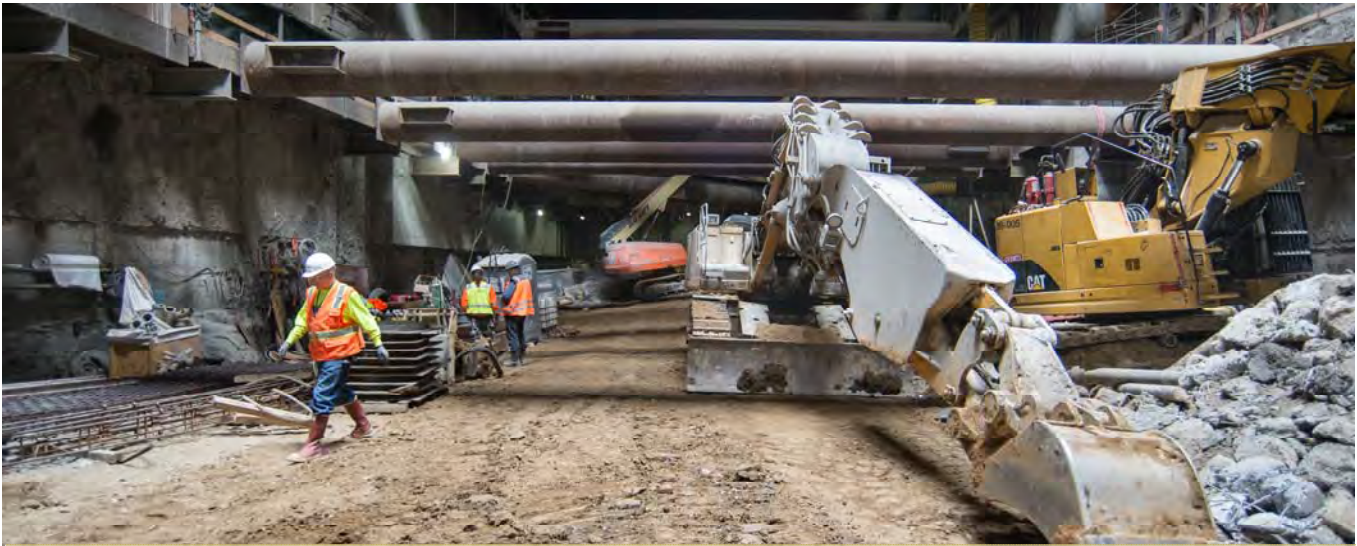
Large excavation equipment is staged at the bottom of the Chinatown Station headhouse during SEM work inside the station cavern archway.
