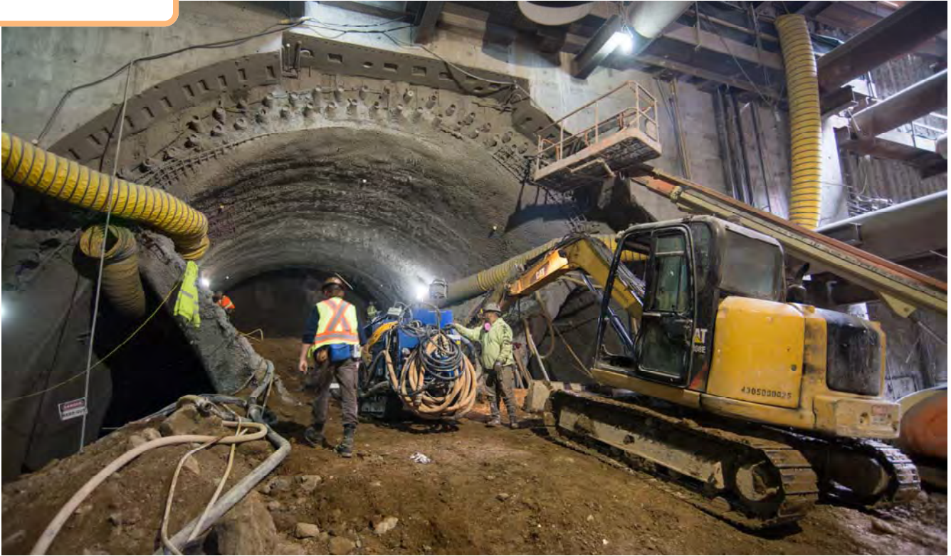
A shotcrete spraying machine is slowly brought out of the top heading of the SEM excavation work for the future station cavern entrance archway.
