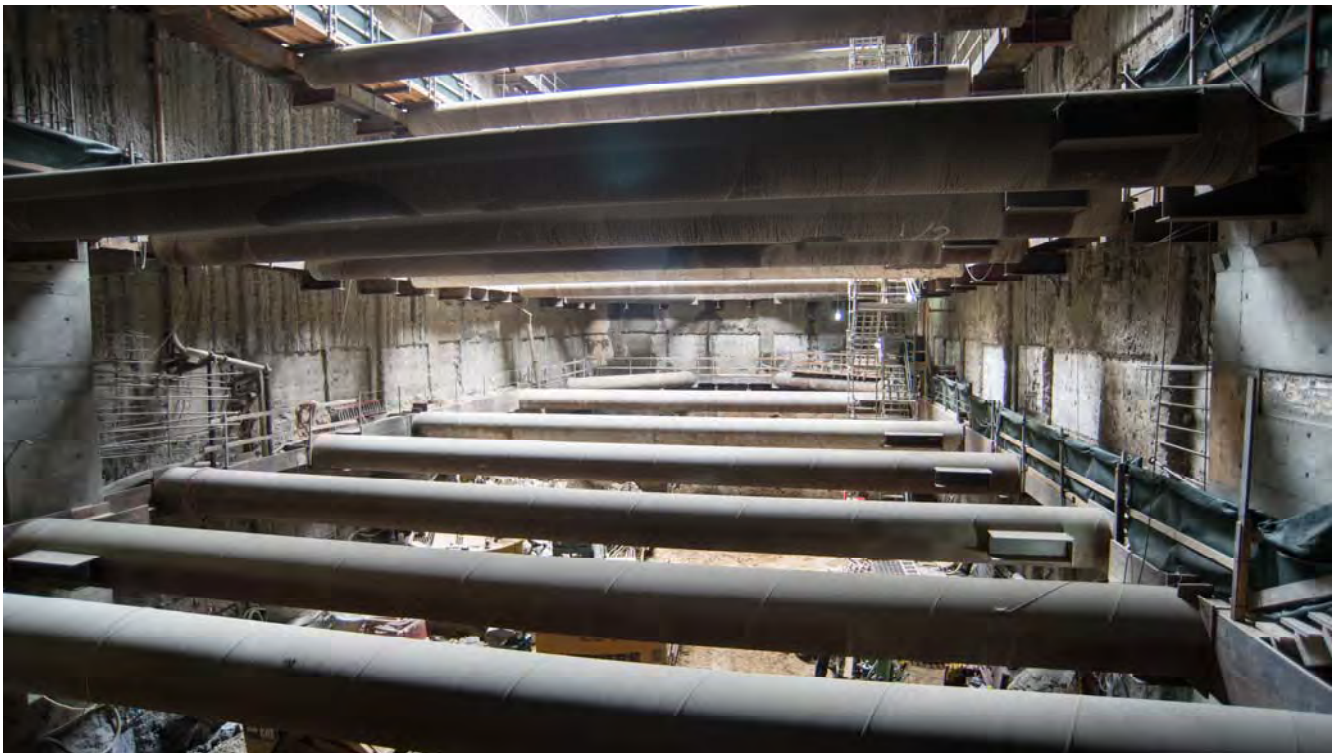
Long steel tubes called struts span across the headhouse at intervals, supporting the exterior walls against the pressure of soil.
