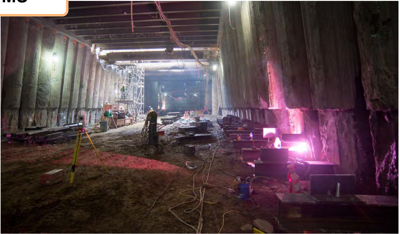
Looking north halfway between Geary and o'Farrell, a welder attaches steel brackets to the outer walls of the station.
