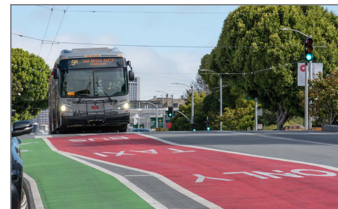
Red bus lane on Potrero Avenue: New red transit lanes and an upgraded bike lane were installed as part of the Potrero Avenue Streetscape Improvement Project.
