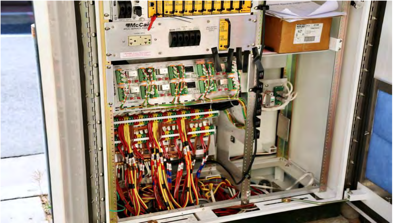
View of electrical cabinet wiring for traffic signals
