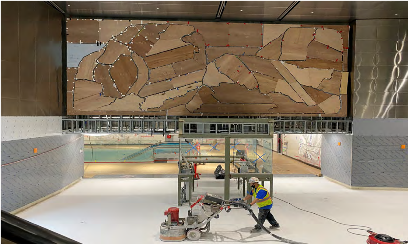
A worker operating a concrete floor grinder to smooth rough surfaces of the floor for Yerba Buena/Moscone Station concourse.
