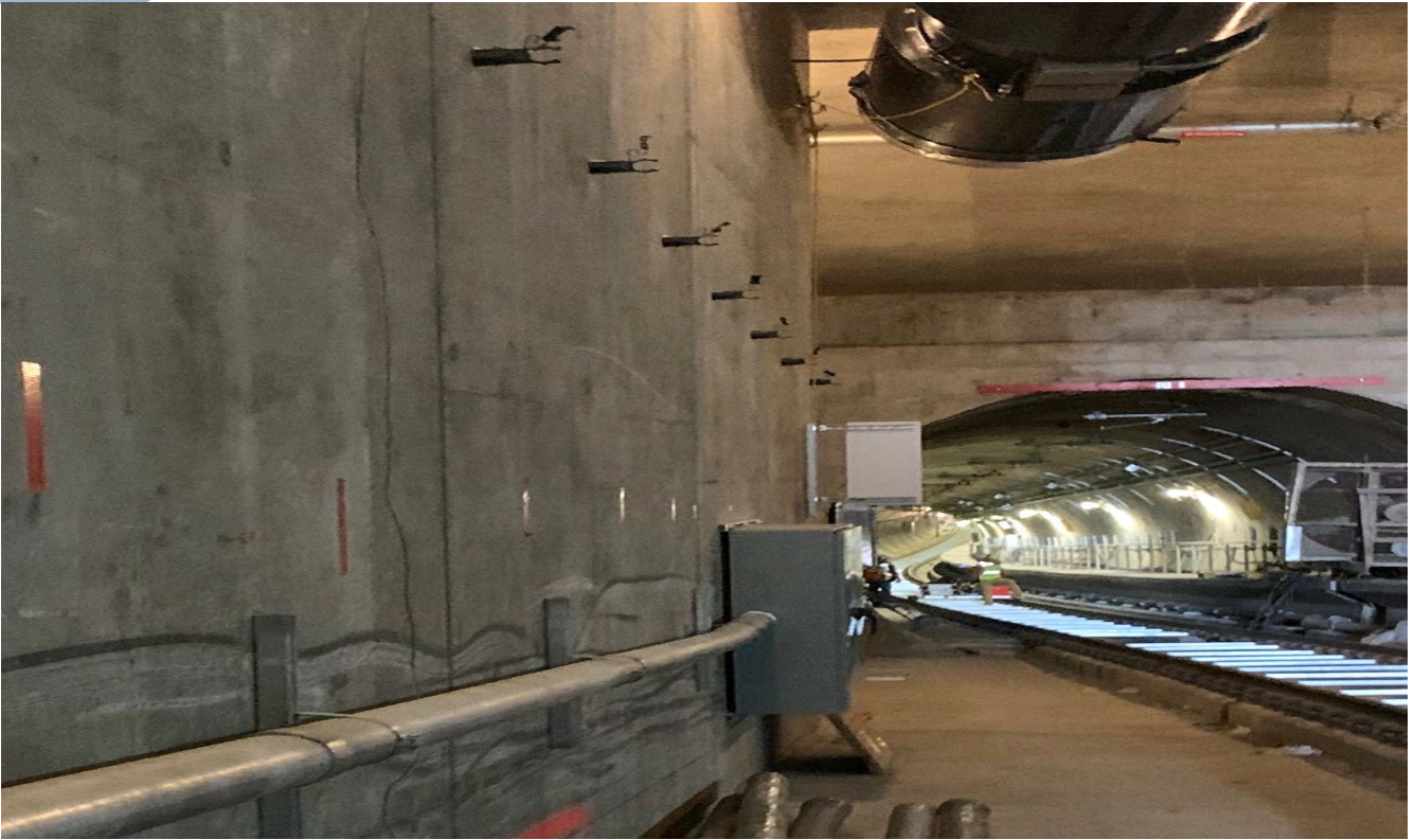
Emergency ventilation jet fans, automatic train control system, OCS, traction power, radio system supports and tunnel signage continue to be installed at tunnel systems portal.
