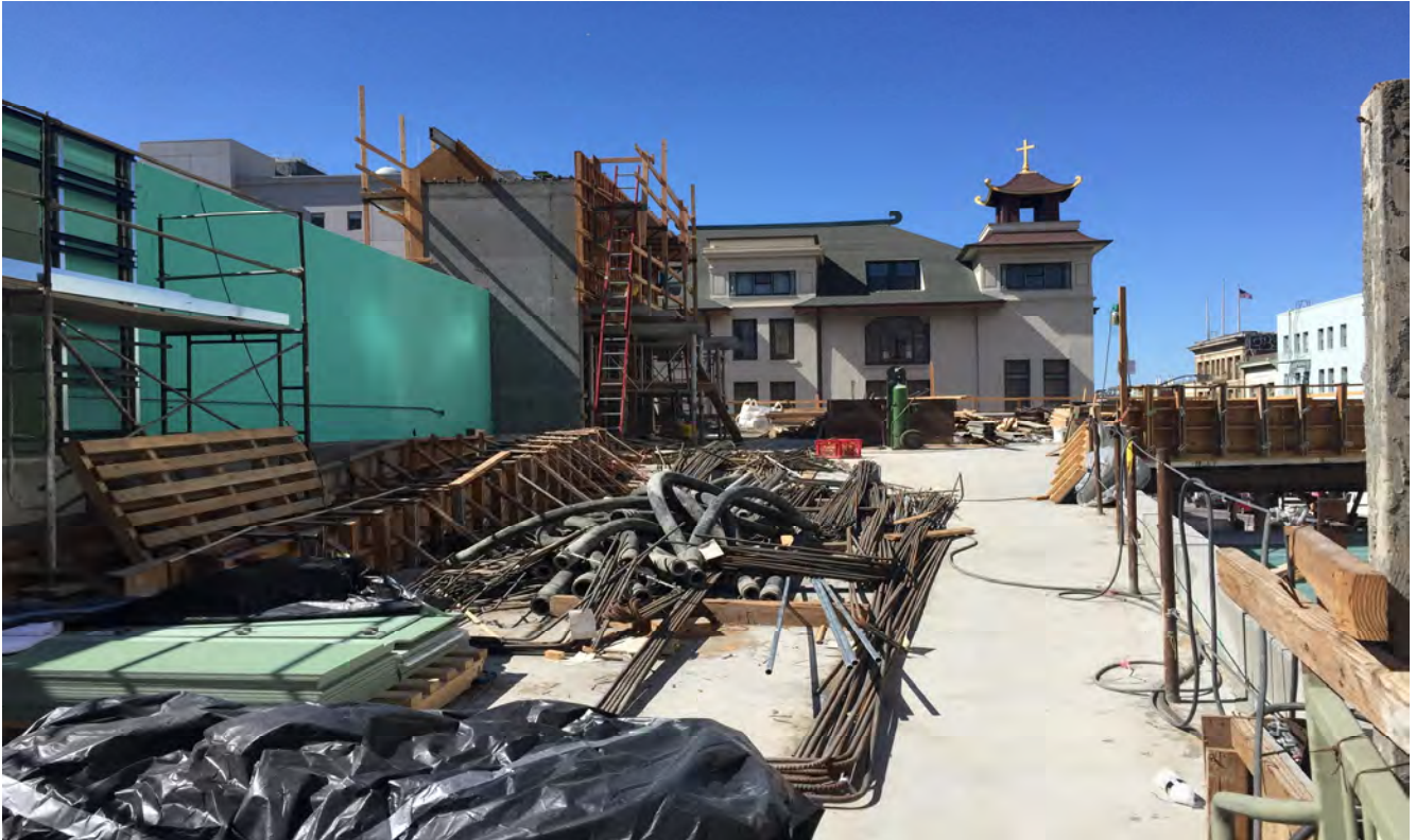
Structural beams and corrugated steel panels which will hold the future Rose Pak-Chinatown Station rooftop plaza are being placed and installed.
