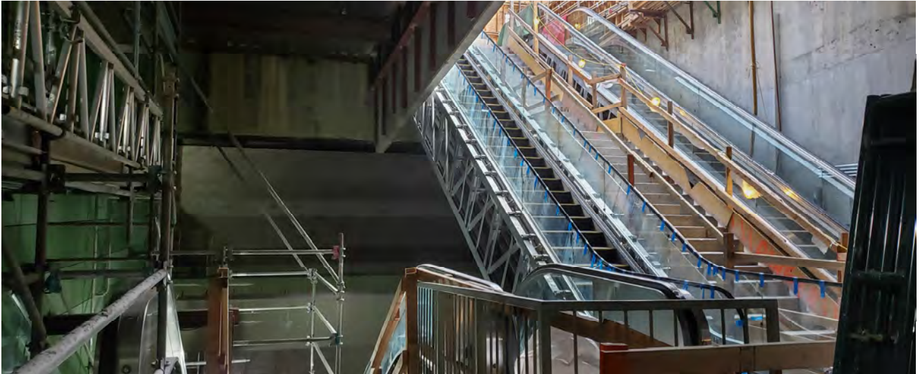
Glass railings, jade-colored wall panels, and other finishing interior elements are being installed inside the upper mezzanine level for Rose Pak-Chinatown Station.
