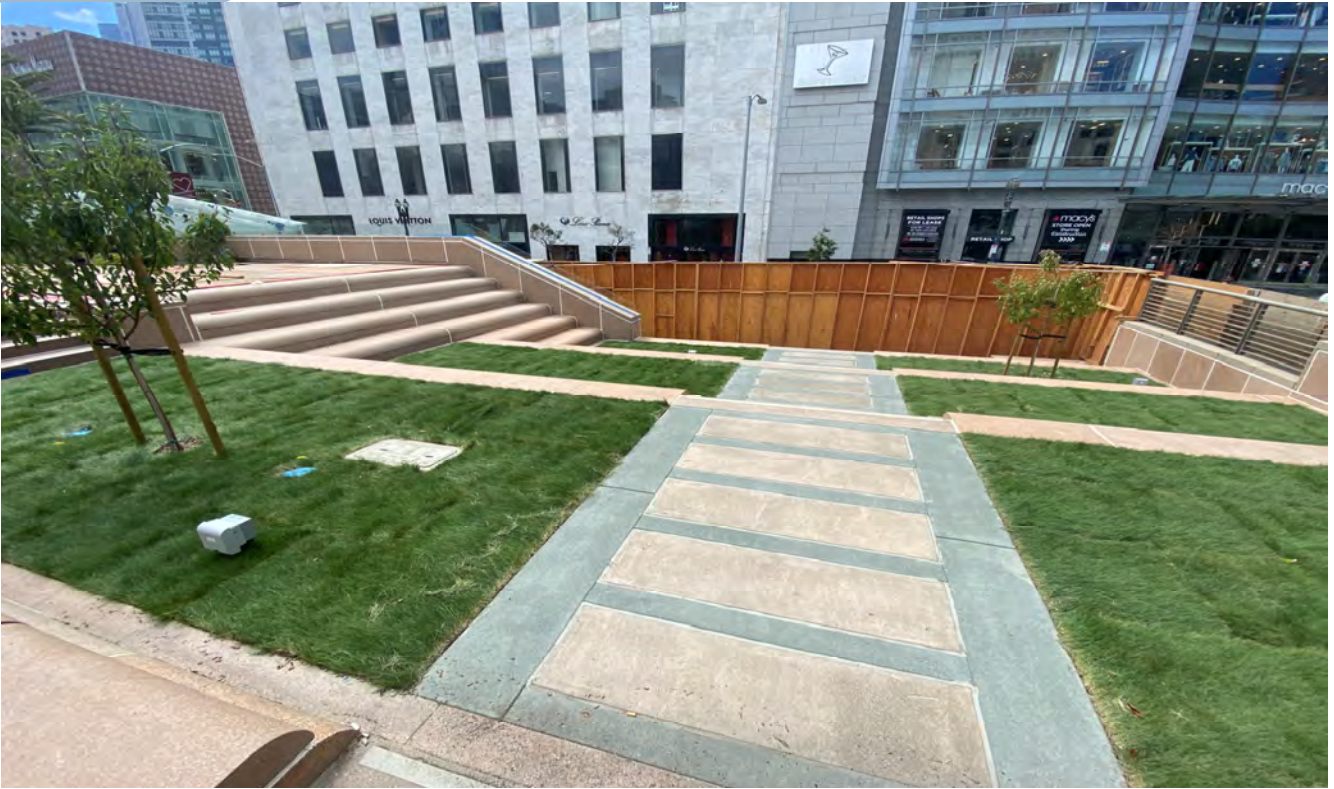
Precast stairs and planters have been installed and landscaping work is being performed at Union Square/Market Street Station terrace
