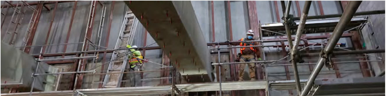
Steel framing has been furred out from the east wall of the concourse lobby for the installation of utilities behind and wall panels against it.
