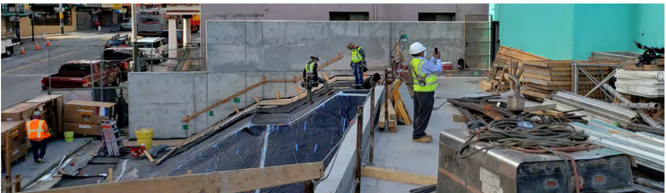
A crew lays out rolls of waterproofing membrane where future stairs will be built leading to the rooftop plaza at Rose Pak-Chinatown Station.
