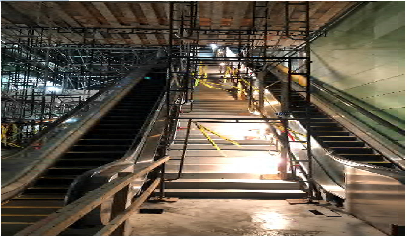
Architectural glass panels are being installed along adjacent to escalators at Ticketing Hall of Rose Pak-Chinatown Station.
